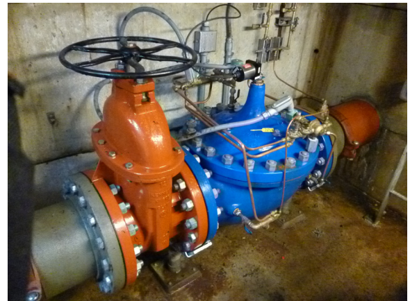
Figure 10.1 - Gate Valve at Bel-Red Inlet Facility
