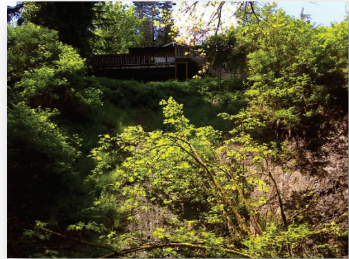
Figure 6. Close Proximity of Residential Property to the Scarp of LS-09
