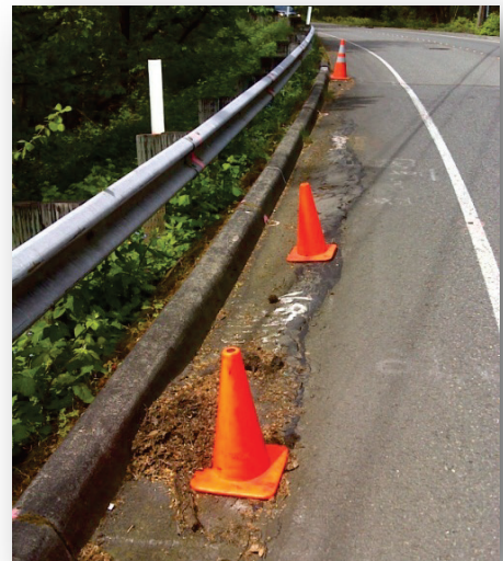
Figure 3. Cracked Road Fill Slope along SE 35th Place (PP-11)
