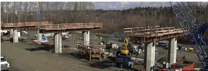
Columns to support the guideway are being built adjacent to the east side of Bellevue Way SE
