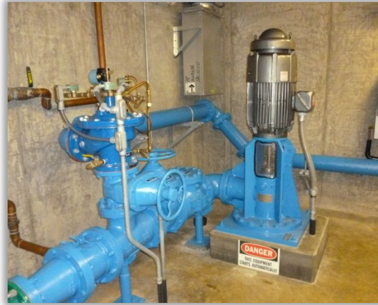
Meydenbauer Pump Station
