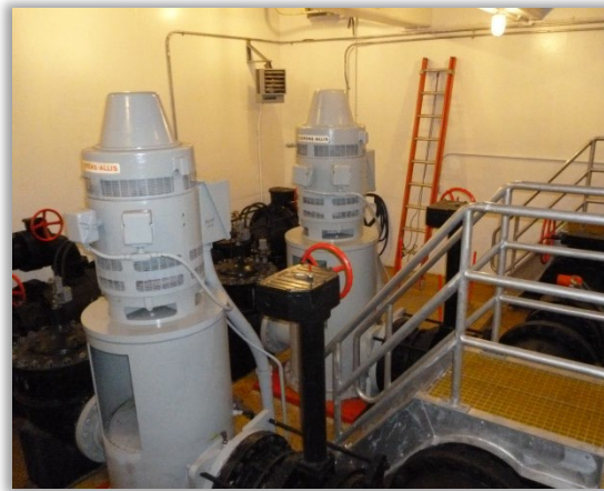
NE 8th Inlet Pump Station
