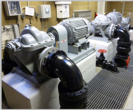
Woodridge Pump Station
