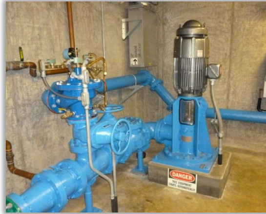
Meydenbauer Pump Station
