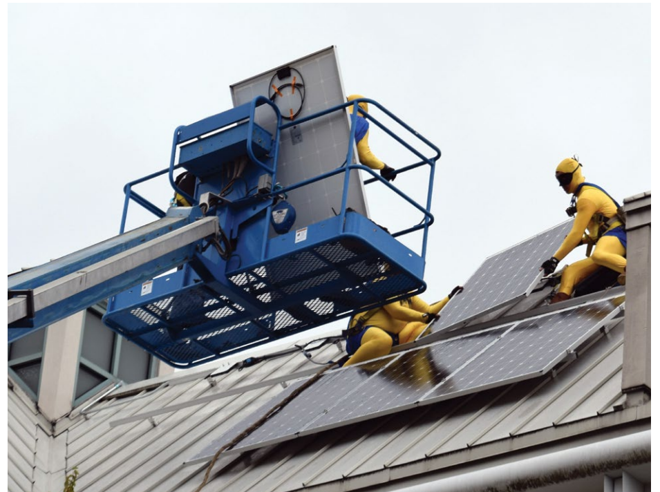
A fun example of outside the box climate action was the grant funded installation of solar panels on the roof of KidsQuest Children's Museum in 2015, with installers dressed as superheroes.
