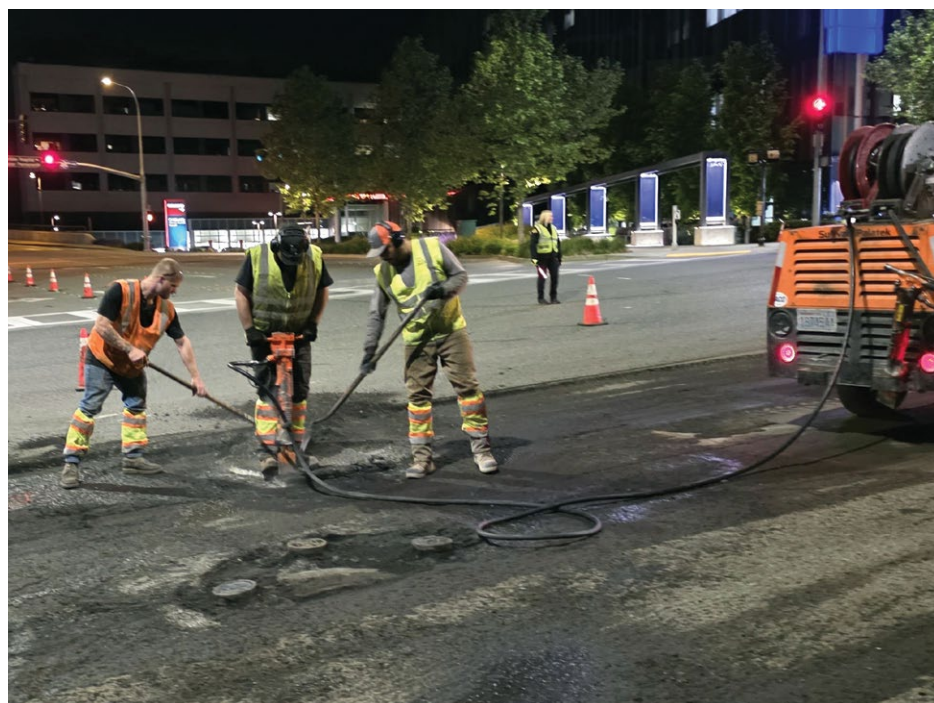
A paving crew uses a jackhammer to remove some existing asphalt in preparation for new pavement along 116th Avenue Northeast.
