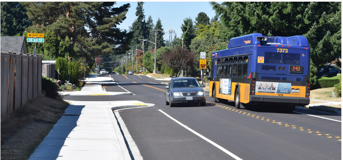
Figure 5: New sidewalks, curb bulb-outs and radar feedback signs installed between Southeast 60th Street and Southeast 65th Place in 2025.
