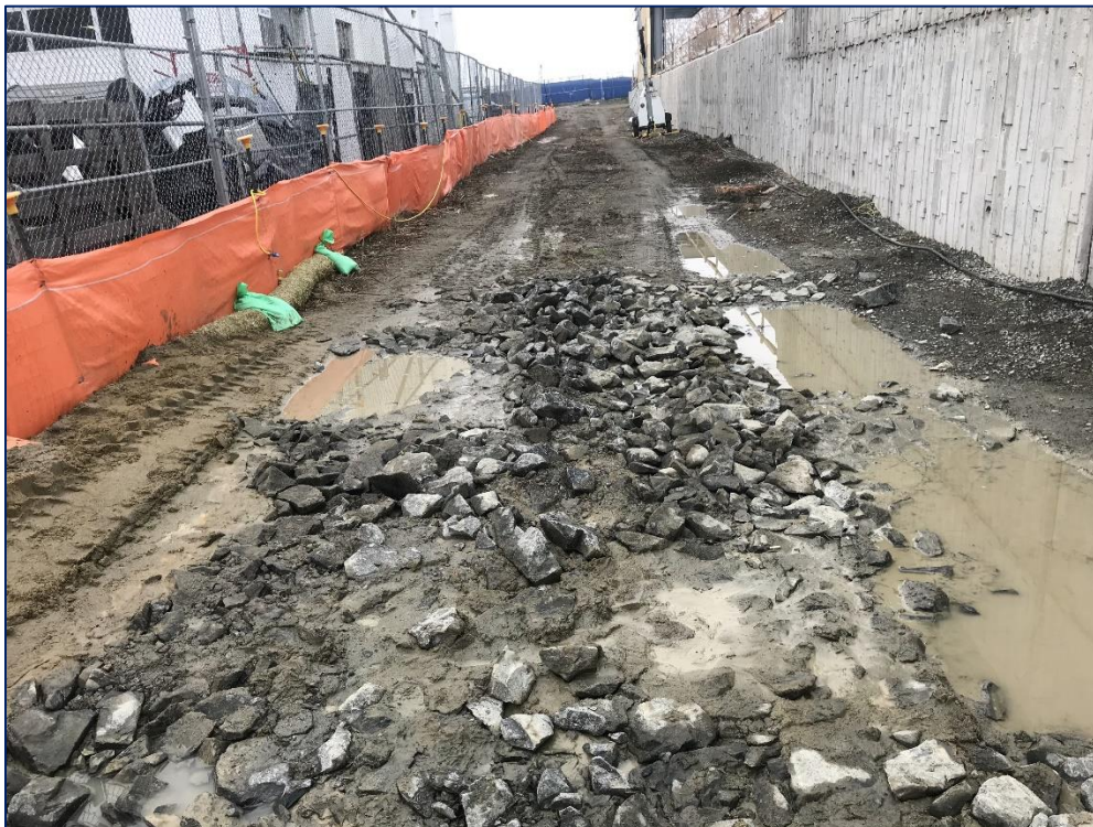
Photo 4. Temporary easement being utilized by Sound Transit along the northern edge of property.
