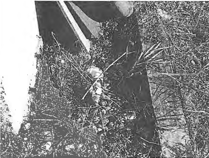
PHOTO #7: OUTLET VALVE FOR ADMIXTURE SECONDARY CONTAINMENT IS LOCATED OVER THE BARE GROUND; NO LOCK.
