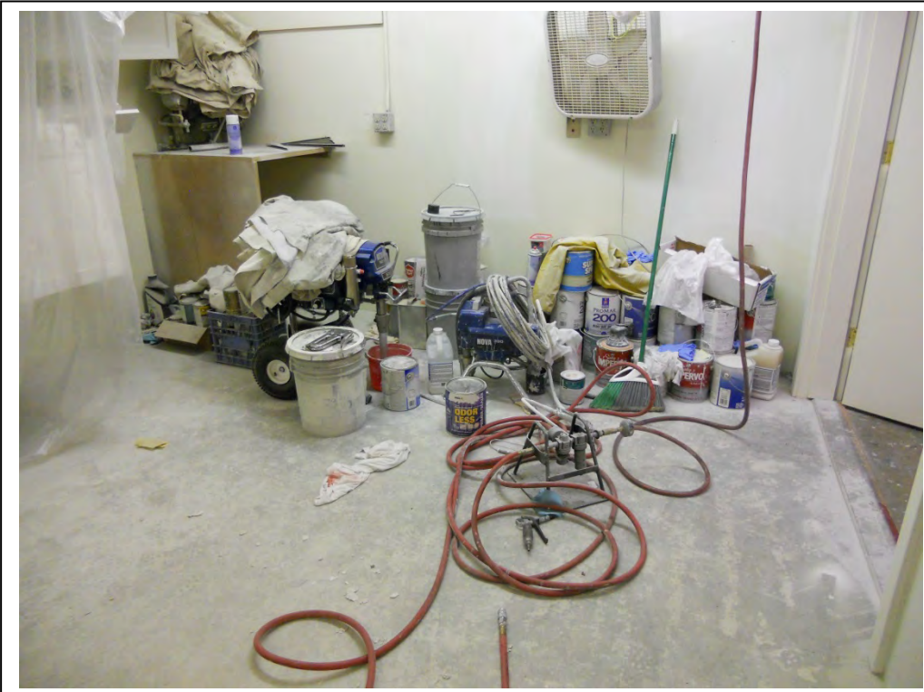
Photo 14: Improperly stored chemicals in the north end of the paint booth.
