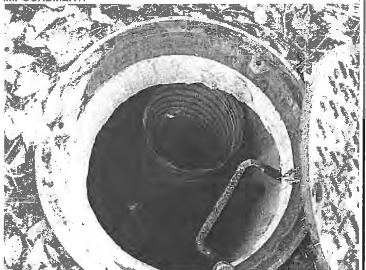
PHOTO #16: THIS MANHOLE IS LOCATED IN THE SOUTHWEST CORNER OF THE PROPERTY.
