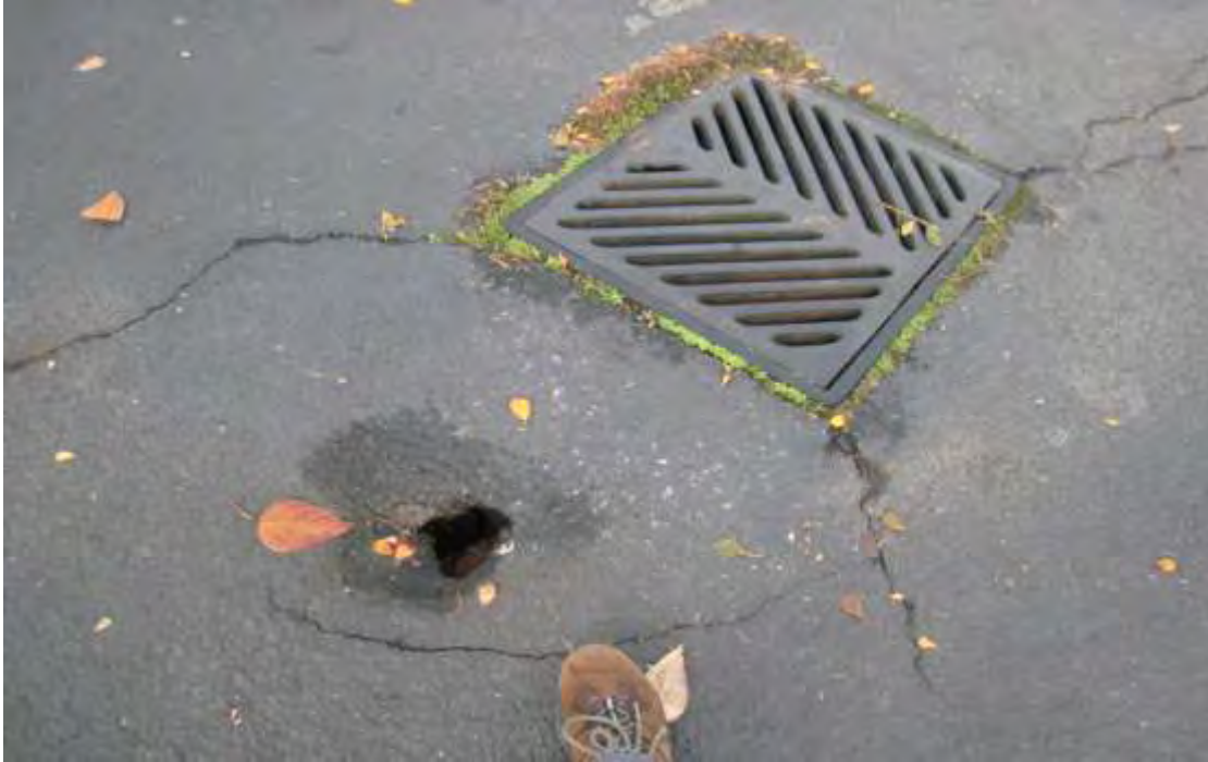
Photo 3: Potential problems with pavement not near contamination - front parking lot
