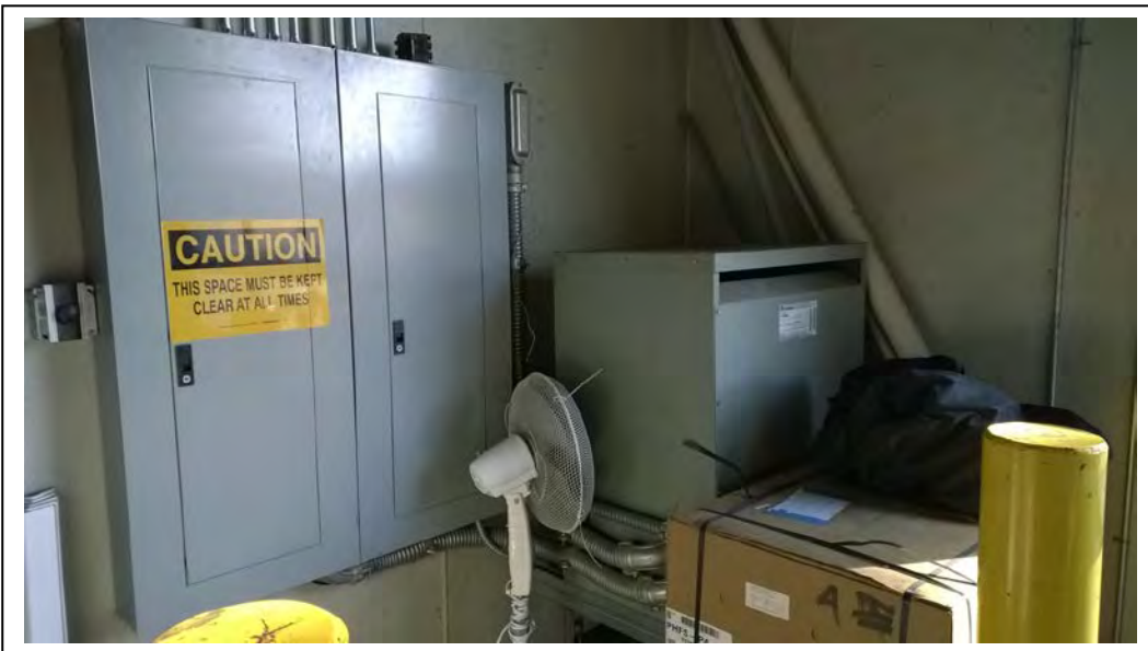
Photo 4: Electric panel and transformer in warehouse are of subject building.
