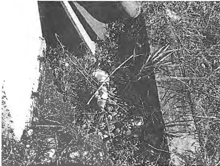
PHOTO #7: , OUTLET VALVE FOR ADMIXTURE SECONDARY CONTAINMENT IS LOCATED OVER THE BARE GROUND; NO LOCK.
