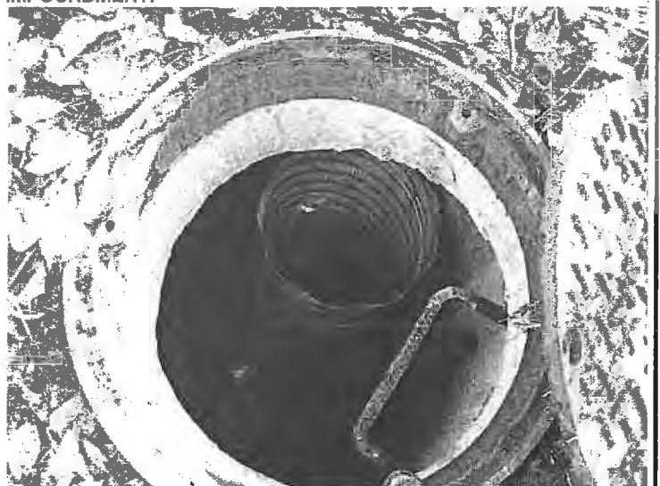
PHOTO #16: THIS MANHOLE IS LOCATED IN THE SOUTHWEST CORNER OF THE PROPERTY.
