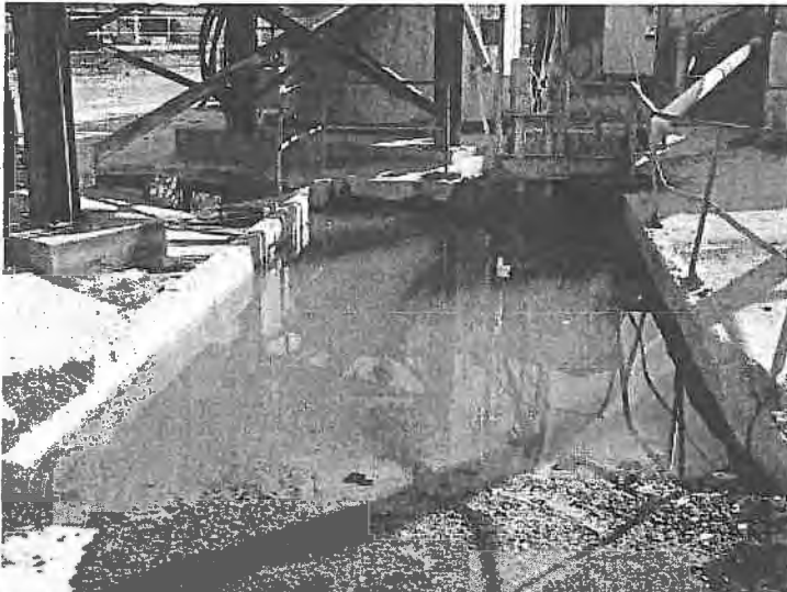
PHOTO #3: CONCRETE-LINED IMPOUNDMENT HOLDS PROCESS WATER WHICH IS CONVEYED TO CO 2 SPARGING TREATMENT SYSTEM.
