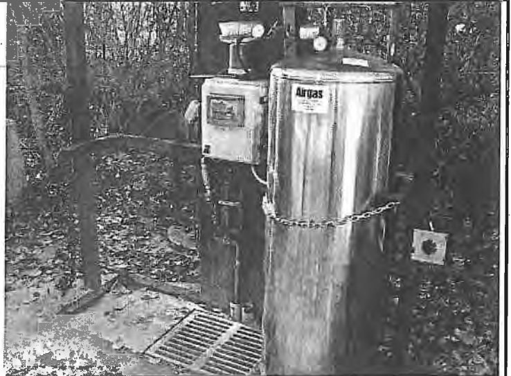
PHOTO #12: CO 2 SPARGING SYSTEM.
