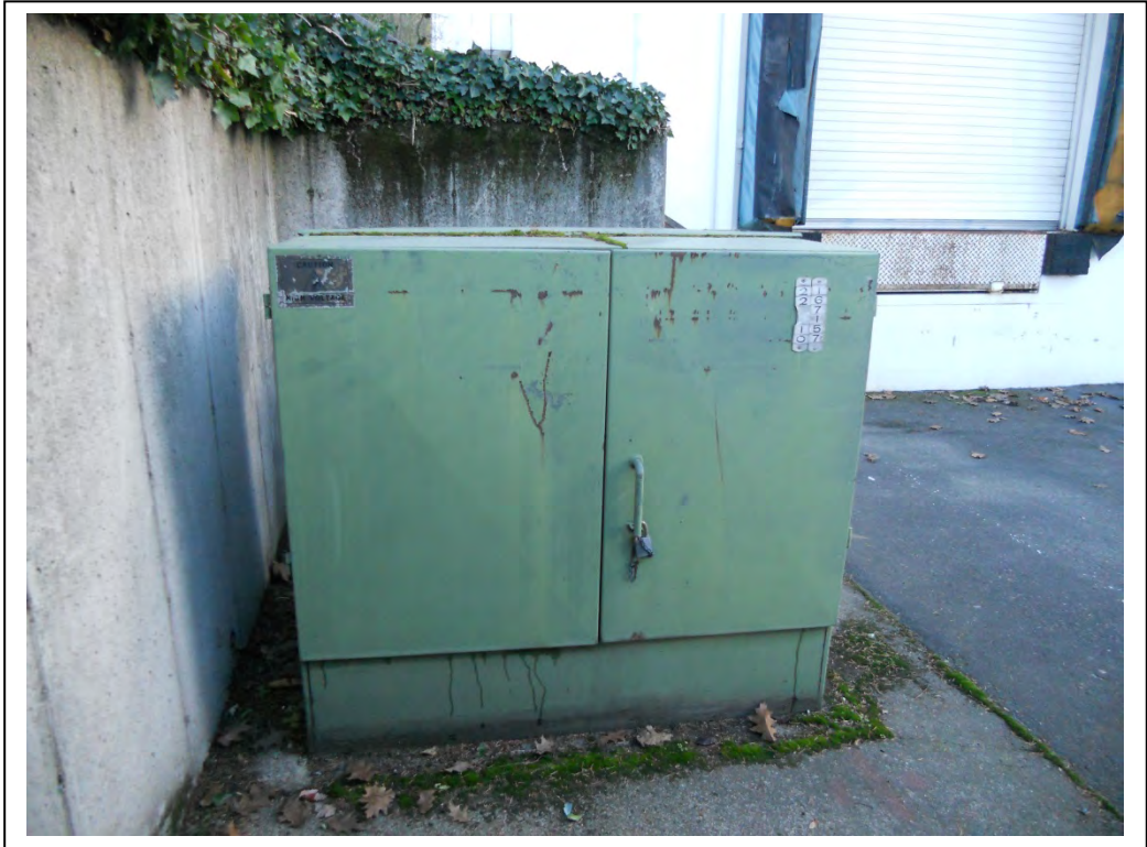
Photo 5: Transformer noted in northwest exterior area.
