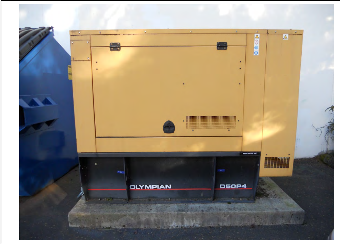
Photo 9: Backup generator noted on southeast exterior of subject building.
