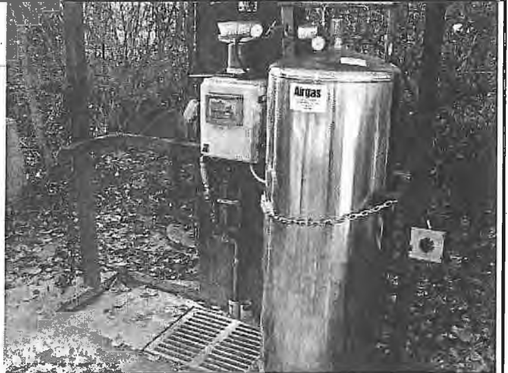
PHOTO #12: CO 2 SPARGING SYSTEM.
