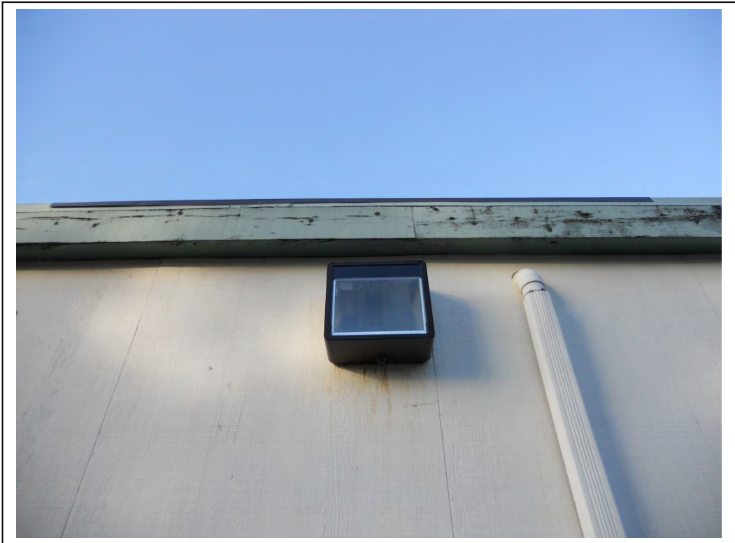
Photo 7: High intensity discharge lighting noted on building exterior.
