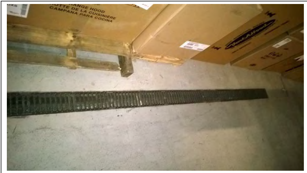
Photo 3: strip drain in warehouse part of subject building.
