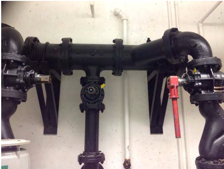
Common discharge piping
