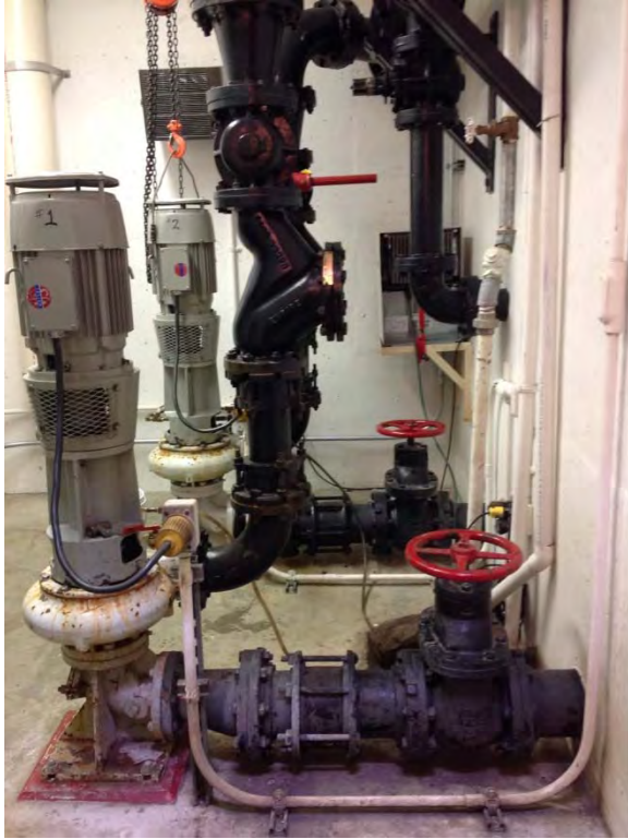
Duplex configuration, Pump 1 in foreground
