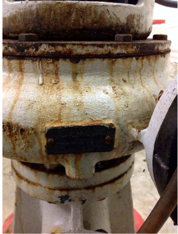
Pump #2 showing signs of aging on exterior
