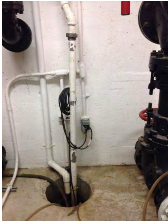
Sump pump in dry pit
