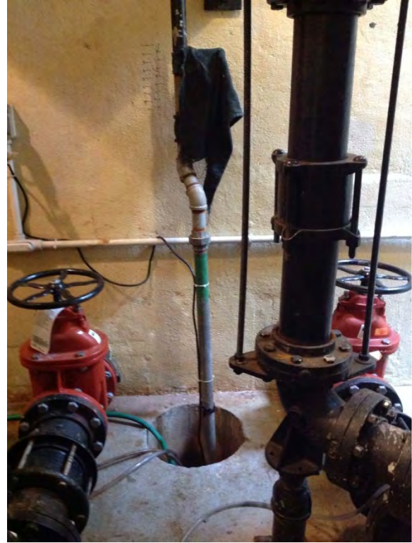
Sump pump in dry pit
