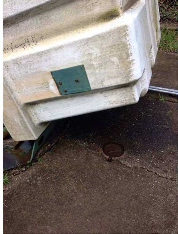
Isolation valve adjacent to site, unknown if operable
