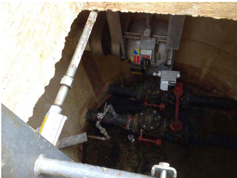
Interior of wet well blower and check valve/isolation valve vault
