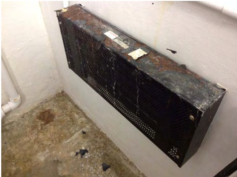
Heater in dry pit is significantly corroded
