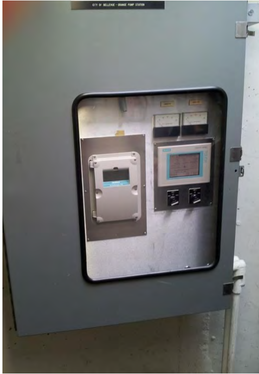
Telemetry control panel located in dry pit with operator interface
