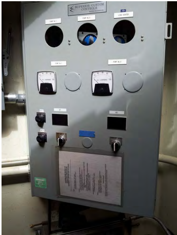
Starters located in dry pit, appears to be in good condition
