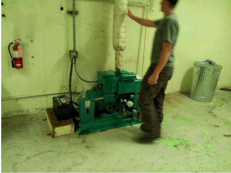
Standby generator located on top floor of control building
