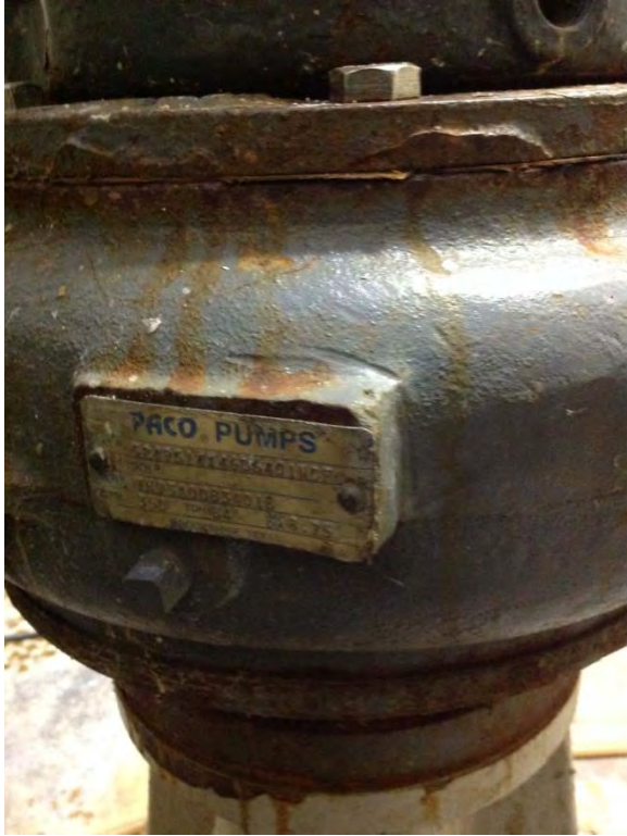
Pump 2 showing signs of aging on exterior
