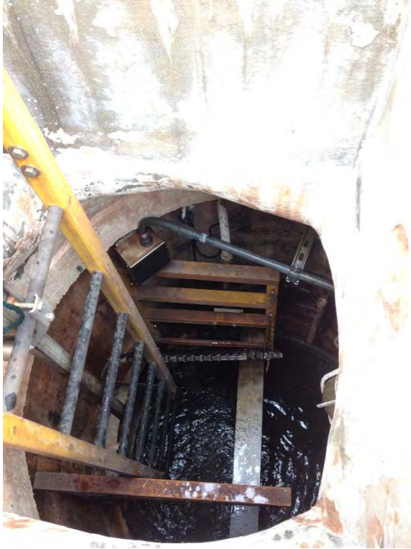
Interior of wetwell, some pitting in lower sections – still coated but should be inspected
