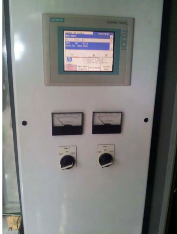
Starters located in outdoor power enclosure, appears to be in good condition
