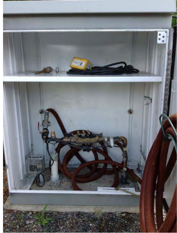
Backflow prevention assembly with heat tape and hose bibb for wash down located in enclosure
