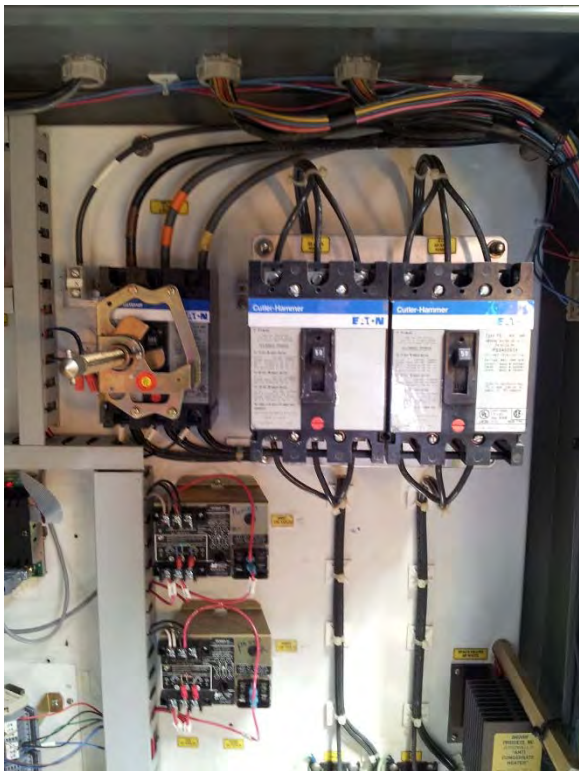
Original starters and circuit breakers are Eaton Cutler Hammer, appear to be in good shape but aging
