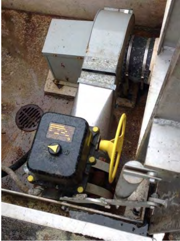
Interior of wet well blower vault appears to be in good condition
