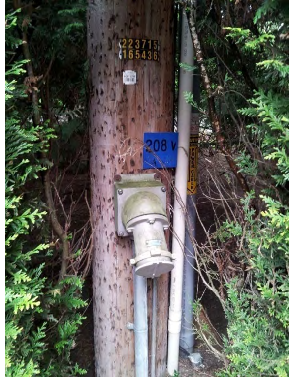
Generator receptacle located on Qwest pole near roadway, appears to be in good condition
