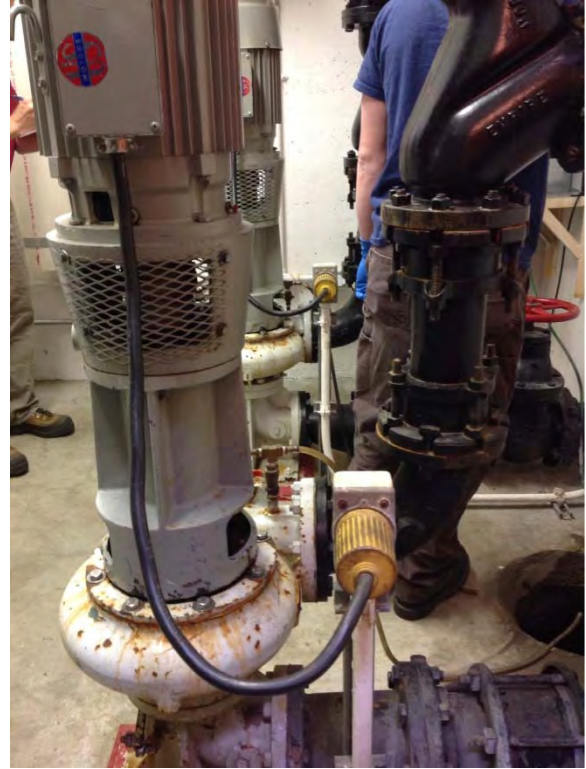
Pump and motor #1
