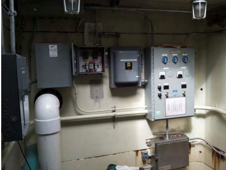
Square D Panelboard located in dry pit on left side
