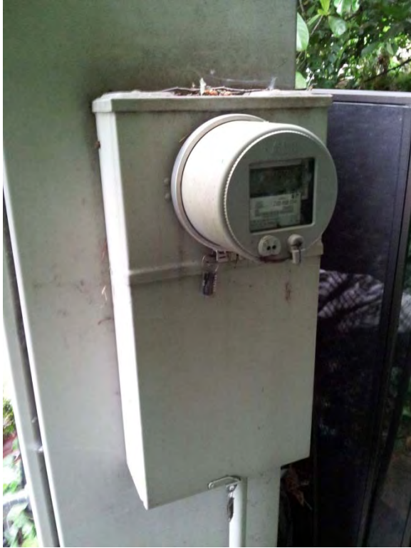
Utility service meter on outside of service equipment cabinet
