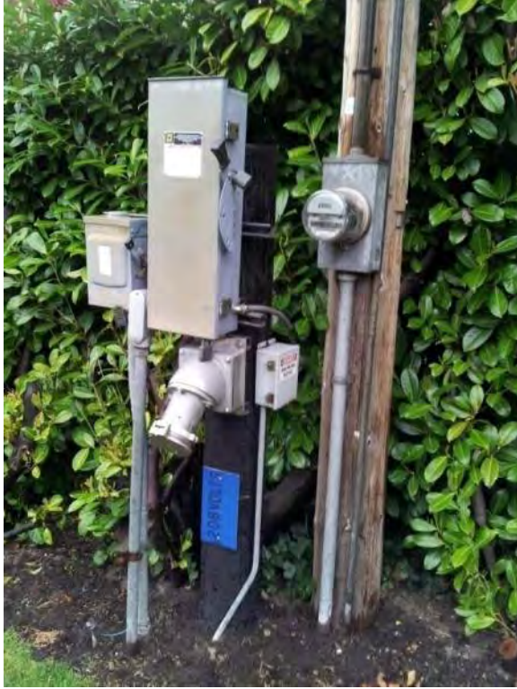
Utility service and generator receptacle
