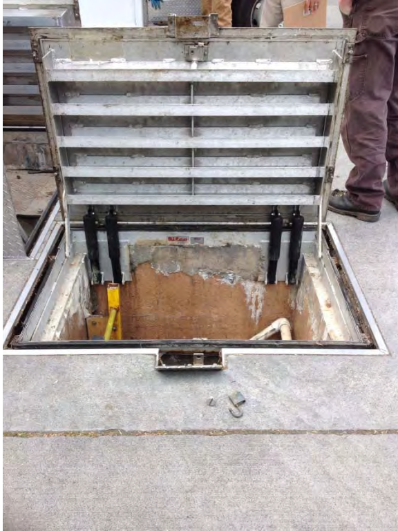
Wet well lift assist hatch, fatiguing evident
