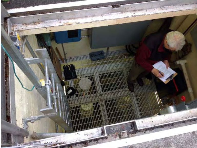
Telemetry and control panel located on upper level of dry pit
