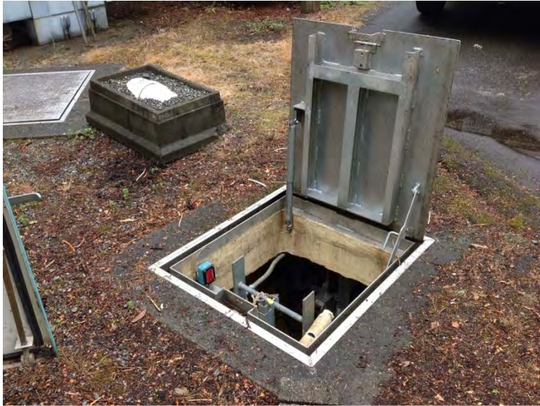
Wet well blower and check valve/isolation valve vault location
