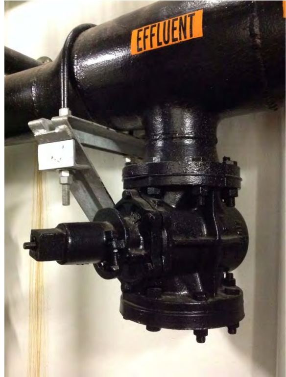
Common discharge piping
