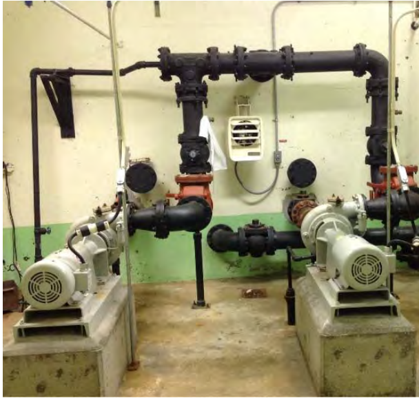
Duplex configuration pump #1 on left
