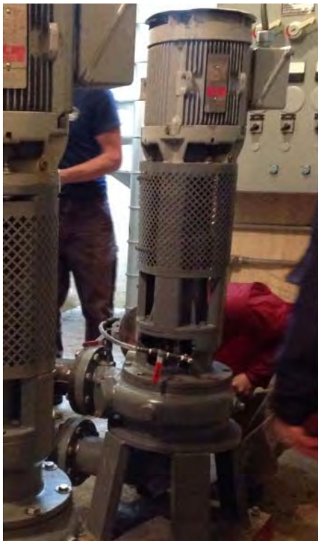
Pump and motor #1
