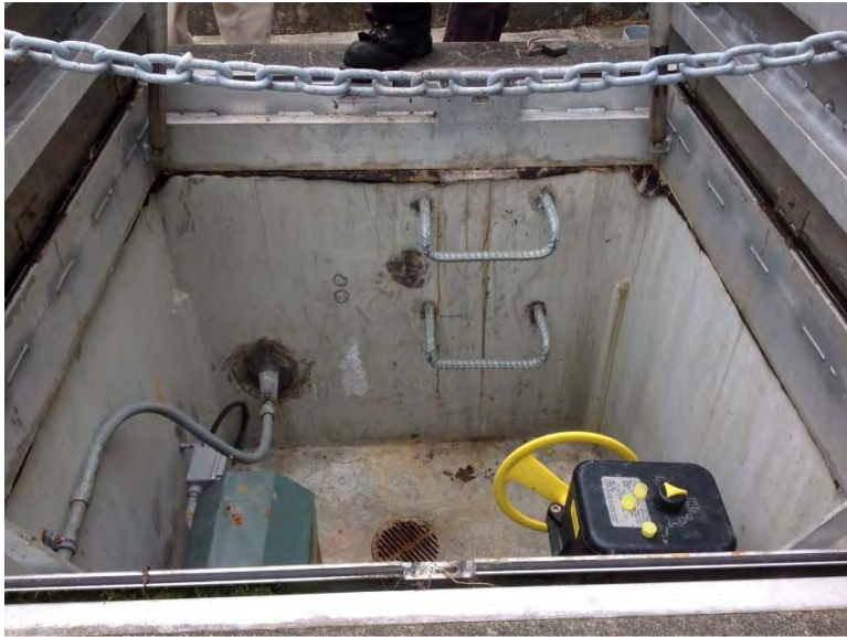
Wet well blower vault hatch, chain fall protection on one side
