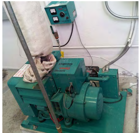
Standby generator located in dry pit
