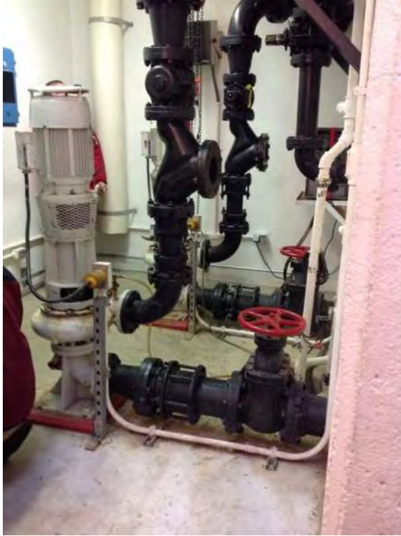
Duplex configuration (Pump 1 in foreground)
