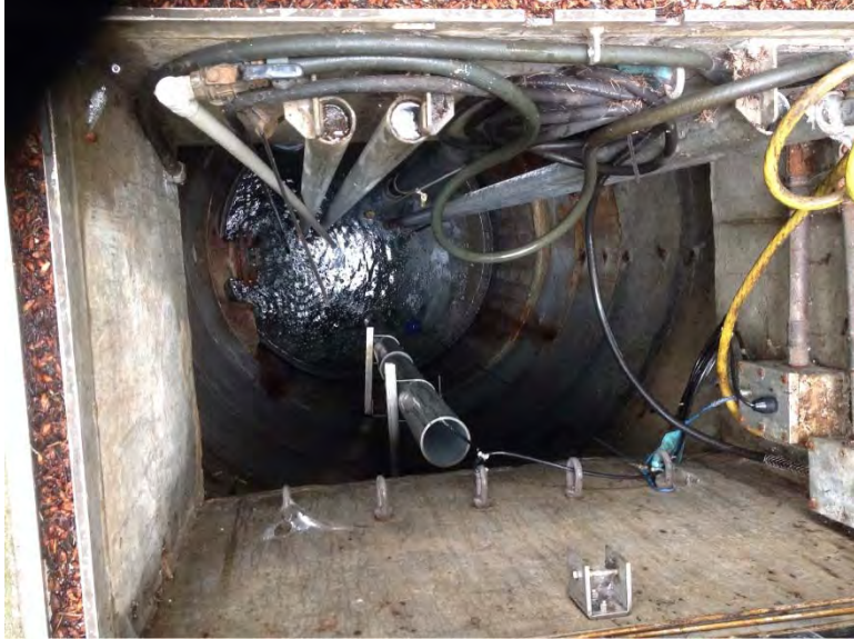
Interior of wet well, no access ladder
