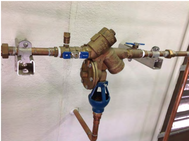
Backflow assembly located in building top floor, drains to daylight
