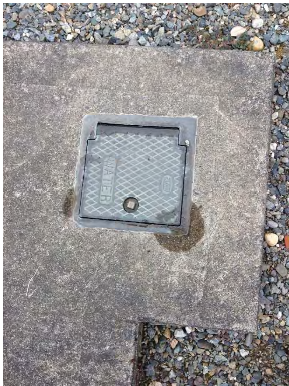
Wash down water supply adjacent to wet well
