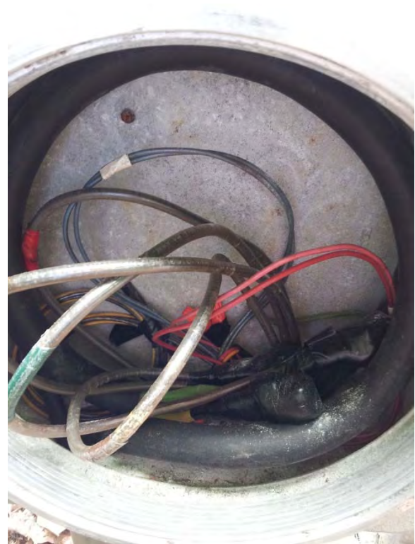
Terminal block spilled in – no terminals
