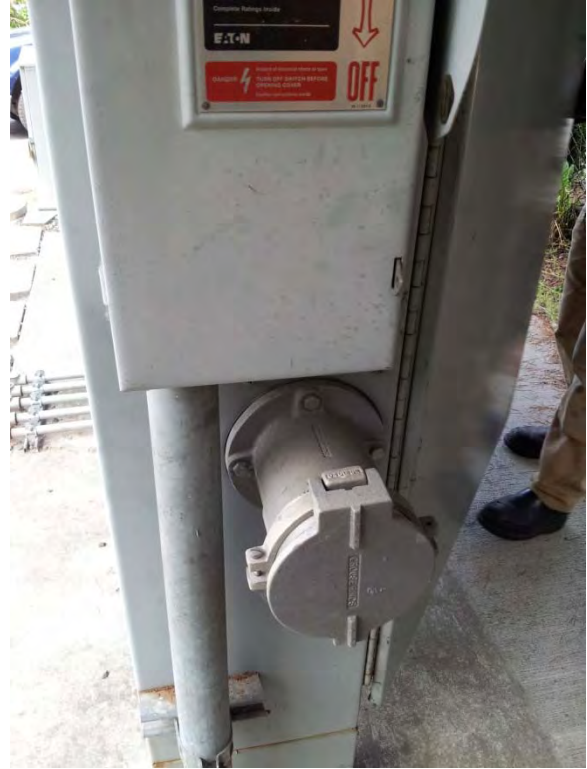
Generator receptacle mounted thru outside of power and control panel
