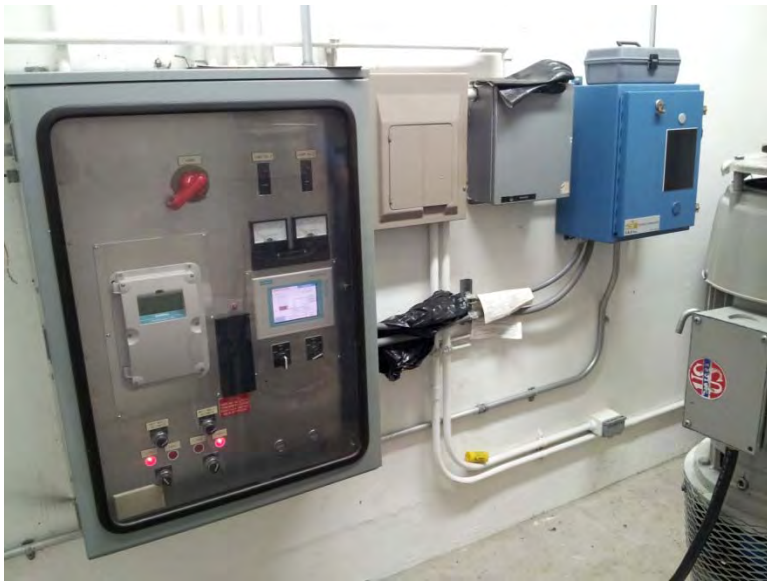
Panelboard and starters located in dry pit
