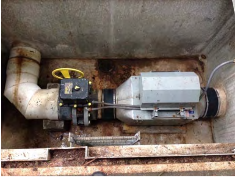
Wet well supply fan in adjacent wet well blower vault
