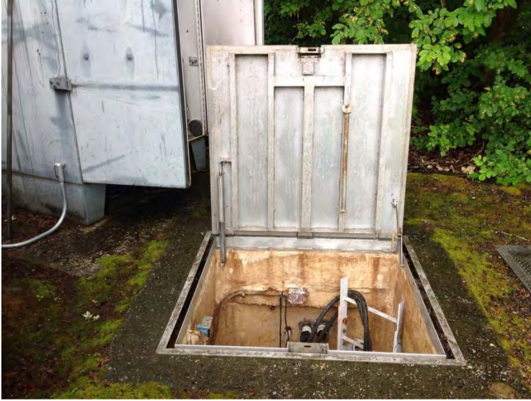
Wet well access hatch and ladder
