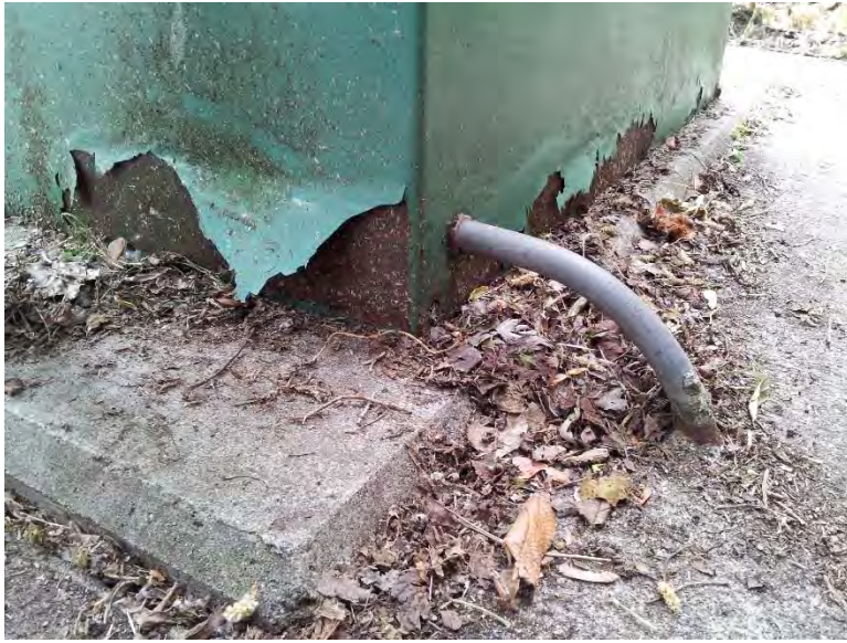
Service cabinet paint is chipping near bottom, conduit corroding near grade
