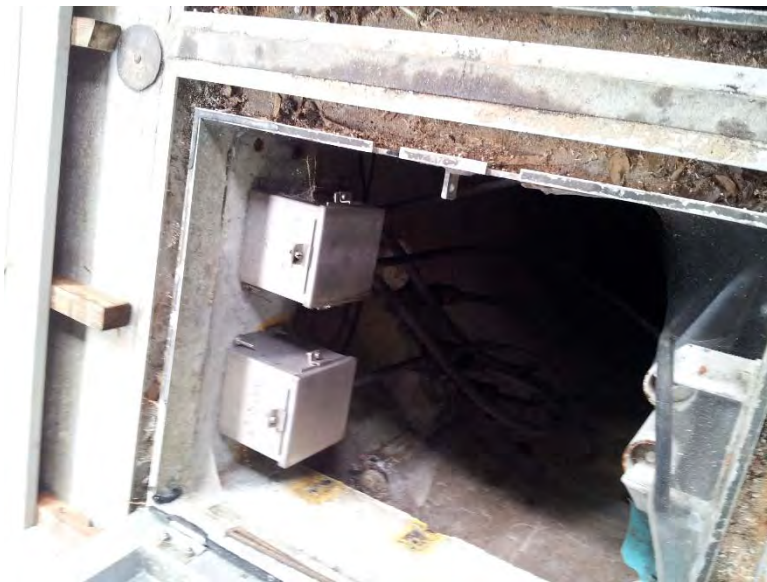
Junction boxes located in mouth of wet well, difficult to access
