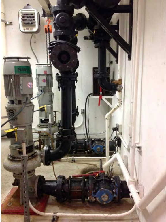
Duplex configuration, Pump 2 in background
