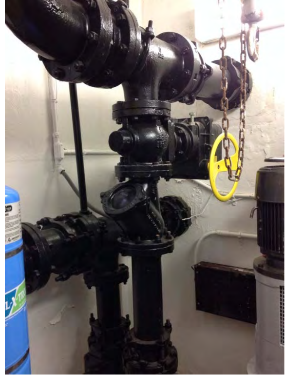
Automated discharge plug valve to prevent siphoning, ball check valve located below discharge plug valve
