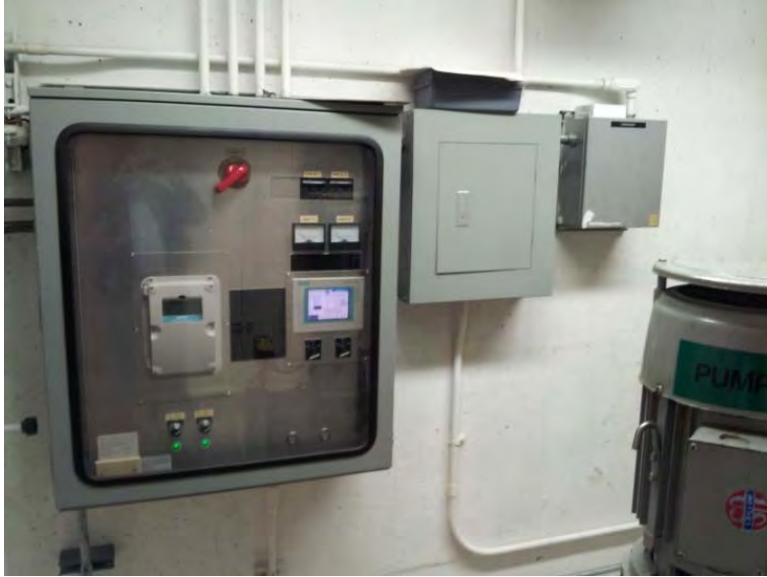
Telemetry control panel located in dry pit, appears to be in good condition
