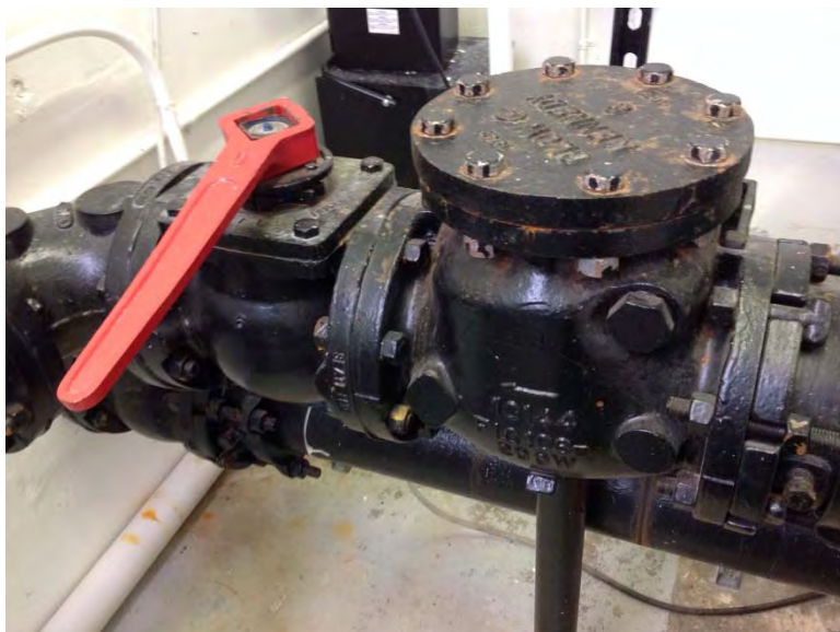
Discharge piping with plug valve and swing check valve with outside lever and spring, plug valve installed with vertical axis of rotation – not ideal
