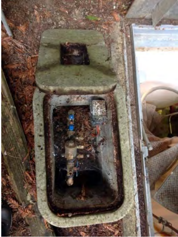
Backflow assembly adjacent to dry pit in above ground concrete meter box
