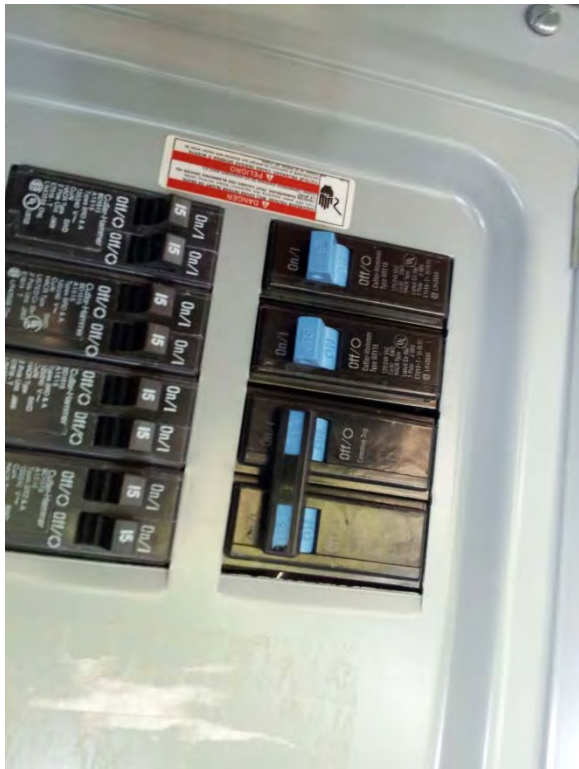
Panelboard located in power and control panel outdoor enclosure, appears to be in good condition
