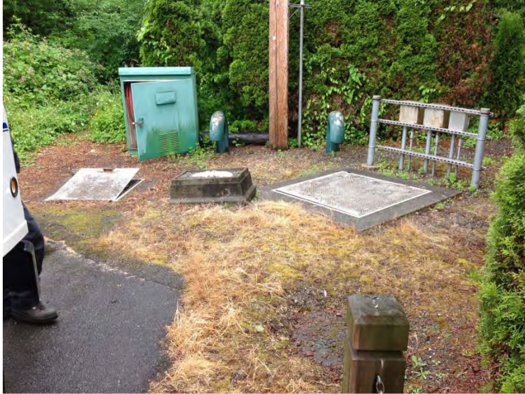
General site, overgrown gravel surfacing and concrete box around high point in vent line approximately 12” high – potential tripping hazard
