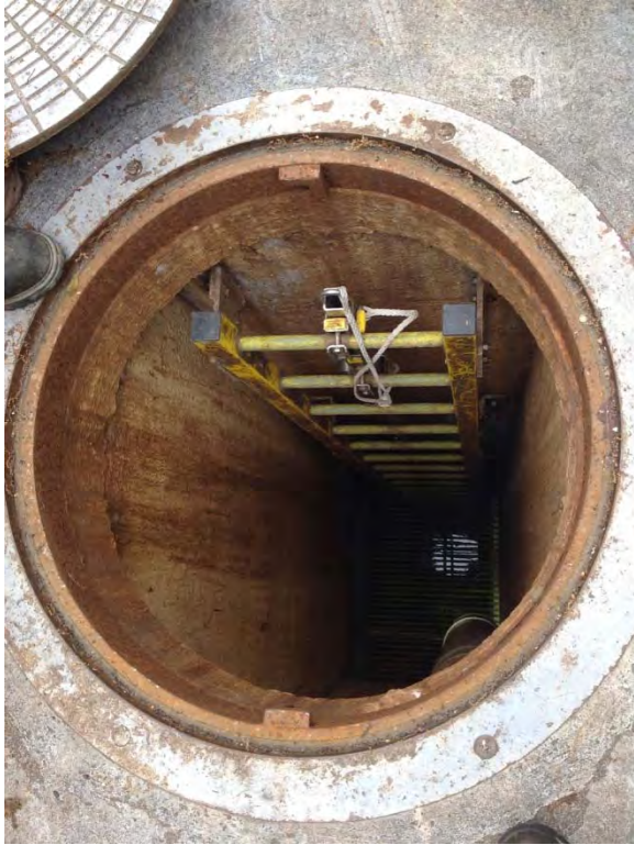
Interior of wet well appears to be in good condition with some degradation
