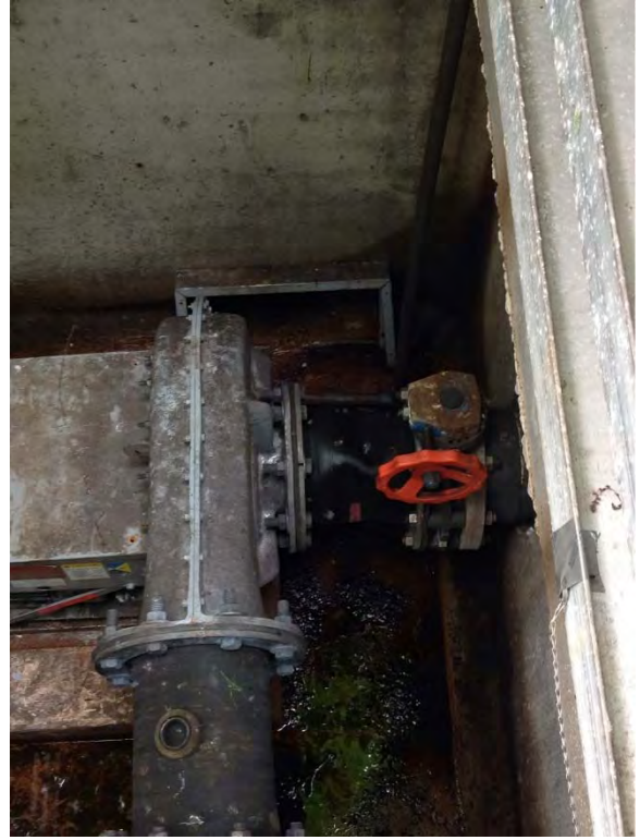
Piping imploded near red hand-wheel, stuck in rigid position even when wet well lid opened
