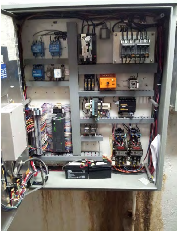
Interior of telemetry control panel
