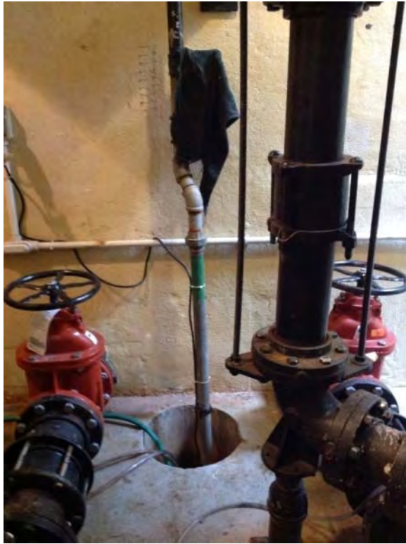
Gate valve with hand wheel on suction piping
