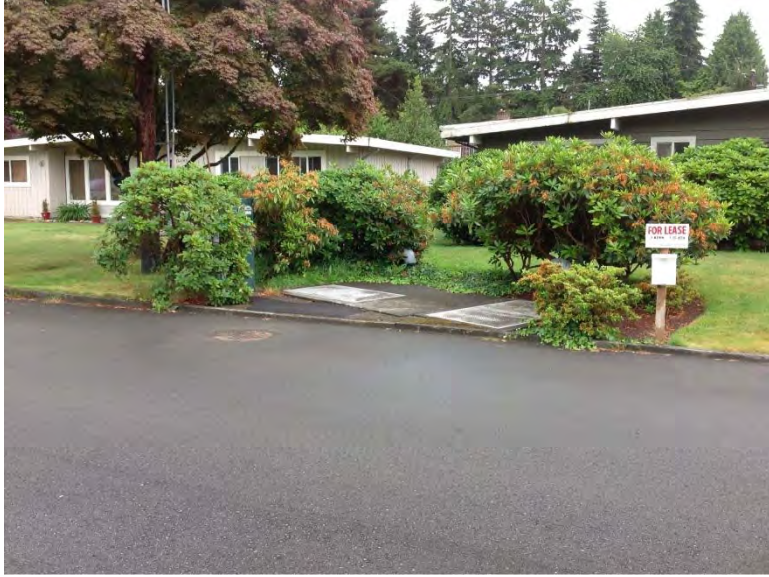
Electrical service meter and generator receptacle located between bushes
