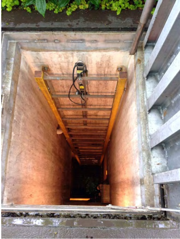
Interior of wet well, showing signs of degradation
