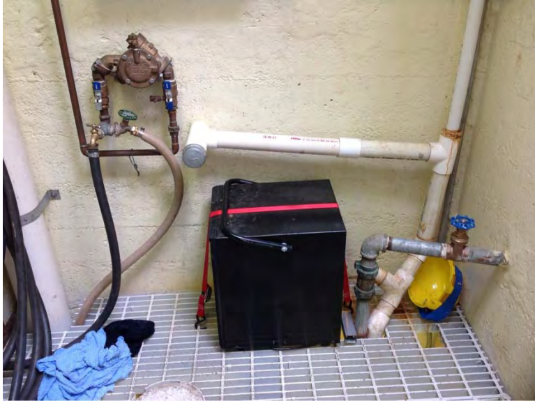
Service valve/connection on top level with hose to pump level
