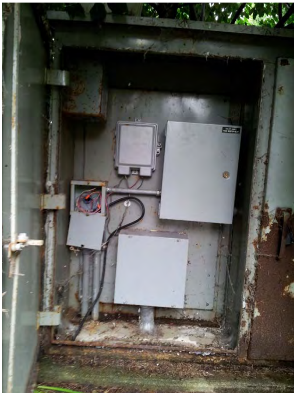
Interior of service cabinet
