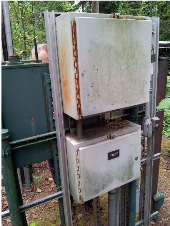
Telephone network interface located on rack along West Lake Sammamish Parkway in NEMA 4 box, showing signs of aging
