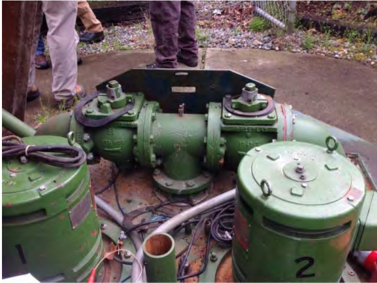
Plug valves, vertical shaft orientation is not desirable due to sediment settling in bottom bearing
