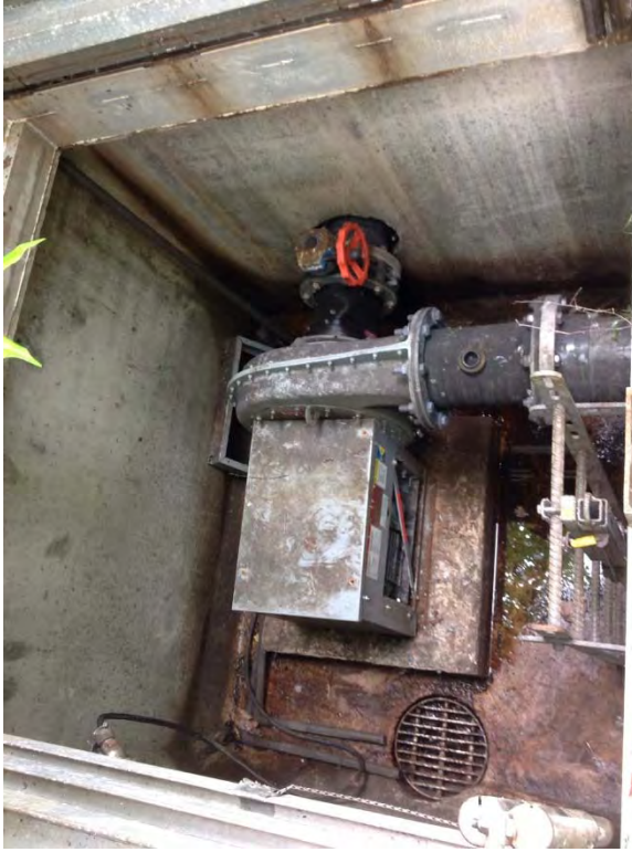
Interior of odor control fan vault, some rusting and water in vault
