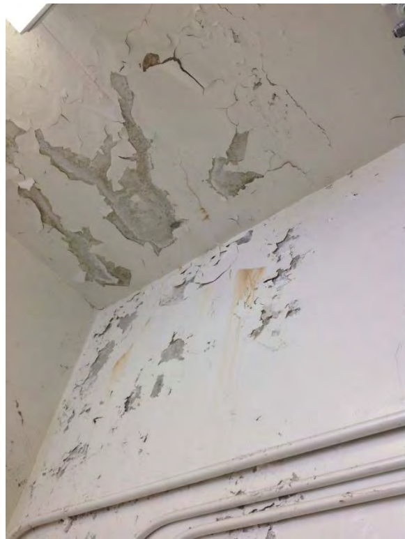
Some coating failure on ceiling – appears to be due to poor prep work
