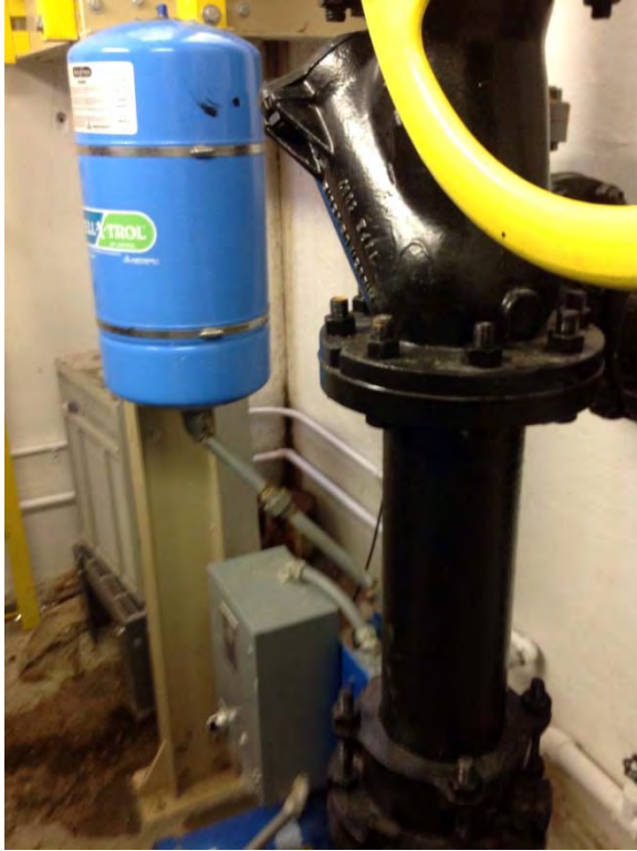
Booster package for water service
