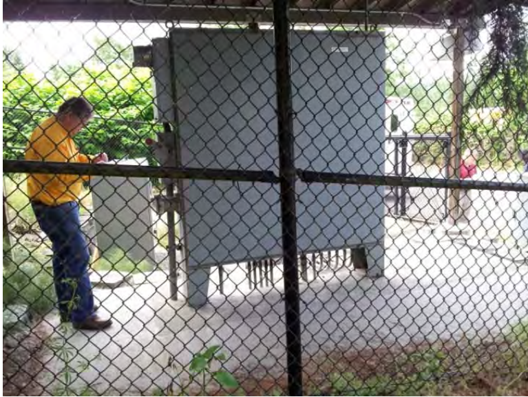
Power and control panel outdoor enclosure located on platform
