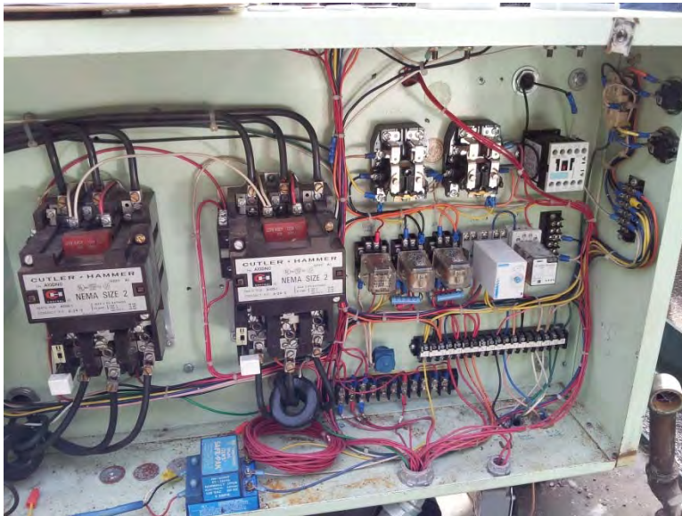
Interior of telemetry control panel, appears to be in good condition
