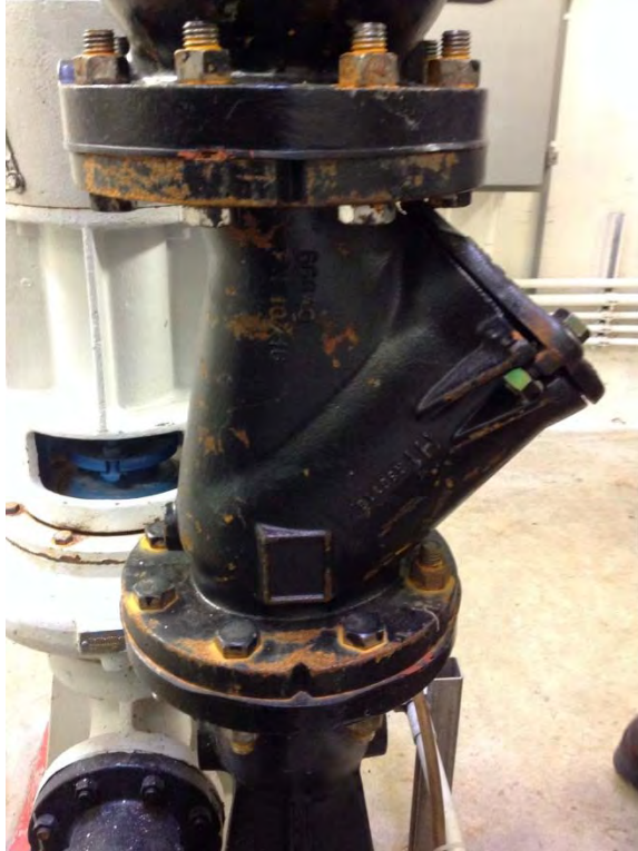
Ball check valve vertical installation on discharge piping
