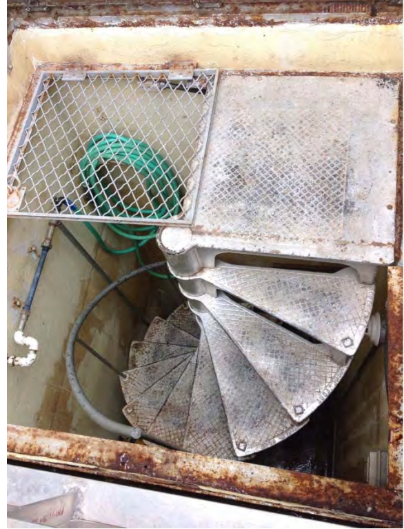
Washdown water supply located in dry pit
