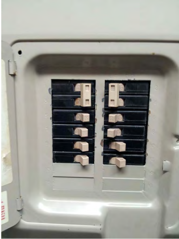
Panelboard located in dry pit, nearing end of its useful life
