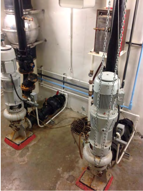
Duplex configuration, pump 2 on the left
