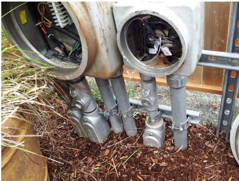
Submersible cable termination enclosure above grade at waterfront
