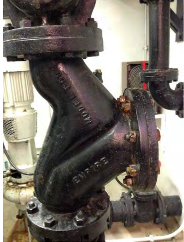
Ball check valve vertical installation on discharge piping
