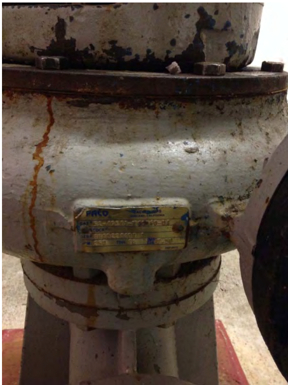
Pump 1 showing signs of aging on exterior
