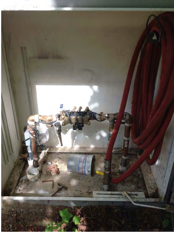
Backflow prevention assembly in above grade stainless steel insulated enclosure
