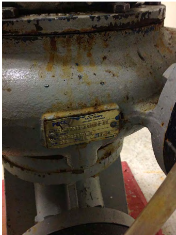
Pump 2 showing signs of aging on exterior
