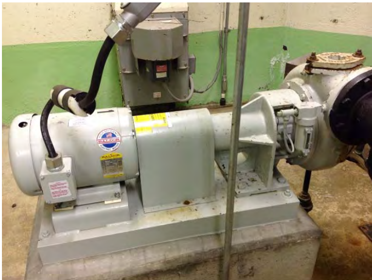
Pump and motor #1
