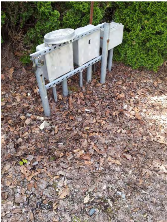
Submersible cable termination enclosure in above grade explosion proof box
