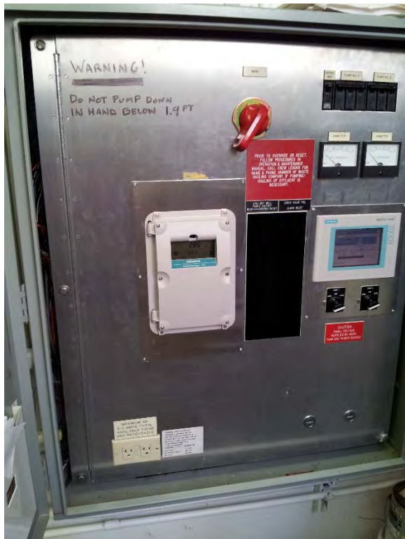
Starters located in dry pit
