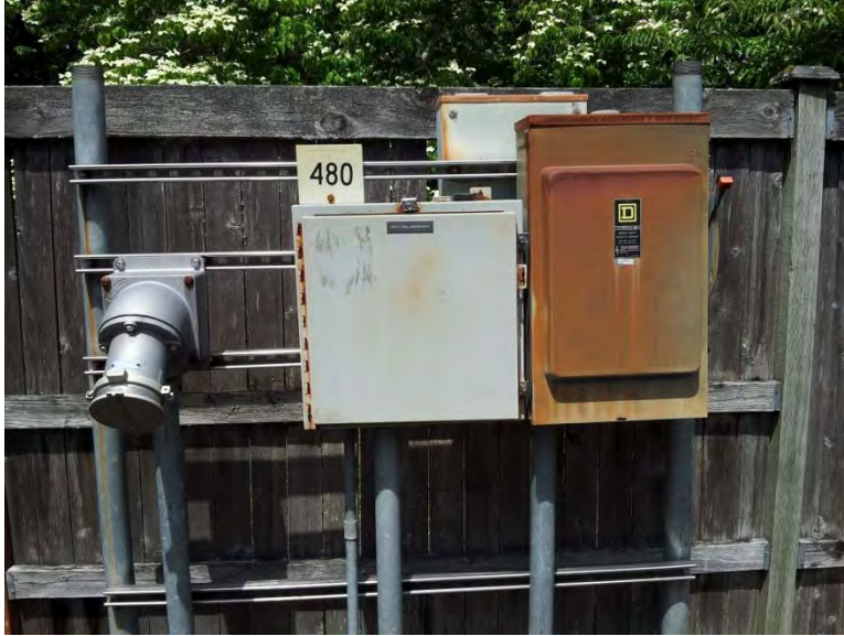
Service entrance equipment rack including generator receptacle located behind arborvitae adjacent to site
