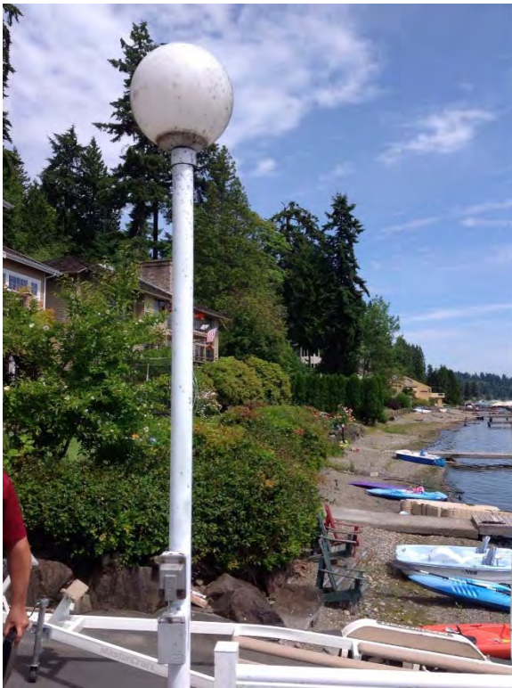
Site lighting between dry pit and wet well on deck area adjacent to station
