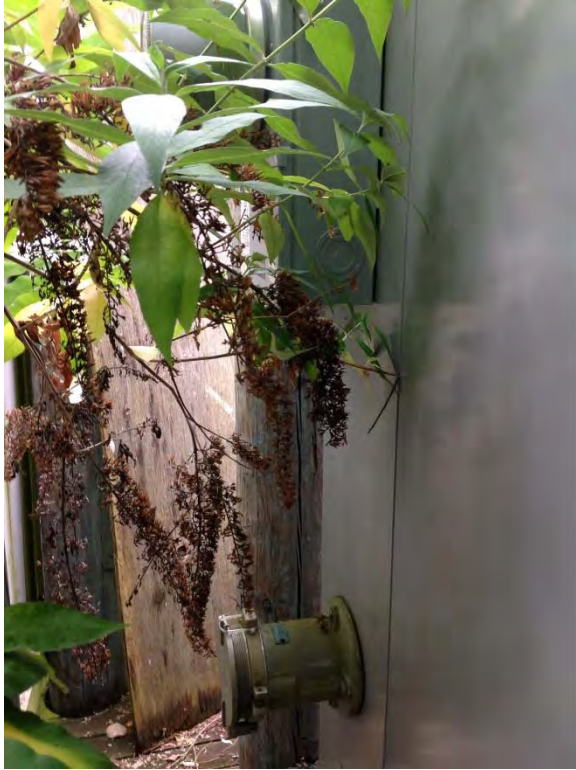
Service meter and generator receptacle located on side of power and control panel enclosure near paved road
