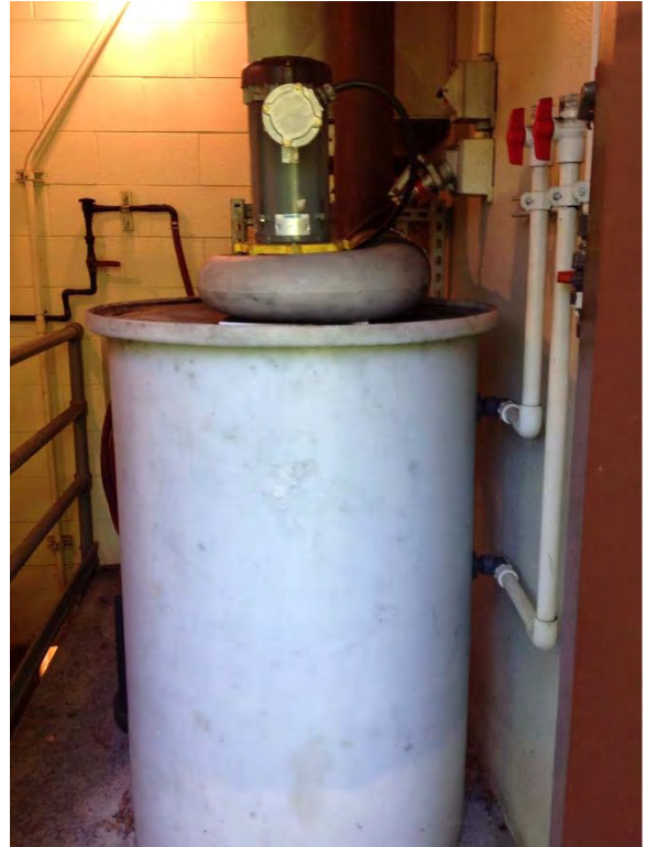
Wet well ventilation exhaust fan and carbon canister located in wet well access room
