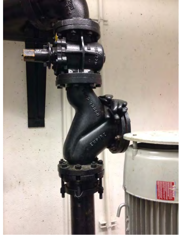
Ball check valve vertical installation and plug valve isolation on discharge piping
