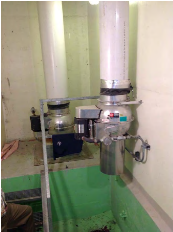
Wet well ventilation configuration in wet well access room, supply fan in foreground, exhaust fan in background
