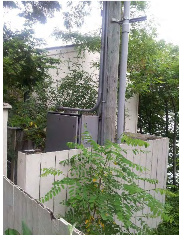
No vent fan in outdoor power and control panel enclosure, it is sheltered however, so it should stay cool
