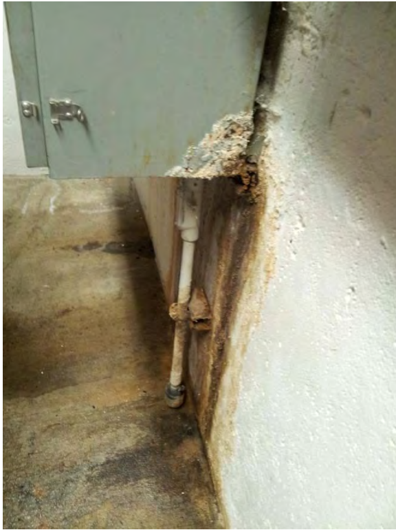
Some corrosion on telemetry control panel but other than that appears to be in good condition
