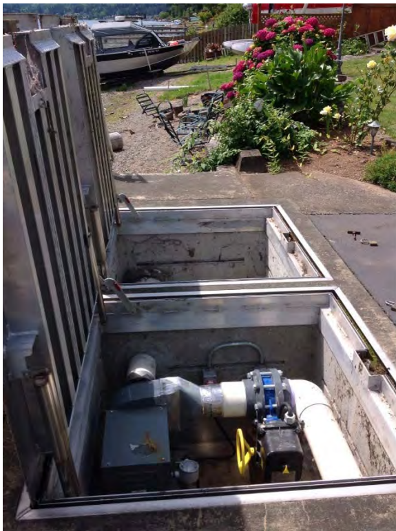
Air intake for wet well supply fan and dry pit exhaust fan located in vault
