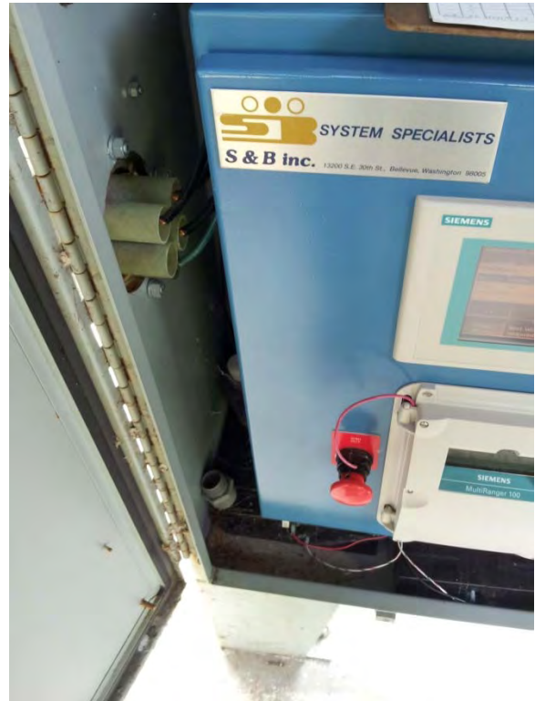
Generator receptacle needs to be mounted for clearance of conductors, alternate view
