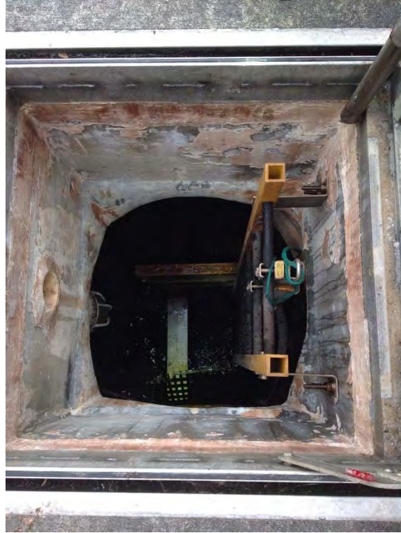
Some delaminating in interior, but no signs of corrosion
