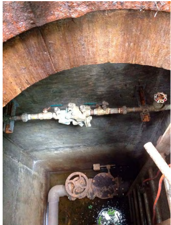
Backflow prevention assembly located in check valve/isolation valve vault
