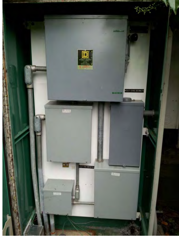
Interior of service equipment cabinet
