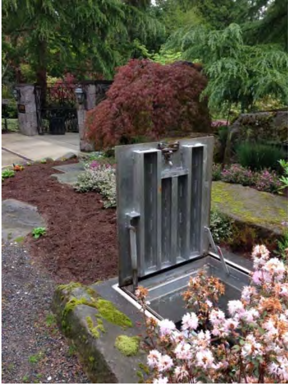
Generator vault located adjacent to street
