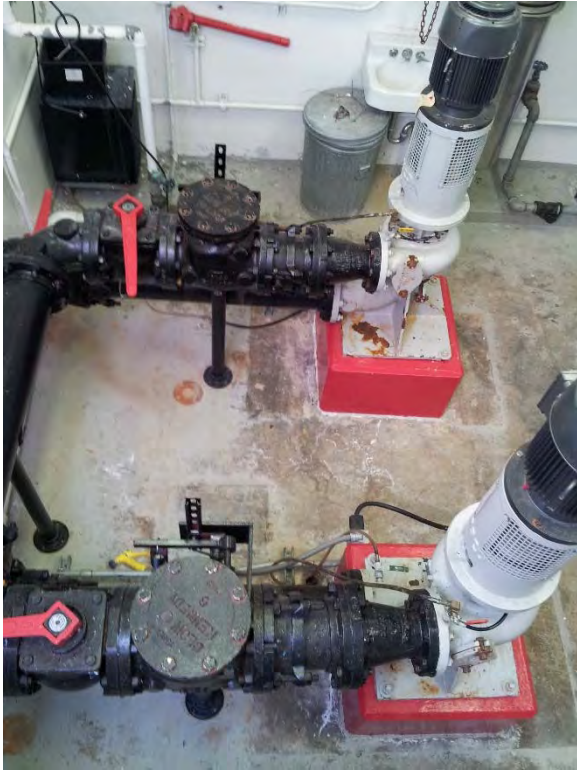
Duplex configuration, pump #2 in background
