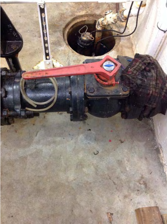
Plug valve isolation for suction piping, vertical axis of orientation – not ideal
