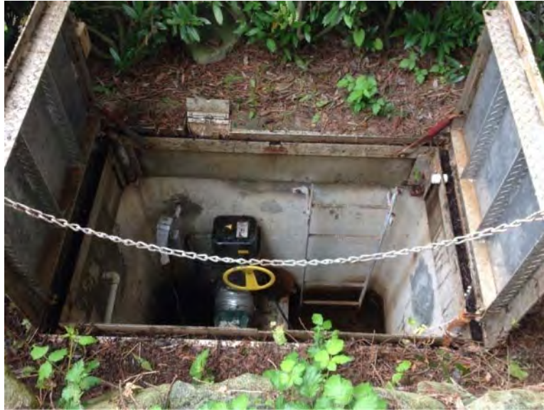
Fall protection on one side of wet well blower vault
