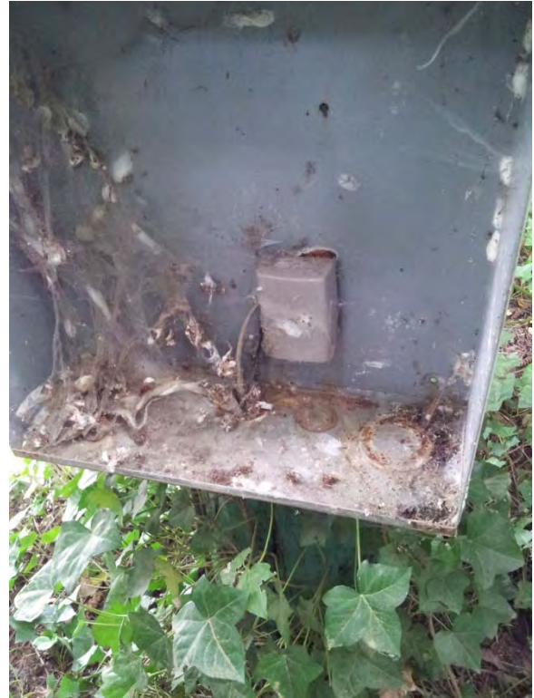
Telephone network interface located in oversized outdoor panel
