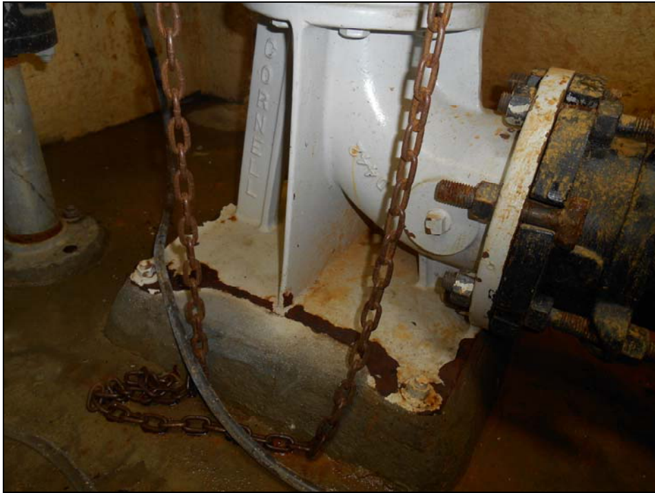
Photo 5: Rust at Pump Base Anchorage Plate
