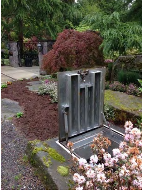
Generator vault on side of road
