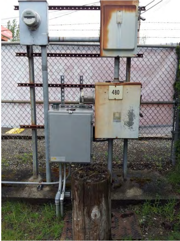
Utility service and generator receptacle, clearance issue with wood pole
