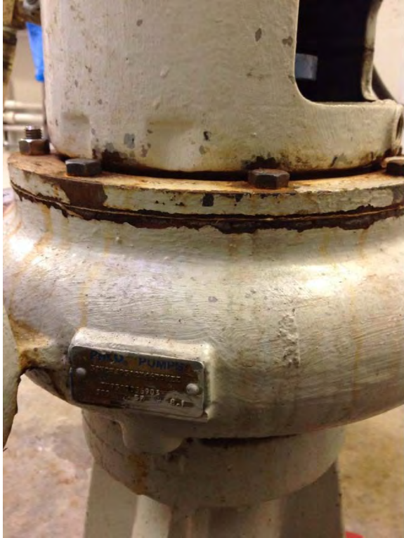
Pump 2 showing signs of aging on exterior
