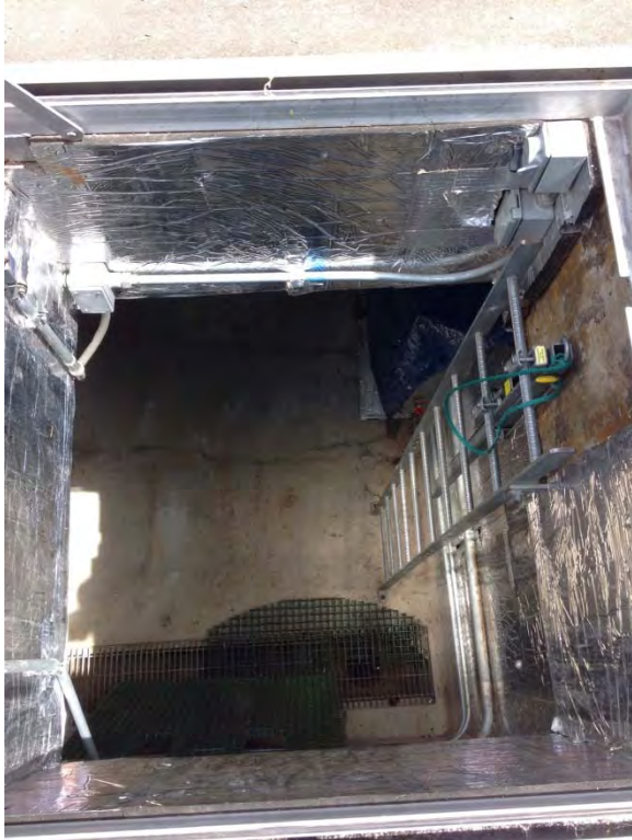
Interior of dry pit/generator vault with sound proof panels
