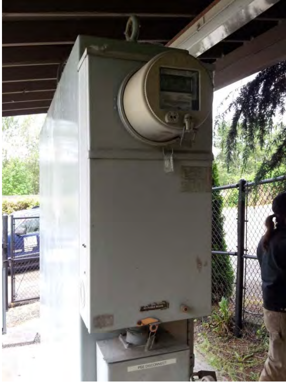
Service meter located on side of power and control panel
