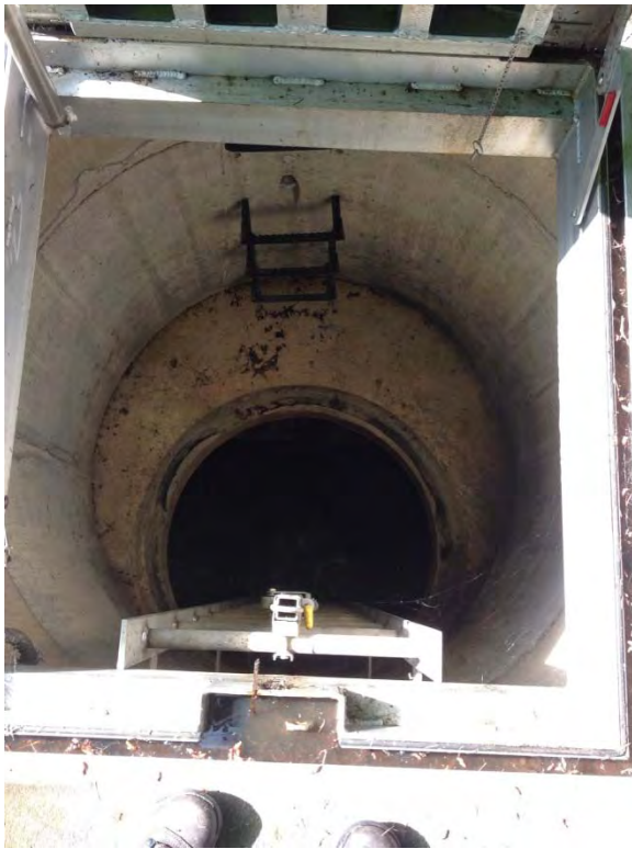
Interior of overflow wet well
