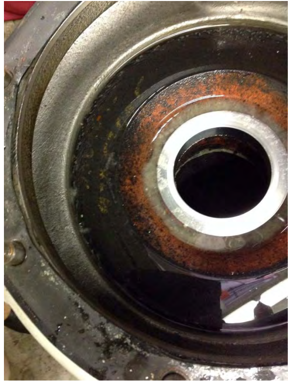
Interior of Pump 2A volute with pitting and grooves
