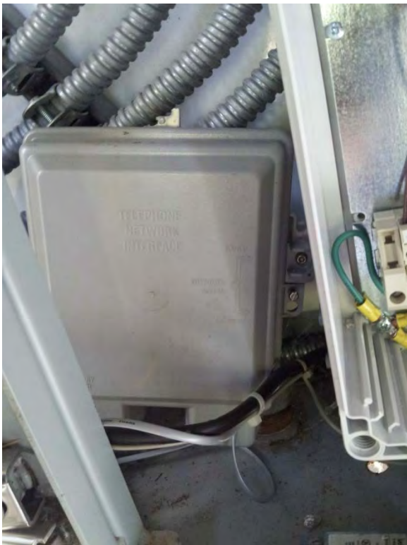
Telephone network interface located in power and control panel enclosure
