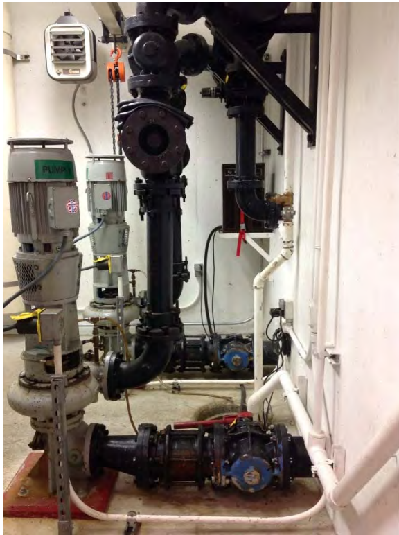
Interior of dry pit appears to be in good condition with good lighting
