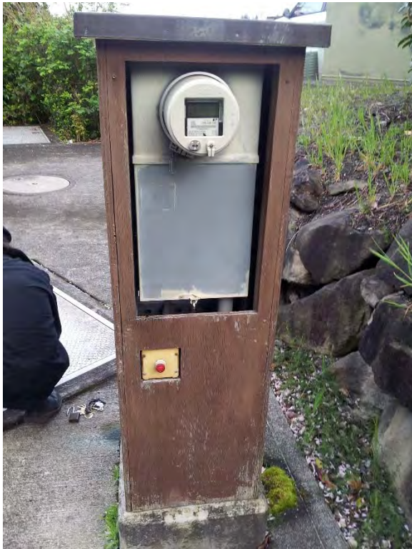
Service meter located on outdoor pedestal, appears to be in good condition
