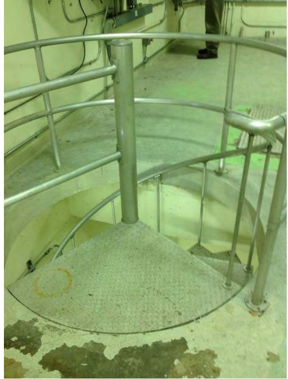
Dry pit/pump level accessed from spiral staircase in control building
