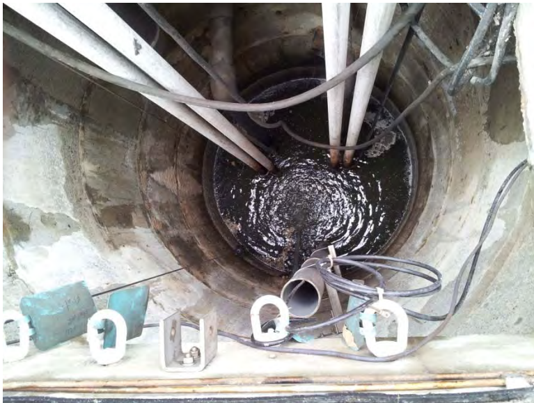
Discharge piping in wet well, piping is grey
