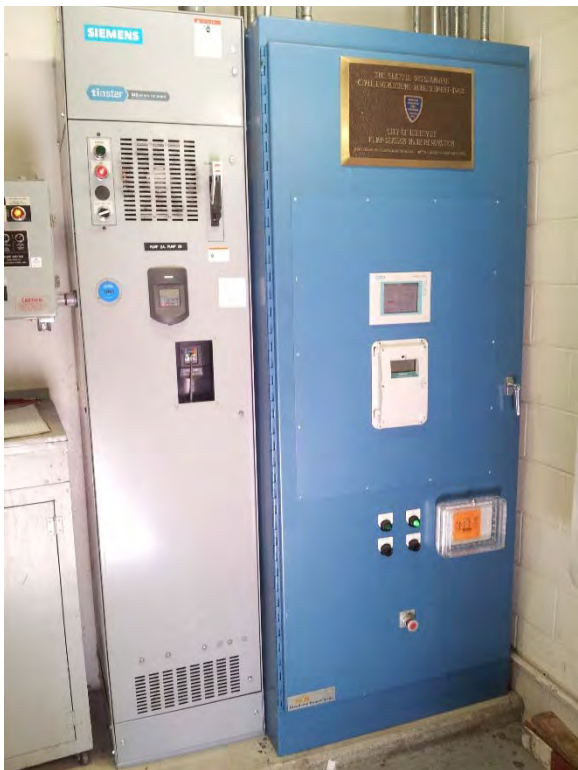
Starters for Pump 2A and 2B, appears to be in good condition but aging
