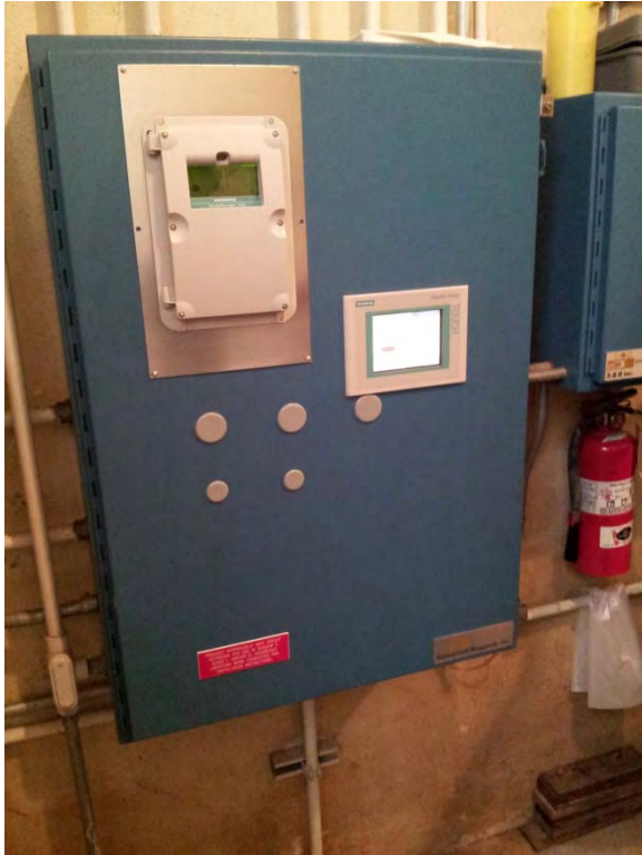
Telemetry control panel located in dry pit, appears to be in good condition
