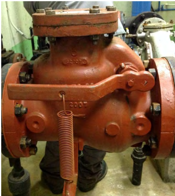
Swing check valve with outside lever and spring on discharge piping
