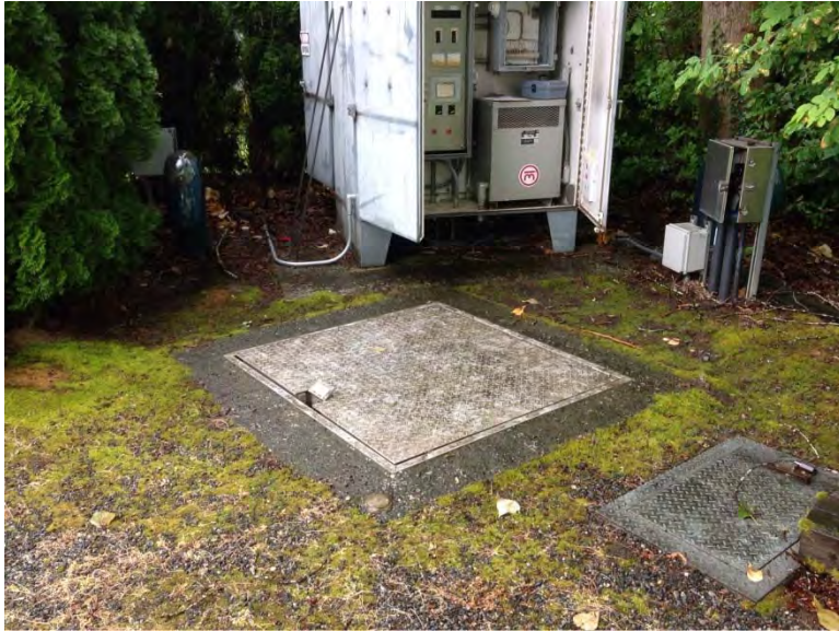
Outdoor power enclosure
