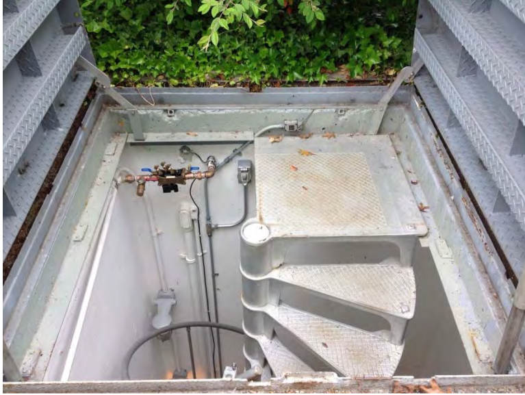
Dry pit access to top of spiral stair case on opposite side of accessibility
