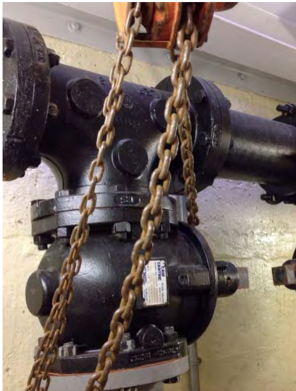
Picking eye is attached to above platform – corrosion issue on mid level grating platform
