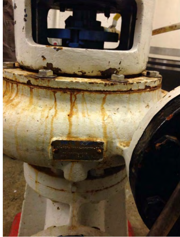
Pump 2 showing signs of aging on exterior
