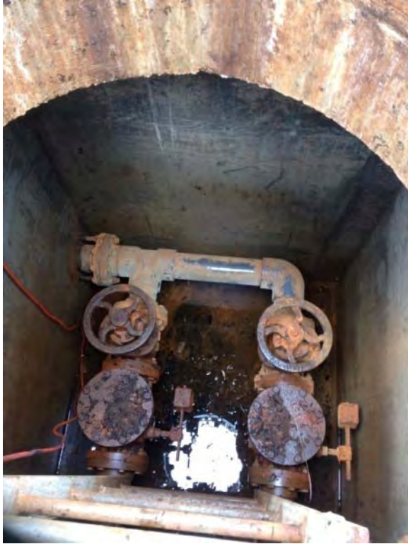
Swing check valves and gate valves with hand wheel
