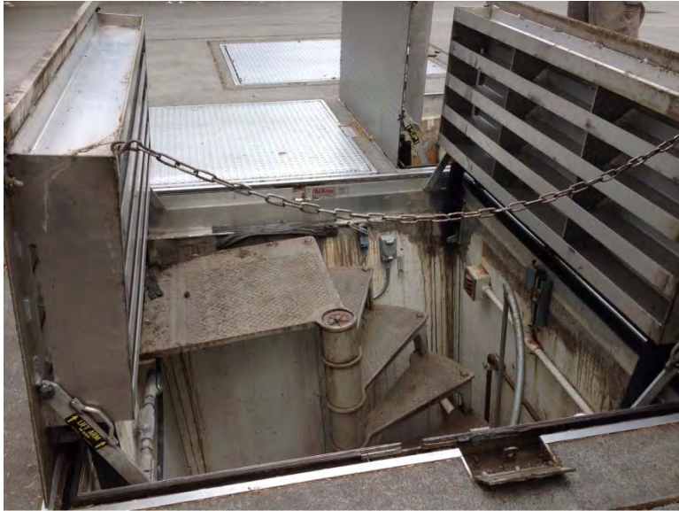
Access fall protection on one side of hatch opening
