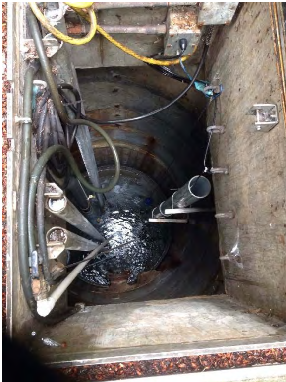
Hose for wash down water located at top of wet well
