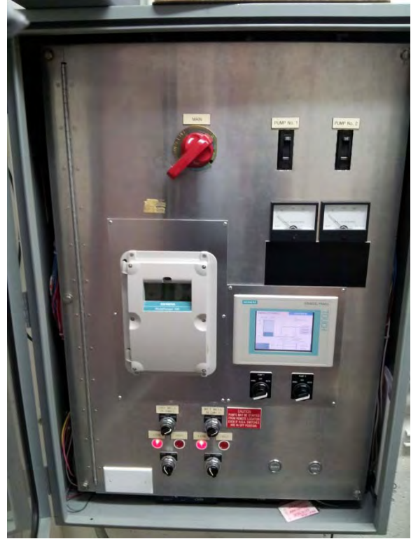
Original starters located in dry pit, nearing end of useful life
