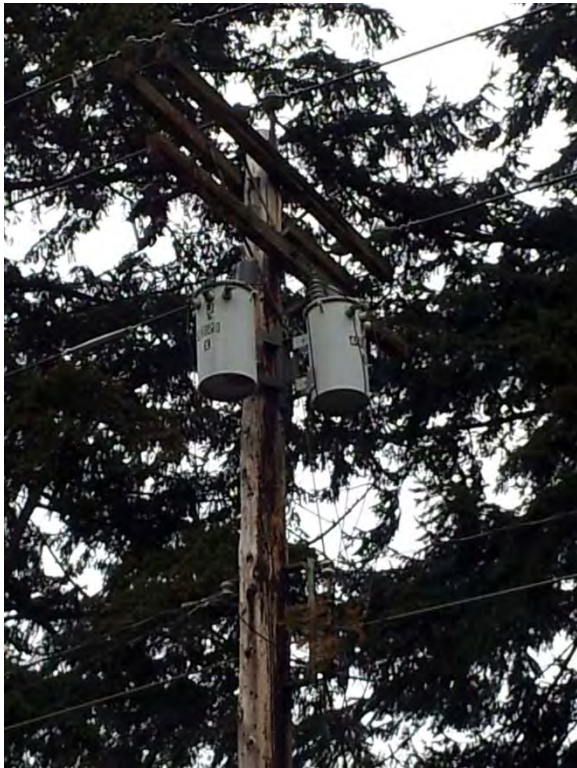
Overhead utility transformer
