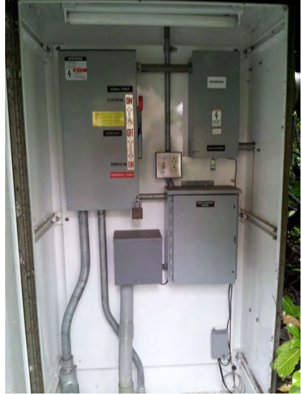
Telephone network interface located in service cabinet
