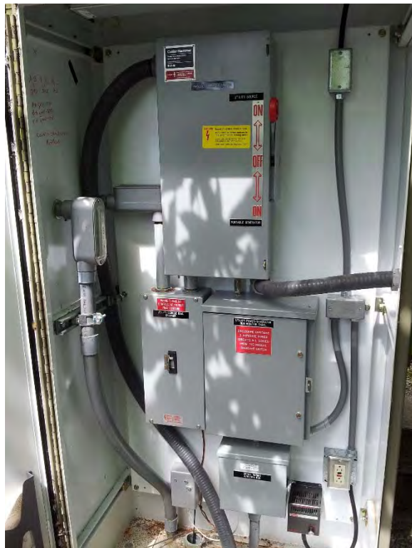
Interior of power cabinet
