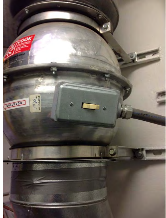
Dry pit supply fan located 6' AFF in dry pit
