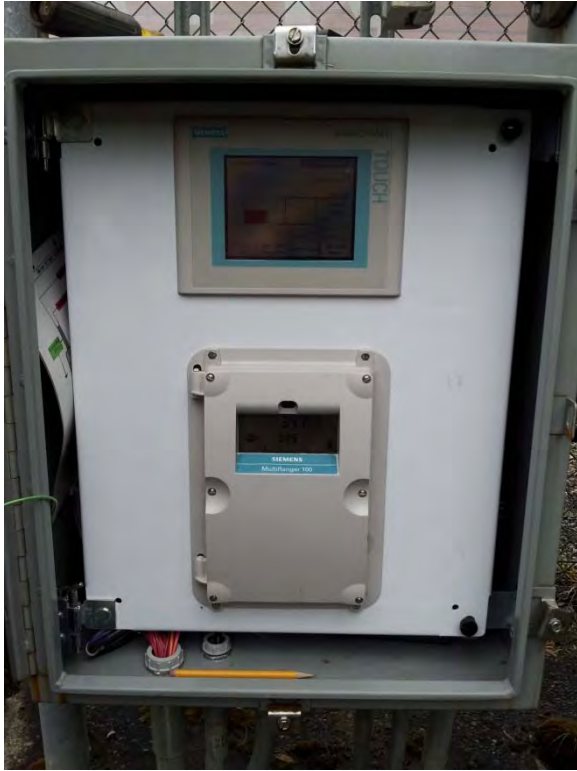
Operator interface located on steel rack
