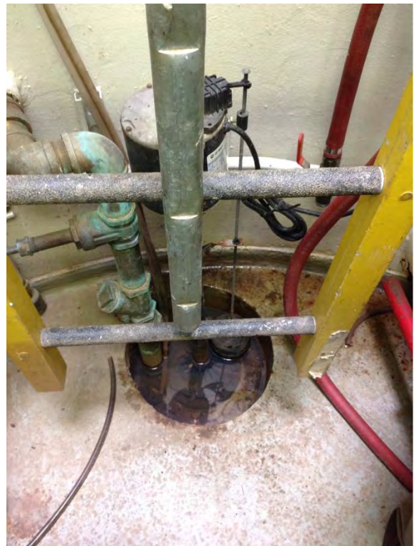
Wash down water hose in dry pit
