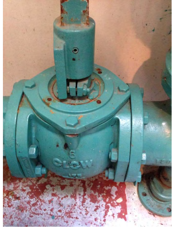
Plug valve isolation for discharge piping, vertical axis of orientation – not ideal
