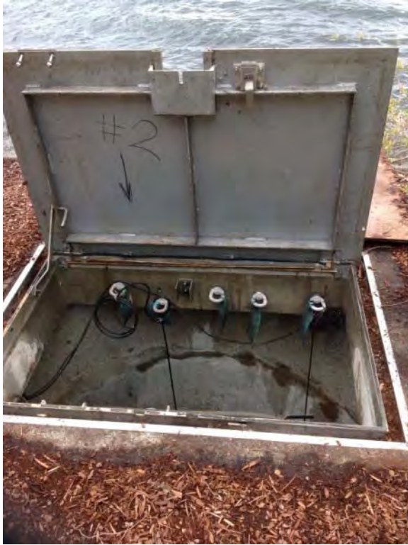
Wet well is located directly adjacent to lake
