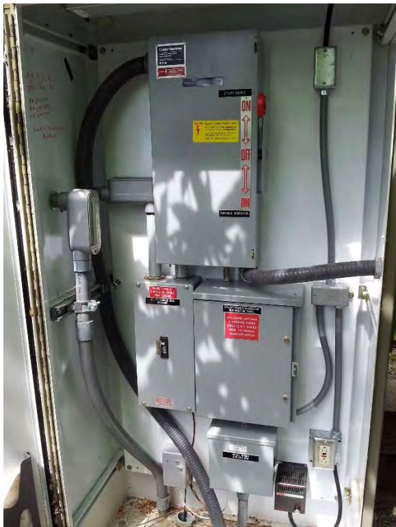
Telephone network interface located in outdoor power cabinet
