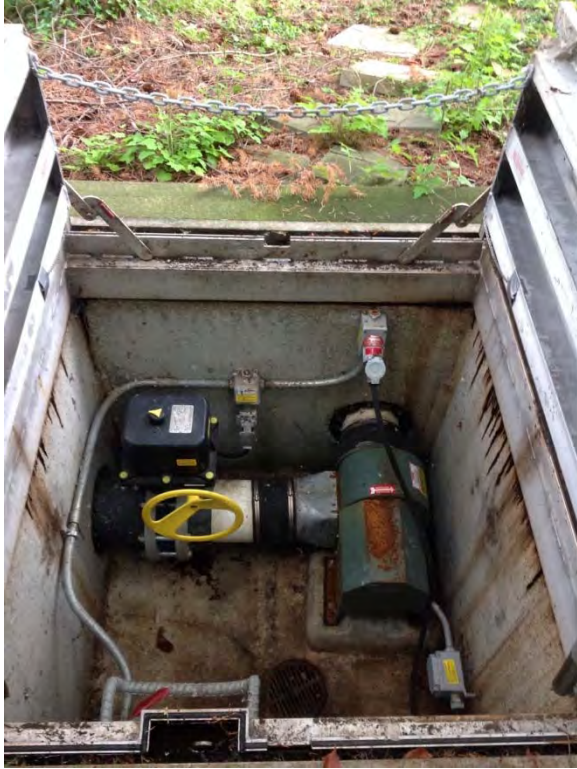
Wet well supply fan located in wet well blower vault
