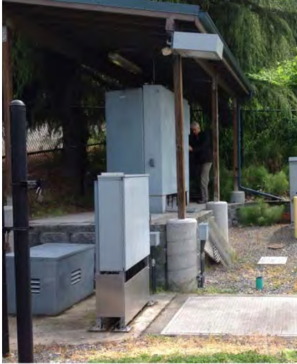
Main control cabinet up 2' – 3', no railing – potential safety issue
