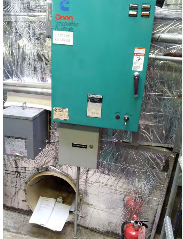
Transfer switch located in generator vault
