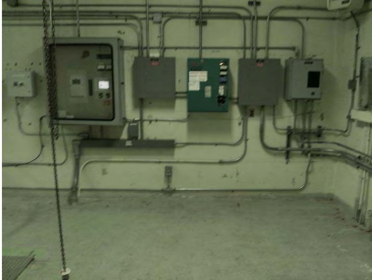
Layout of electrical/telemetry equipment on top floor of control building
