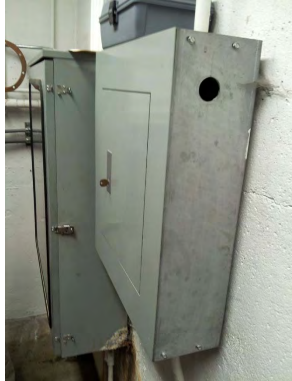
Hole in panelboard
