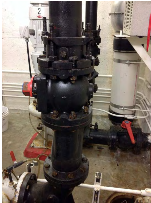
Ball check valve and plug valve on discharge piping
