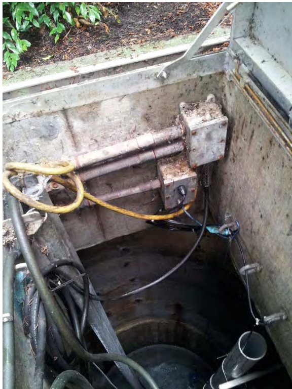
Submersible cable termination enclosure located in wet well, not fully secured and some corrosion evident
