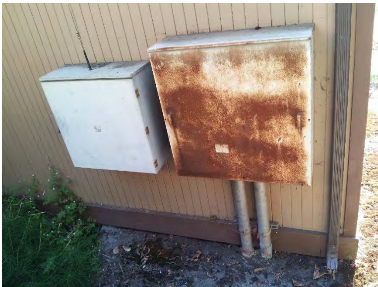
Utility service meter located in back of building, current transformer compartment very rusty
