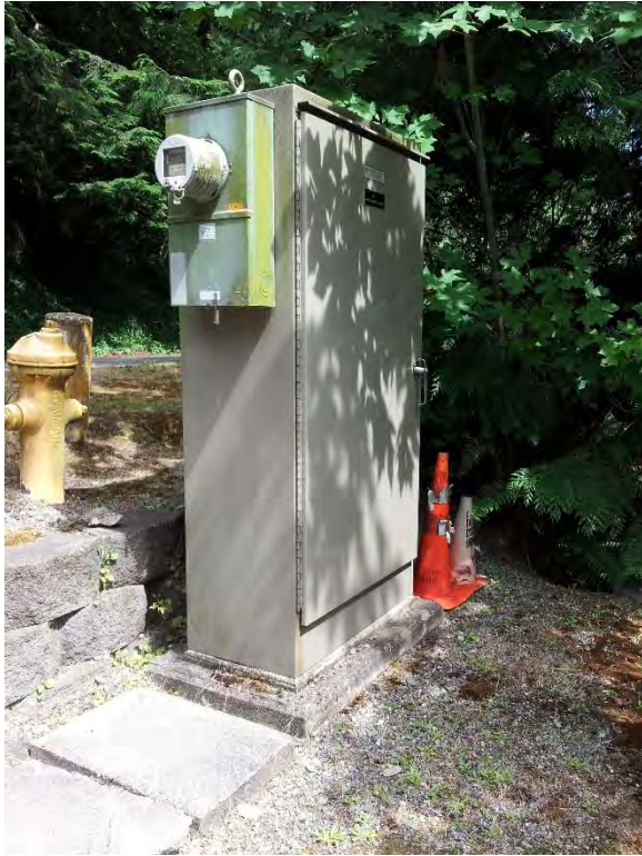
Service meter located on outdoor power cabinet
