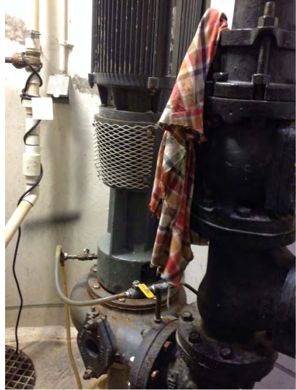
Pump and motor #1
