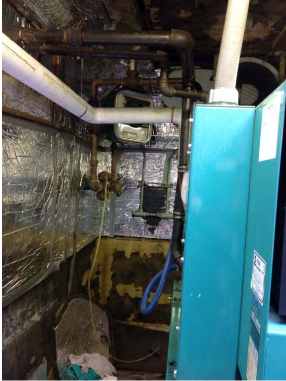
Backflow prevention assembly in generator vault
