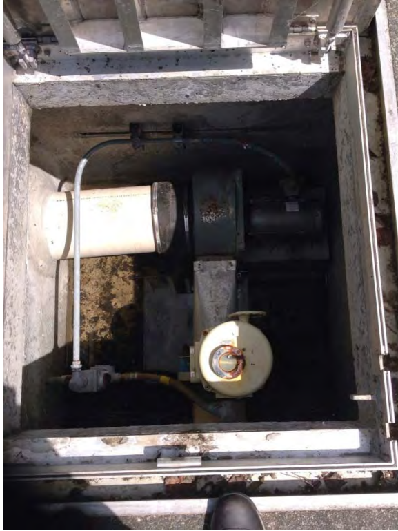
Wet well fan located in wet well blower vault
