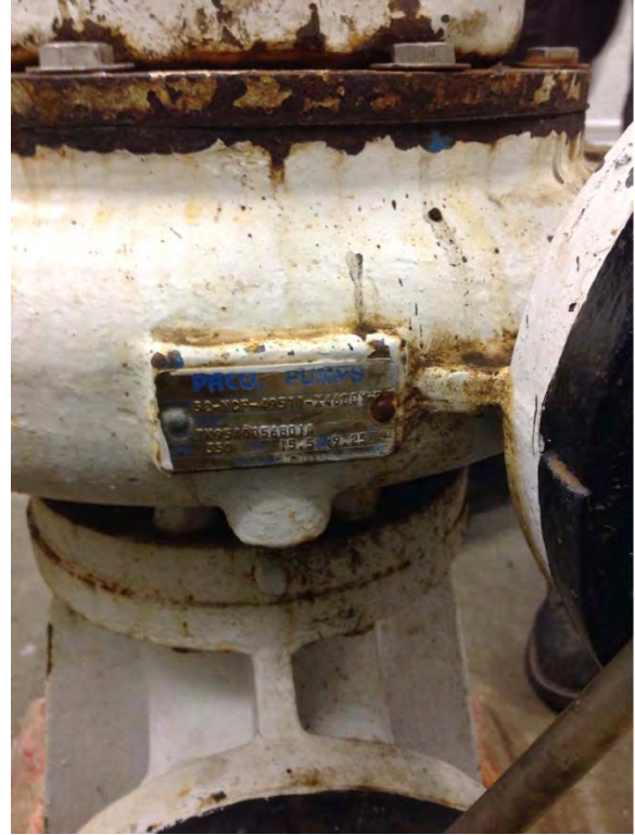
Pump 1 showing signs of aging on exterior
