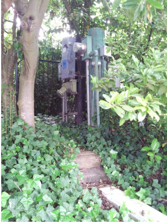
Utility service and generator receptacle located in raised landscaping area
