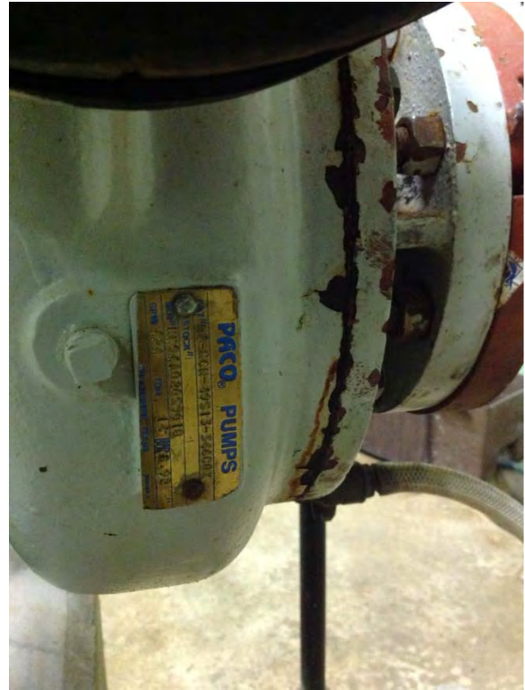
Pump 1 showing signs of aging on exterior
