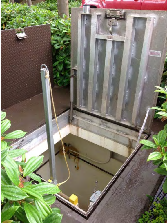
Lift assist hatch and post to access ladder to first level
