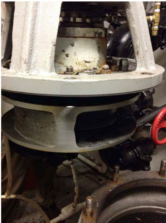
Pump 2B disassembled upon site visit to observe interior of volute
