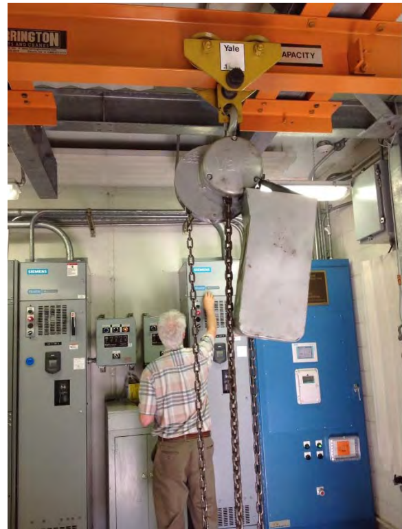
Box for chain fall is 5' -6" AFF, potential safety hazard
