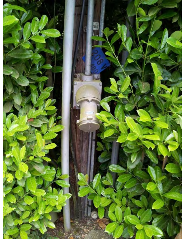
Generator receptacle located on pole near Evergreen Point Road
