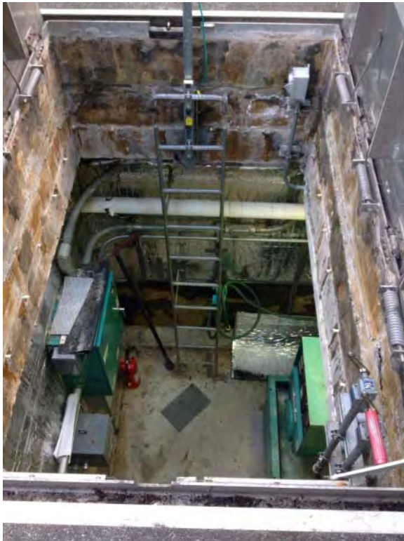
Interior of generator vault, no fall protection
