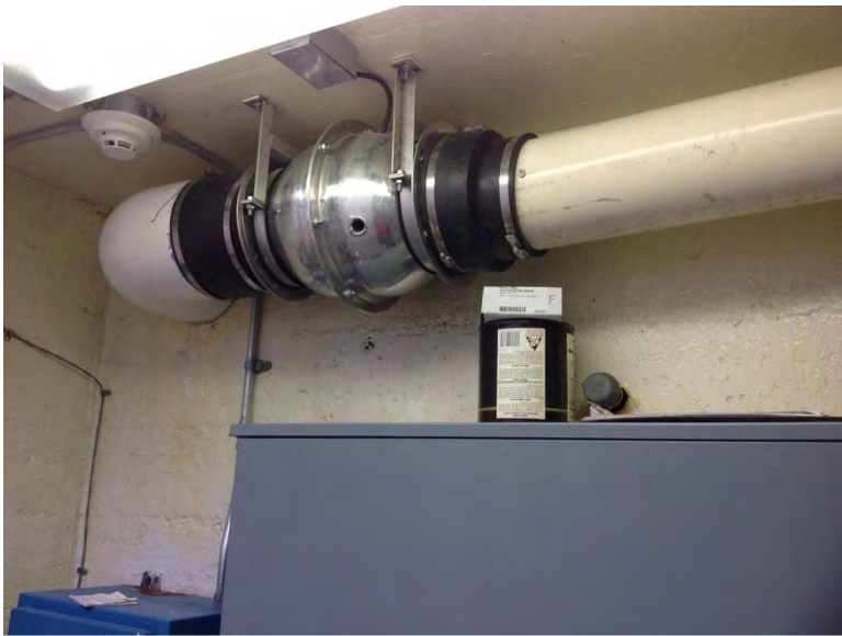
Dry pit supply fan located at ceiling at upper level
