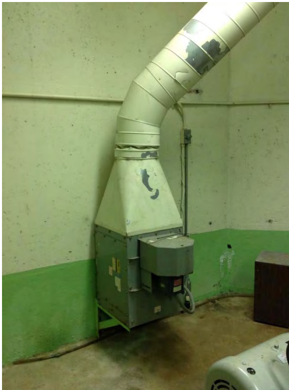
Exhaust fan located 2' AFF at pump level
