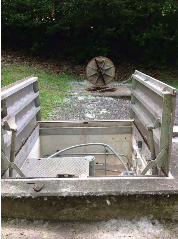
Lift assist hatch and chain fall protection on one side
