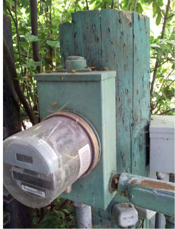
Service meter located on wood pole
