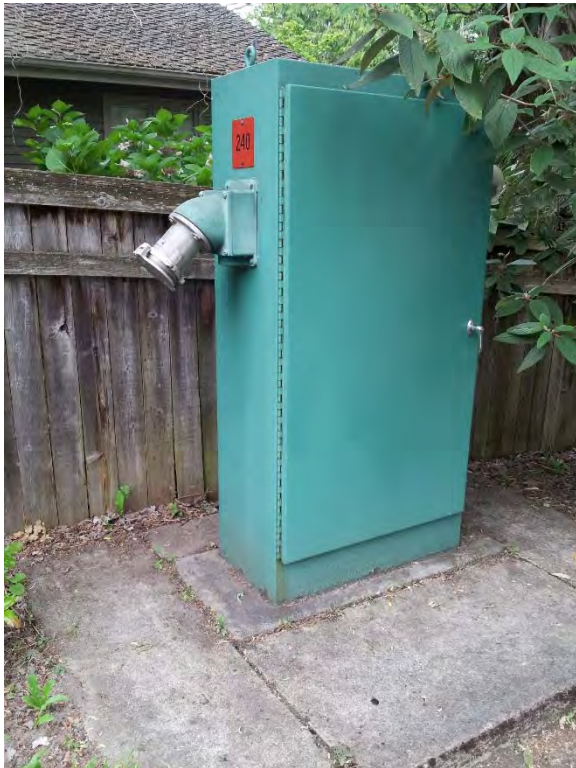
Generator receptacle located on outside service cabinet
