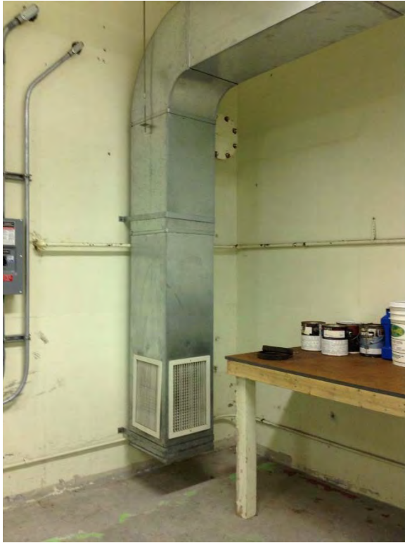
Supply fan duct work located in control building
