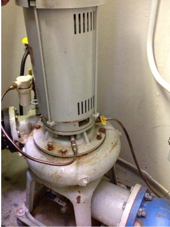
Pump and motor #2
