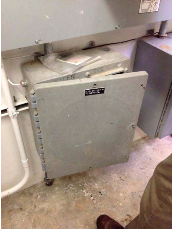
Flush 10 telemetry panel
