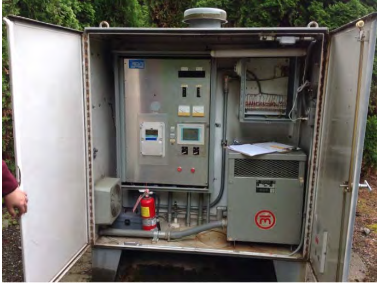
Control enclosure located on opposite side of outdoor power enclosure
