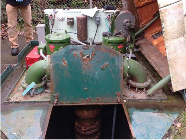
Pumps below steel plate, could not observe
