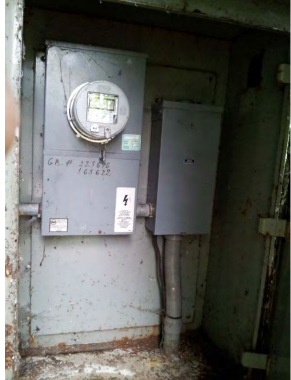
Service meter located in rusty service cabinet
