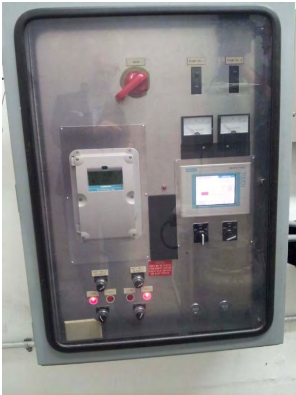
Telemetry control panel appears to be in good condition
