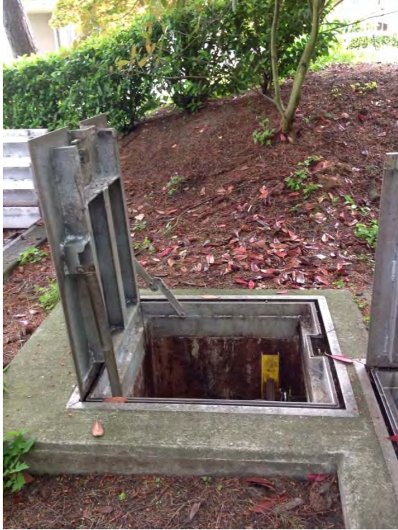
Wet well access hatch
