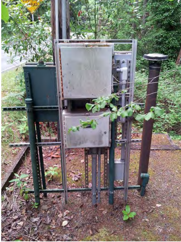
Utility service and back-up power located adjacent to West Lake Sammamish Parkway on steel rack
