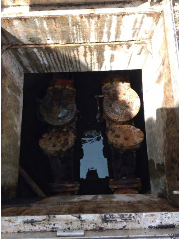
Isolation and check valve vault, flooding evident, check valve leaking upon site visit
