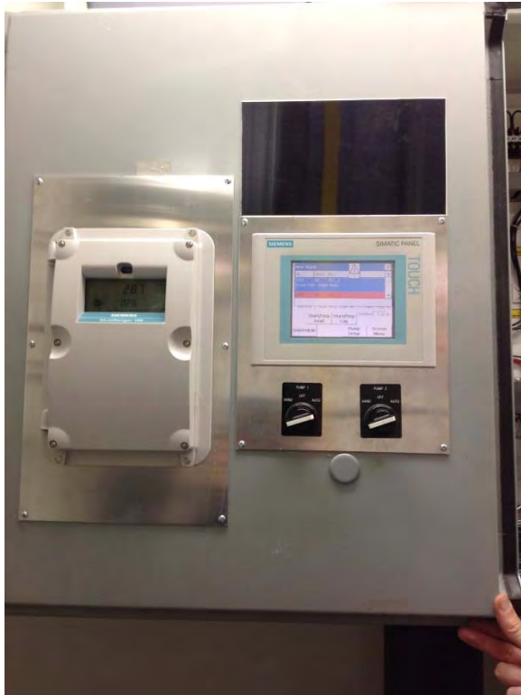
Telemetry control panel located in dry pit with operator interface, appears to be in good condition but with some clearance violations
