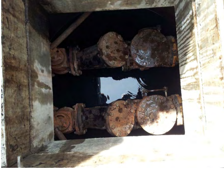
Plug valve and swing check valve with outside level and spring located in isolation and check valve vault, some rusting evident
