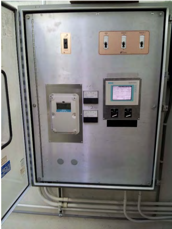
Telemetry control panel with operator interface located in dry pit, appears to be in good condition
