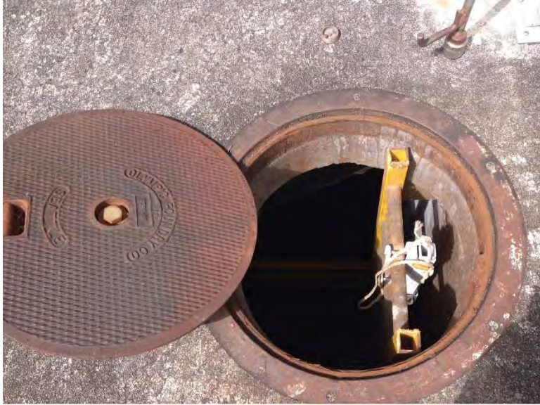
Wet well manhole lid and ladder, interior appears to be in good condition
