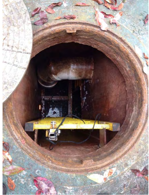
Interior of wet well, 30" back from ladder to 12" diameter PVC vent pipe
