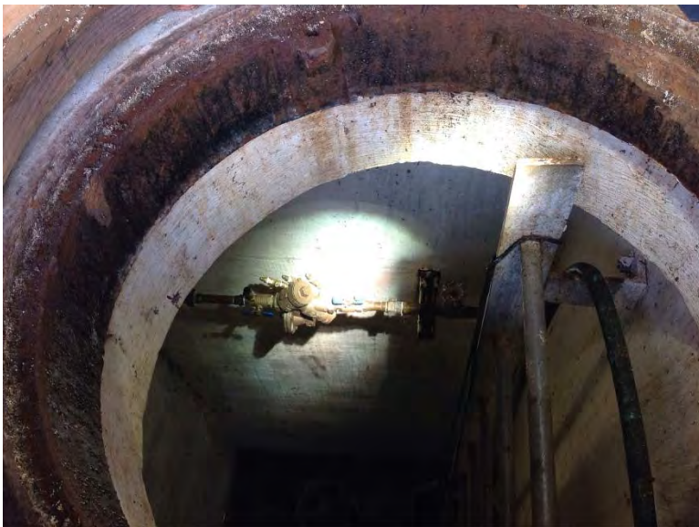
Reduced pressure backflow assembly located in check valve and isolation valve vault
