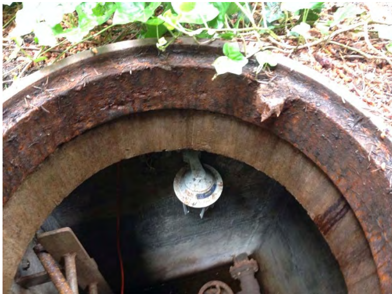
Valve vault light can be plugged in with extension cord, extension cord located in vault upon site visit
