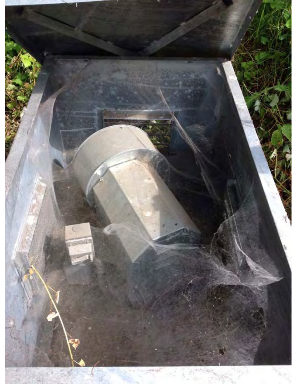
Interior of above grade supply fan vents, a lot of cobwebs, some branches inside
