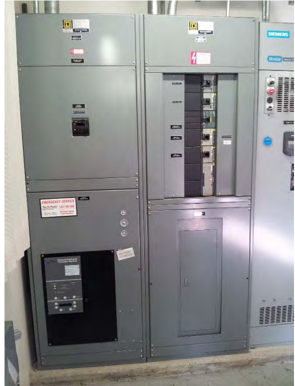
Transfer switch located in top floor of building, appears to be in good condition but aging
