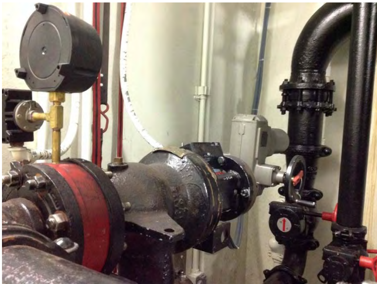
Discharge piping with automated check valve
