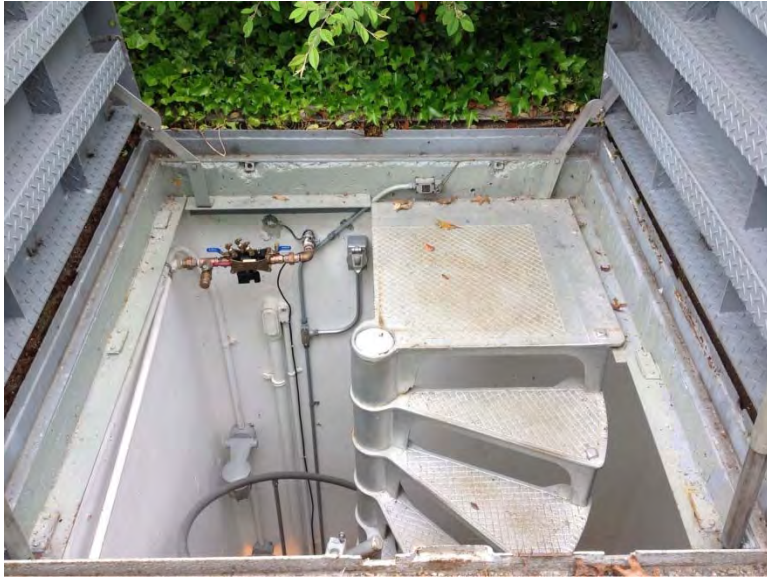
Potential safety issue, stepping over to spiral staircase landing
