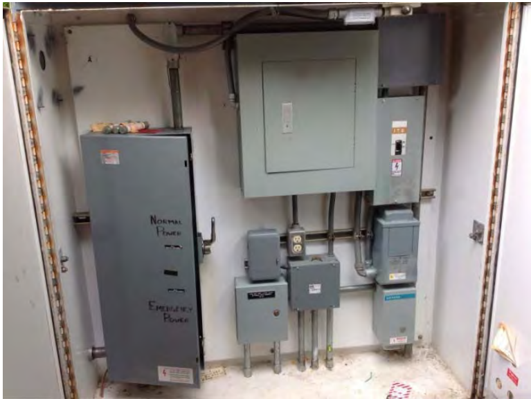
Panelboard located in outdoor power enclosure
