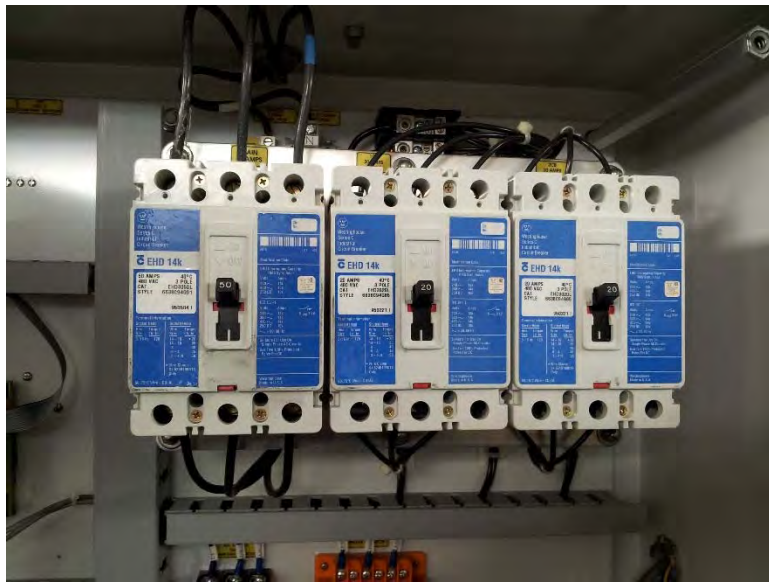
Westinghouse circuit breakers appear to be in good condition
