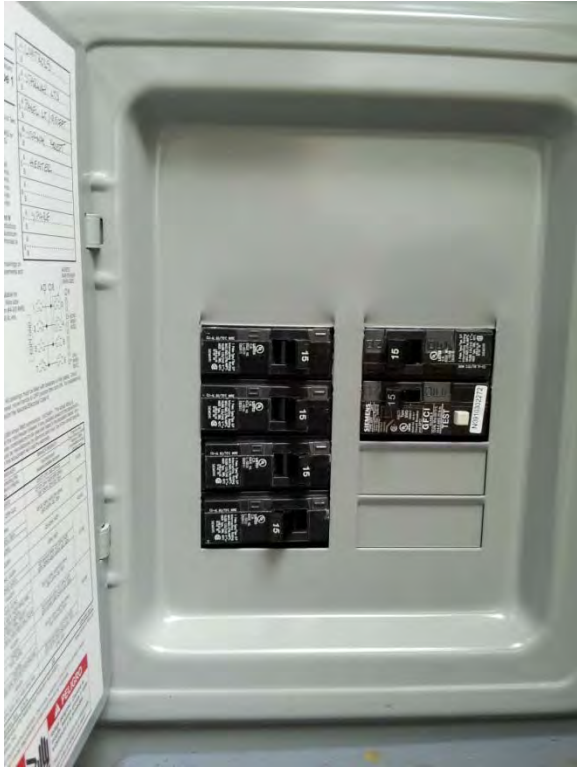
Panelboard located adjacent to street
