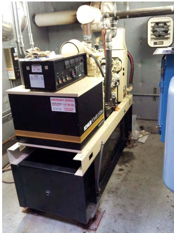
Interior of generator vault
