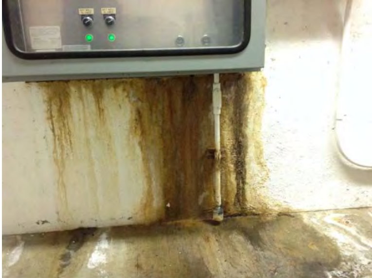
Evidence of water damage behind panel – no new leakage observed
