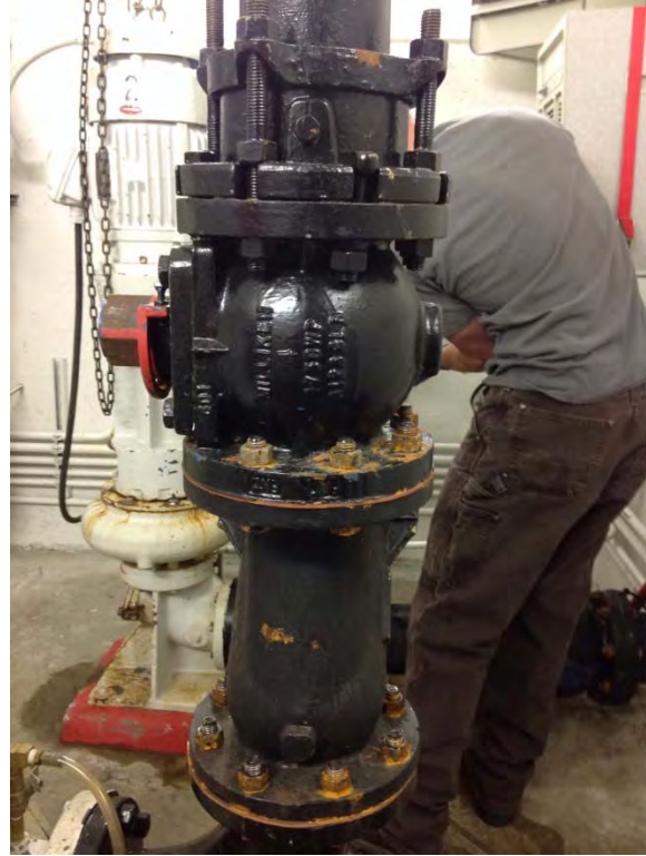
Ball check valve vertical installation and plug valve on discharge piping
