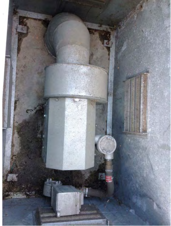
Wet well exhaust fan located in above grade enclosure
