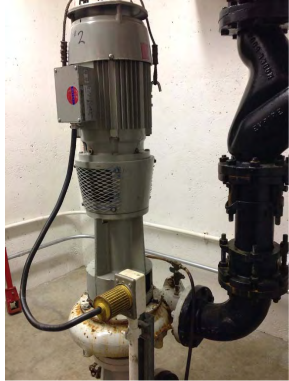
Pump and motor #2
