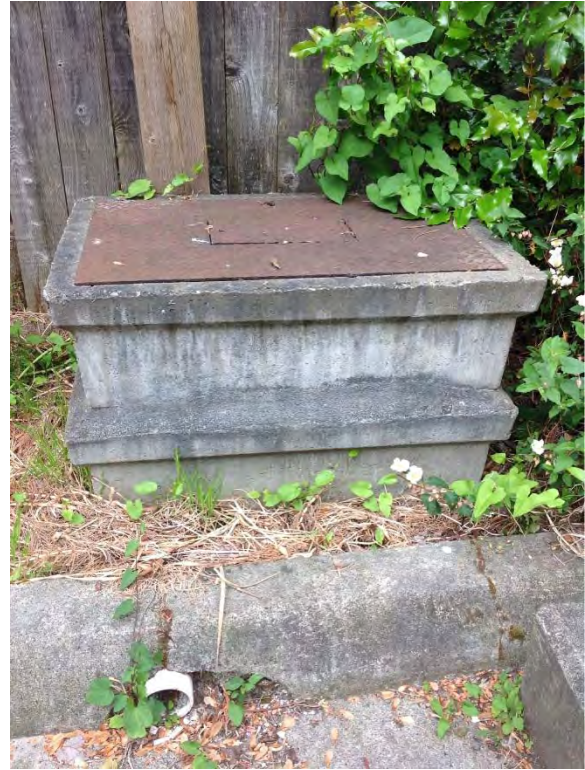
Backflow prevention assembly in two stacked water boxes, 12" above grade
