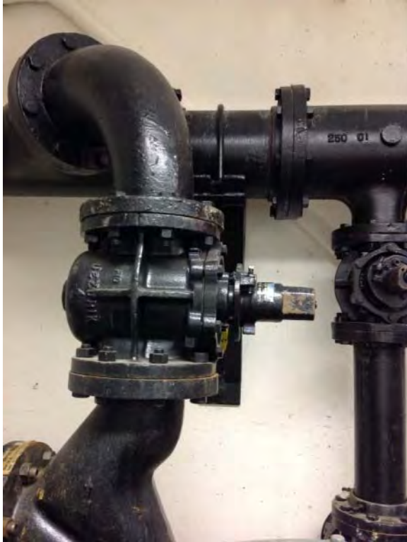
Discharge plug valve – set up to prevent debris collection in valve
