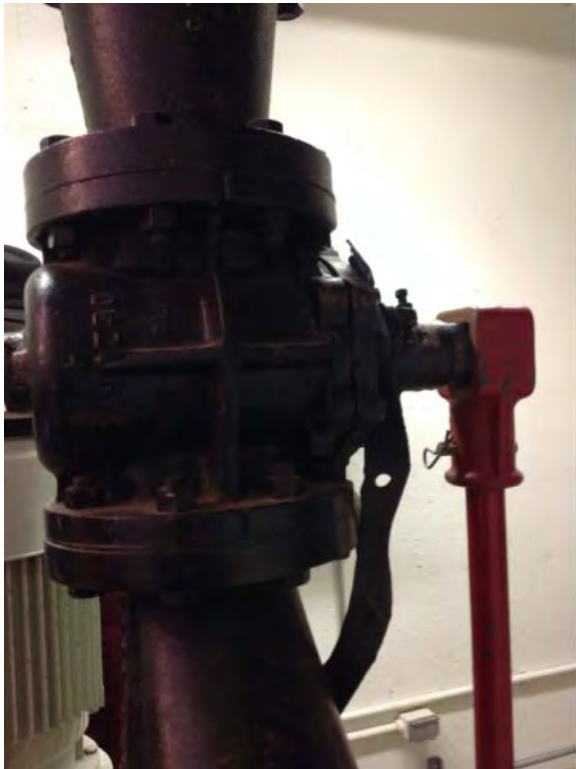
Plug valve on discharge piping
