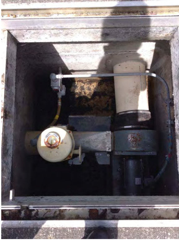
Interior of wet well blower vault, flooding evident
