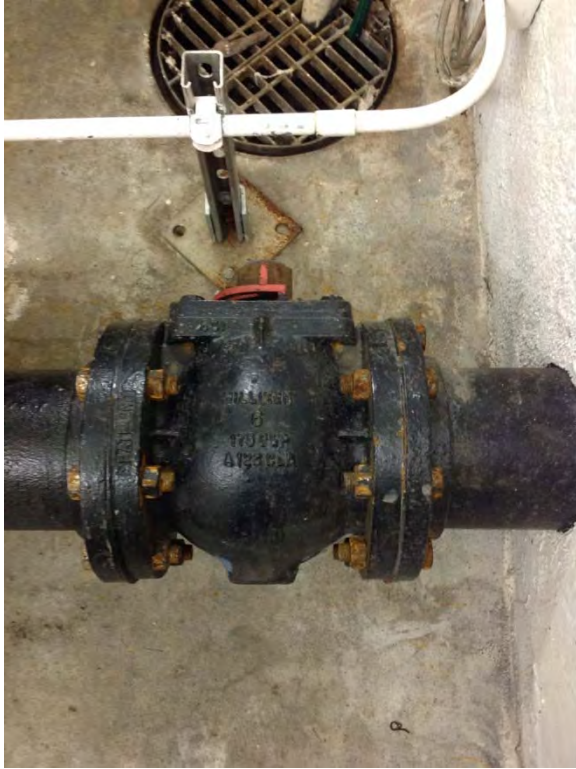
Plug valve isolation for suction piping
