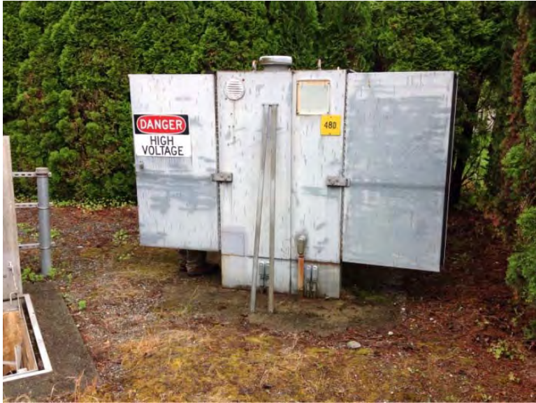
Outdoor power enclosure
