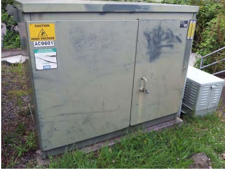
Utility service cabinet
