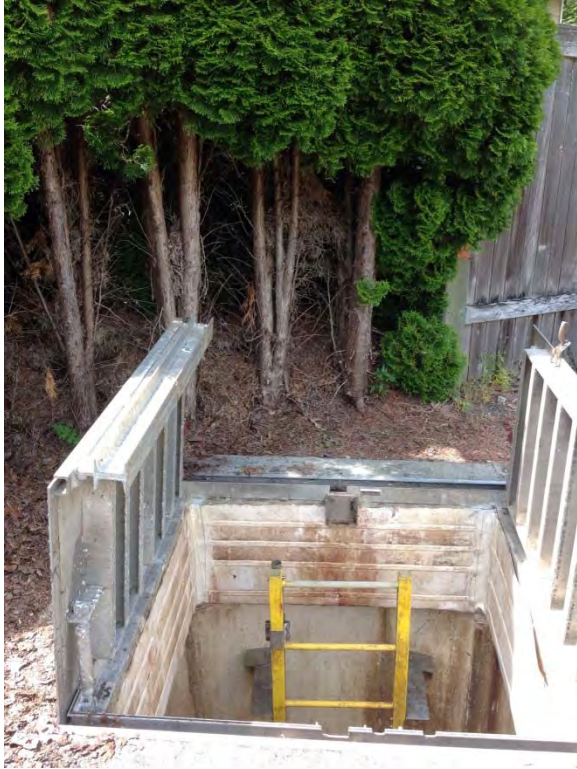
Wet well hatch and ladder
