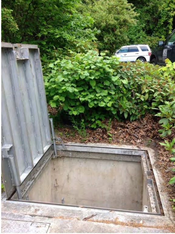
Wet well blower vault hatch
