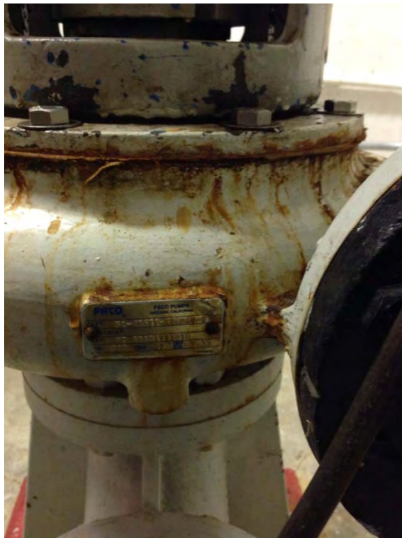
Pump 2 showing signs of aging on exterior
