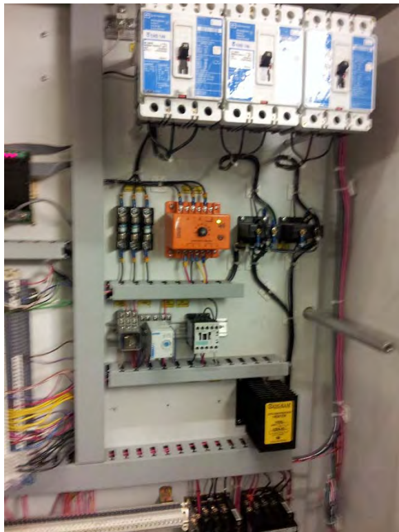
Westinghouse circuit breakers appear to be in good condition
