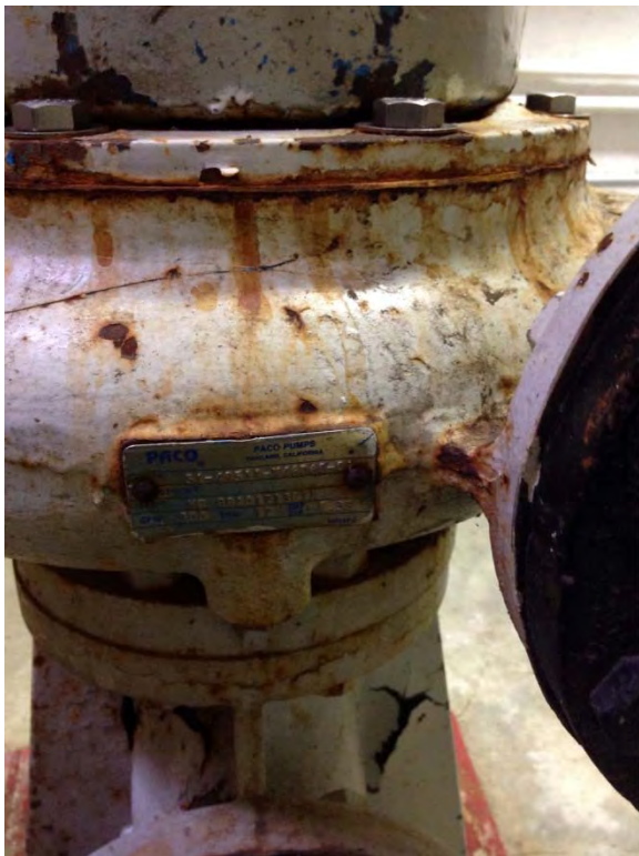
Pump 1 showing signs of aging on exterior
