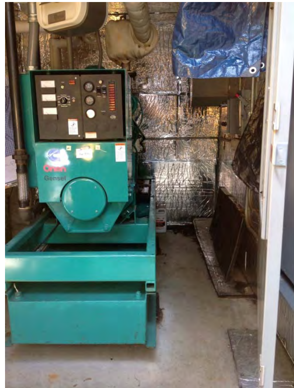
Standby generator located in dry pit/generator vault
