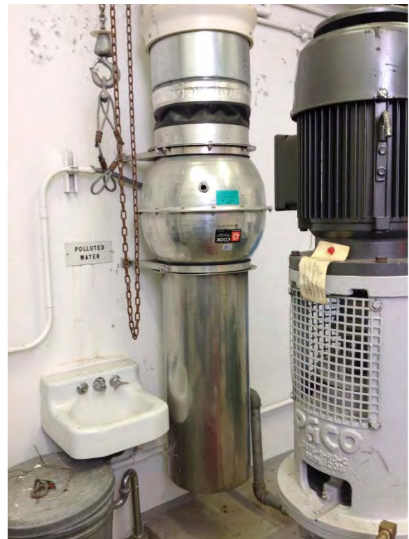
Dry Pit exhaust fan located 5' AFF in dry pit
