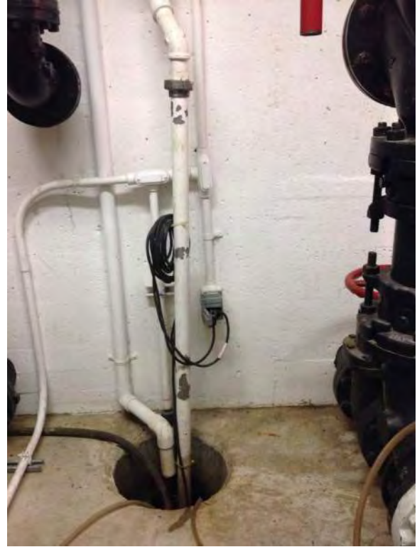
4" drain off header to wet well, near sump
