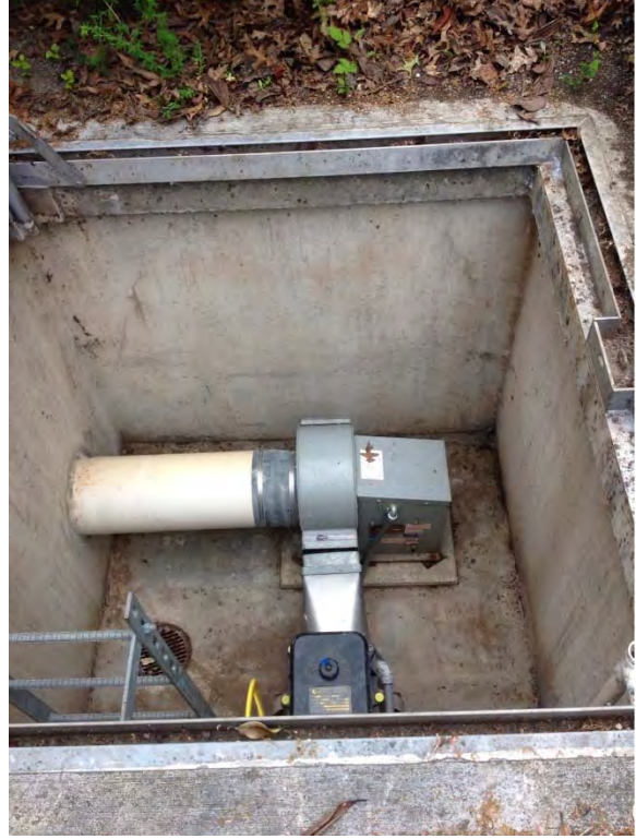
Interior of wet well blower vault
