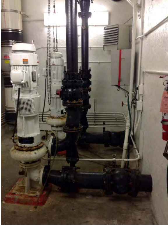
Duplex configuration, Pump 1 in foreground
