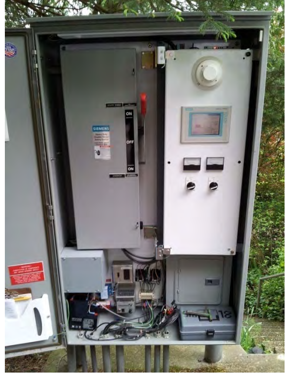
Starters located in cabinet, appears to be in good condition
