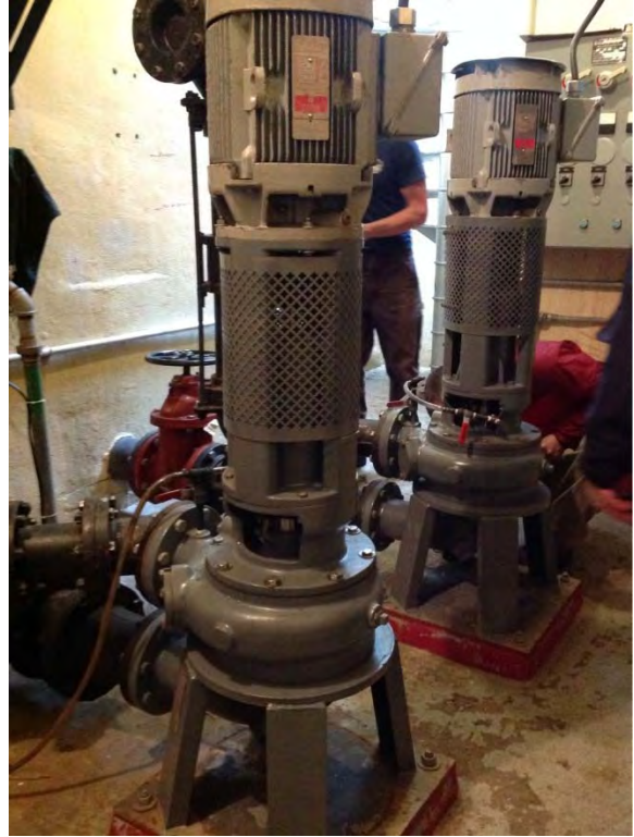
Pump and motor #2
