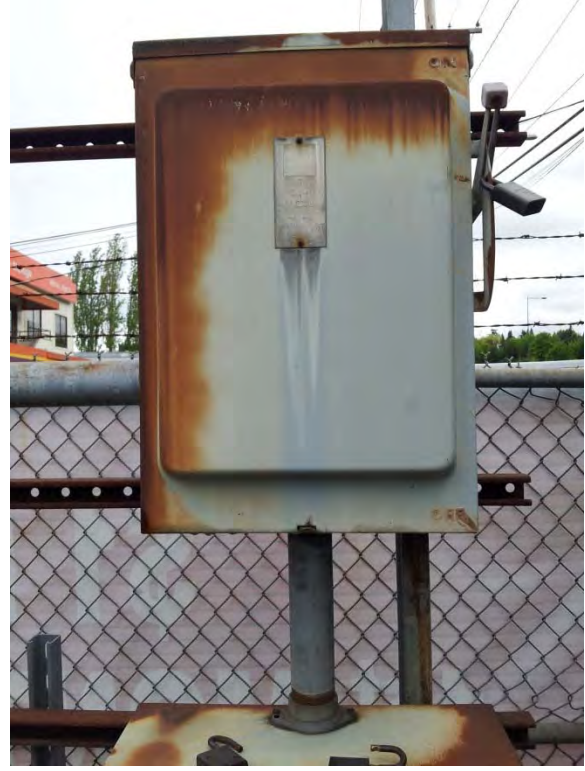
Rust on main disconnect
