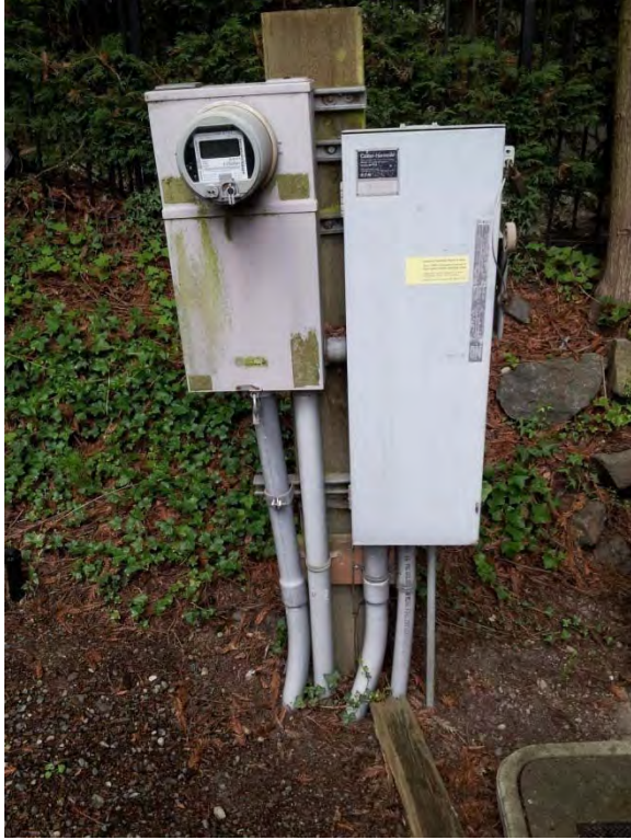
Power meter base and service entrance disconnect equipment, appears to be in good condition
