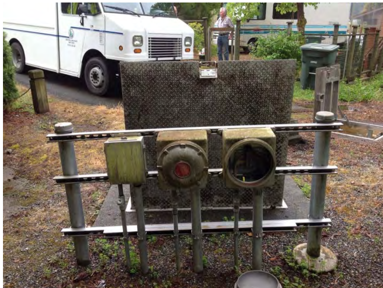
Submersible termination enclosure located in explosion proof junction box on pipe rack
