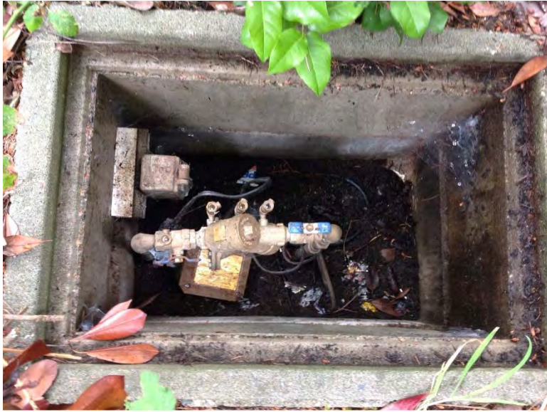
Reduced pressure backflow assembly located in below grade water meter vault adjacent to West Lake Sammamish Parkway
