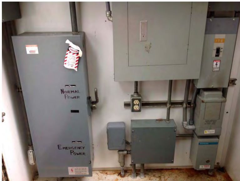
Panelboard and starters located in outdoor enclosure. Panel in good condition, Cutler Hammer starters aging
