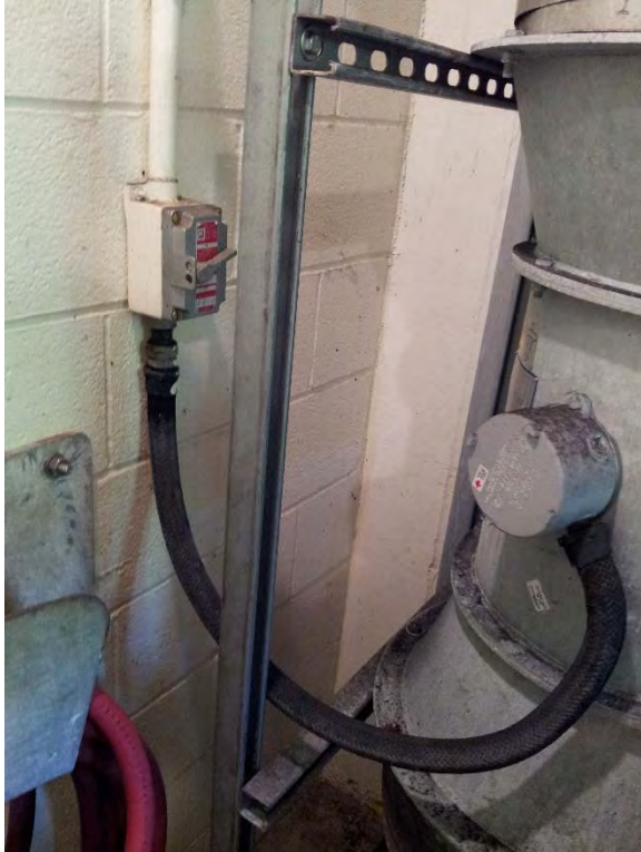
Wet well supply fan located behind exhaust fan in wet well access room
