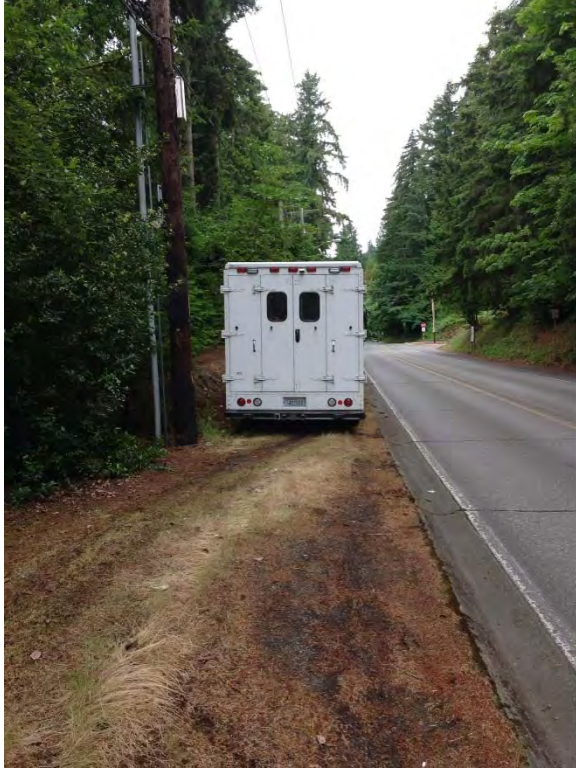
Parking along busy two way street on West lake Sammamish Parkway adjacent to main electrical equipment
