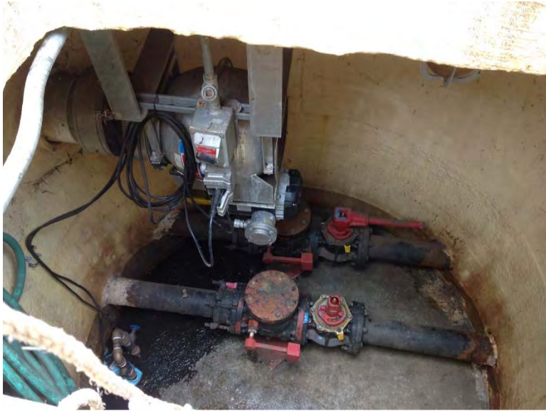
Wet well supply fan located in wet well blower and check valve/isolation valve vault
