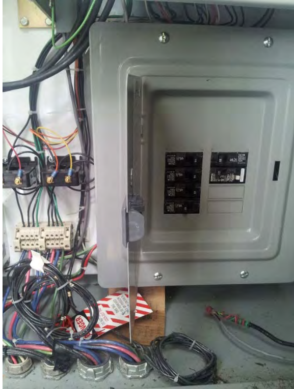
Panelboard located in outdoor power enclosure, appears to be in good condition
