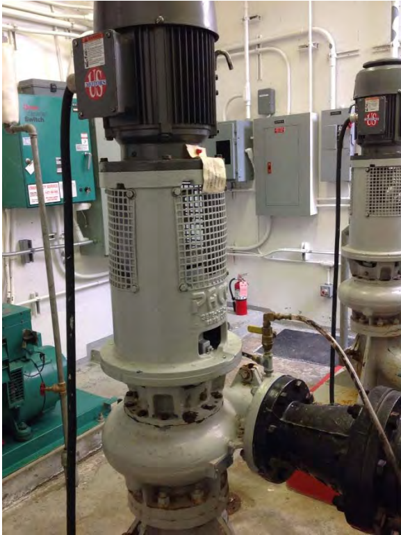
Pump and motor #2
