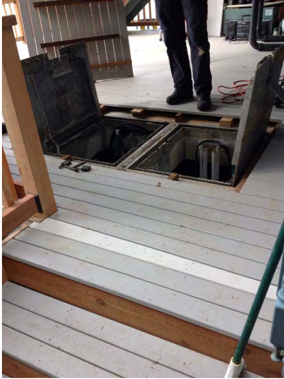
Wet well double hatch and ladder
