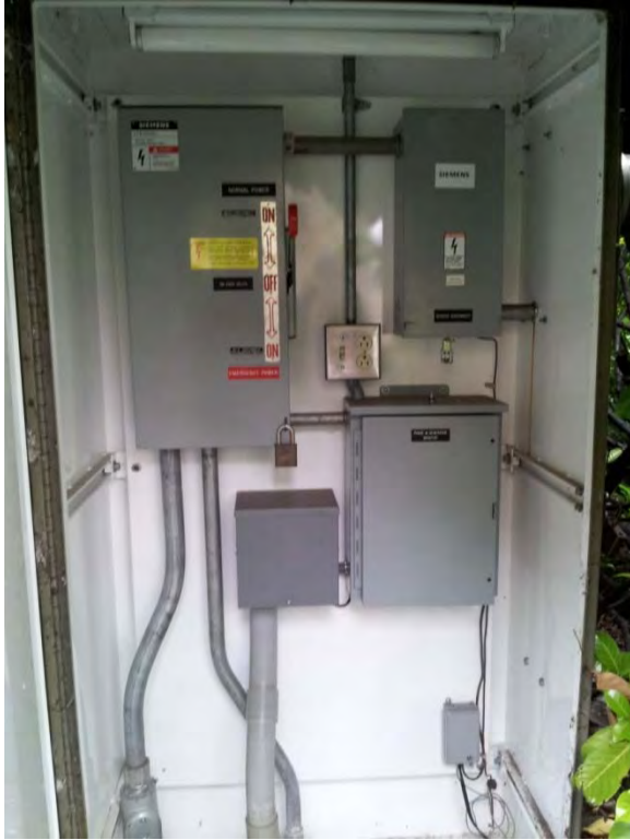
Manual transfer switch located in service cabinet
