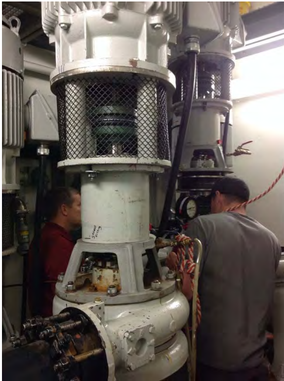
Pump and motor 1A
