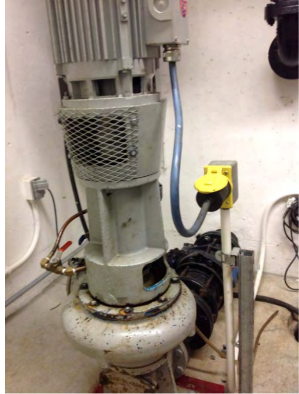
Pump and motor #2
