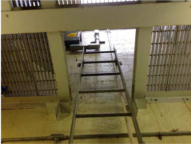
Ladder used to access pump level, somewhat challenging access for maintenance
