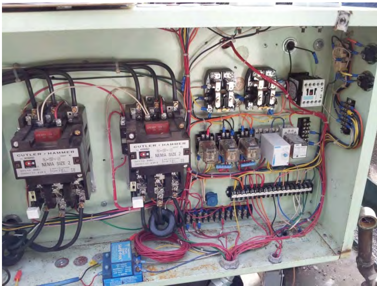
Interior of power and control panel with Cutler Hammer starters
