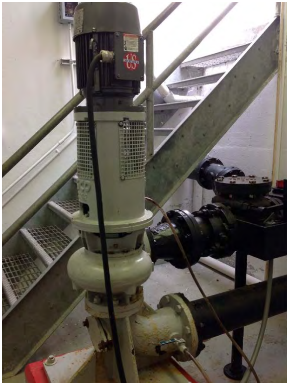
Pump and motor #1
