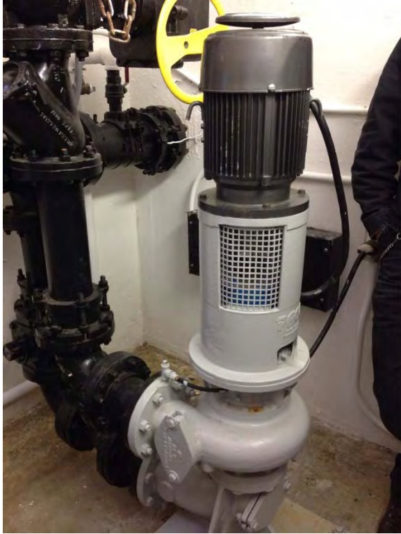
Pump and motor #1
