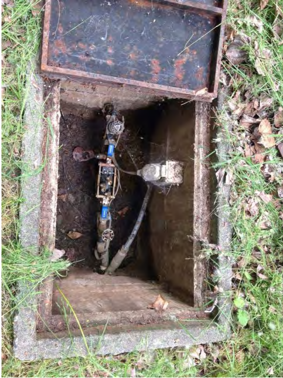
Backflow prevention assembly in below grade box
