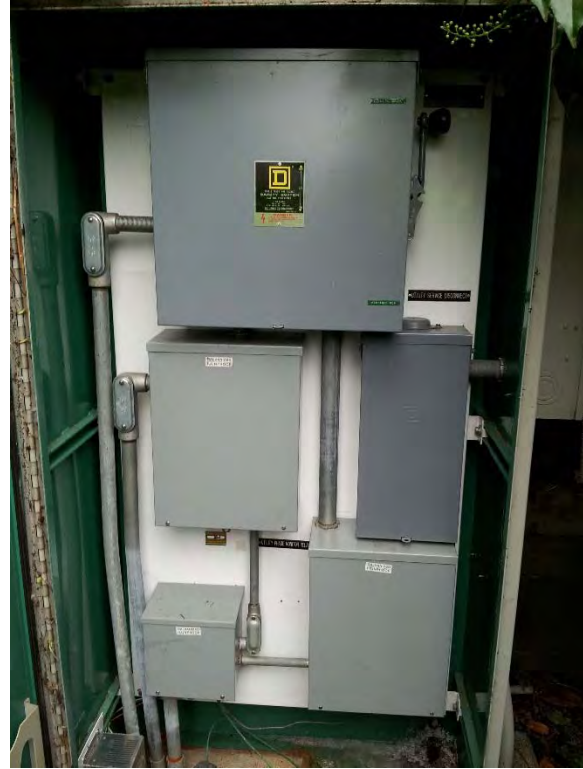
Telephone network interface located in service equipment cabinet
