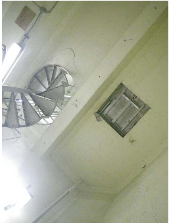
Minor concrete spall on ceiling of dry pit, should be monitored
