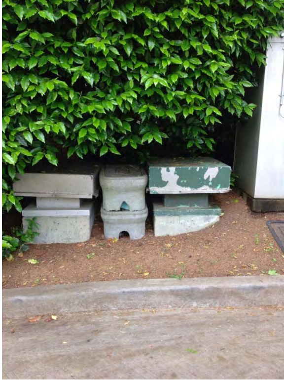
Backflow prevention assembly in two stacked water meter boxes between supply vents
