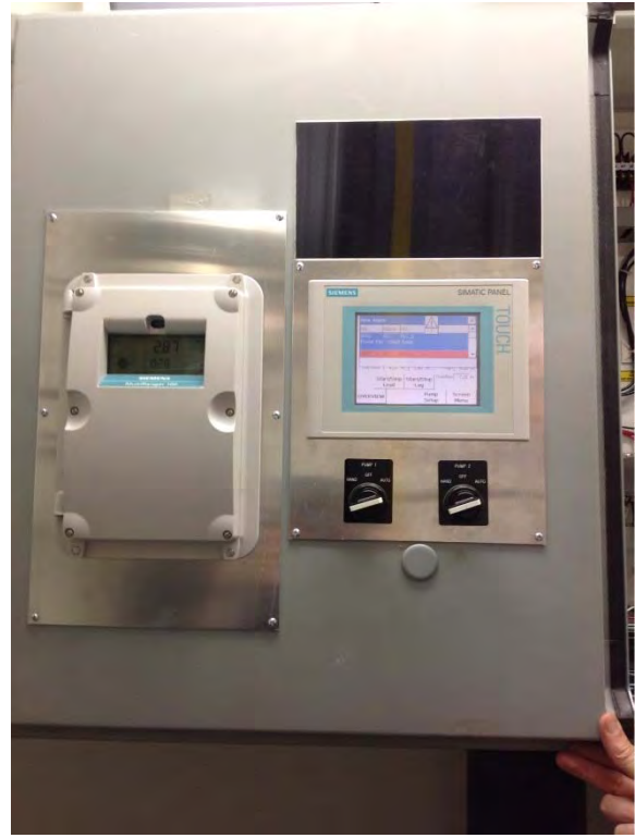
Starters located in dry pit, appears to be in good condition but aging
