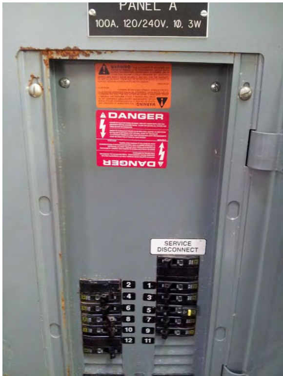
Panelboard located in dry pit, appears to be in good condition with some surface rust
