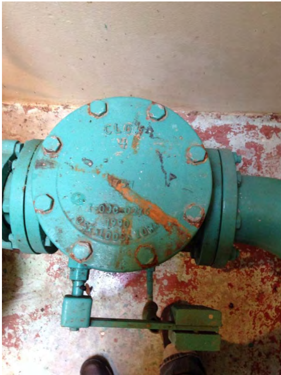
Swing check valve on discharge piping, with outside weight level and spring
