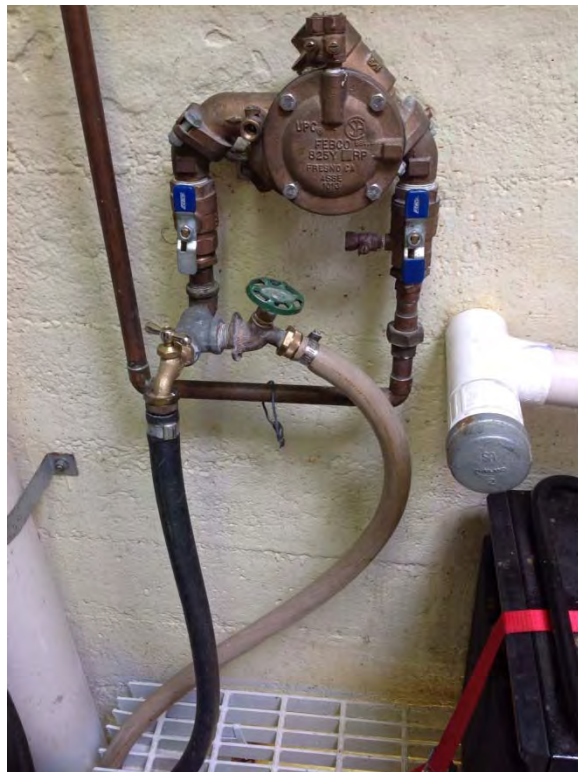
Backflow prevention assembly located in upper level of dry pit
