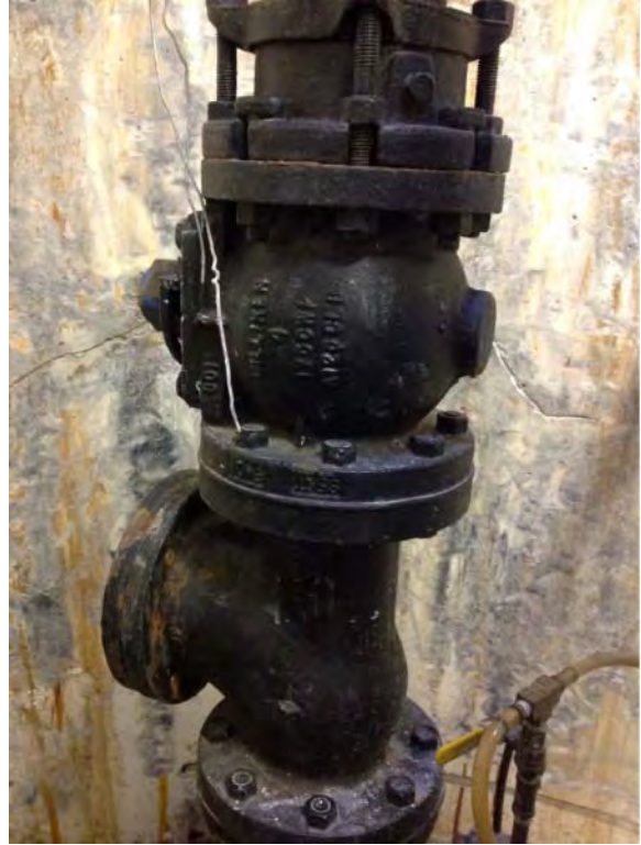
Discharge ball check valve and plug valve
