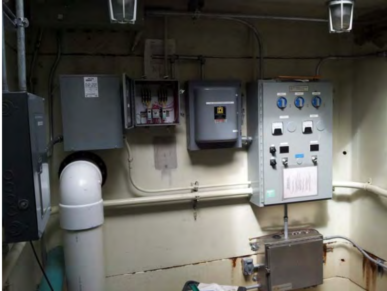
Power and control panel layout in dry pit
