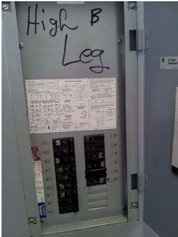
Panelboard located in dry pit
