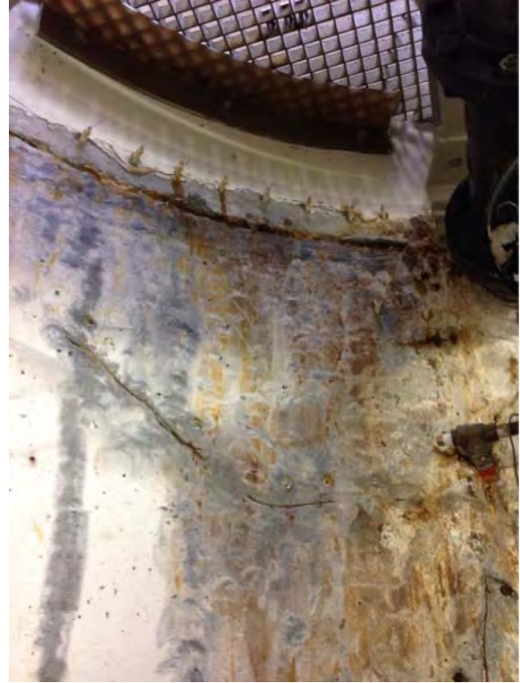
Rusting and epoxy injections on interior wall
