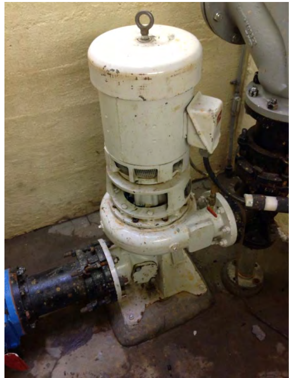
Pump and motor #1, showing signs of aging on exterior
