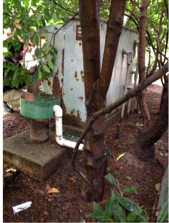
Service cabinet overgrown with bushes
