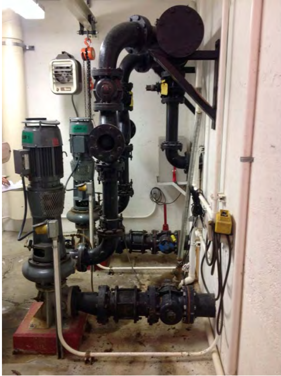
Duplex configuration (Pump 2 in background)
