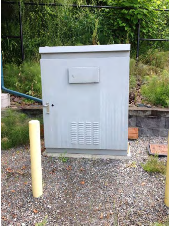
Backflow prevention assembly in above grade stainless steel enclosure
