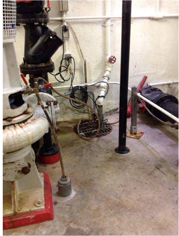
Grating on sump drain
