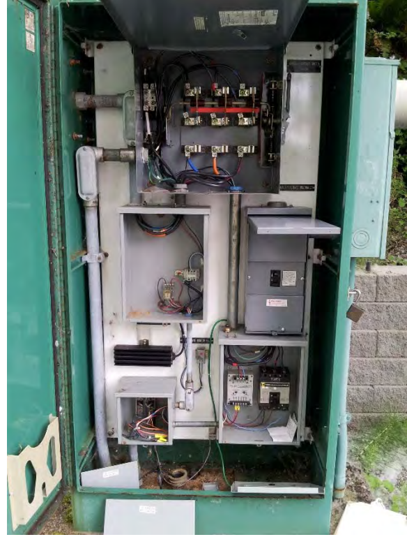
Telephone network interface in service cabinet
