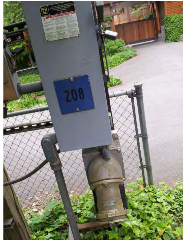
Generator receptacle located below manual transfer switch
