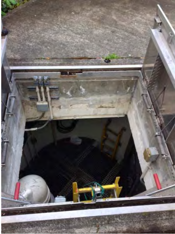
Entry to dry pit, no fall protection
