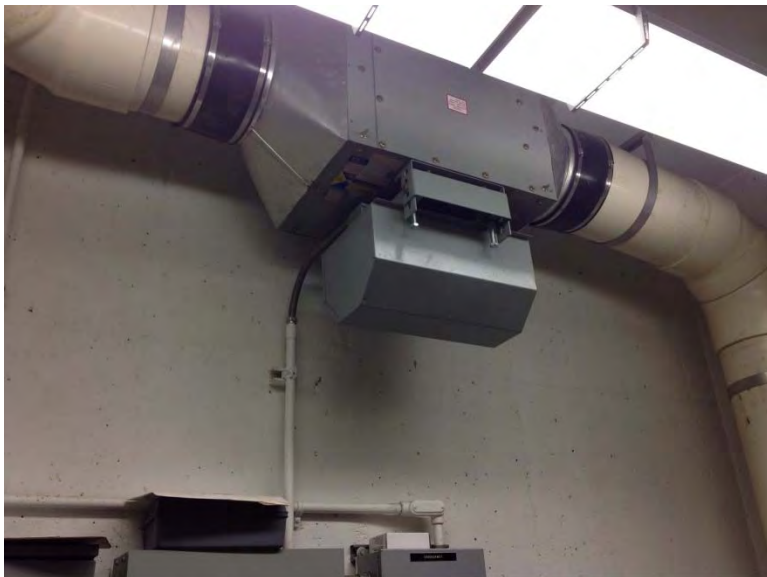
Supply fan located near ceiling of dry pit
