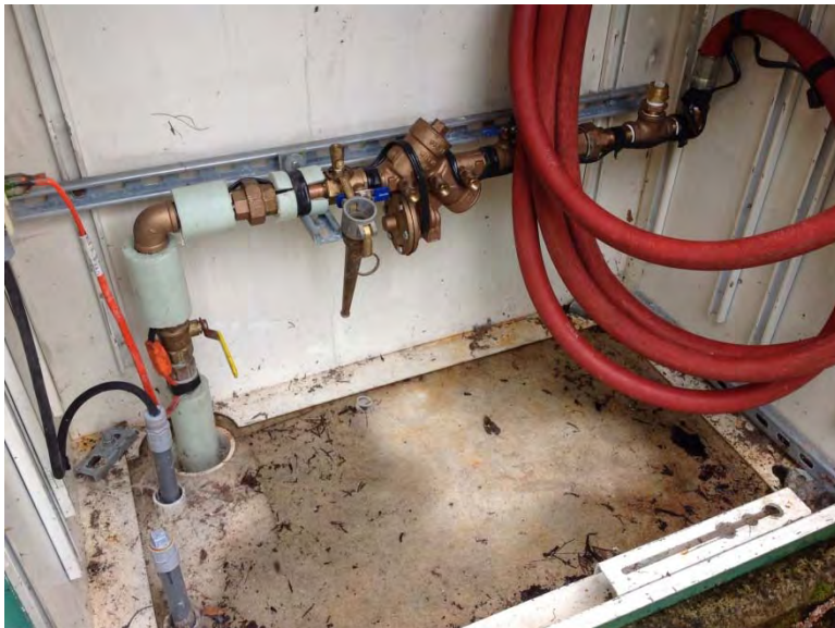
Wilkins reduced pressure backflow assembly located in enclosure with heat tape
