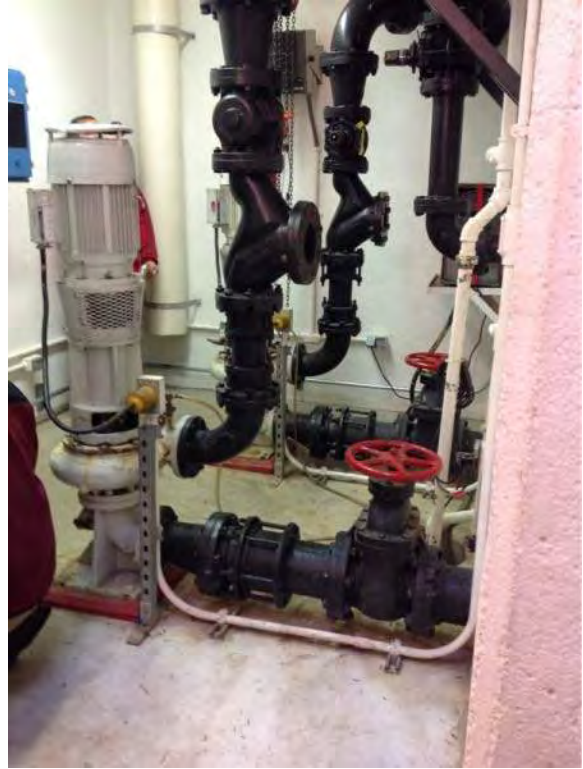
Pump and piping configuration
