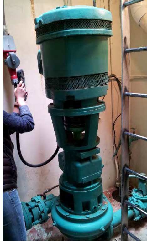
Pump and motor #1
