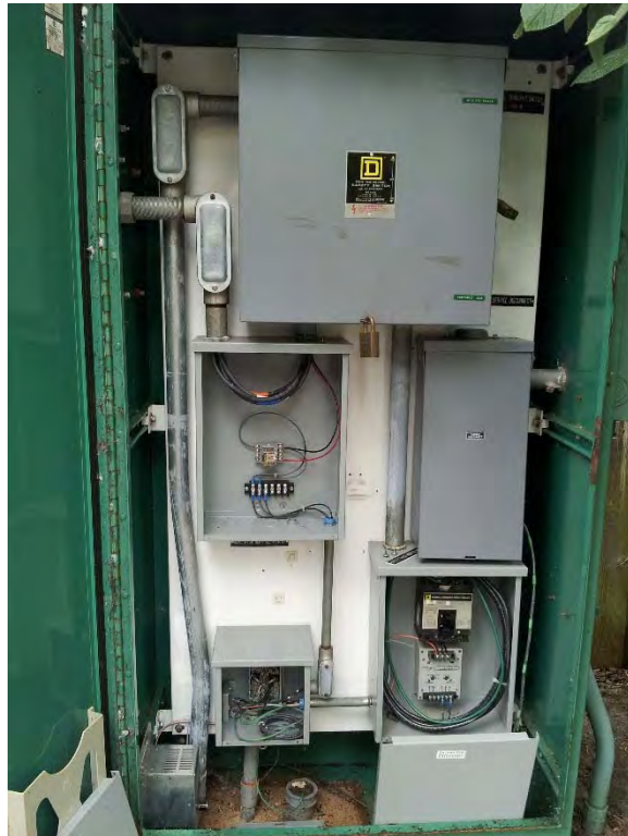
Transfer switch located in service cabinet
