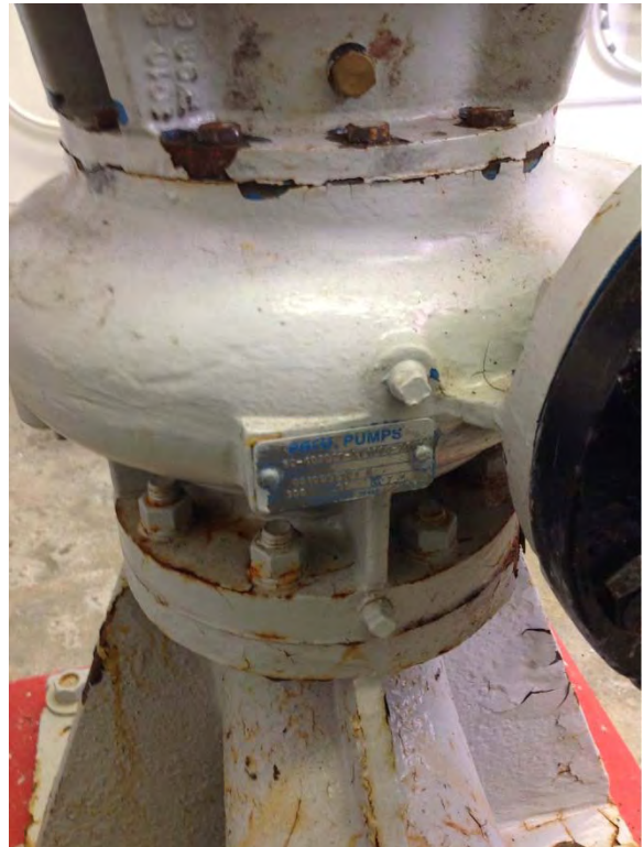
Exterior of pump #2 showing signs of aging
