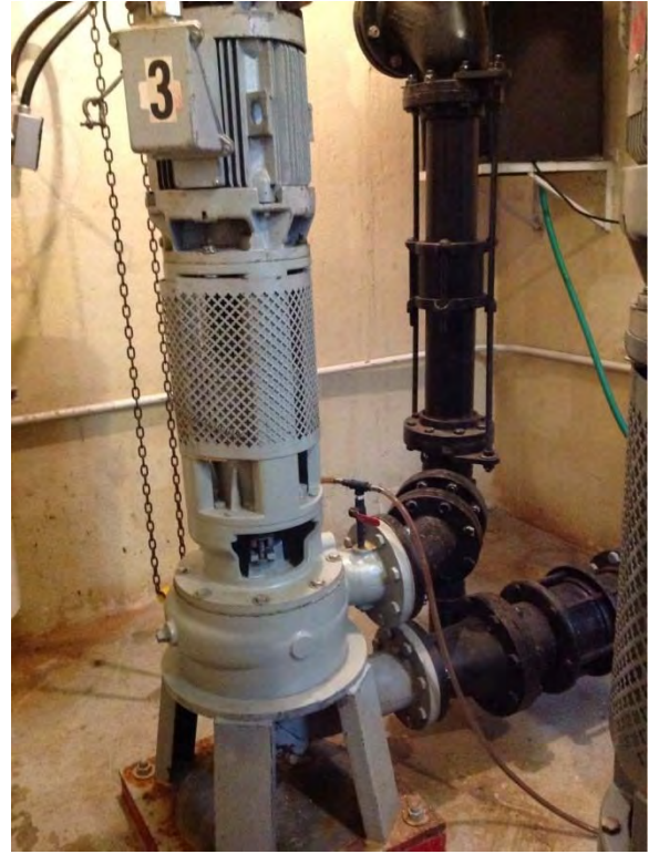
Pump and motor #3
