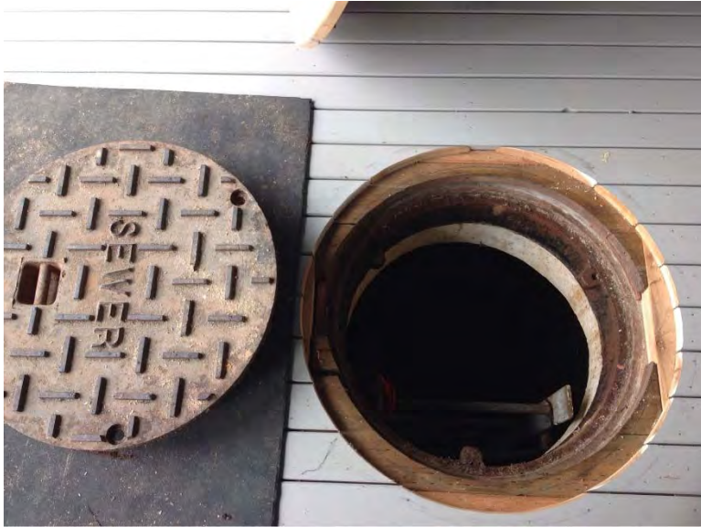
Check valve and isolation valve vault with manhole lid and ladder
