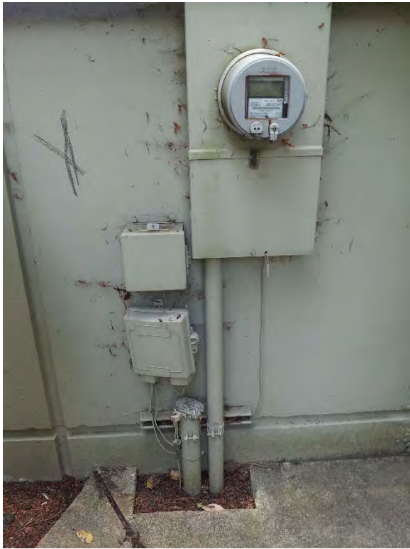
Service meter located outside west wall of control building
