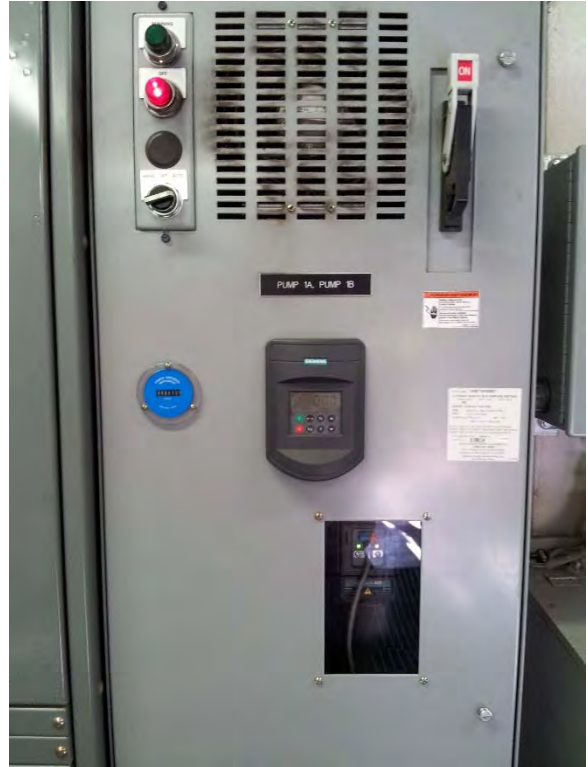
Starters for Pump 1A and 1B, appears to be in good condition but aging
