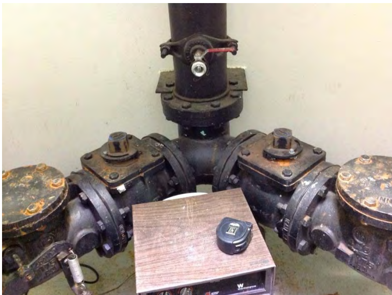
Plug valve and swing check valve with outside weight and lever located on discharge piping, plug valve vertical installation – not ideal
