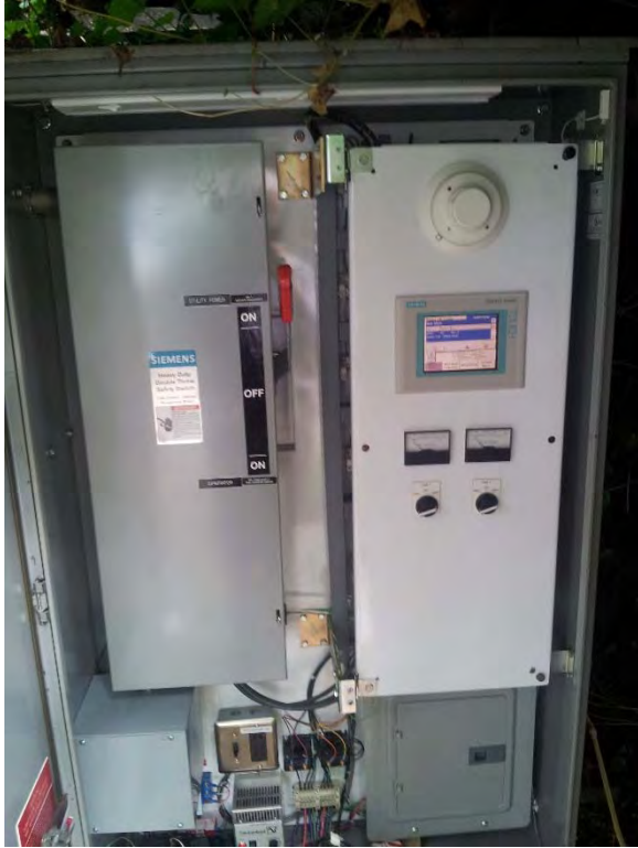
Telemetry control panel with operator interface located in outdoor power enclosure, appears to be in good condition
