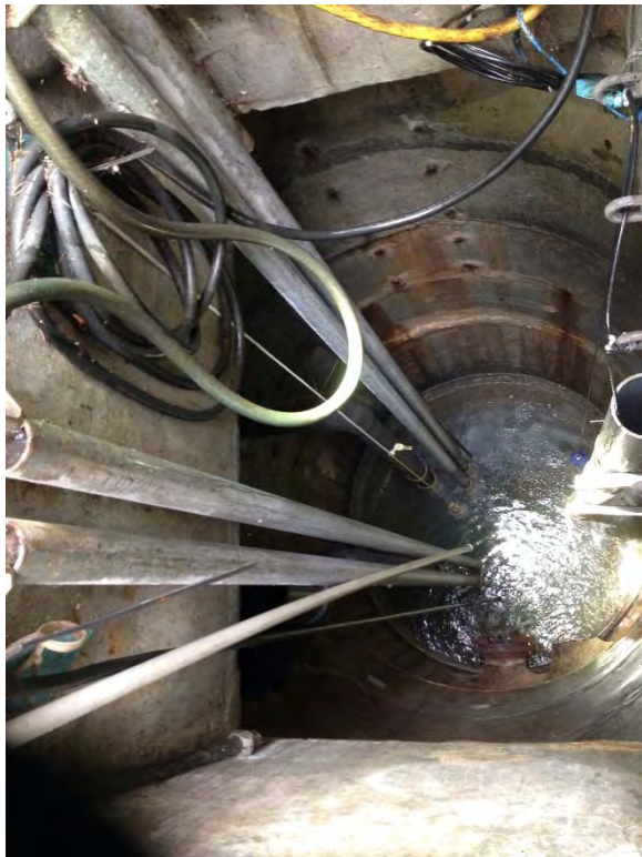
Some lower level corrosion and exposed aggregate on the lower 1'-2' of well
