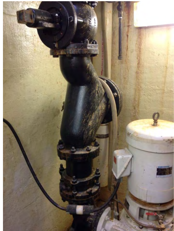
Plug valve on discharge piping, seat end is down toward pump, better for sealing flow but can accumulate debris behind plug and stop valve from working
