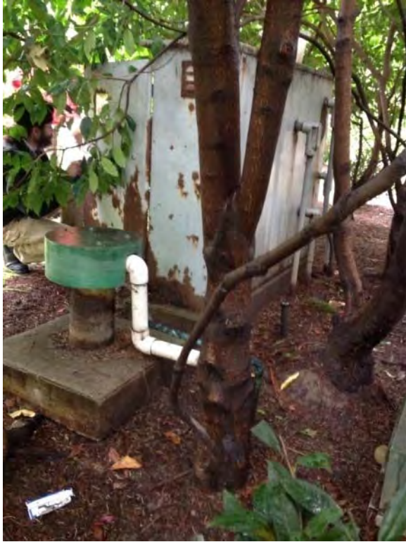
Wet well vent approximately 18" from service cabinet
