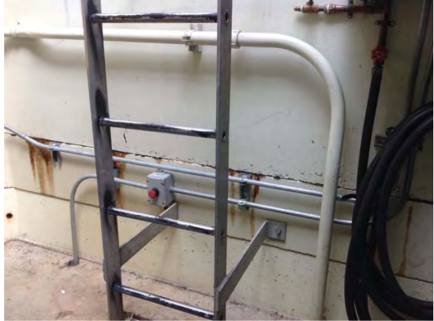
Some rusting near bottom of first floor seam
