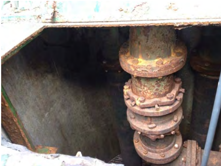
Significant rust on discharge piping
