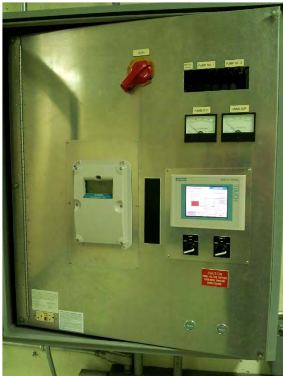
Telemetry control panel with operator interface located in control building
