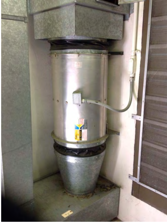
Dry pit supply fan located in corner of control building 4' AFF
