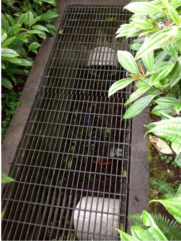
Backflow prevention assembly in underground air intake vault
