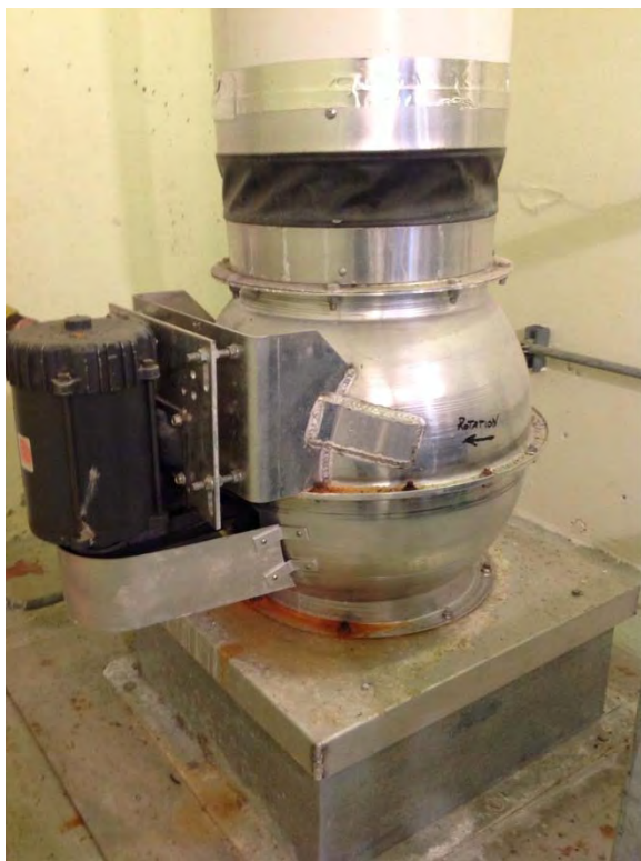
Wet well exhaust fan located in raised area in wet well access room
