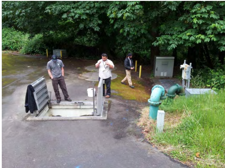
General site layout, more moss growth on asphalt concrete and a lot of vegetation maintained by others
