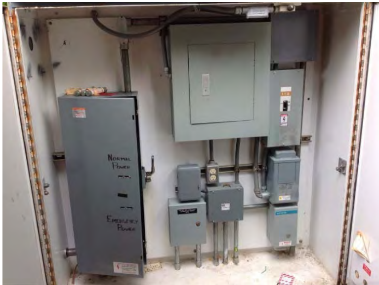
Manual transfer switch located in outdoor power enclosure
