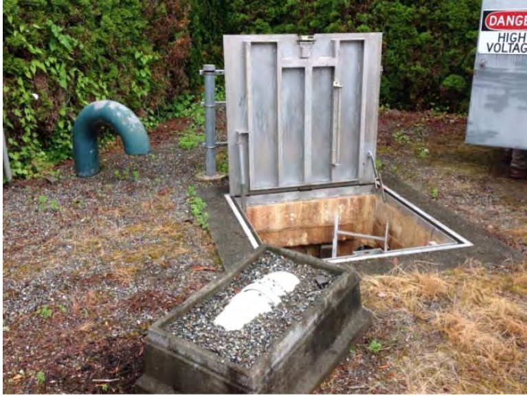
Wet well access hatch and ladder
