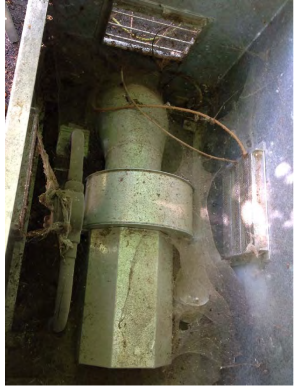
Wet well exhaust fan located in above grade enclosure
