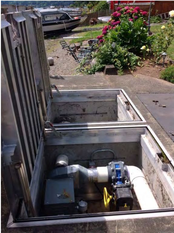
Wet well blower vault and air intake vault in deck area
