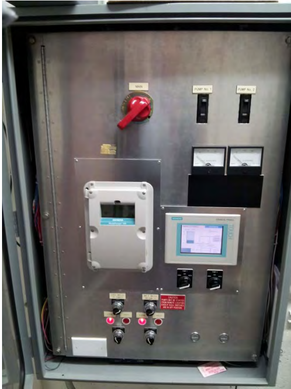
Starter/control panel with operator interface
