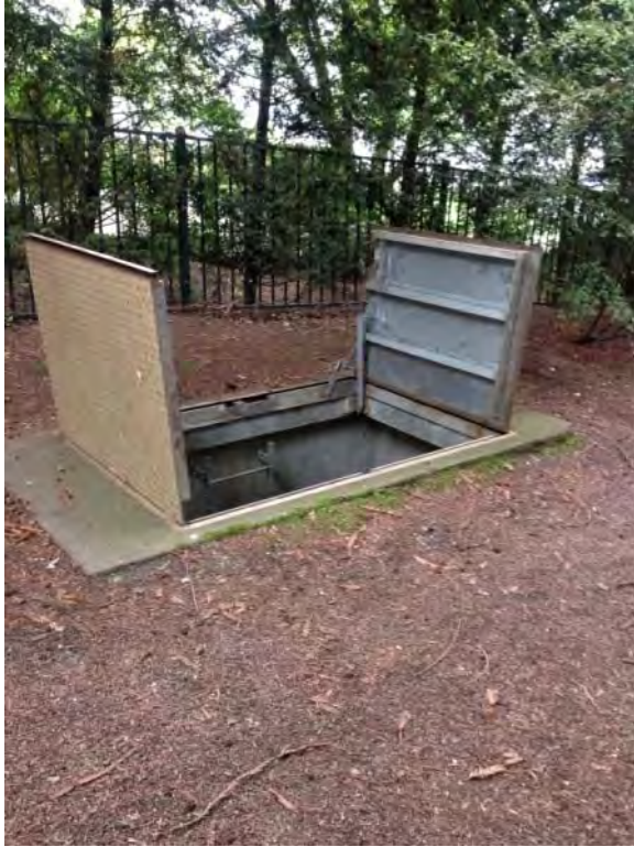
No fall protection for blower vault
