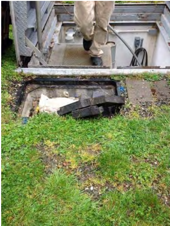
Backflow preventer assembly adjacent to dry pit
