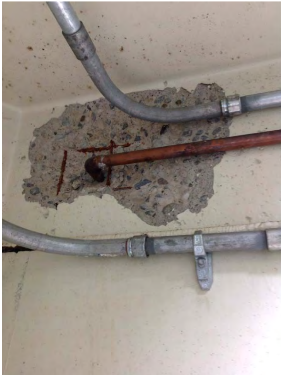
Concrete spalled in top corner – reinforcing exposed and rusted
