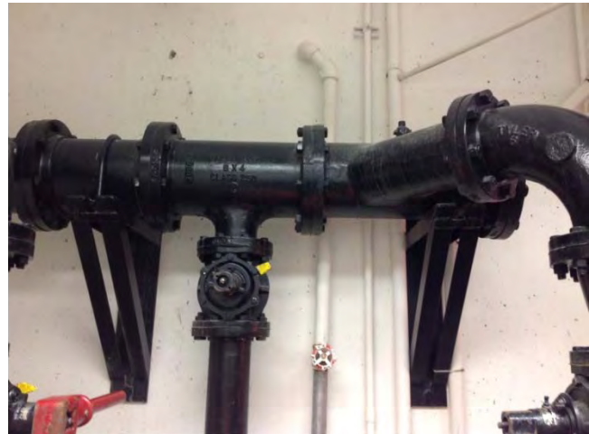
Common discharge piping
