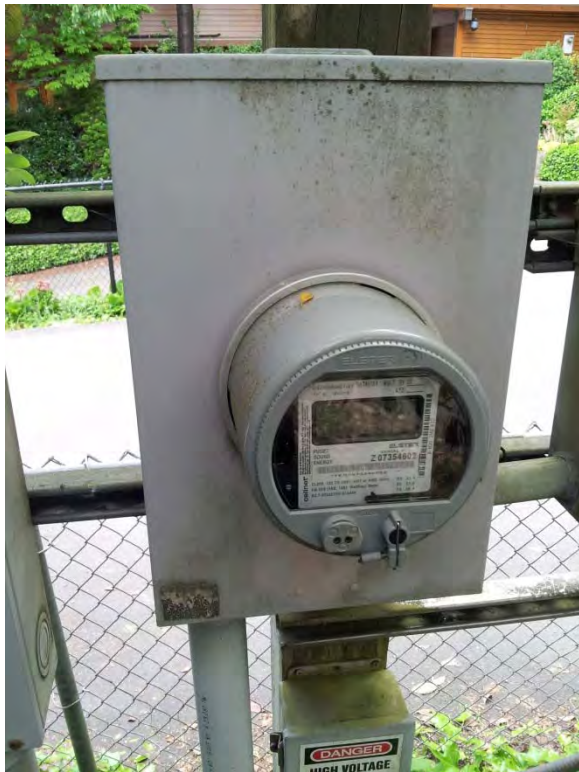
Utility service meter
