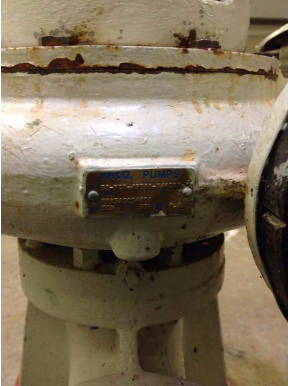
Pump 1 showing signs of aging on exterior
