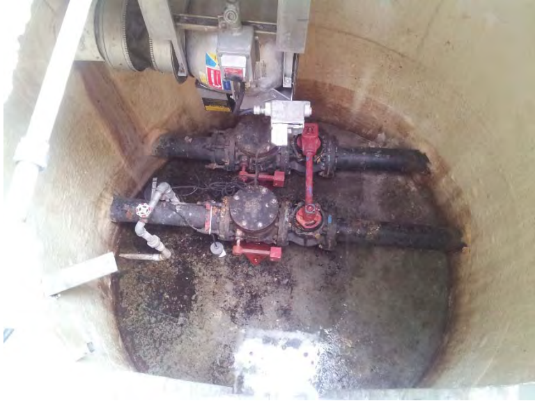
Wet well blower vault located in adjacent underground vault
