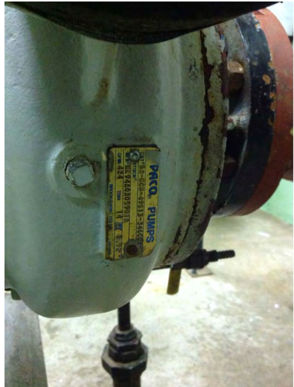
Pump 2 showing signs of aging on exterior
