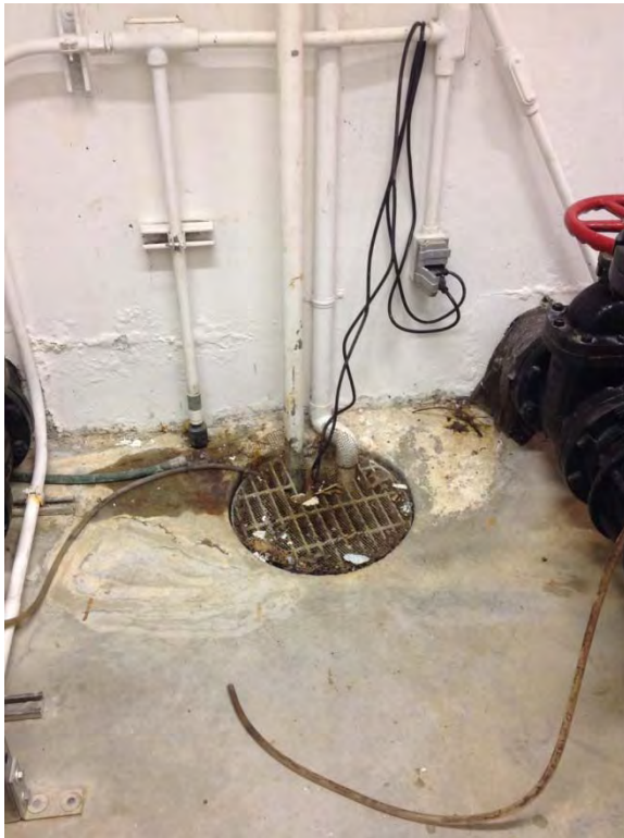
Metal grating and wire mesh on sump, no hazard for stepping into sump
