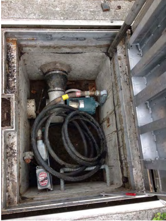
Interior of wet well blower vault, appears to be in good condition.
