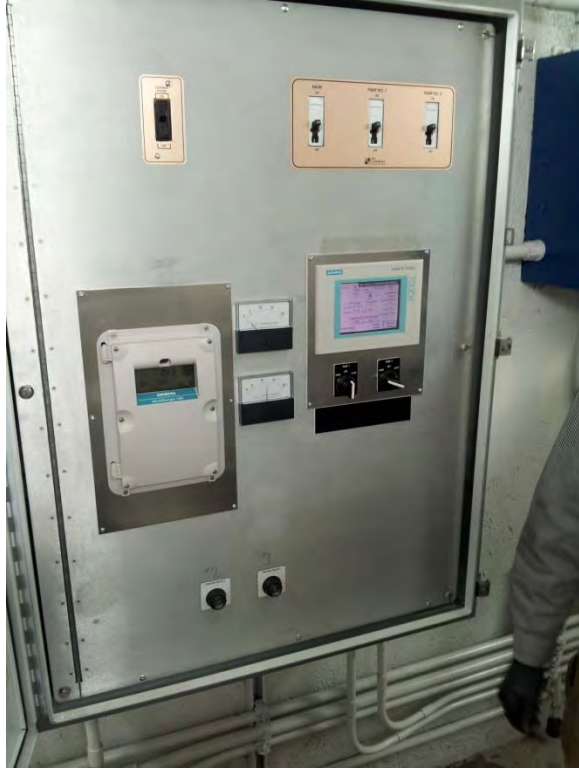
Telemetry control panel located in dry pit, appears to be in good condition
