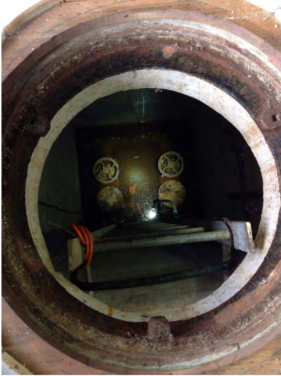
Gate Valve with hand wheel for isolation and swing check valve with outside weight and lever located in check valve and isolation valve vault, submerged in water upon site visit
