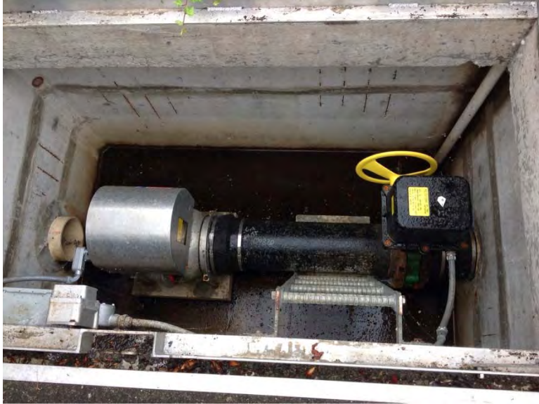
Interior of wet well blower vault, vault is damp but appears to be in good condition
