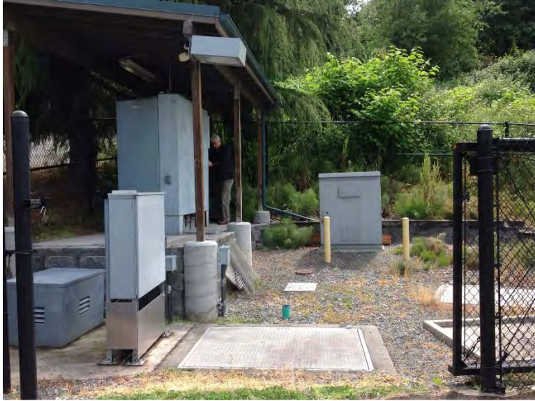
Timber shed with metal roof on platform providing cover for power and control equipment
