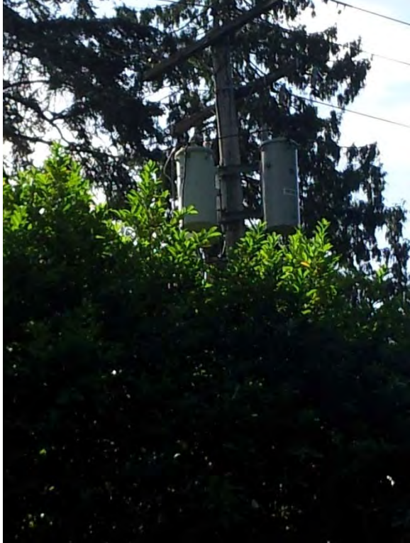
Utility transformer overhead adjacent to station
