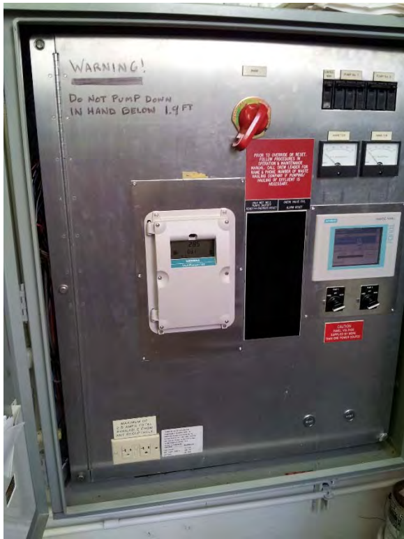
Telemetry control panel with operator interface
