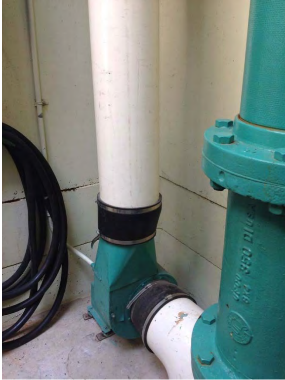
Exhaust fan located on first floor in dry pit
