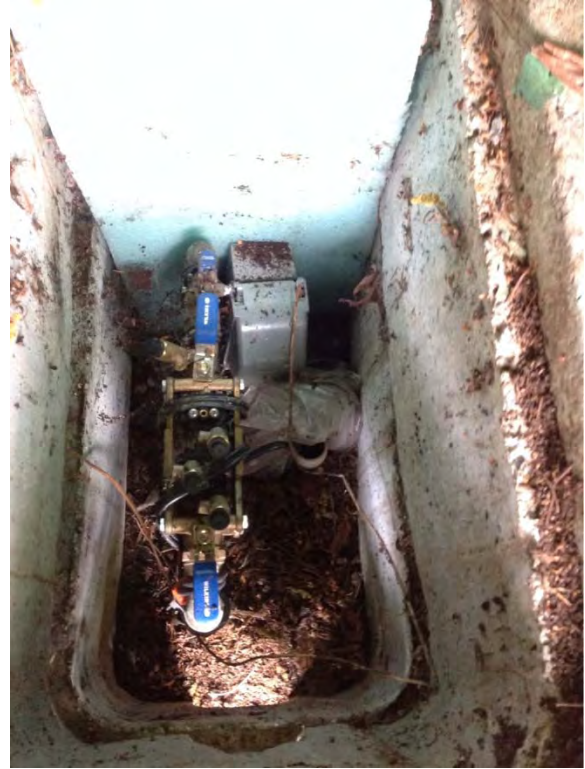
Backflow prevention assembly above grade
