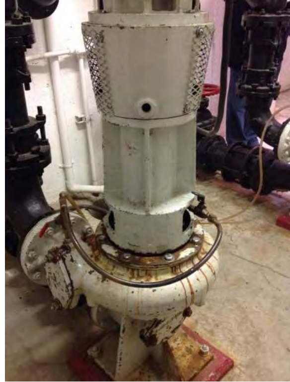
Pump and motor #2
