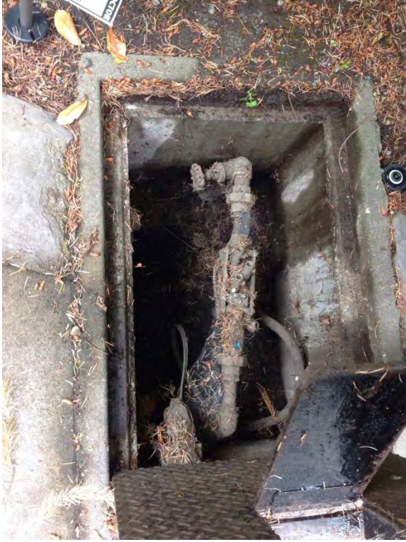
Backflow prevention assembly in below grade box
