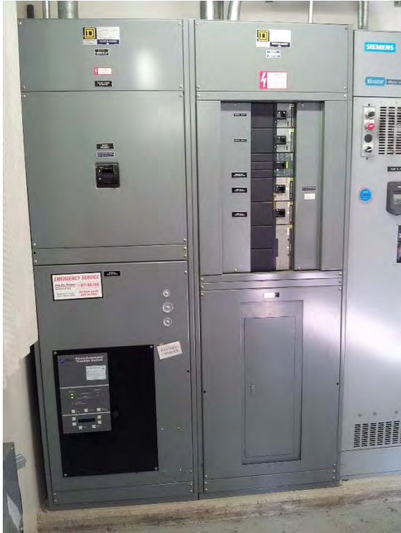
Panelboard located on top floor of control building
