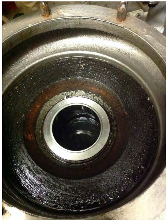
Interior of Pump 2B volute with pitting and grooves
