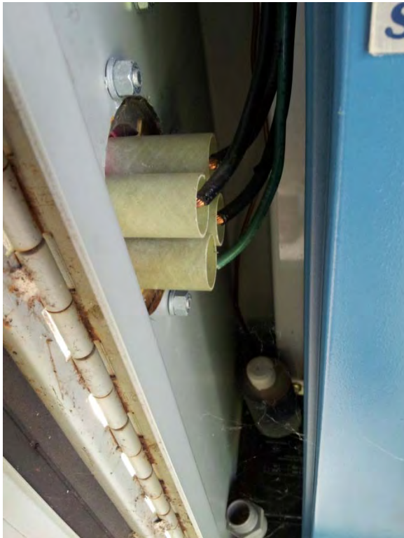
Generator receptacle needs to be mounted for clearance of conductors
