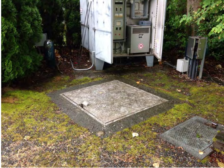
Outdoor power enclosure
