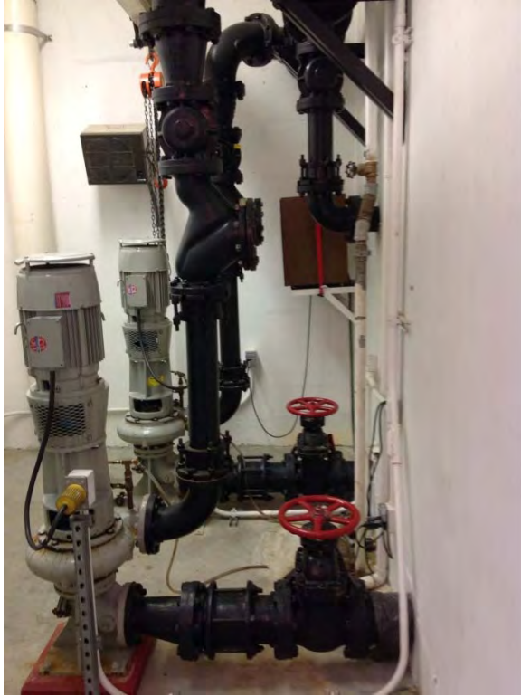
Duplex configuration, Pump 1 in foreground
