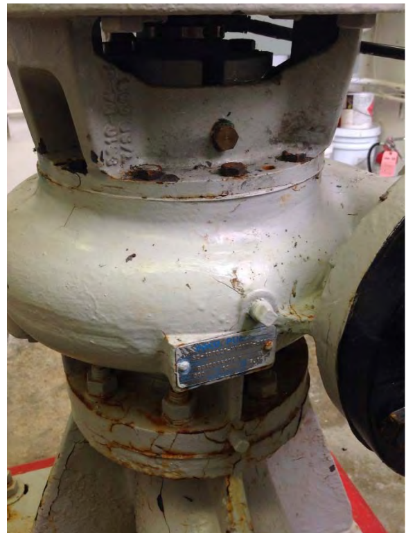
Exterior of pump #1 showing signs of aging
