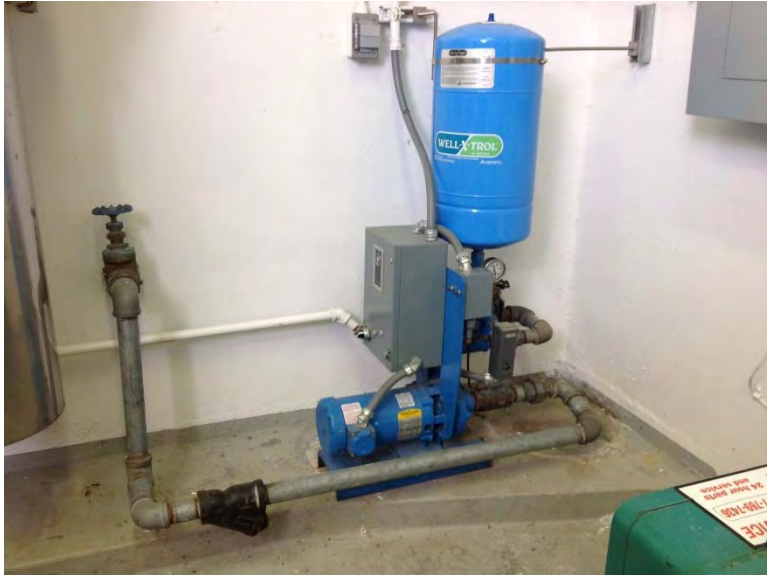
Washdown water supplied from lake using pressure tank system located in corner of dry pit
