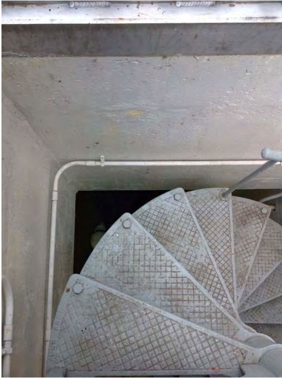
Gap between spiral staircase and wall, no rail on staircase by gap
