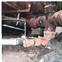
This is an example of older cast iron pipe in good shape
