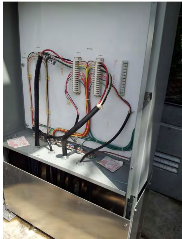
Submersible cable termination enclosure adjacent to wet well in above grade enclosure, fairly new appears to be in good condition
