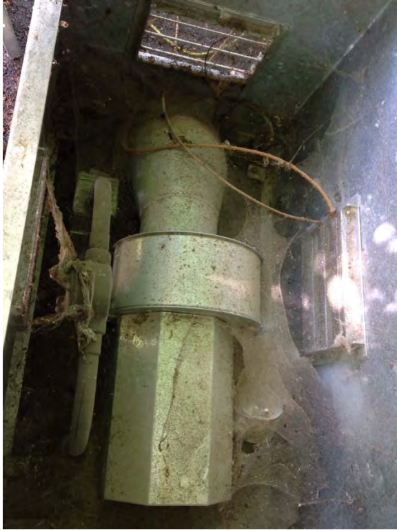
Interior of above grade exhaust fan vents, a lot of cobwebs, some branches inside
