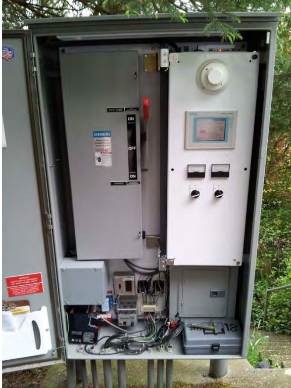
Telemetry control panel with operator interface
