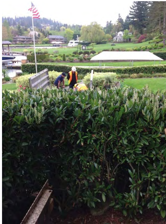
Overall hatch to wet well and dry pit located in yard
