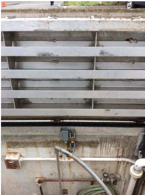
Dry pit hatch, fatiguing evident
