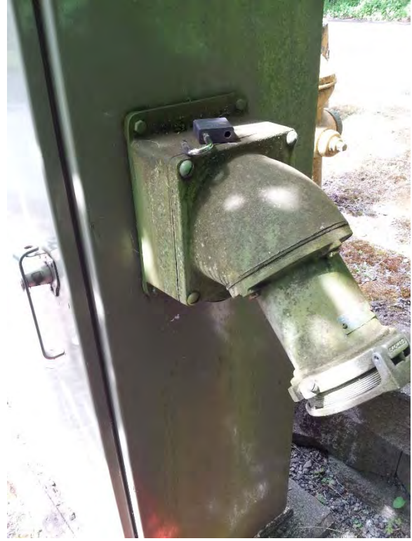
Generator receptacle located on outdoor power cabinet
