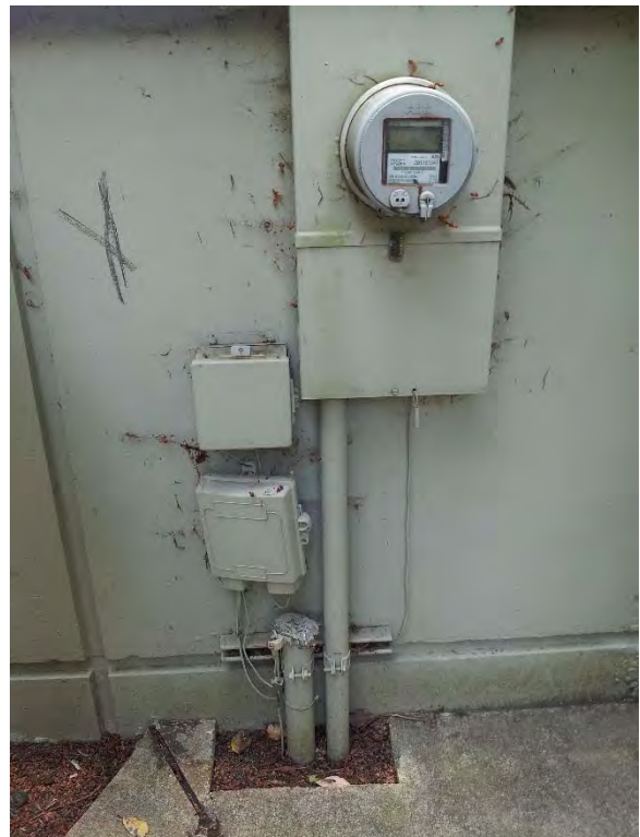
Telephone network interface located outdoor on west wall
