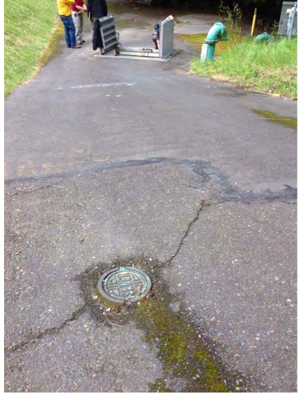
Isolation valve in access road approximately 20 feet from station
