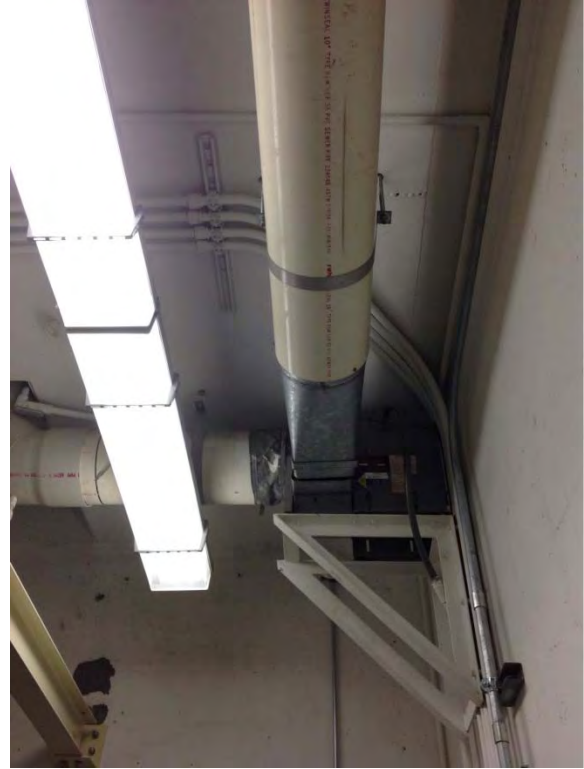
Supply fan located near ceiling of dry pit
