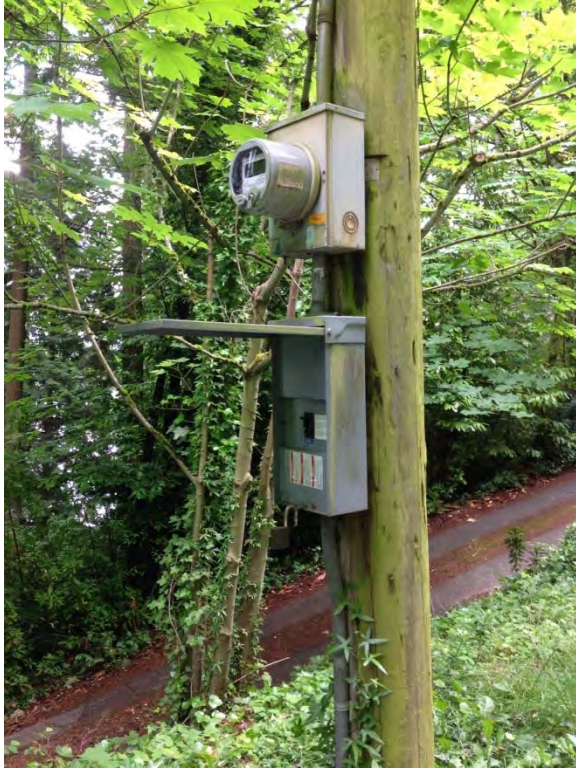
Service meter located on pole along West Lake Sammamish Parkway
