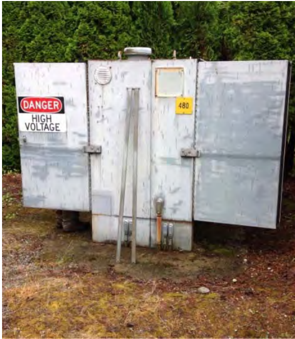
Outdoor power enclosure
