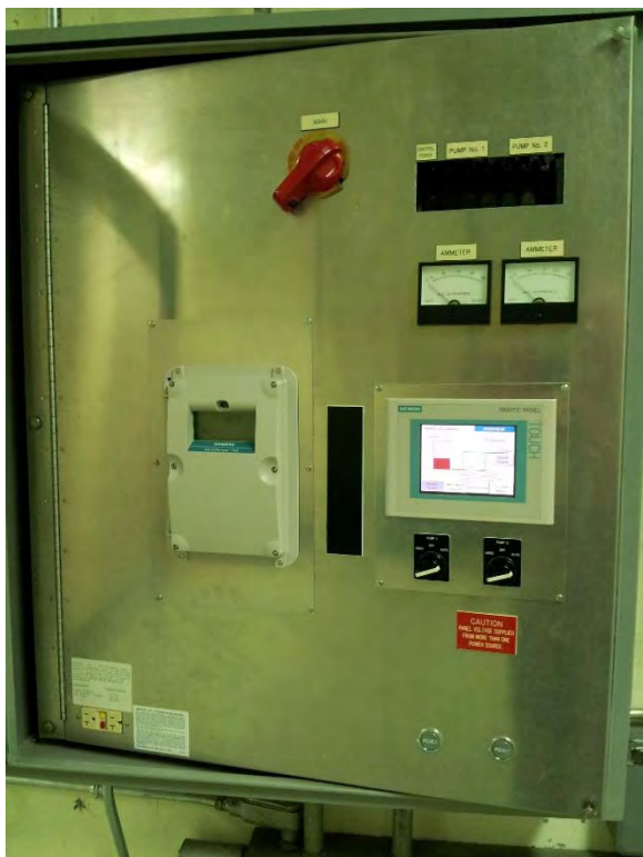
Starters located in control building
