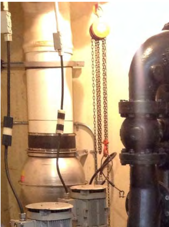
Supply fan located in corner of dry pit
