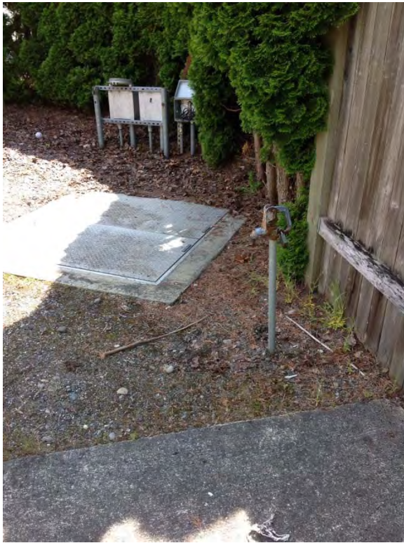
Freeze-less yard hydrant near wet well
