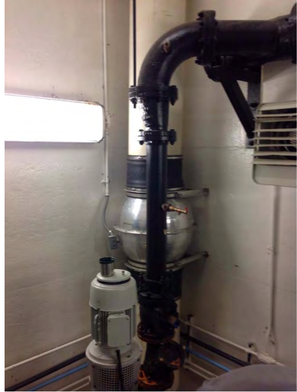
Supply fan located 5 feet AFF in dry pit
