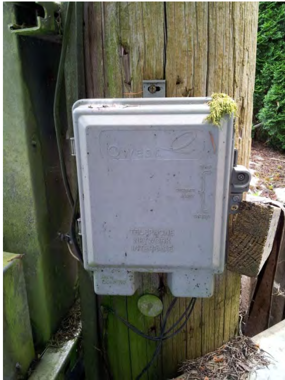
Telephone network interface located in outdoor junction box
