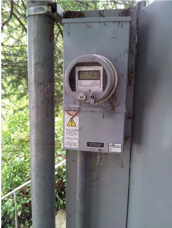
Utility meter base
