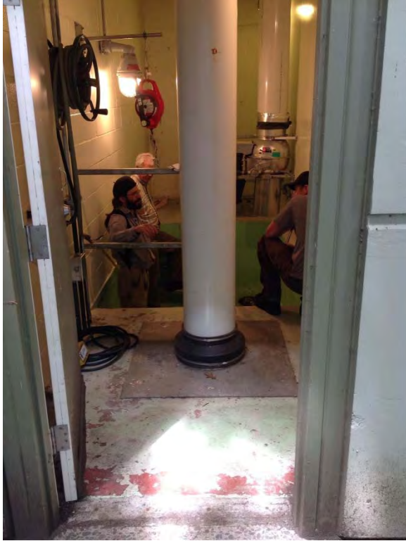
Wet well accessed through separate door adjacent to control building
