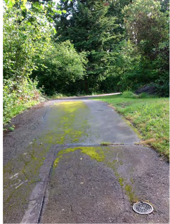
Moss growth on asphalt concrete
