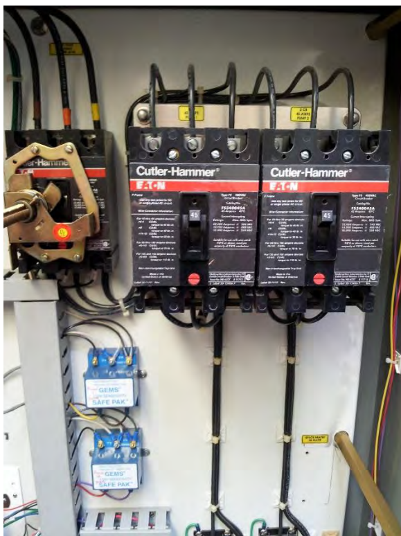
Cutler Hammer starters located in telemetry control panel
