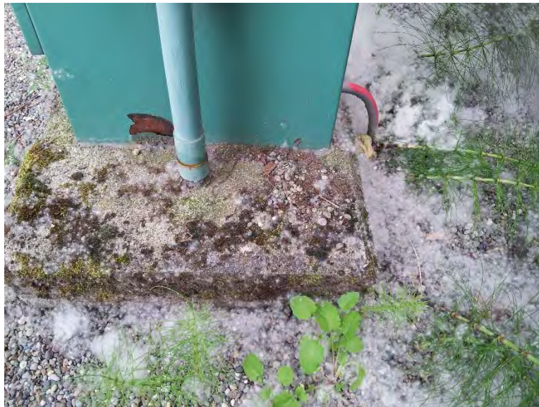
Some paint chipping/rusting near bottom of service cabinet
