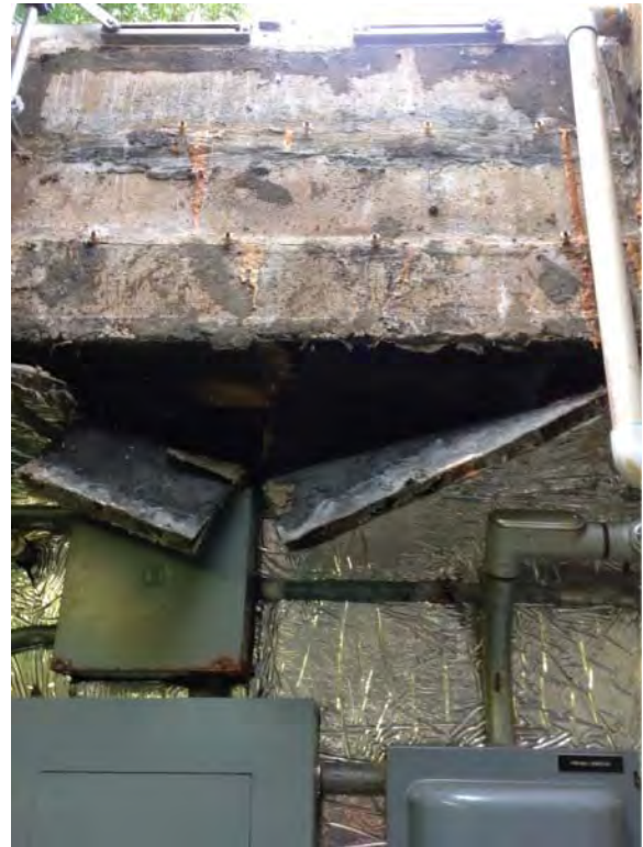
Insulation in generator vault falling off
