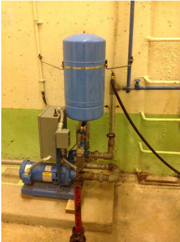
Washdown water supply from lake using pressure tank system
