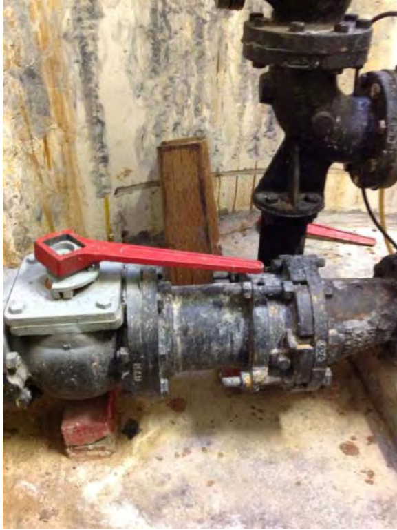
Suction plug valve, vertical shaft orientation – not desirable
