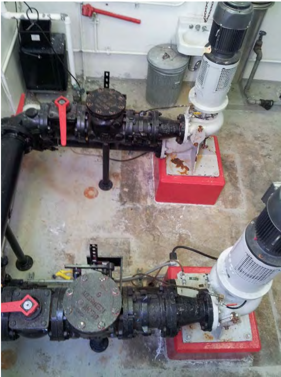
Duplex configuration, pump #1 in foreground
