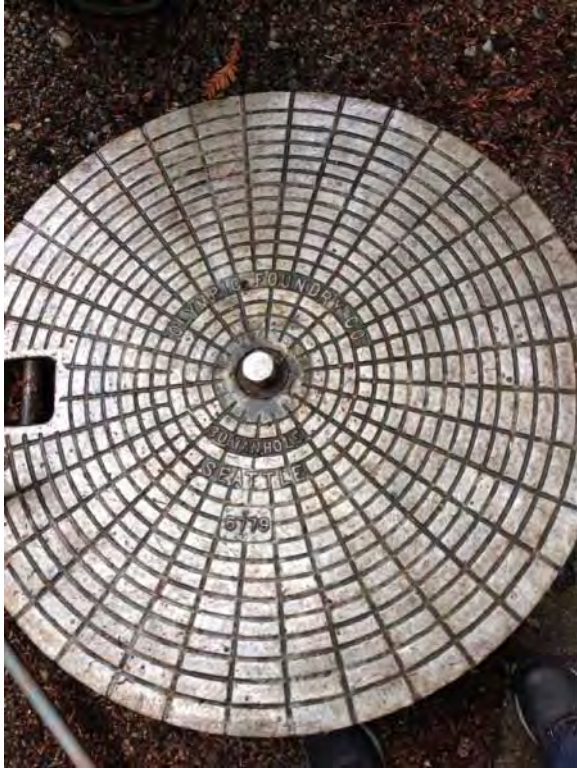
Wet well manhole lid (locking)
