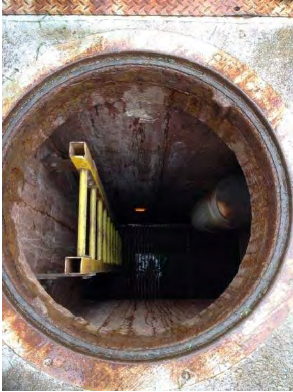
Wet well interior shows signs of corrosion and partial coating failure
