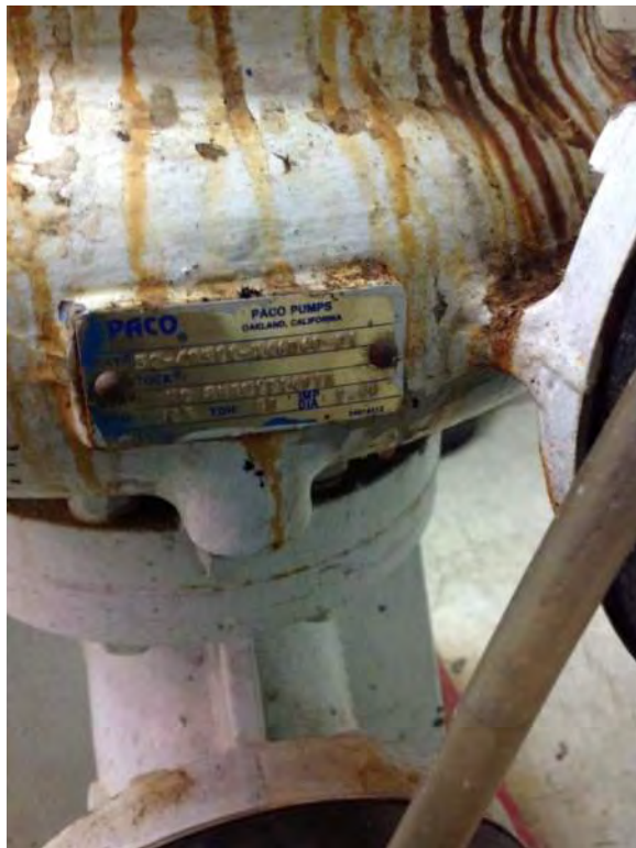
Pump 2 showing signs of aging on exterior
