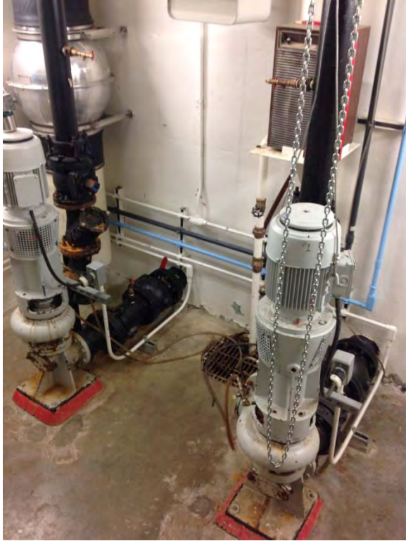
Duplex configuration, pump 1 on the right
