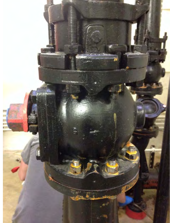
Plug valve vertical installation on discharge piping
