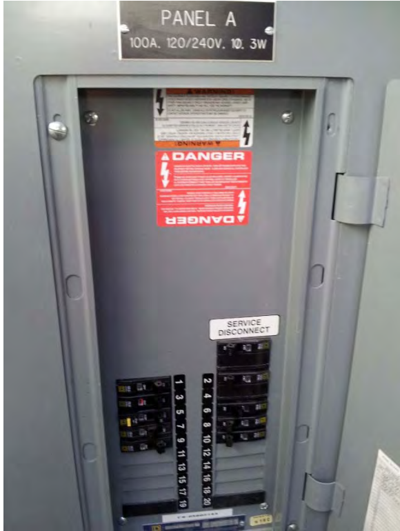
Panelboard located in dry pit
