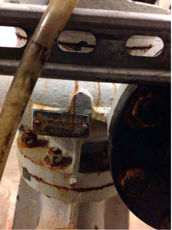
Pump 2 showing signs of aging on exterior
