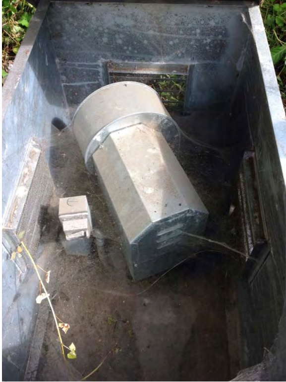
Wet well supply fan located in above grade enclosure
