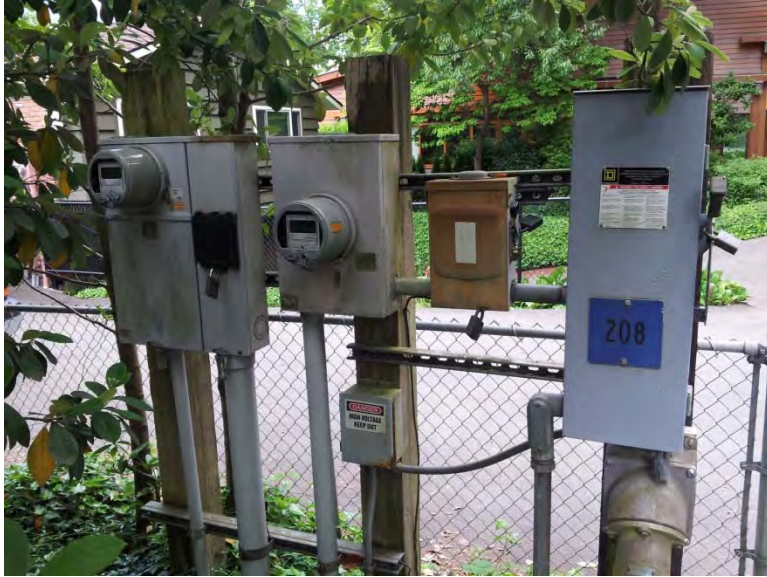
Utility service and generator receptacle located on steel rack near gate, disconnect equipment needs replacement
