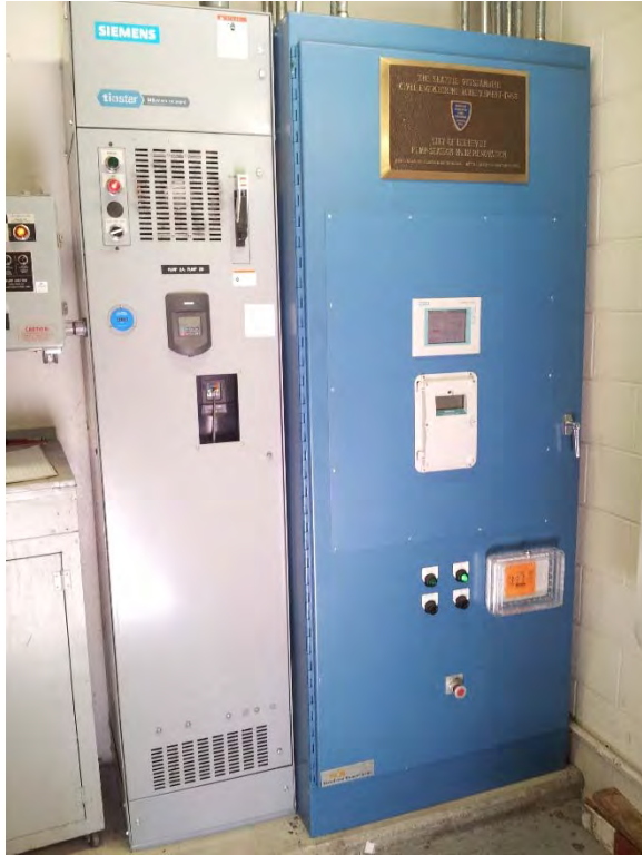
Telemetry control panel with operator interface located on top floor of control building, appears to be in good condition
