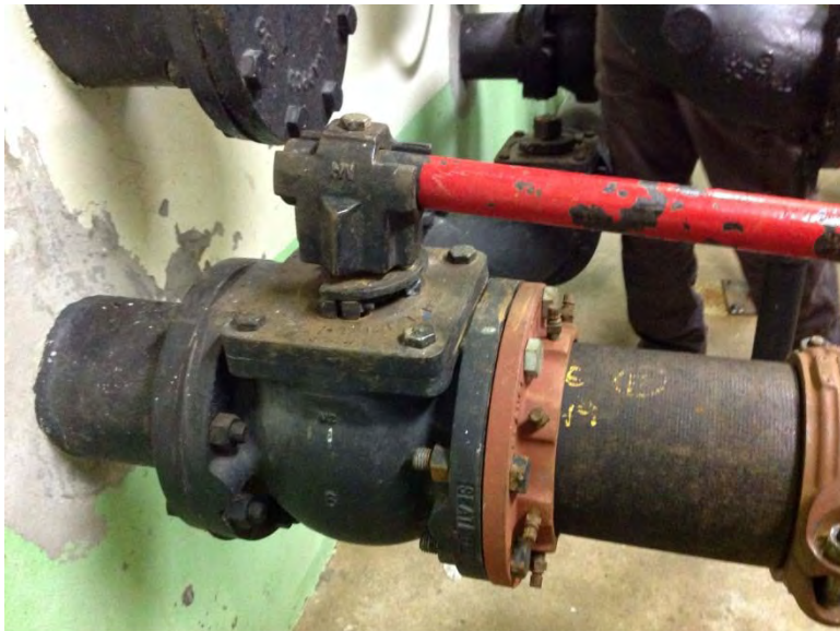
Plug valve on suction piping with vertical axis of rotation – not ideal
