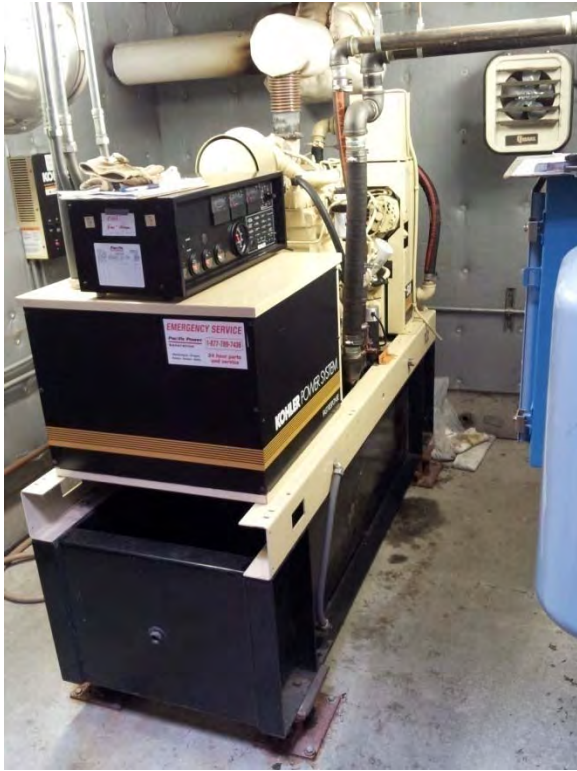
Emergency generator located in underground vault, appears to be in good condition but with decreasing useful life
