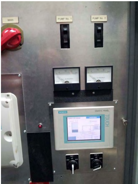
Original Cutler Hammer starters and GE circuit breakers appear to be in good condition but have limited remaining life
