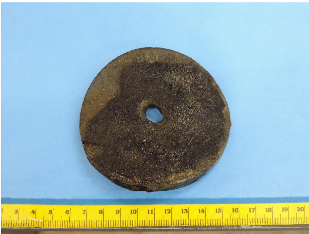
Close up of the inside surface of sample N-2. Note a layer of cement is present.
