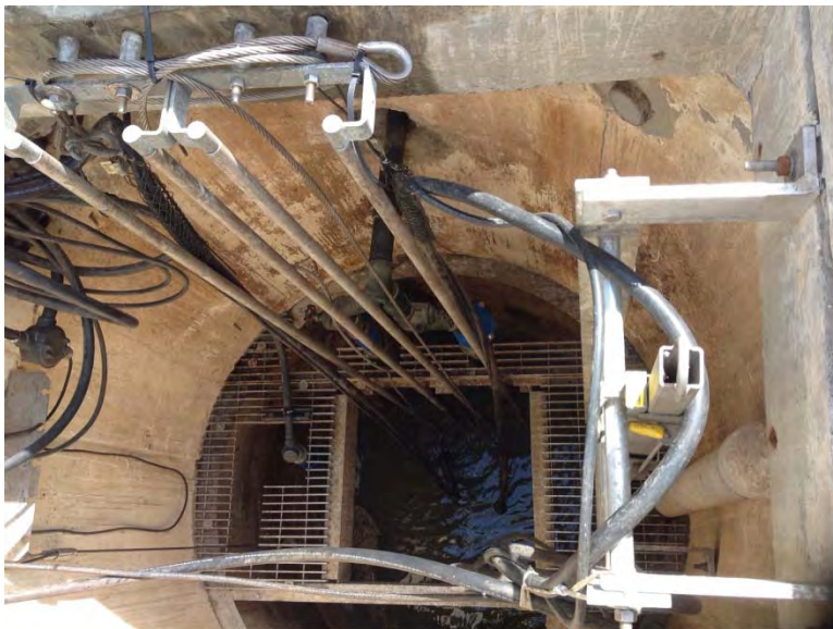
Gateway valve and ball check valve located in wet well, PVC and galvanized discharge piping
