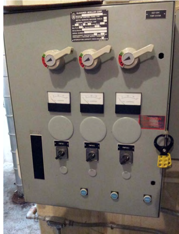
Klockner-Moeller starter and circuit breakers appear to be in good condition, but with decreasing useful life and parts are no longer made
