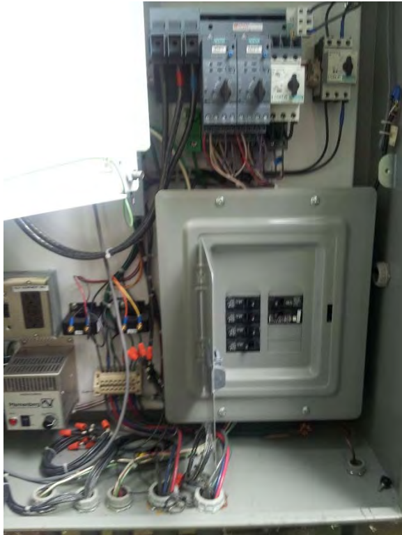
Panelboard located in outdoor power and control panel enclosure, appears to be in good condition
