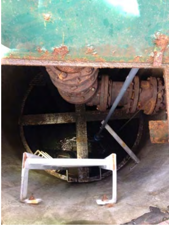
Interior of wet well, small opening for access – underside of hatch showing corrosion
