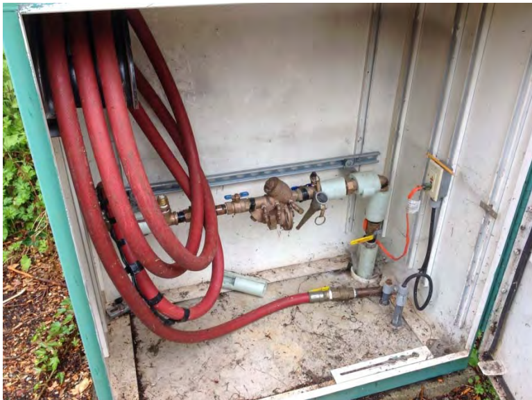
Wilkins reduced pressure backflow assembly and hose bibb located in enclosure with heat tape
