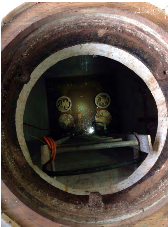
Valves look to be completely submerged in water with just the tops of the valves above water
