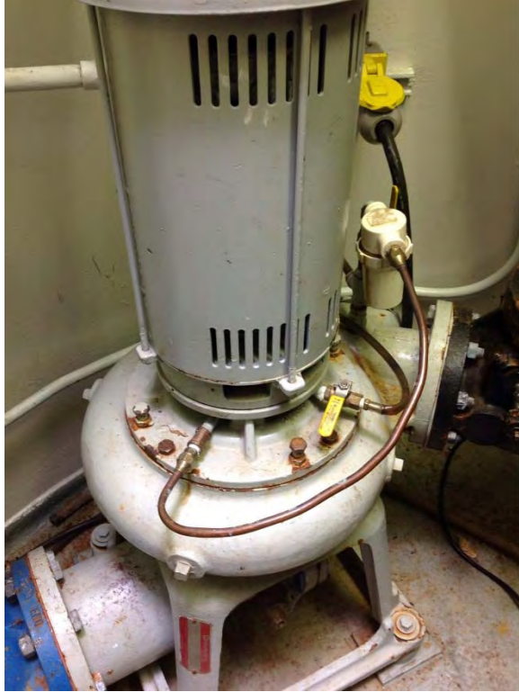
Pump and motor #1
