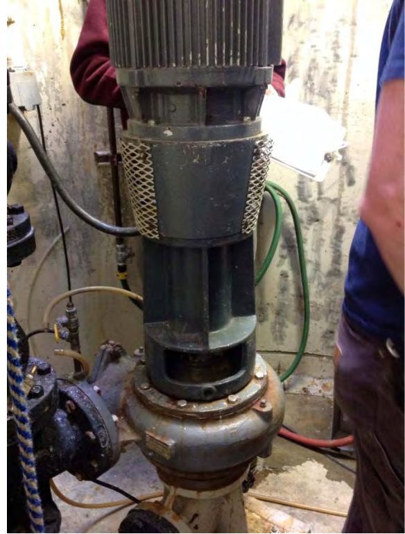
Pump and motor #2
