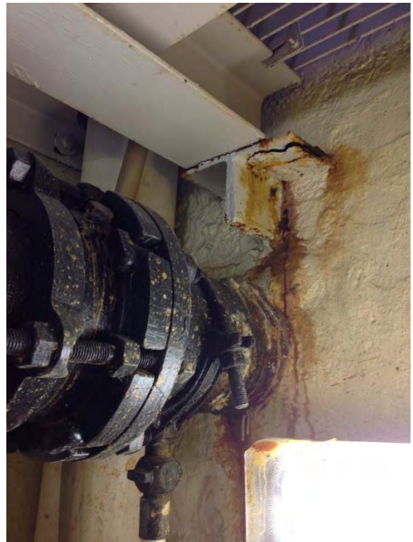
Support bracket for mid level grating platform appears to be significantly corroded, potential failure point
