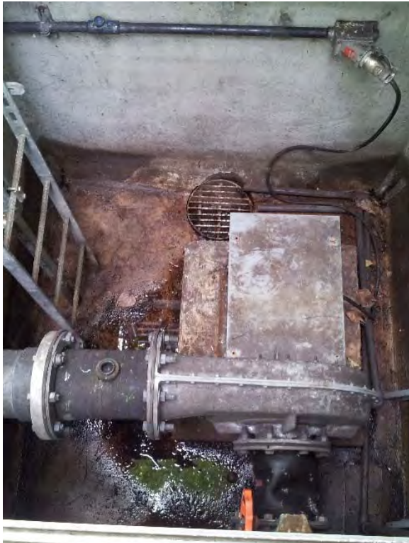
Wet well exhaust fan located in odor control fan vault
