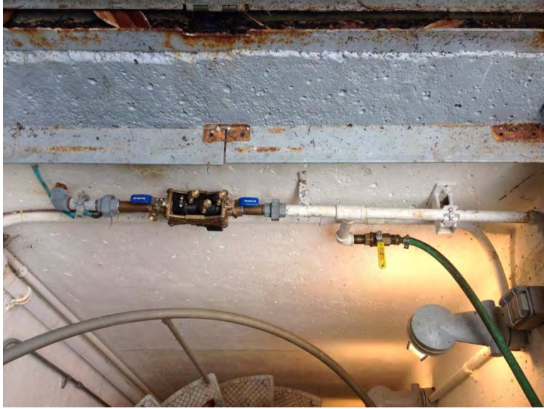
Backflow prevention assembly located near dry pit opening
