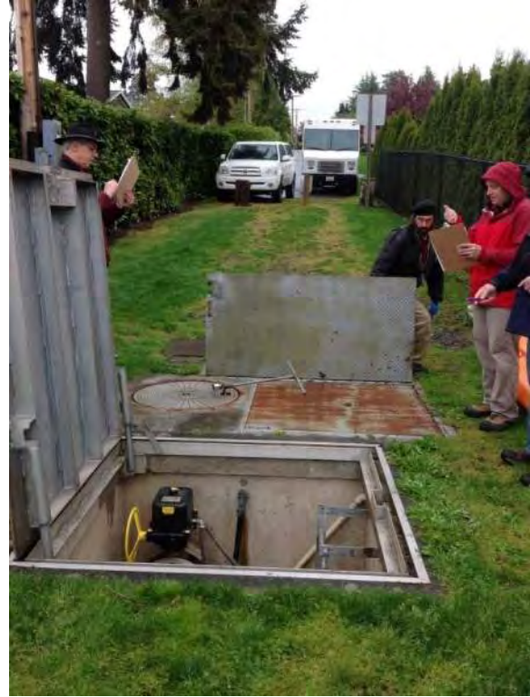
Wet well blower vault hatch opening
