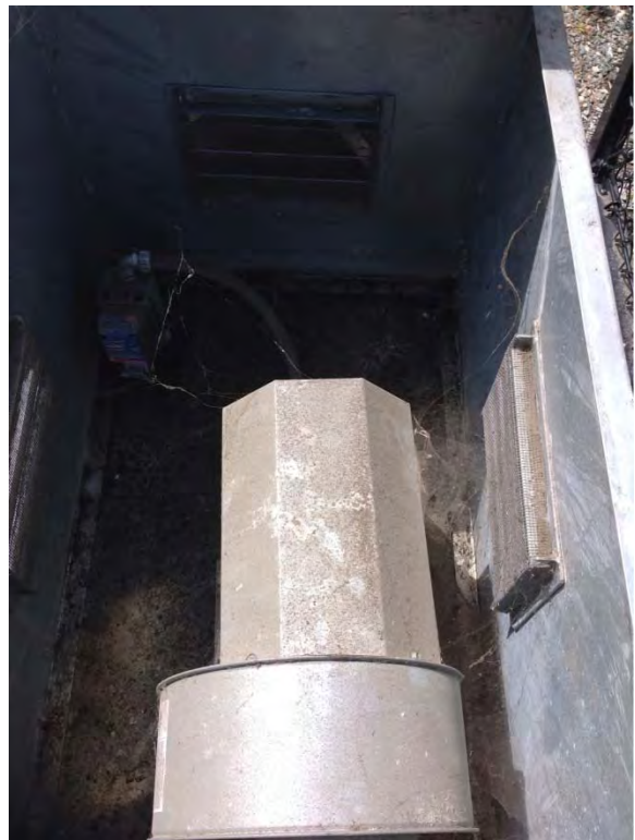
Interior of supply fan above grade steel enclosure
