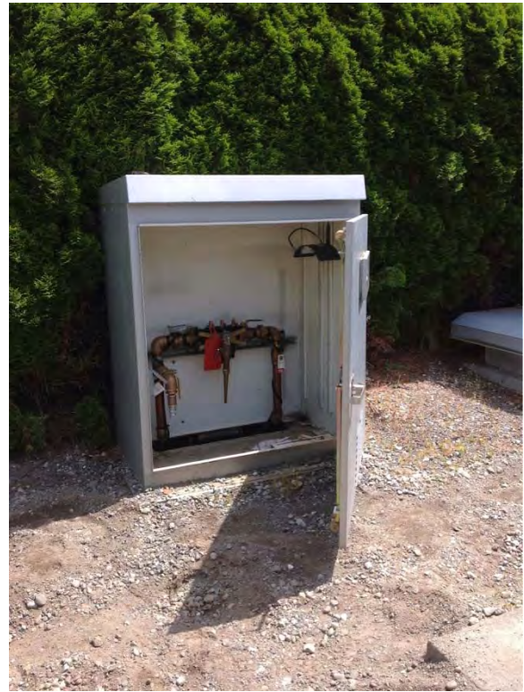
Backflow prevention assembly in above grade enclosure
