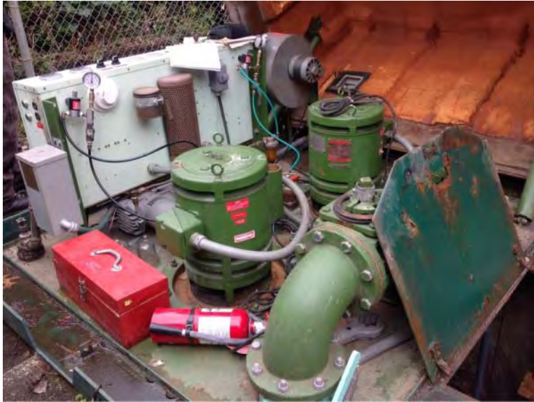
Pumping system sits on top of wet well
