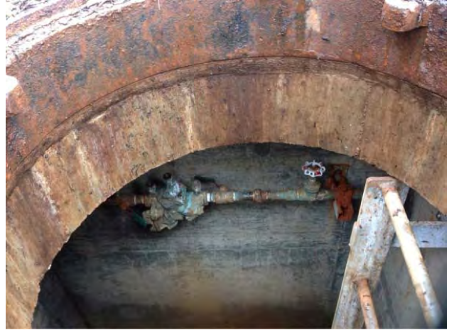
Backflow preventer in check valve and isolation vault
