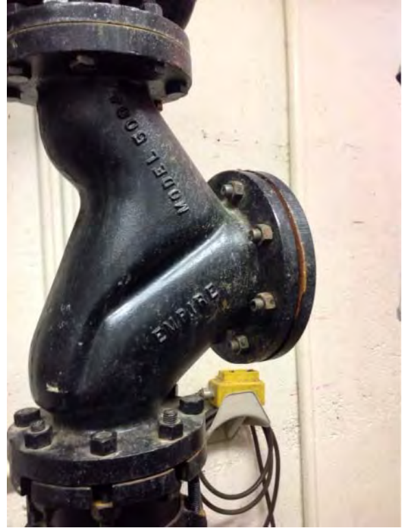
Discharge ball check valve, installed vertically
