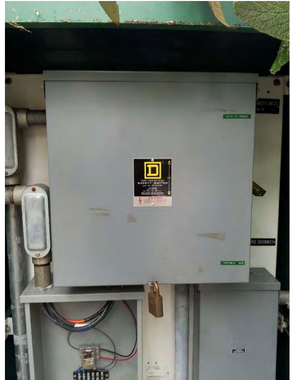
Telephone network interface located in service cabinet
