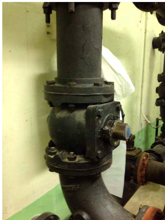
Plug valve on discharge piping seats down – potential gravel trap
