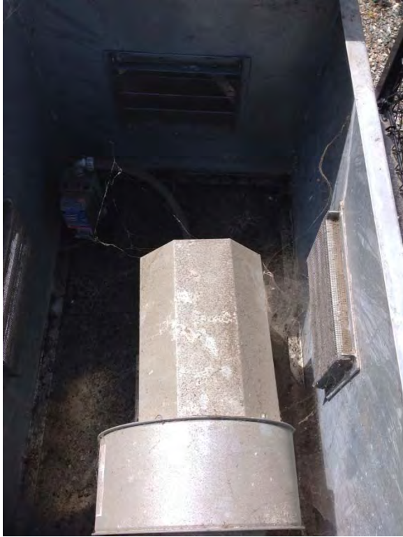
Wet well supply fan located in above grade steel enclosure
