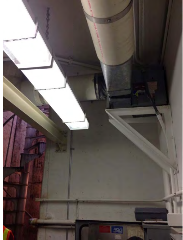
Supply fan located near ceiling of dry pit
