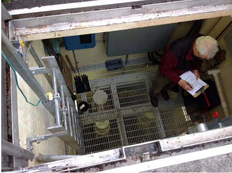
Panelboard and starters located on upper level of dry pit
