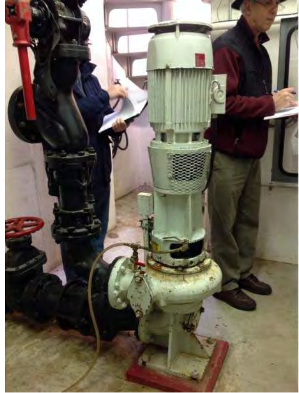
Pump and motor #1
