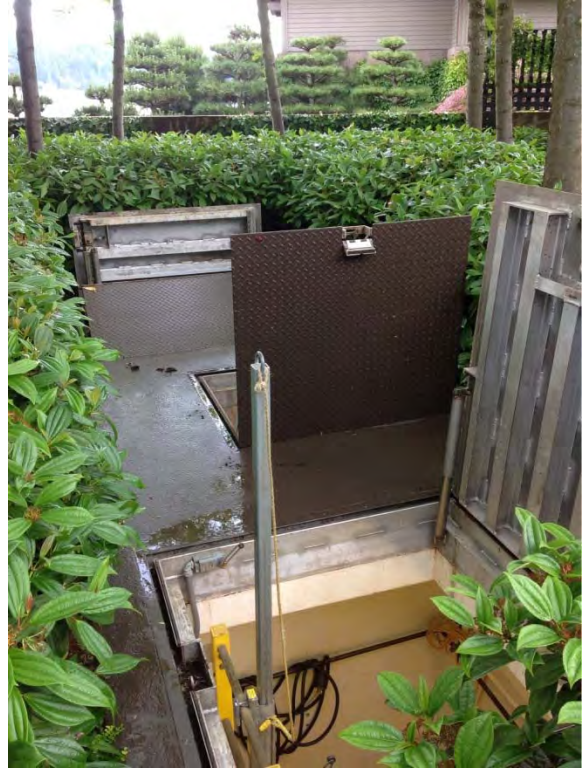
A lot of shrubs surrounding station, maintained by others
