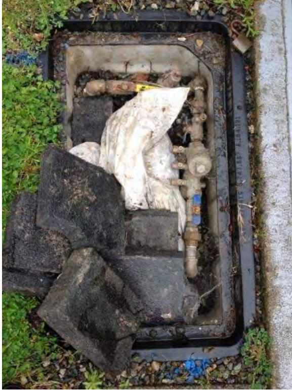
Backflow preventer assembly, below grade
