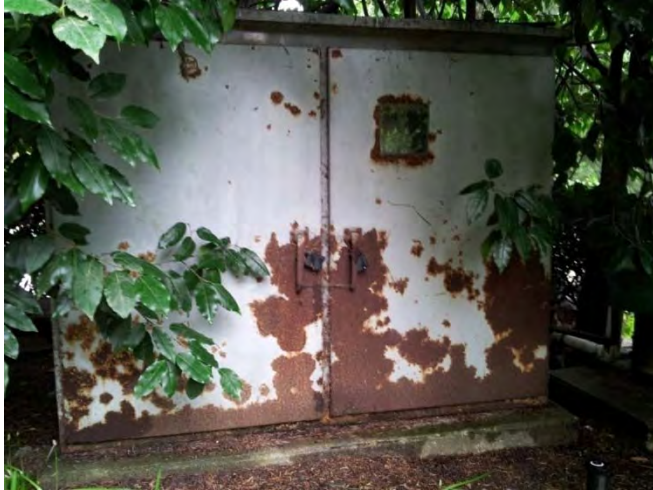
Rusted service cabinet near vent
