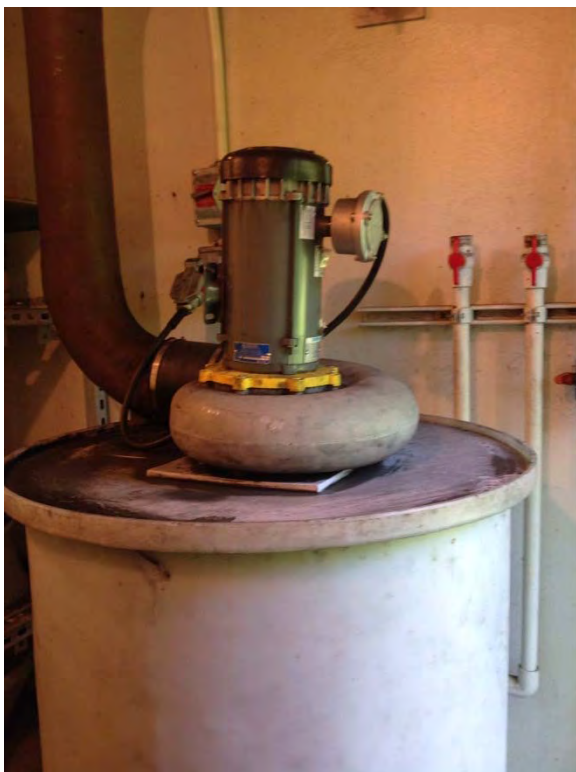
Centrifugal exhaust fan located on top of carbon canister
