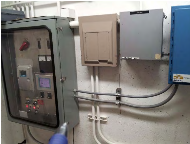
Starter/control panel located in dry pit
