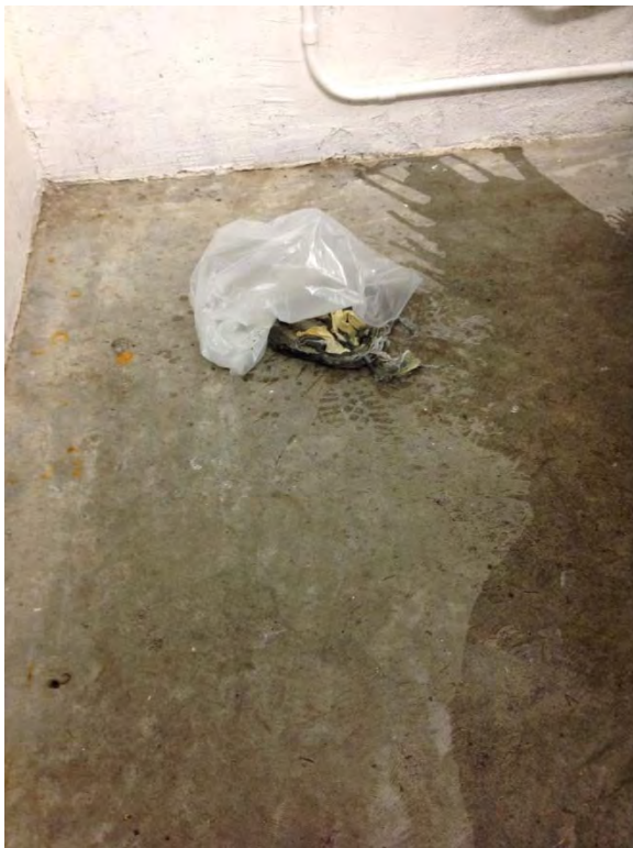
Rag removal from Pump 1 was performed during evaluation visit
