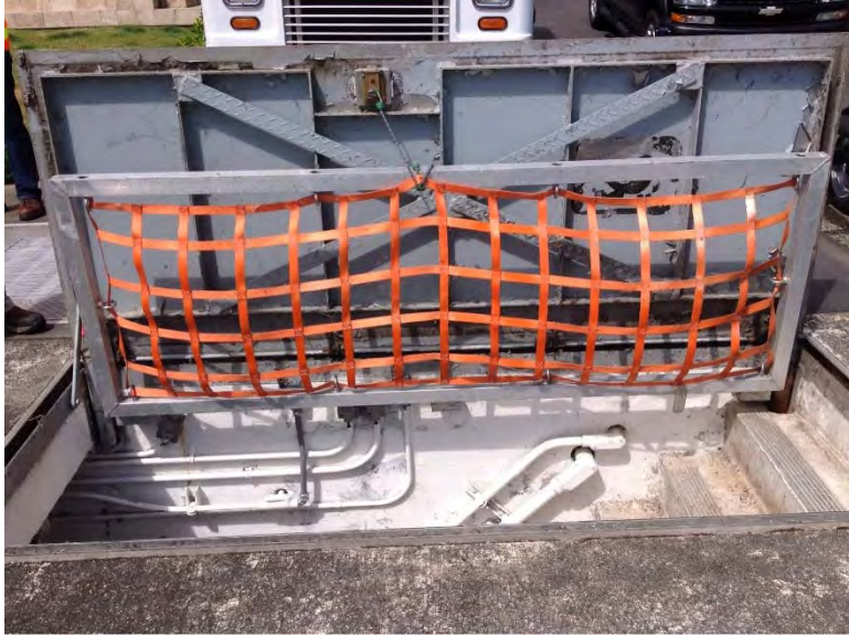
Dry pit fall protection net near stairway
