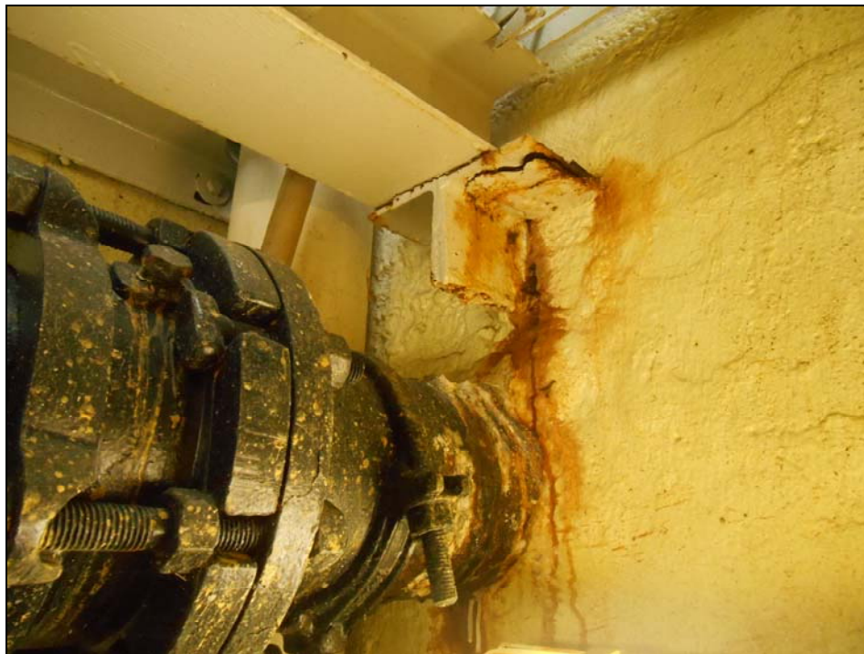
Photo 2: Beam Seat in Need of Replacement & 6" Cast Iron Pipe with Surface Rust
