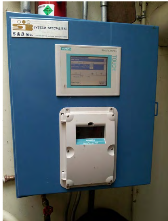
Telemetry control panel located in dry pit, appears to be in good condition
