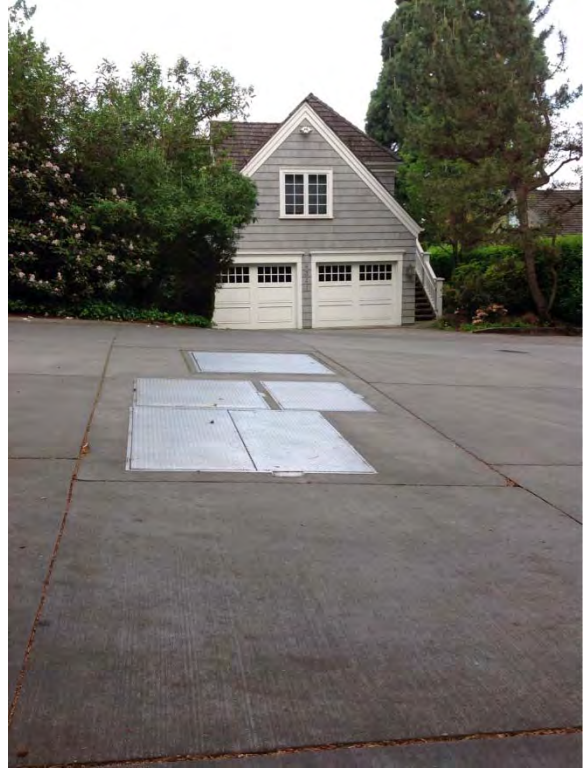
Potentially blocking access to several homes with large service truck and with vault hatches open
