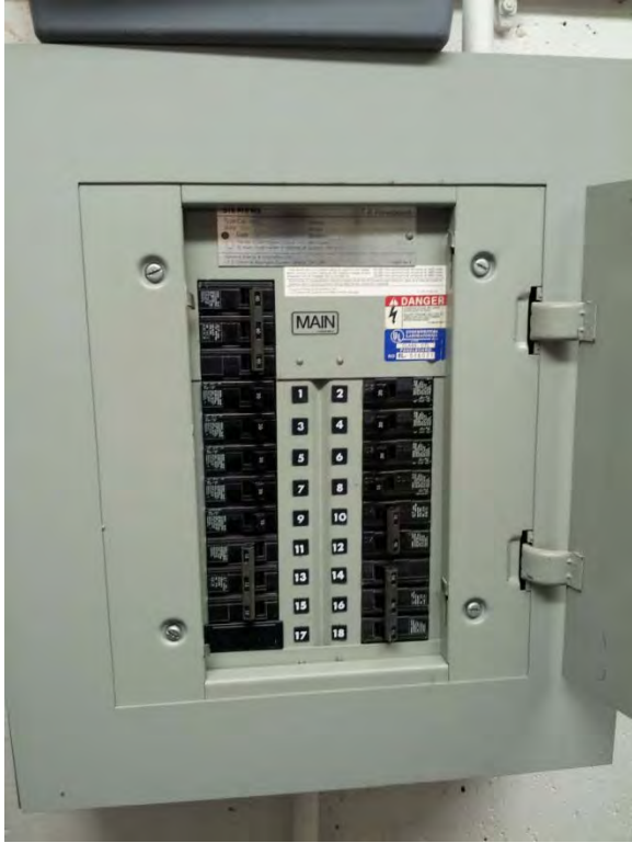
Panelboard located in dry pit, appears to be in good condition
