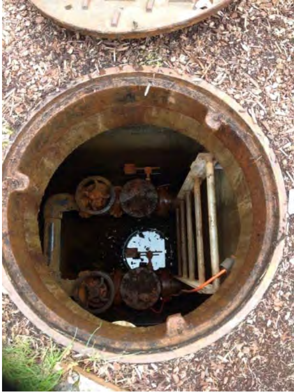
Underground vault accessed through manhole lid. Standing water present.
