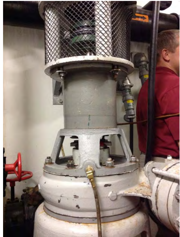
Pump and motor 1B
