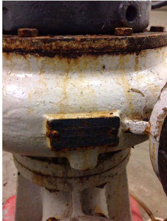
Pump #1 showing signs of aging on exterior
