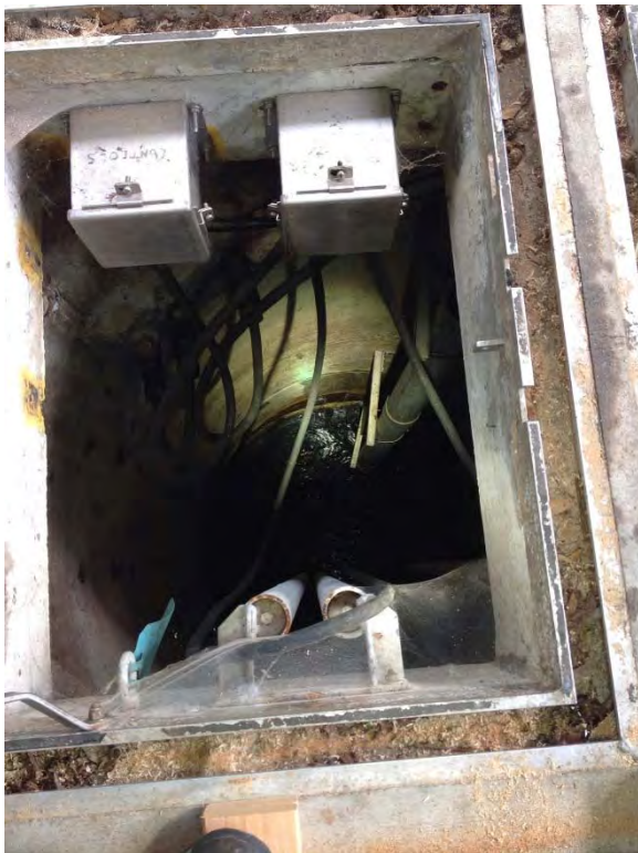
Some seepage in wet well, ground water intrusion in three locations, near bottom of wet well
