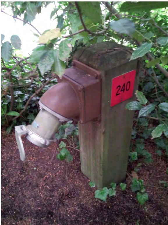
Generator receptacle on wood post
