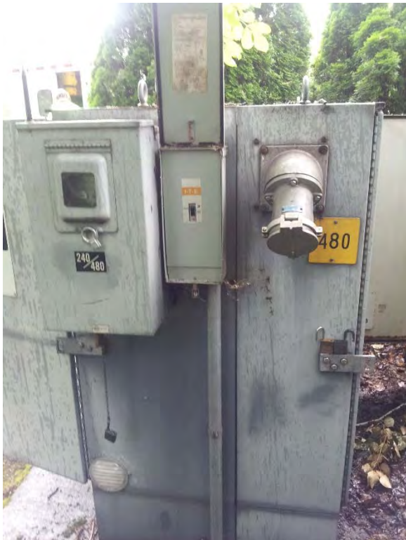
Electrical service meter and generator receptacle located outside of power enclosure
