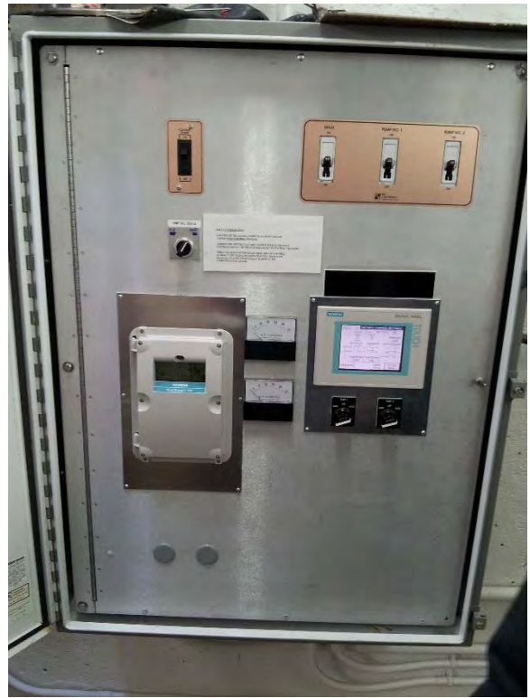
Starters located in dry pit, appears to be in good condition
