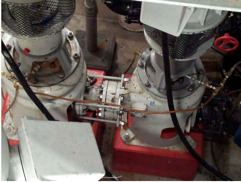
Pumps 1A and 1B
