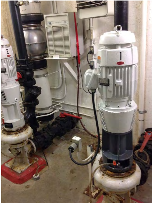
Duplex configuration, pump #1 in foreground
