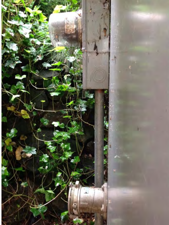
Service meter and generator receptacle located on side of power and control panel enclosure near paved road
