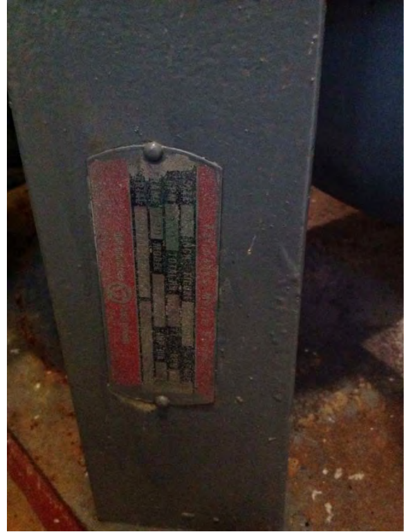
Pump name plate, painted over, difficult to read information, typical of all three pumps
