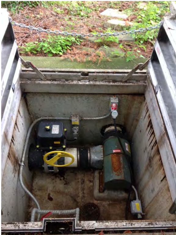
Interior of wet well blower vault
