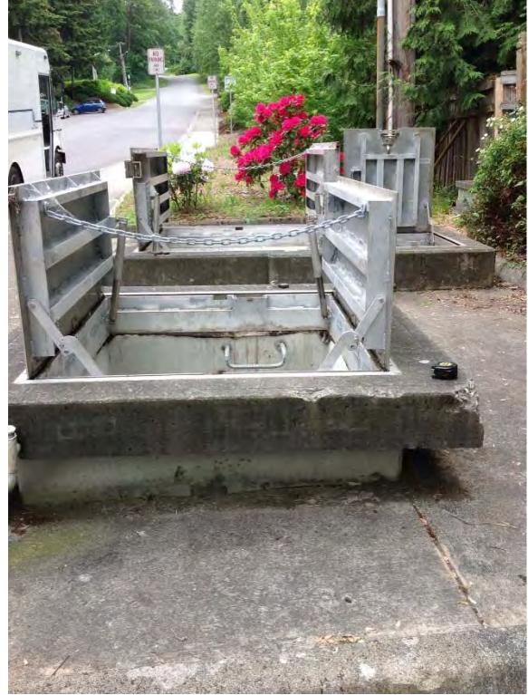
All vaults raised 12” – 18” above grade
