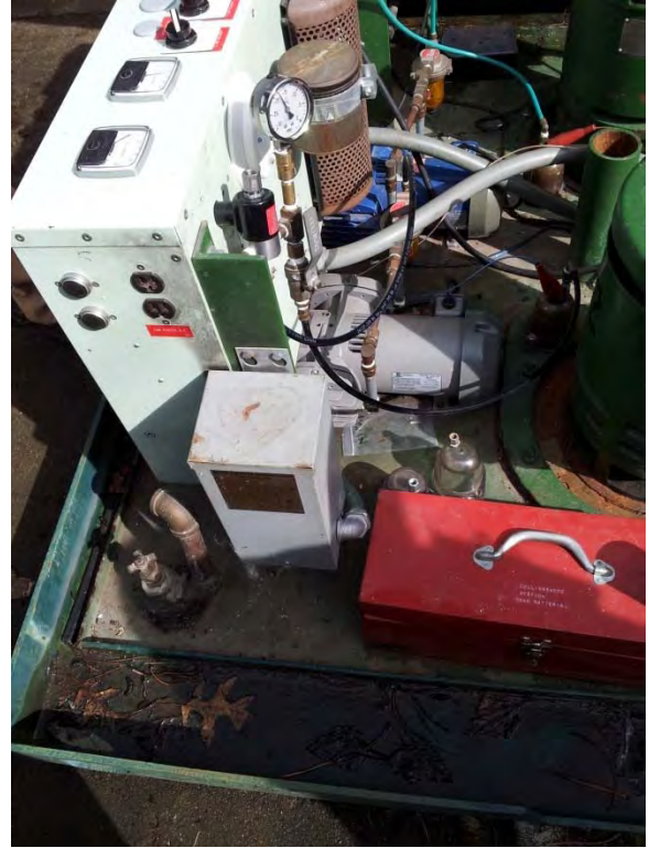
Heat sensors for ventilation cooling on power and control panel
