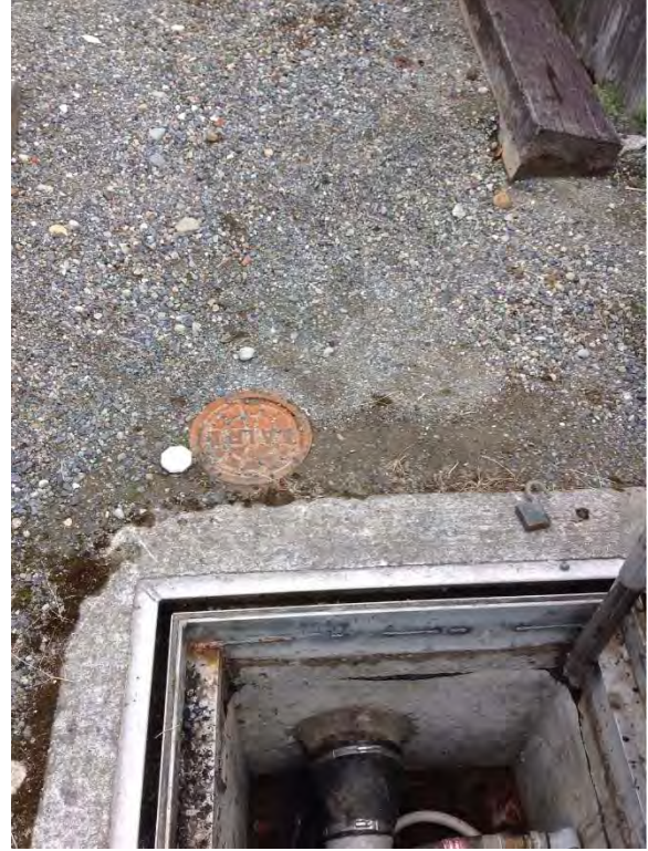
Air valve adjacent to vault
