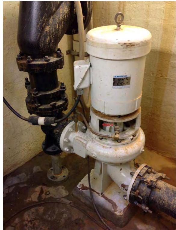
Pump and motor #2, showing signs of aging on exterior
