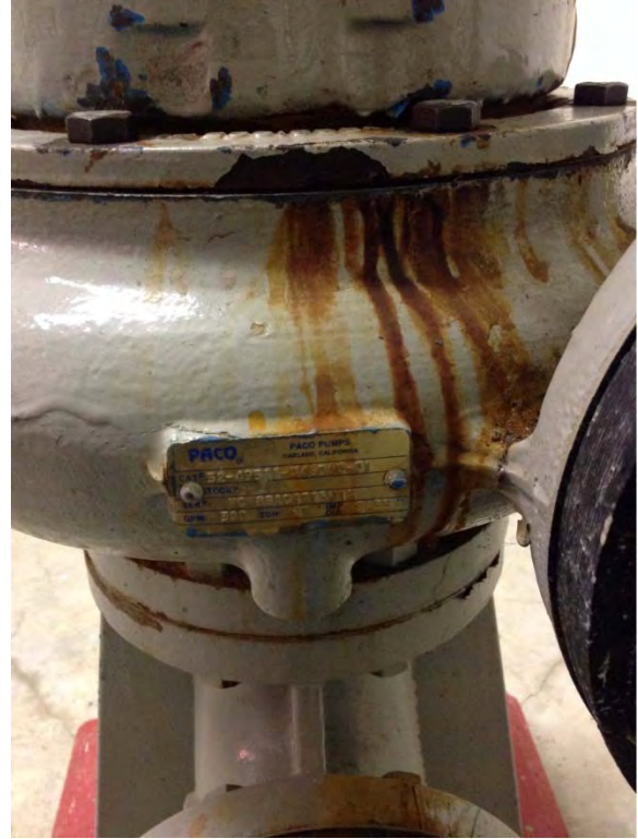
Pump 2 showing signs of aging on exterior
