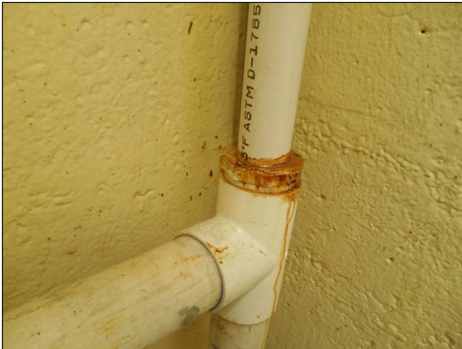
Photo 4: Water Leak at Tee Fitting
