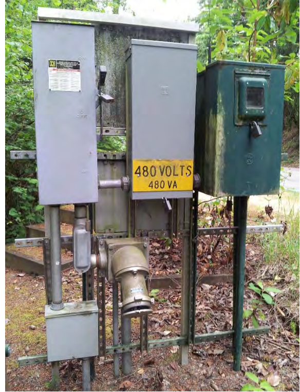
Generator receptacle located on rack
