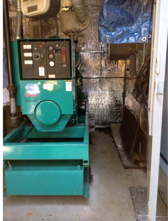
Generator located in vault
