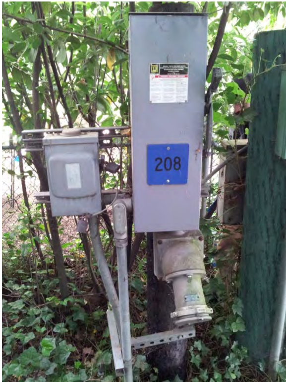
Generator receptacle located below manual transfer switch
