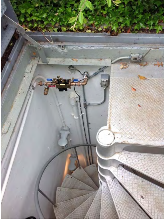
Backflow prevention assembly near top of dry pit
