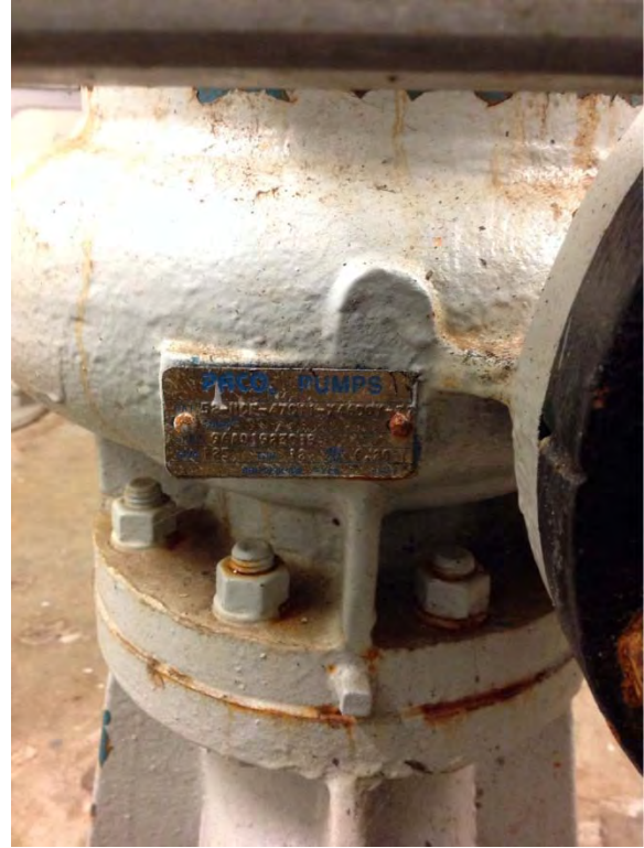
Pump 1 showing signs of aging on exterior
