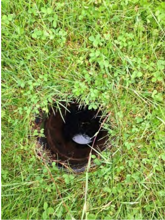
Force main isolation valve not accessible
