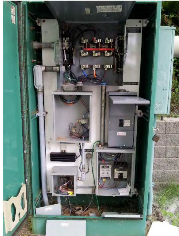
Interior of service cabinet including manual transfer switch
