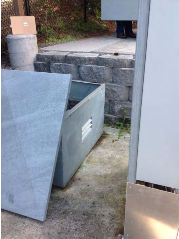
Above grade steel enclosure for exhaust fan
