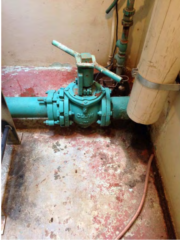
Plug valve isolation for suction piping, vertical axis of orientation – not ideal
