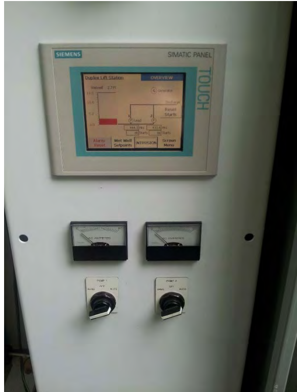
Starters located in outdoor power and control panel enclosure, appear to be in good condition
