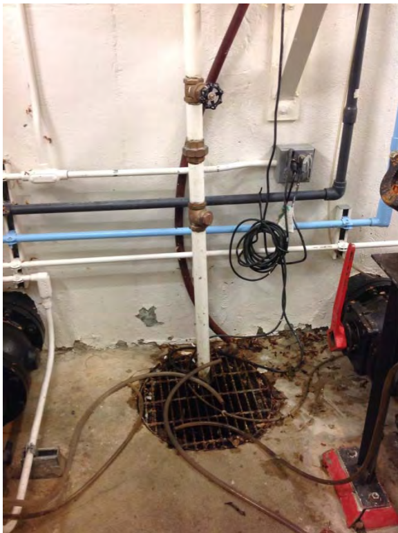
Grating on sump drain, note some coating failing near bottom of wall
