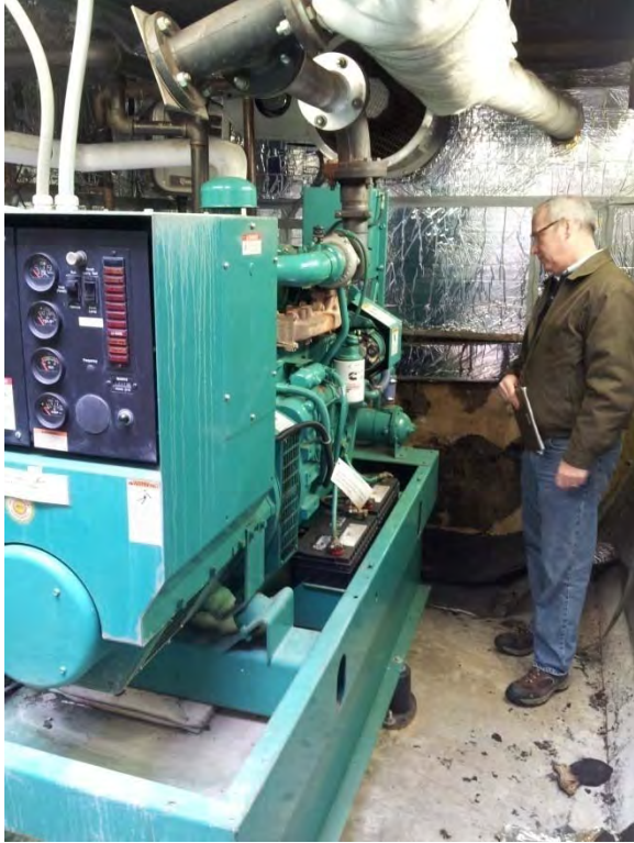
Emergency generator located in underground vault, appears to be in good condition but with decreasing useful life
