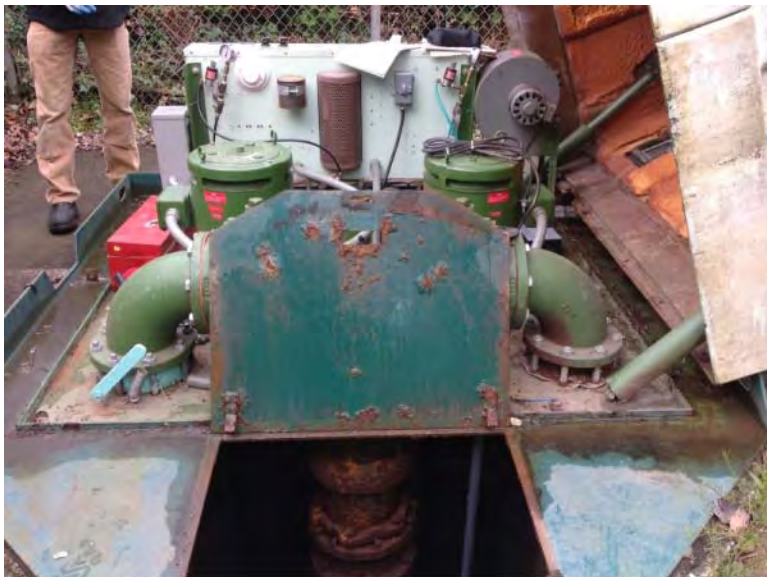
Some rusting on interior of steel plate – likely indicates corrosion on underside of metal floor. Wet well hatch is not sized to prevent dropping into wet well.
