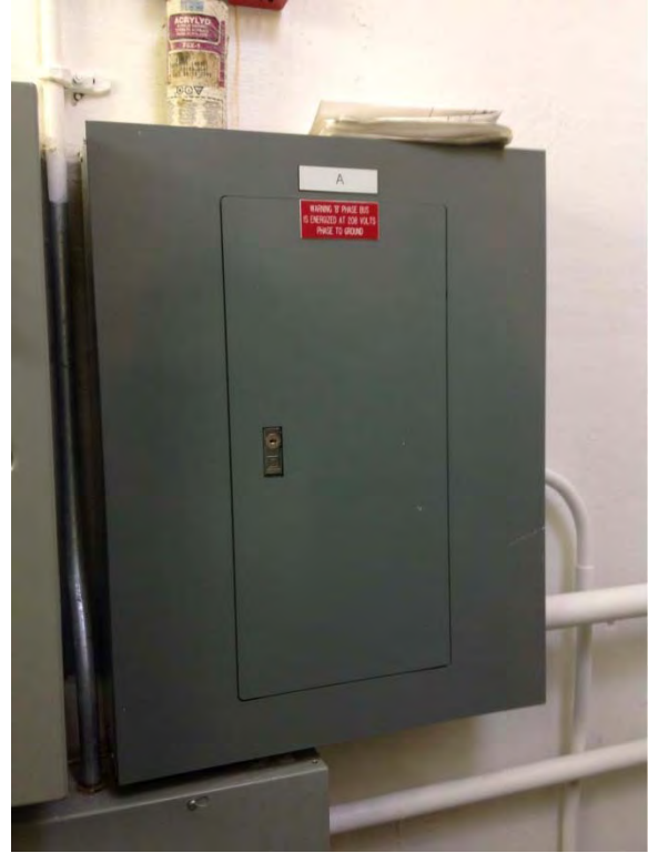
Panelboard for both Flush 9 and 10 located in Flush 10 dry pit, appears to be in good condition but aging
