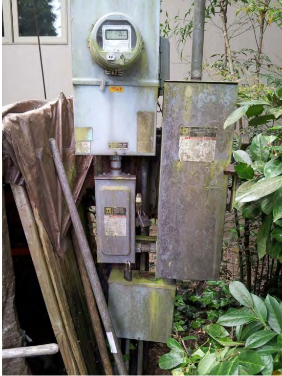
Utility service, service meter and manual transfer switch located on pole adjacent to site
