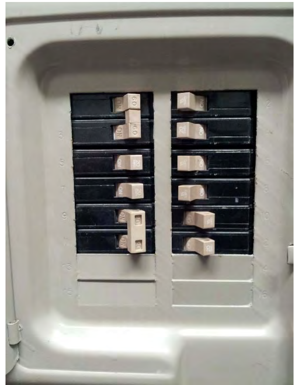
Cutler Hammer Load Center is nearing end of useful life
