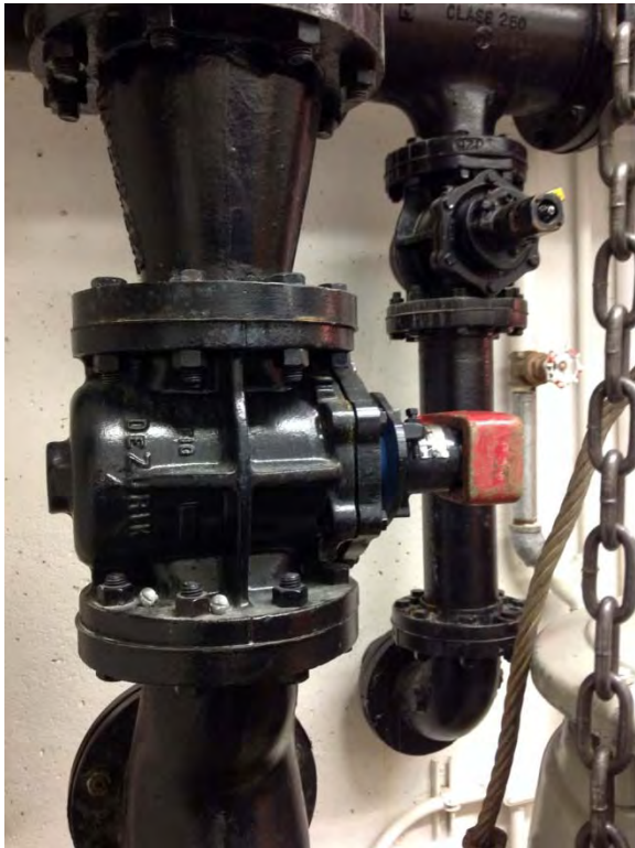
Plug valve on discharge piping
