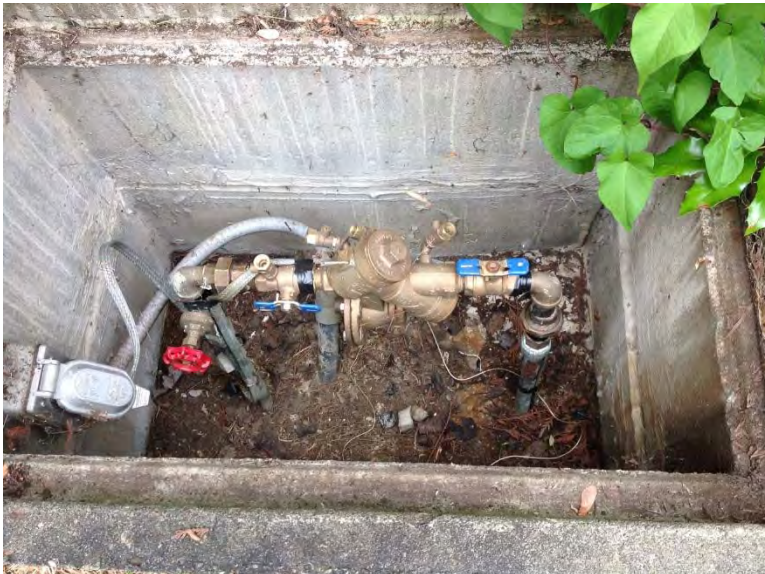
Backflow prevention assembly in water boxes
