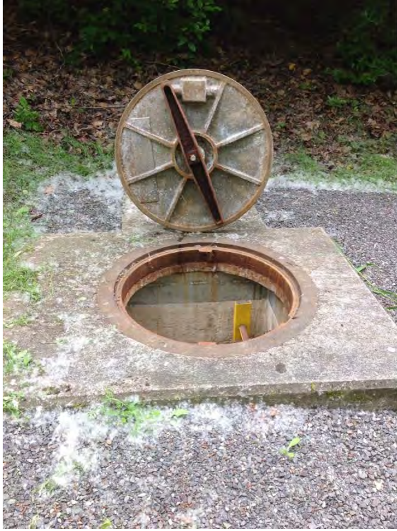
Manhole lid and top portion of wet well
