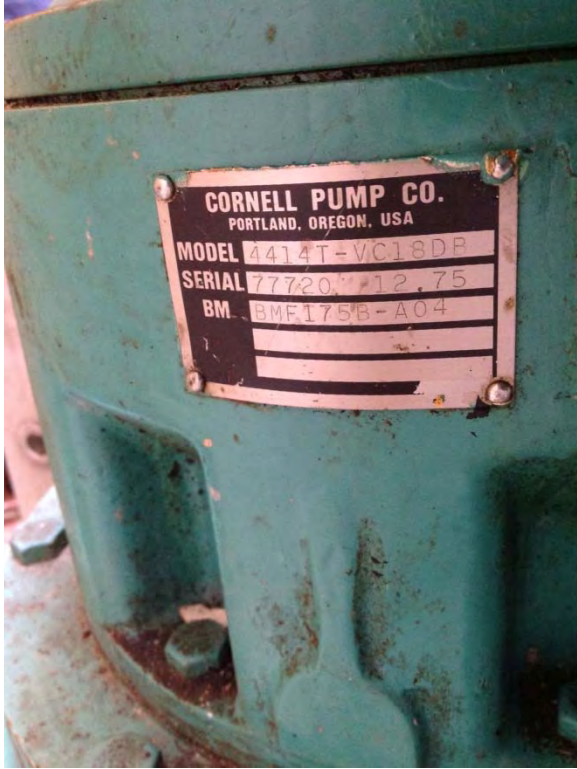
Pump 1 showing signs of aging on exterior
