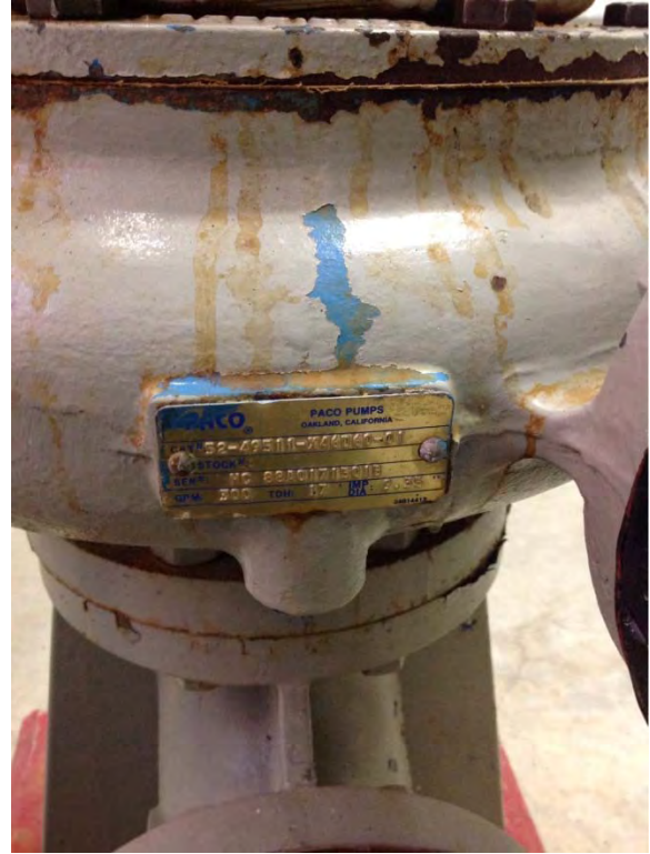
Pump 1 showing signs of aging on exterior
