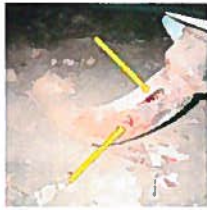
An example of older cast iron in bad shape
