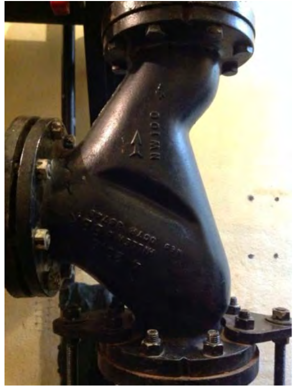
Discharge ball check valve, installed vertically
