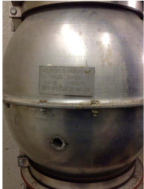
Supply fan located 5 feet AFF in dry pit
