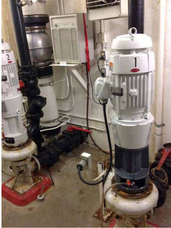
Duplex configuration, pump #1 on the right
