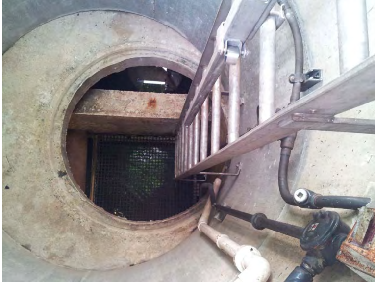
Interior of wet well including connected overflow wet well
