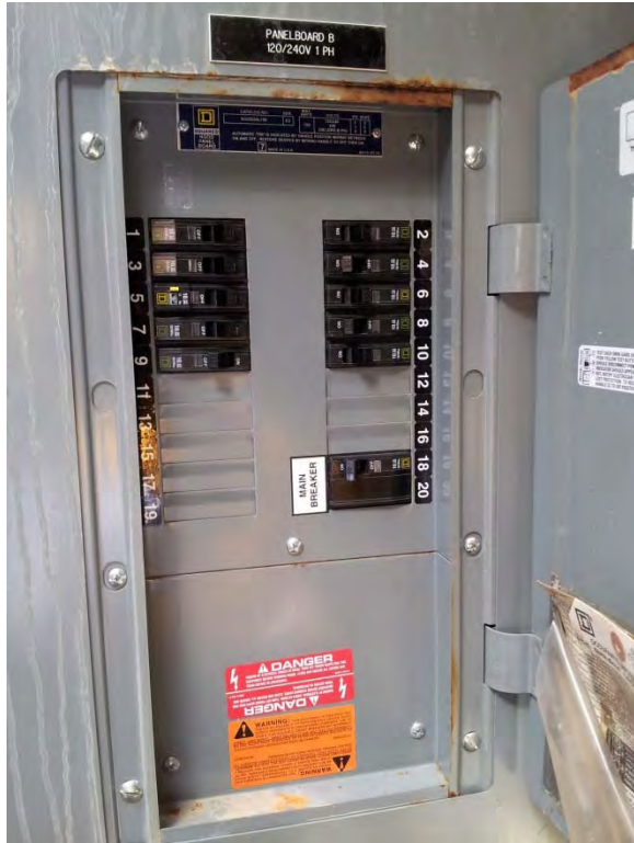
Panelboard located in dry pit/generator vault, some surface rust
