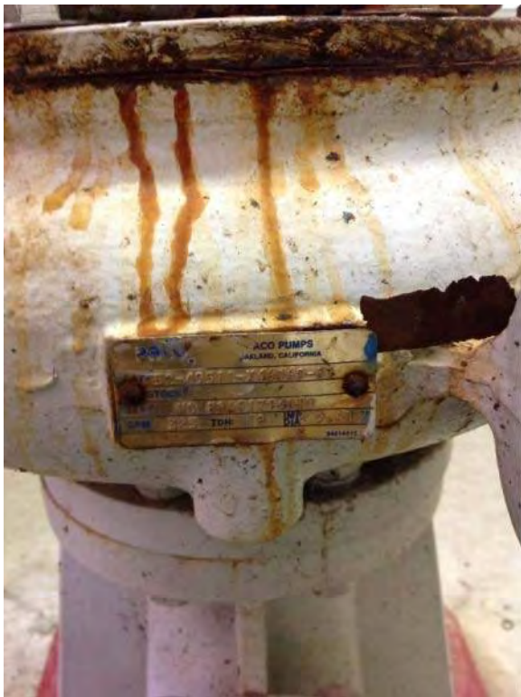
Pump 1 showing signs of aging on exterior
