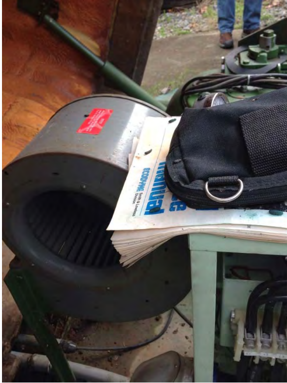
Supply fan on steel plate
