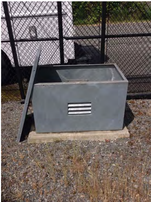
Above grade steel enclosure for supply fan
