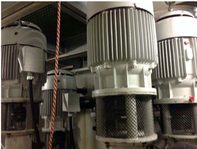
Interior of dry pit pump level
