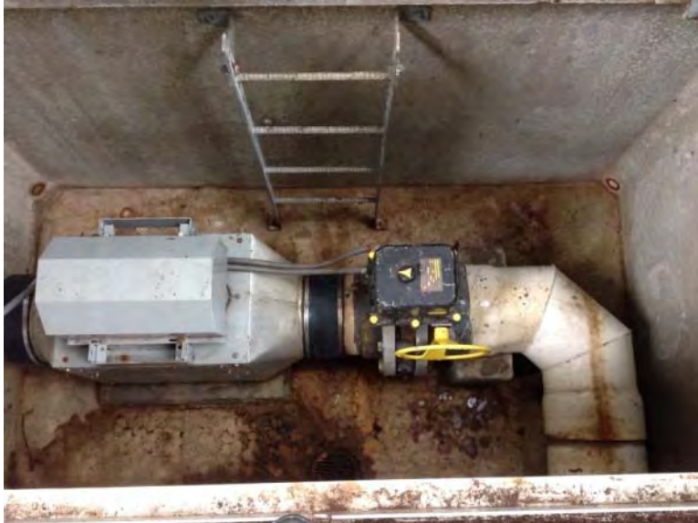
Interior of blower vault shows concrete in good shape, but ladder location presents a slightly challenging access
