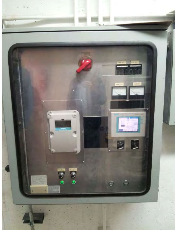
Starters located in dry pit, one original starter approaching end of useful life, the other has been replaced with a newer model
