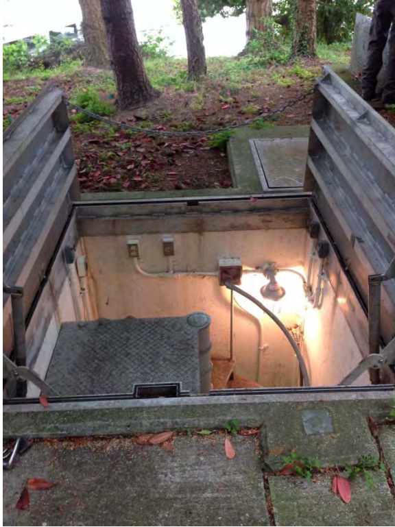
Lift assist access hatch and spiral staircase, chain fall protection on one side
