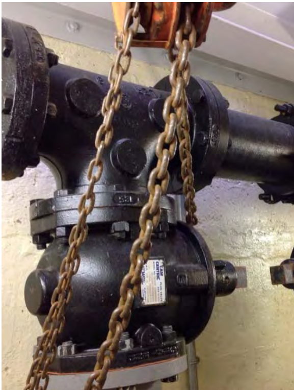
Picking eye is attached to above platform – corrosion issue on mid level grating platform
