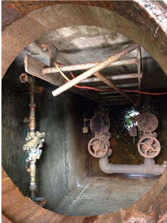
Gate valve with hand wheel for isolation and swing check valve with outside weight and lever
