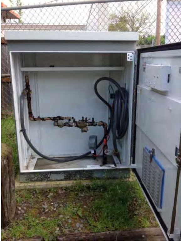
Backflow preventer in above ground enclosure
