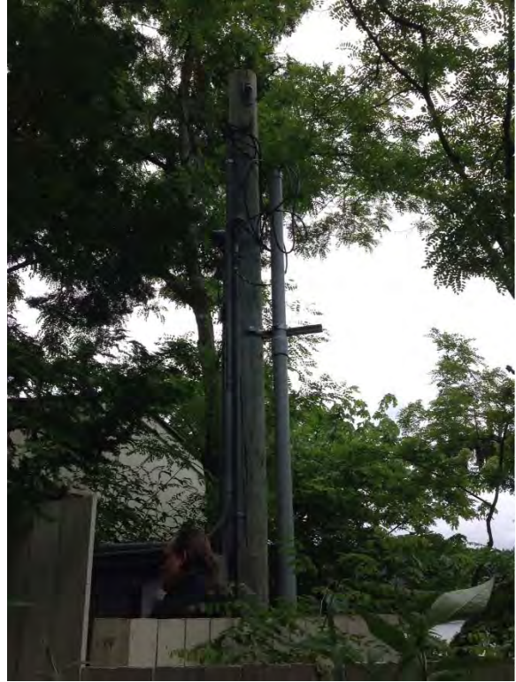
Overhead utility transformer, a lot of exposed cable
