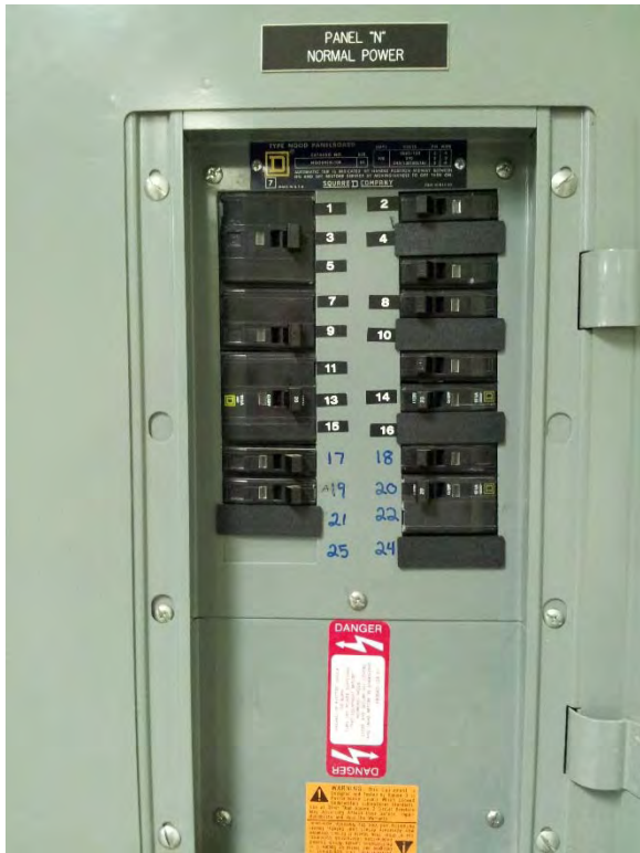
Panelboard located on south wall in the control building
