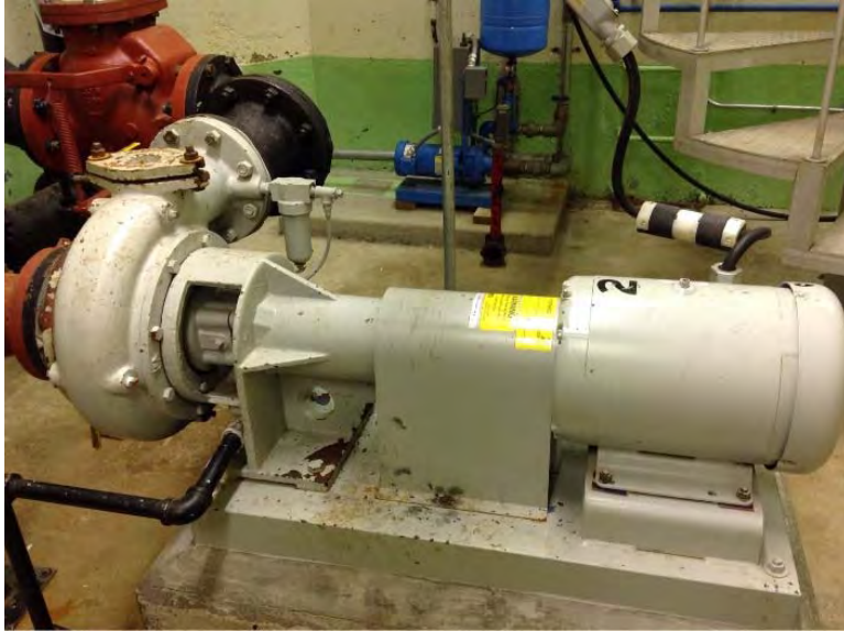
Pump and motor #2
