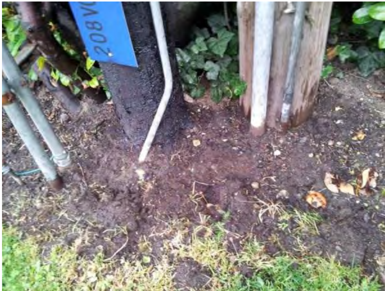
GRC conduit corroded at grade
