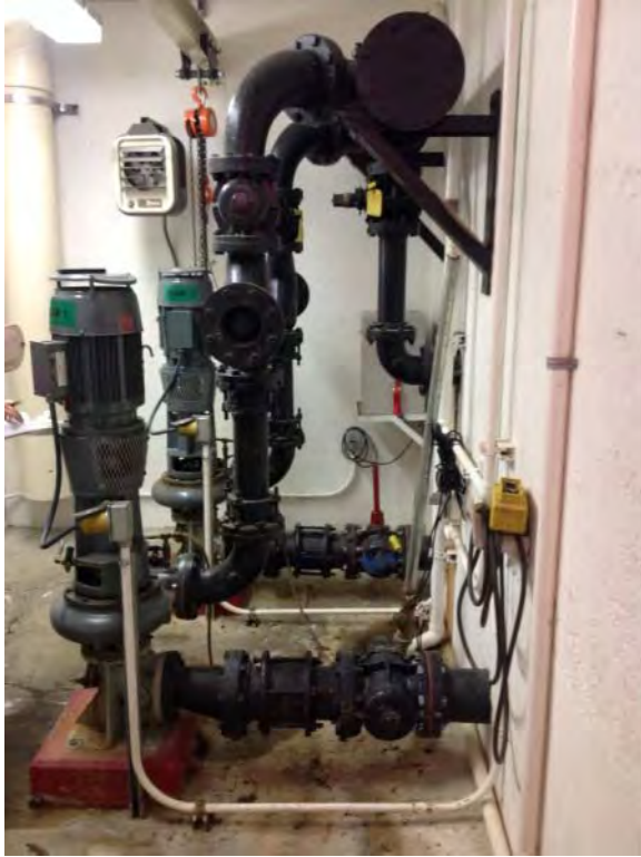
Pumps and piping in dry pit
