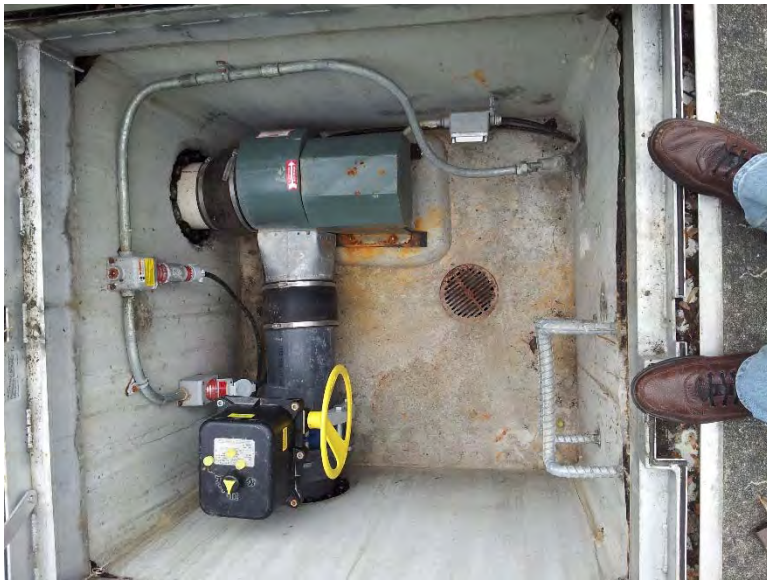
Interior of wet well blower vault
