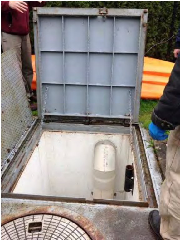
Equipment access hatch
