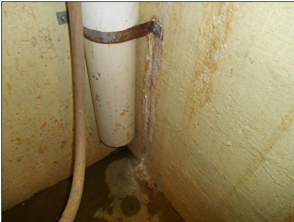
Photo 6: Efflorescence at Concrete Wall
