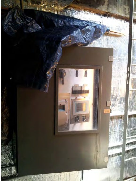
Starter/control panel with operator interface located under tarp in dry pit/generator vault
