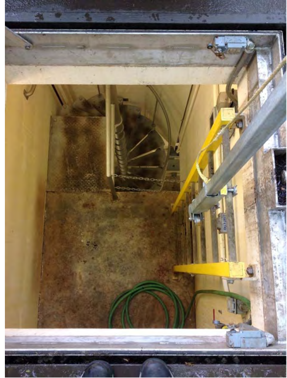
Ladder to first level landing, spiral stair case down to bottom level
