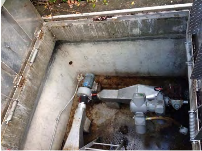
Interior of wet well blower vault appears to be in good condition
