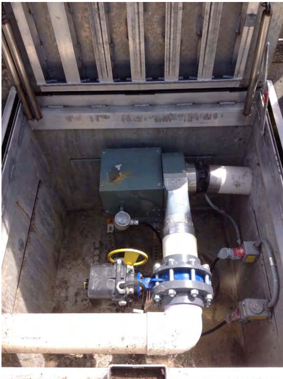
Interior of wet well blower vault appears to be in good condition
