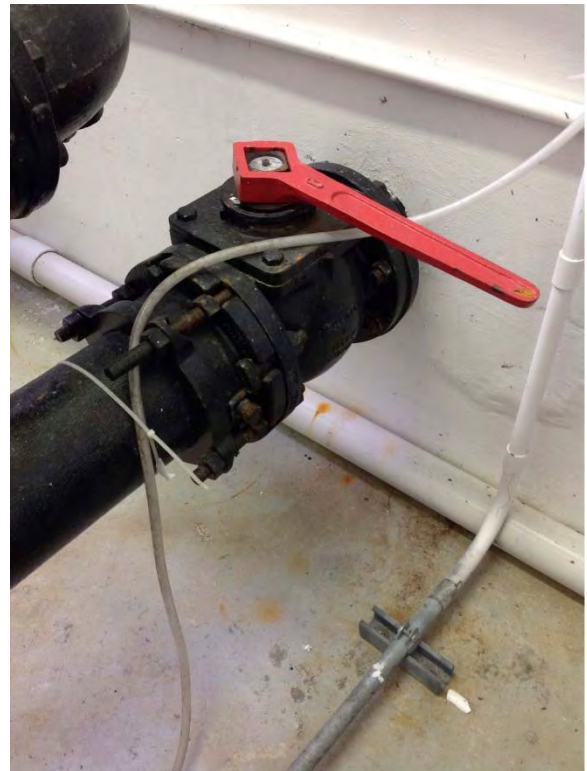
Plug valve installed with vertical axis of rotation on suction piping for pump 2 – not ideal
