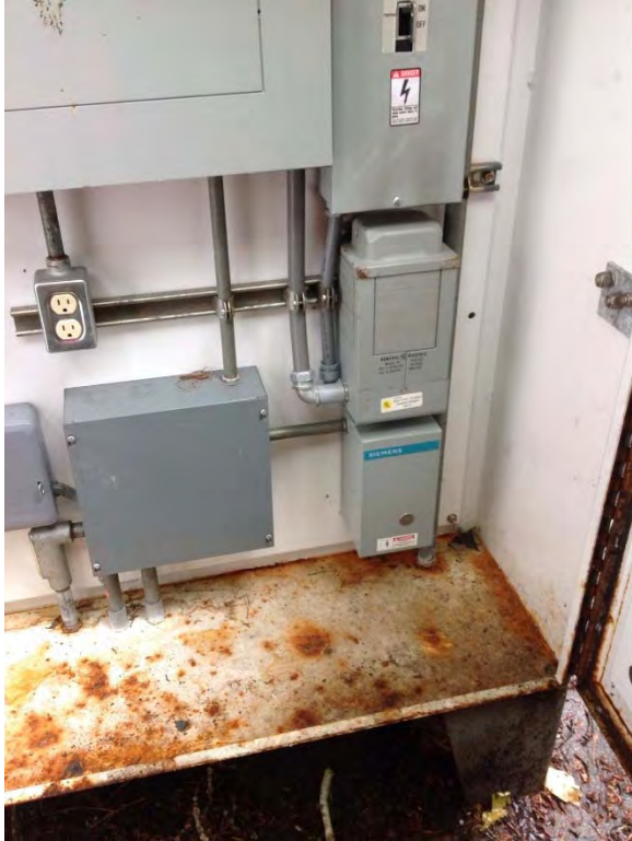
All power and control conductors come through 1-3/4" galvanized rigid conduit with seal rotting
