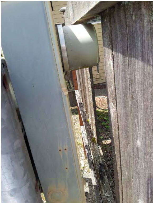
Service meter located on service entrance equipment rack
