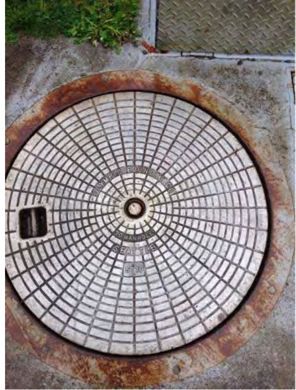
Wet well lid locks to secure access
