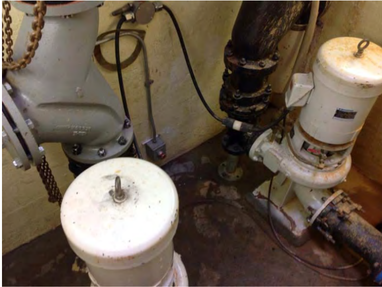
Duplex station configuration, pump 1 on left
