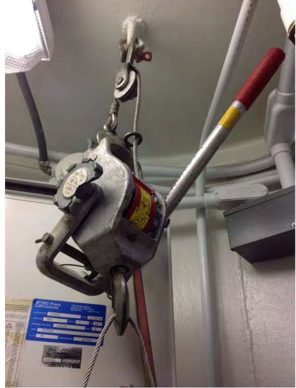
Lifting eye and chain fall attached to ceiling of metal can#1
