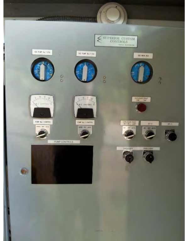
Starters located in power and control panel outdoor enclosure, appears to be in good condition
