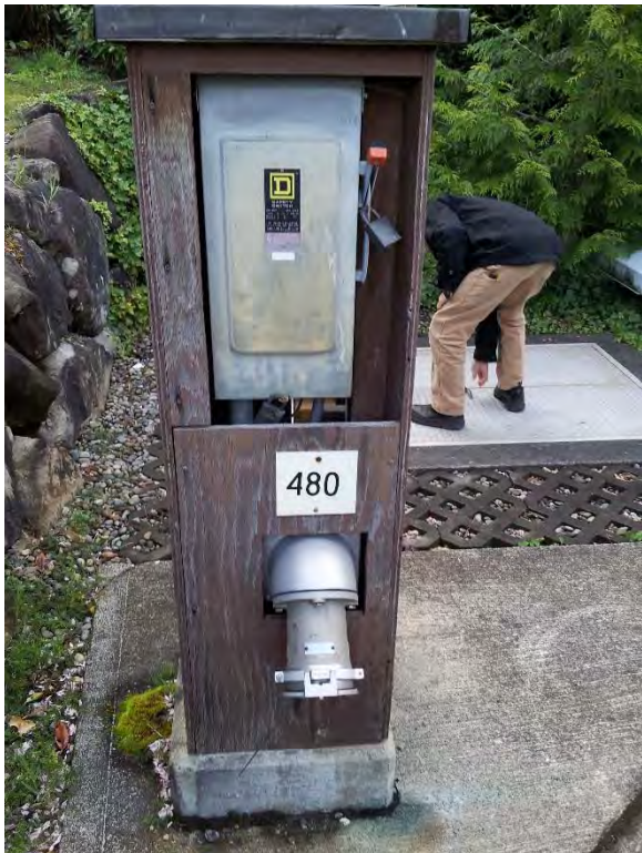
Generator receptacle and transfer switch appear to be in good condition but aging
