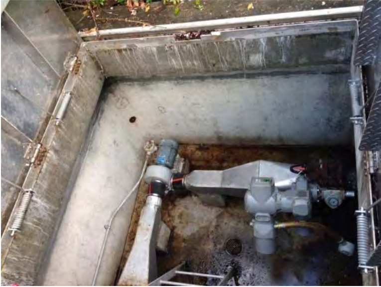
Interior of wet well blower vault appears to be in good condition
