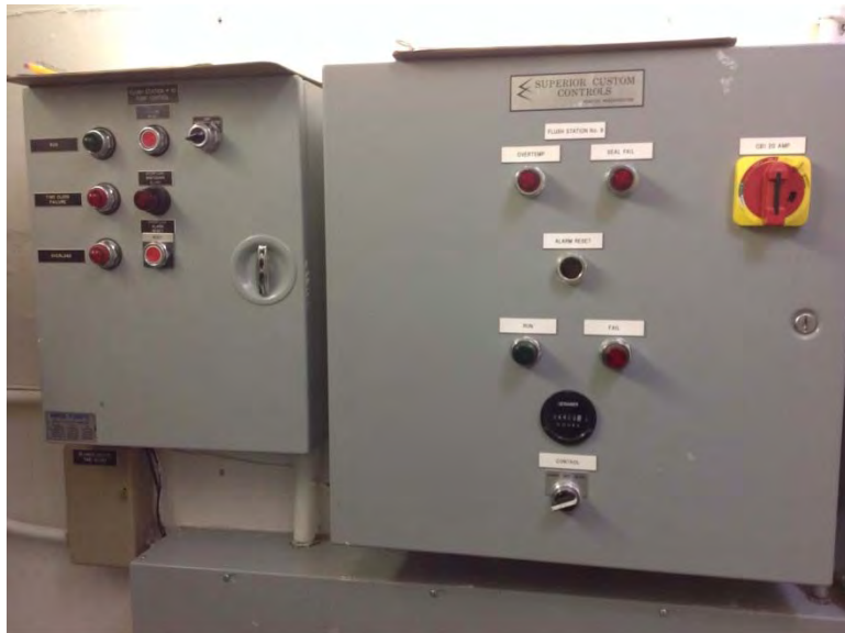
Flush 10 starter/control panel adjacent to Flush 9 starter/control panel in Flush 10 dry pit
