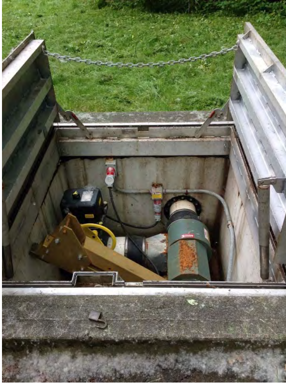
Wet well blower vault hatch, chain fall protection on one side
