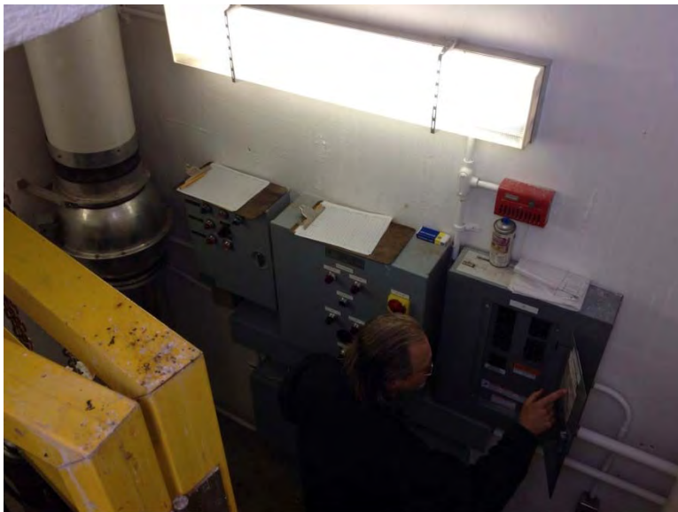
Supply fan located 5'-6" AFF in dry pit
