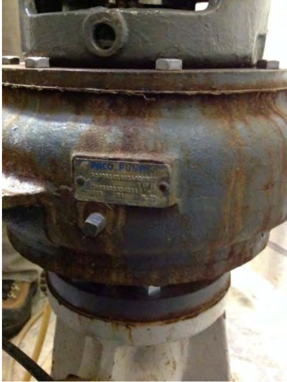
Pump 1 showing signs of aging on exterior
