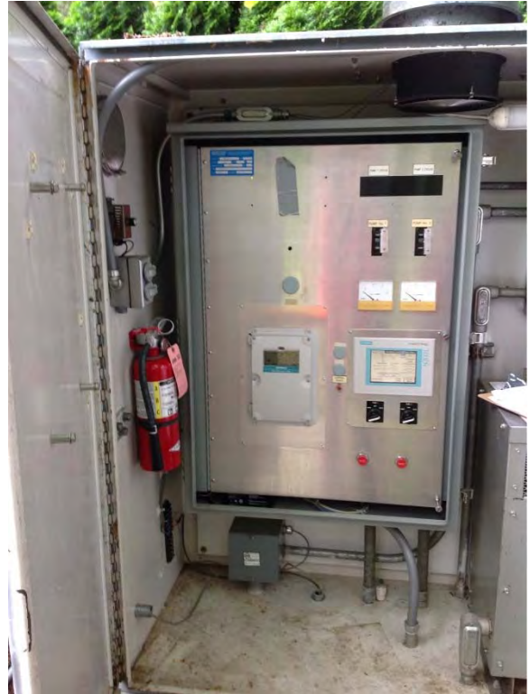
Telemetry control panel with operator interface located in control enclosure
