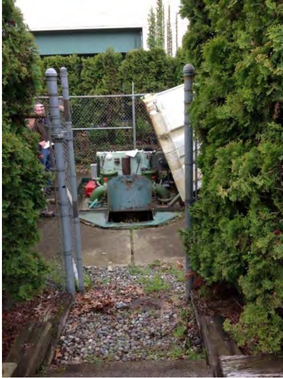
Access to station through locking personnel gate. No vehicle gate access to station
