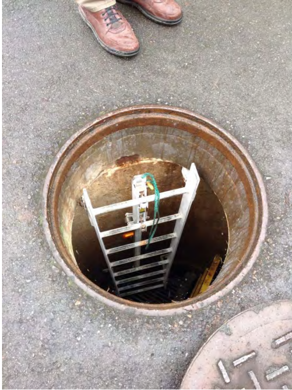
Wet well manhole lid and ladder, access adjacent to station in roadway
