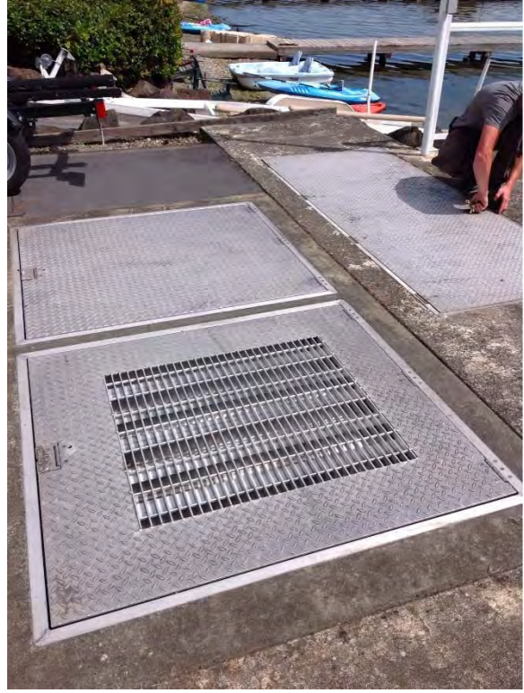
Station in paved deck area, site drops off to lake level with no railing around, potential safety issue
