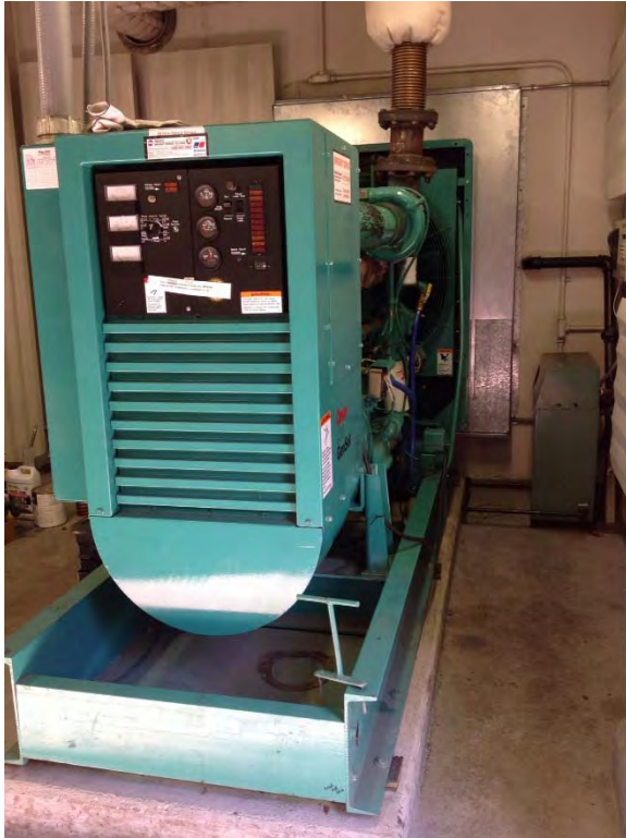
Standby generator located on top floor of control building, appears to be in good condition but aging
