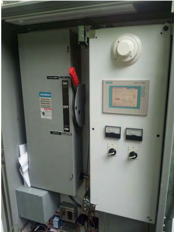
Telemetry control panel with operator interface located in outdoor power and control panel enclosure, appears to be in good condition
