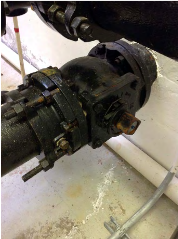
Plug valve installed with horizontal axis of rotation on suction piping for pump1 - ideal
