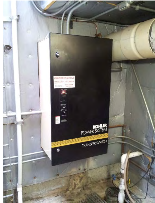
Transfer switch located in generator vault, appears to be in good condition
