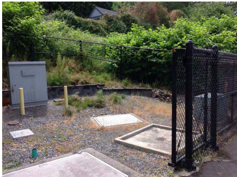
Station layout, green davit base for pump hoisting approximately 4" above grade, tripping hazard next to wet well
