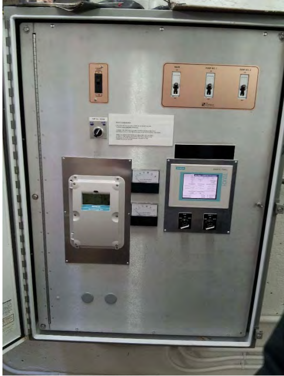
Telemetry control panel with operator interface located in dry pit, appears to be in good condition
