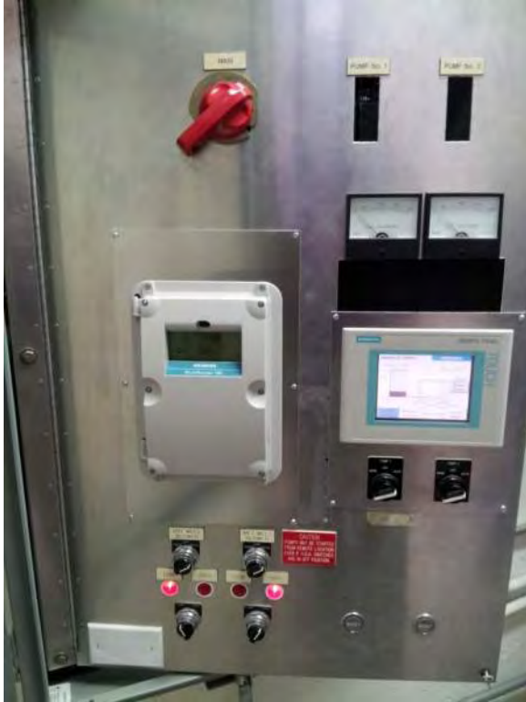
Telemetry control panel with operator interface, appears to be in good condition
