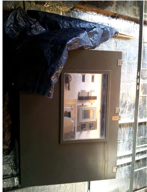
Starter/control panel with operator interface located under tarp in dry pit/generator vault
