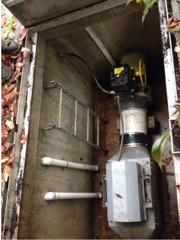
Interior of wet well blower vault appears to be in good condition
