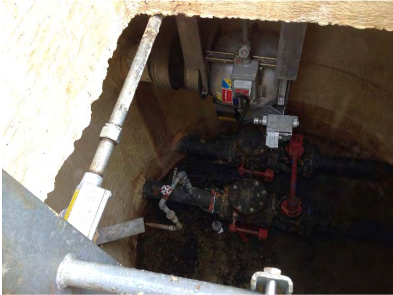
Plug valve and swing check valve located in adjacent underground vault
