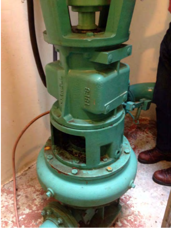
Pump 2 showing signs of aging on exterior
