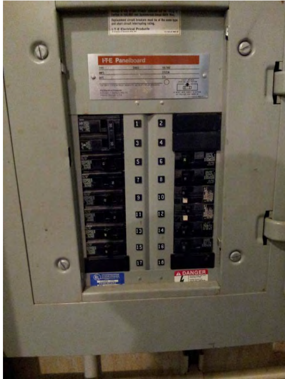
Power panel for dry pit
