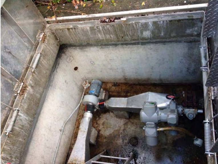
Wet well supply fan located in wet well blower vault
