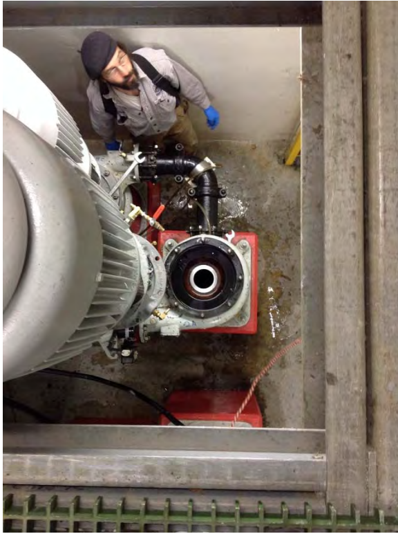
Pump 2A disassembled upon site visit to observe interior of volute
