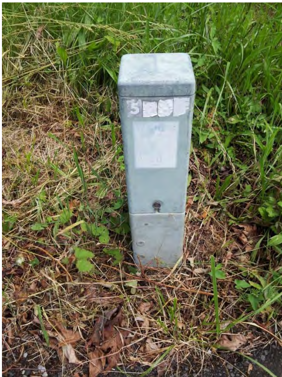
Telephone network interface located in outdoor telephone pedestal adjacent to station
