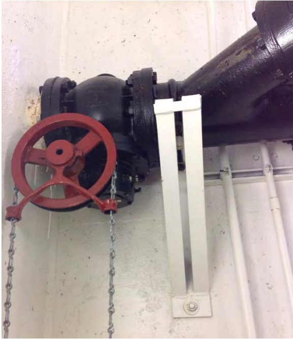
8" plug valve for force main isolation inside dry pit
