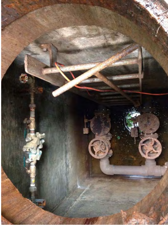
Check valve and isolation valve vault, flooding evident
