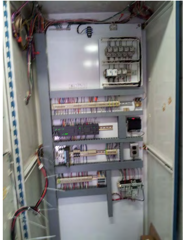
Interior of telemetry control panel
