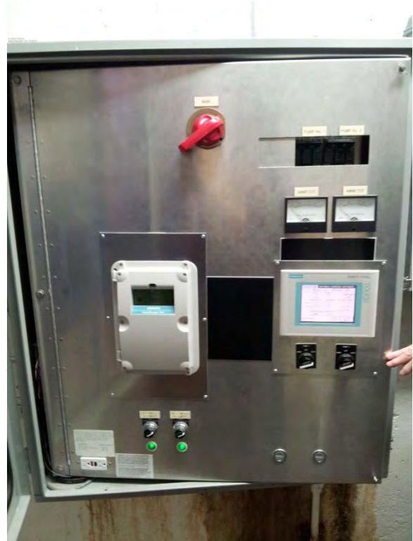
Telemetry control panel with operator interface
