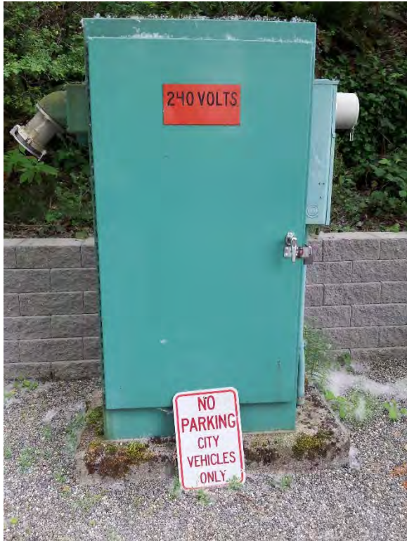
Generator receptacle and service meter located on service cabinet
