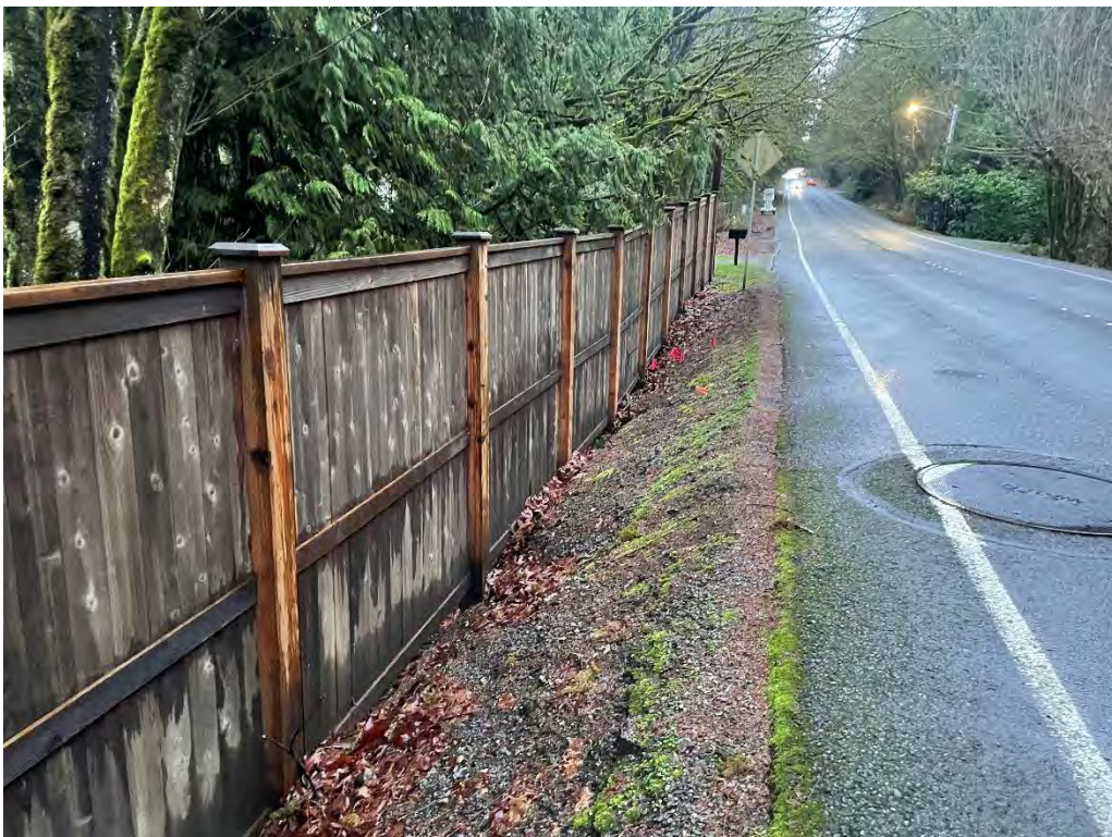
Photo 18. Location of Wall 2, standing at PN 1525059259 above culvert, looking east at frontside of NE 40th Street fence. Image captured January 27, 2024, by DEA staff. .
