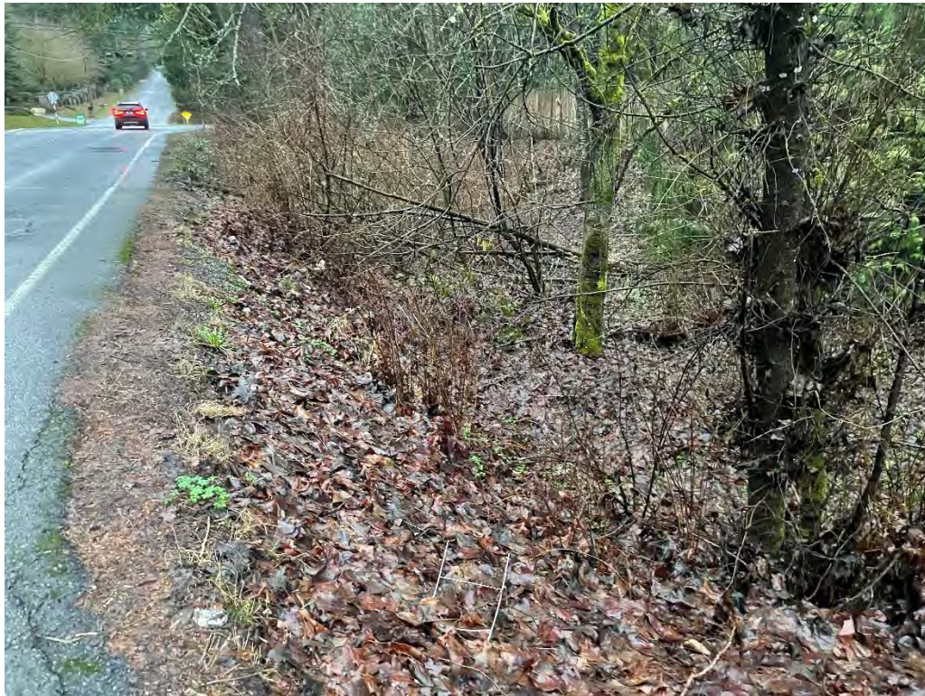
Photo 14. Location of Wall 1, standing at private driveway of PN 1525059036, looking west at ditch line. Image captured January 24, 2024, by DEA staff.
