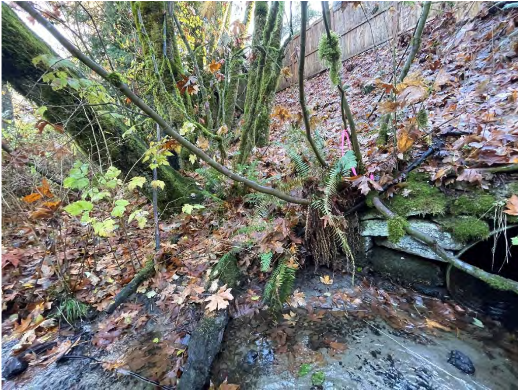
Photo 3. Standing in channel of Valley Creek on PN 1525059253 looking southeast at left streambank of culvert. Image captured November 16, 2023, by DEA staff.
