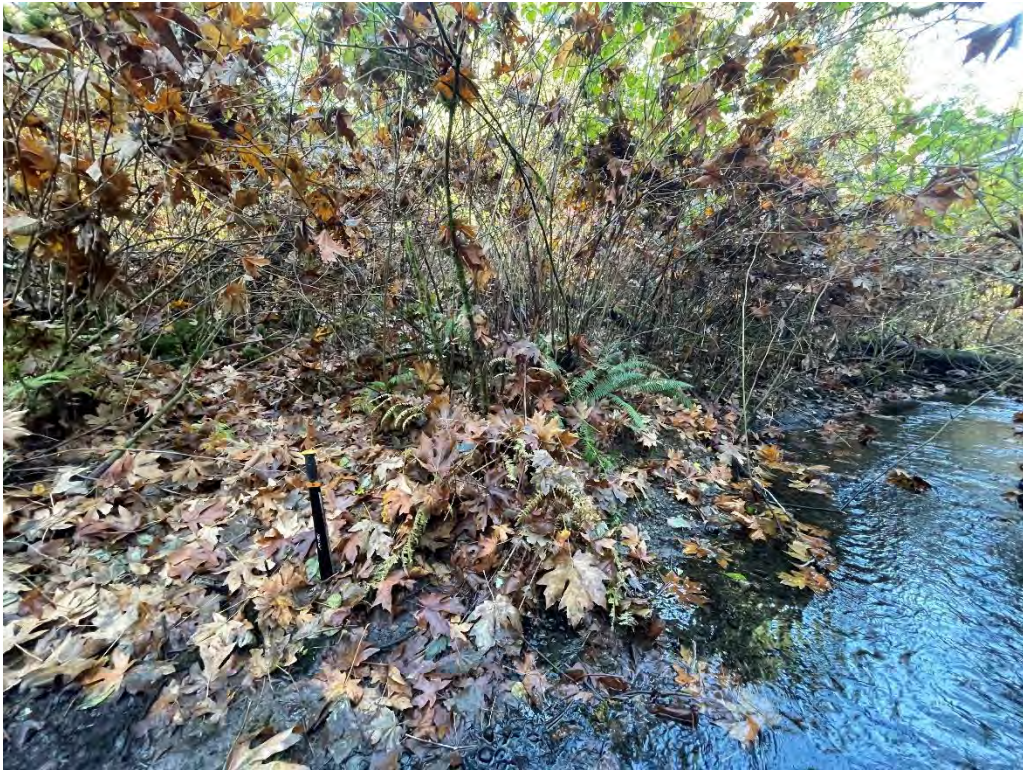
Photo 6. Standing in channel of Valley Creek on PN 1525059253 at culvert looking northwest at right streambank of Valley Creek. Image captured November 16, 2023, by DEA staff.
