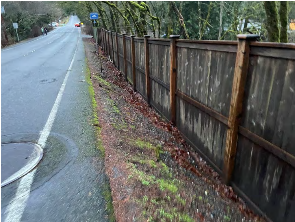
Photo 20. Location of Wall 2, standing at PN 1525059259 above culvert, looking west at frontside of NE 40th Street fence. Image captured January 27, 2024, by DEA staff.
