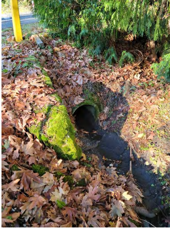
Photo 11. Looking west at culvert outlet receiving flow west to east from under NE 40th Street/140th Avenue NE intersection and into ditch at location of Wall 1. Image captured November 16, 2023, by DEA staff.
