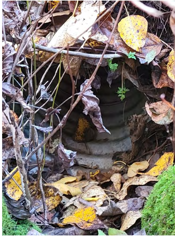
Photo 13. Looking east at culvert inlet carrying flow west to east from ditch to under private driveway of PN 1525059036 location of Wall 1. Image captured November 16, 2023, by DEA staff.
