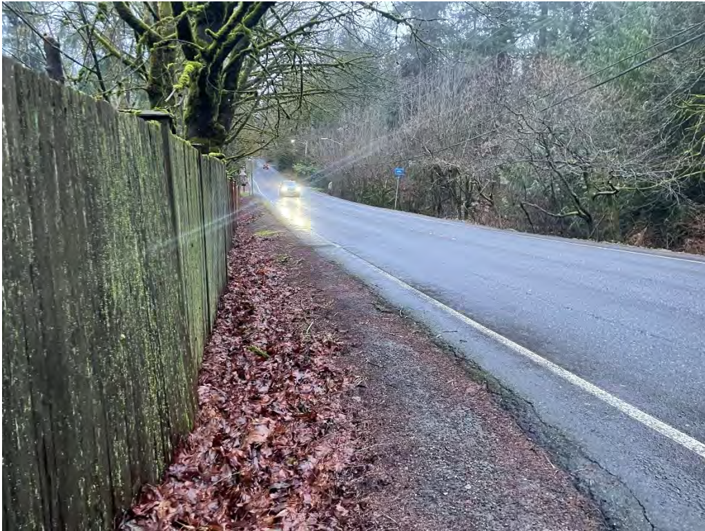
Photo 17. Location of Wall 2, standing on private driveway of PN 1525059036, looking east at frontside of NE 40th Street fence. Image captured January 27, 2024, by DEA staff.
