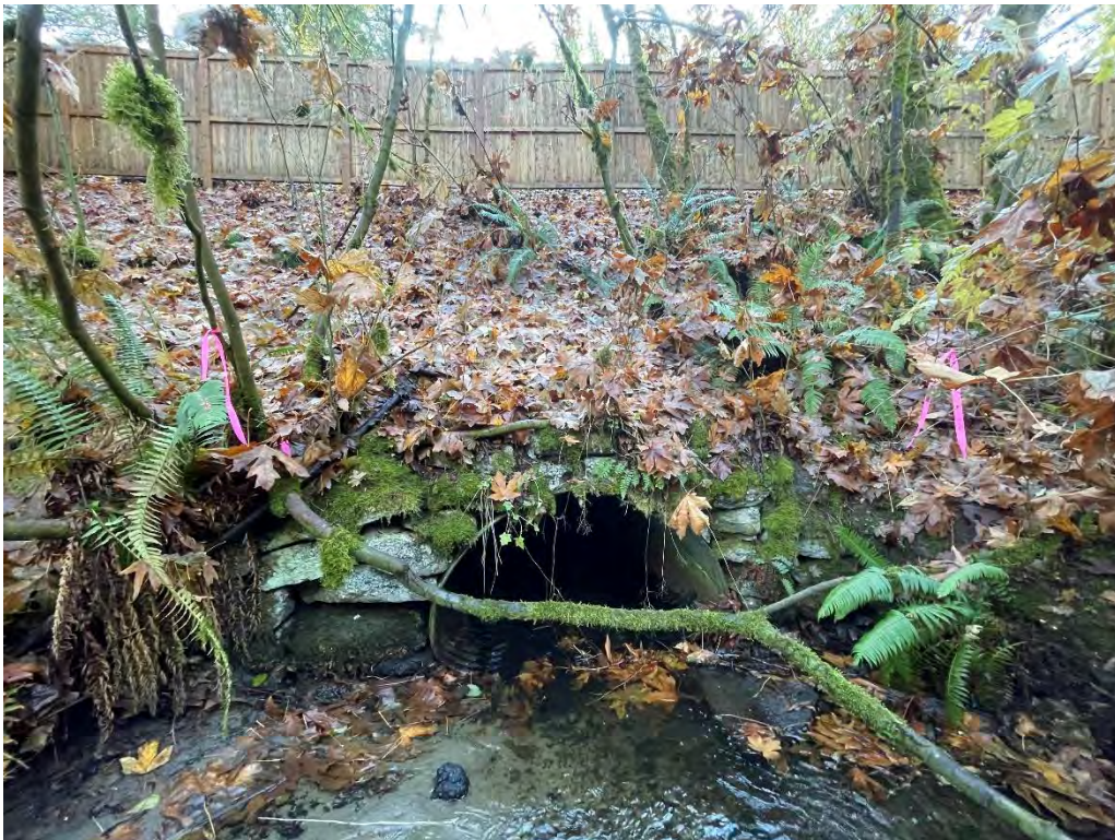
Photo 2. Standing in channel of Valley Creek on PN 1525059253 looking south at culvert. Image captured November 16, 2023, by DEA staff.
