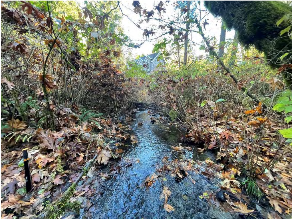
Photo 5. Standing in channel of Valley Creek on PN 1525059253 at culvert looking north at upstream of Valley Creek. Image captured November 16, 2023, by DEA staff.
