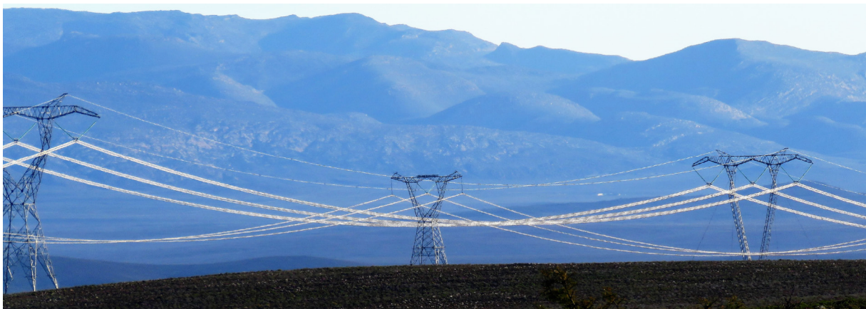
Figure 3: An example of a 400 and a 220 kV power line in parallel with staggered towers showing the greater visibility of the lines with a tower placed opposite the mid span.
