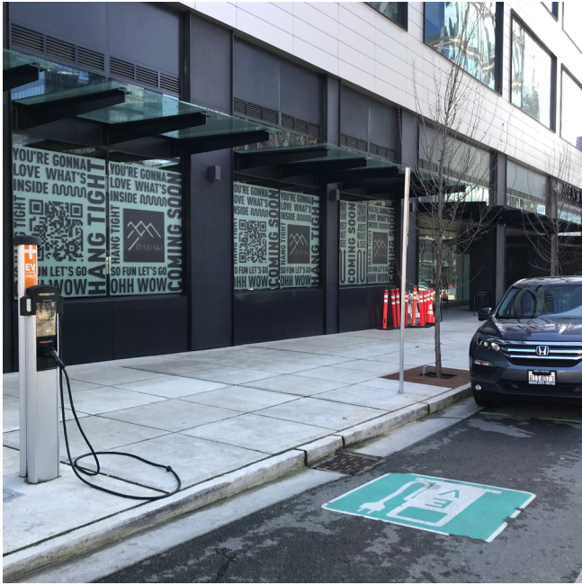
Electric Vehicle Charging in Downtown
