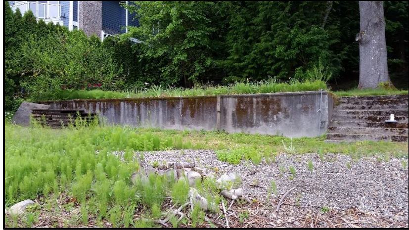
Figure 6. Existing retaining wall, with shoreline area in the foreground and trees to the south of the existing residence in the background.
