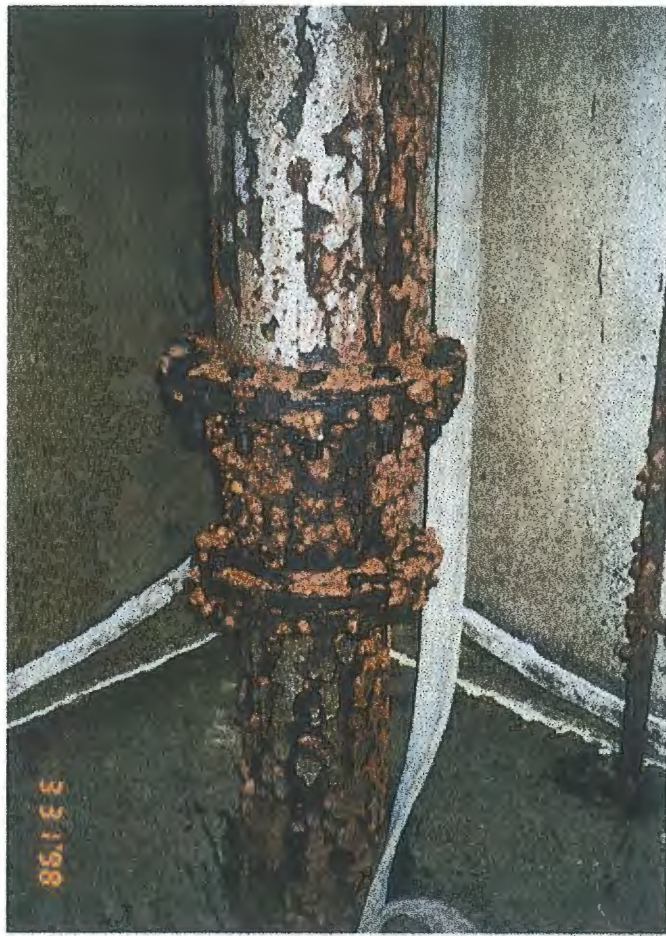
Somerset No. 1 - Corroded Overflow
