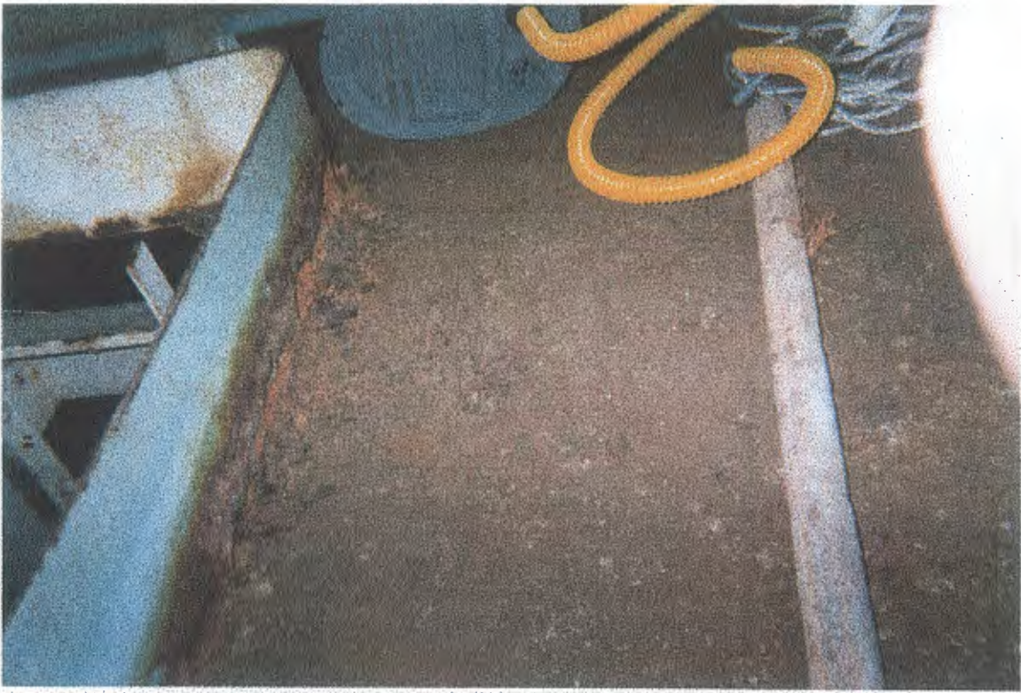
Lake Hills North - Corrosion Adjacent to Access Hatch
