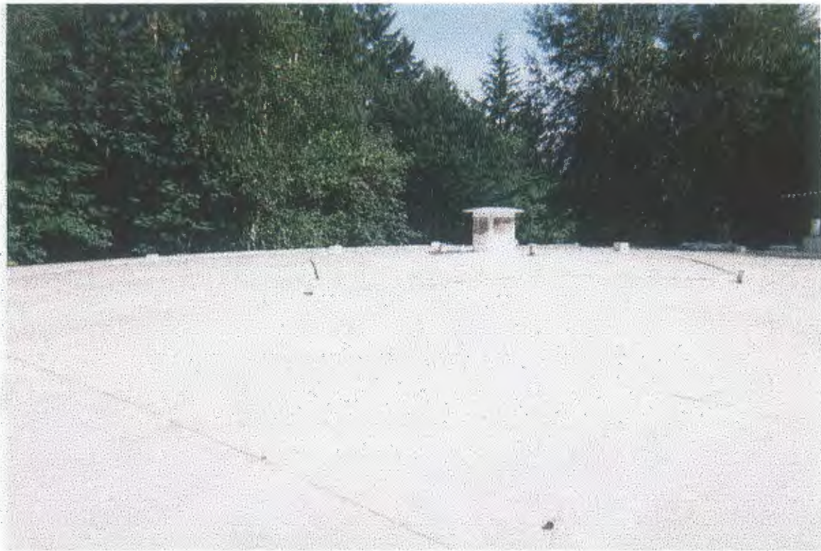
Parksite - Roof Vent and Safety Cables
