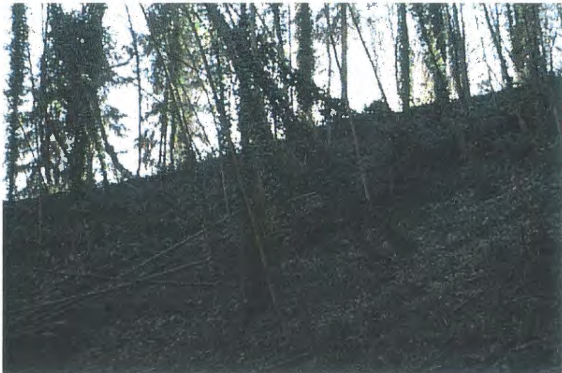
Parksite - Existing Cut Slope
