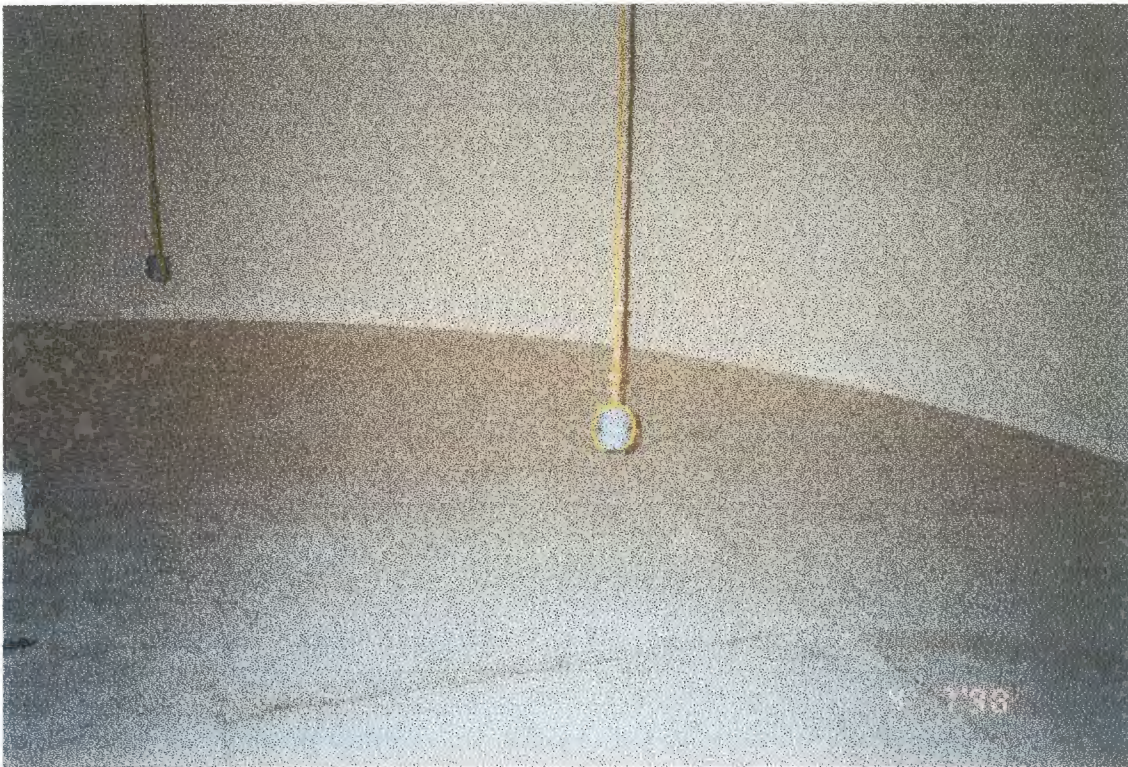
Horizon View No. 1 - Cathodic Protection
