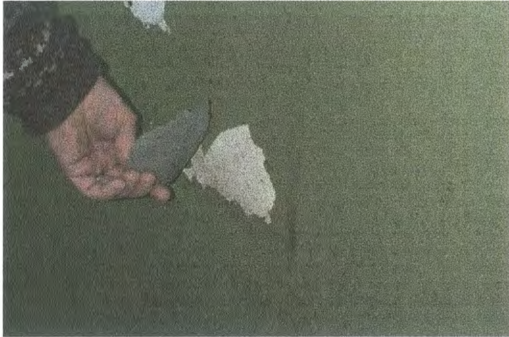
Parksite - Delaminated Exterior Coating
