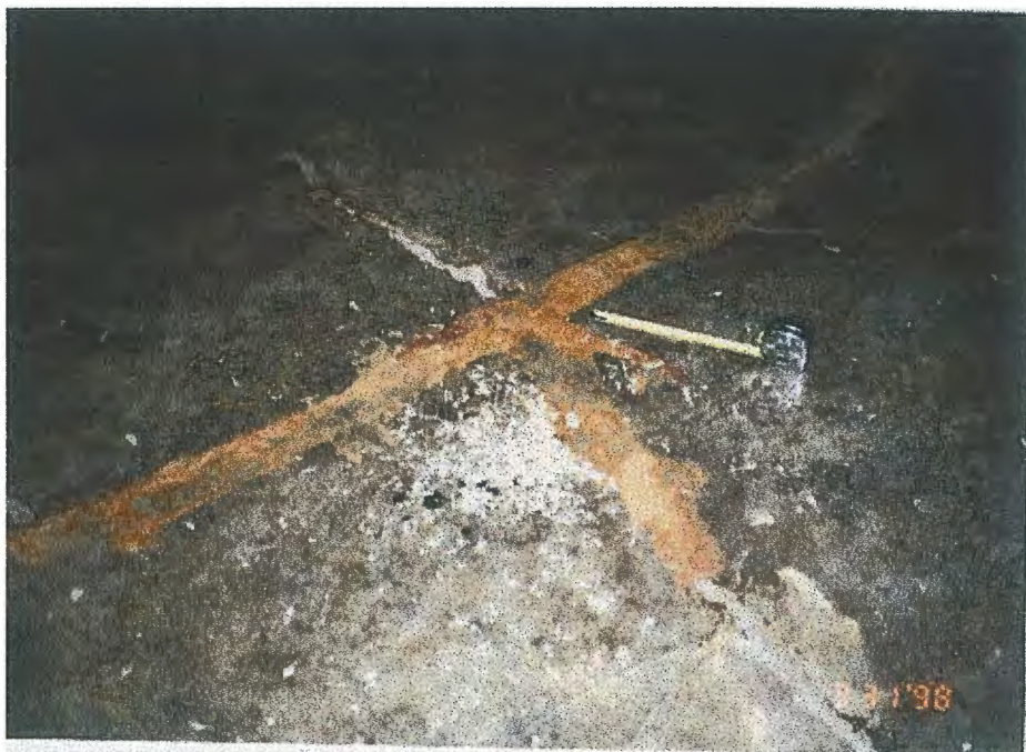
Somerset No. 1 - Cracks in Floor Slab
