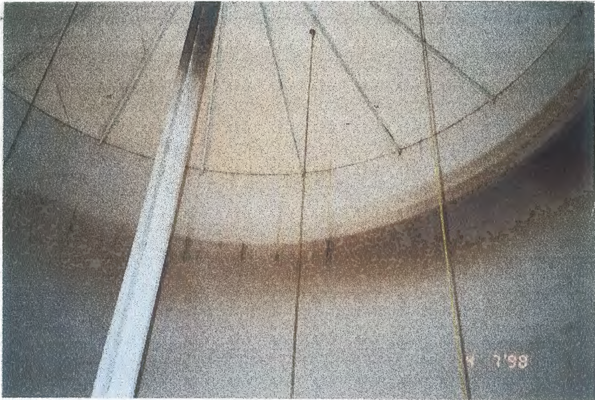
Horizon View No. 1 - Corroded Shell Plate
