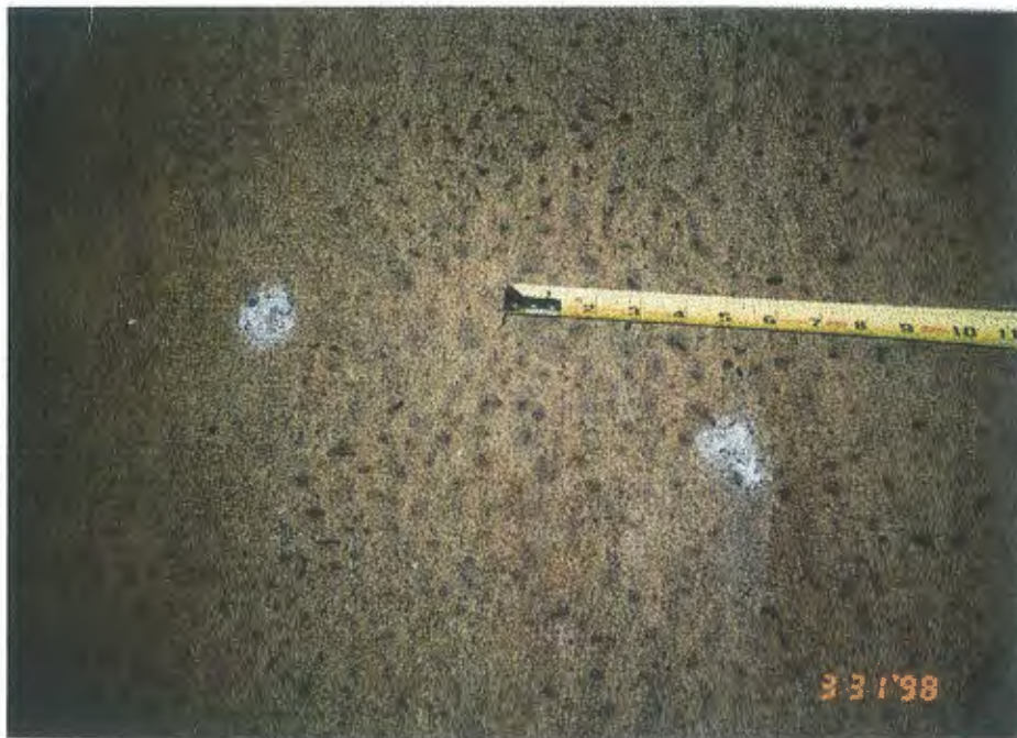
Somerset No. 1 - Deteriorated Wall
