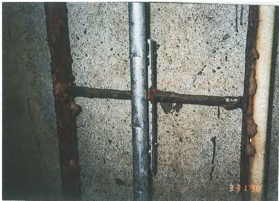
Somerset No. 1 - Corroded Access Ladder
