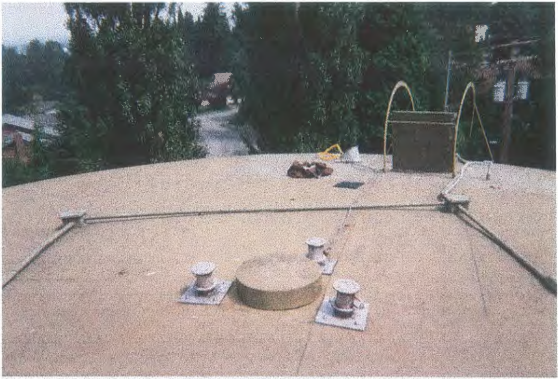
Horizon View No. 1 - Access Hatch
