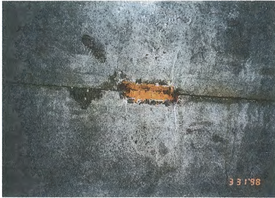
Somerset No. 1 - Spalled Concrete at Diaphragm Connection
