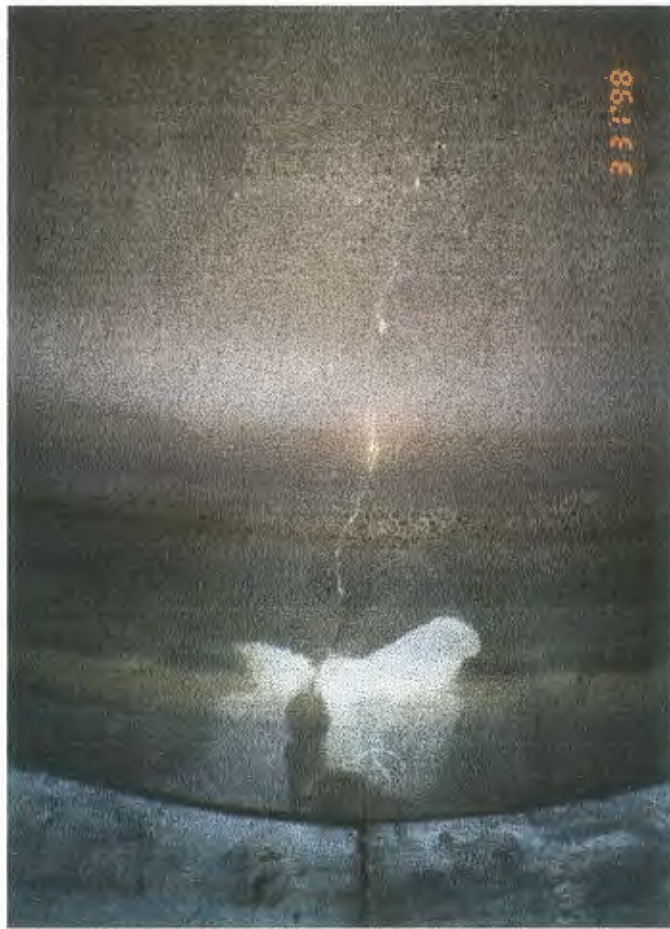
Somerset No. 1 - Vertical Wall Crack
