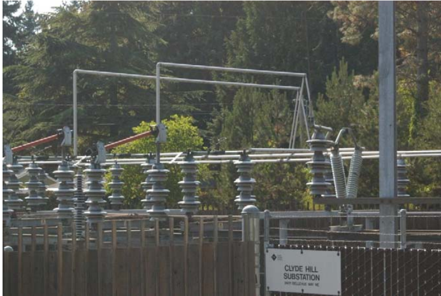
Figure 28. Clyde Hill Substation
