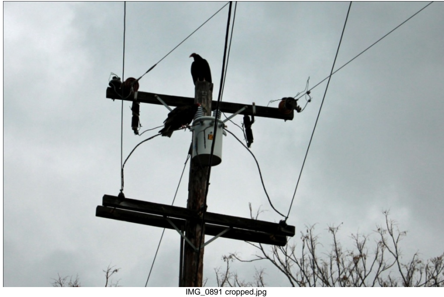
Figure 46. Turkey Buzzards Perched on Top of a 15 kV Distribution Pole and Transformer
