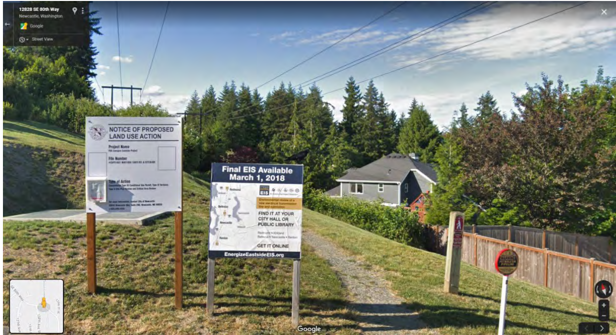
Figure 11. Existing two 115kV electric transmission facilities on H-frame poles travel in existing transmission corridor through Newcastle around SE 80th Way, Newcastle, WA 98056
