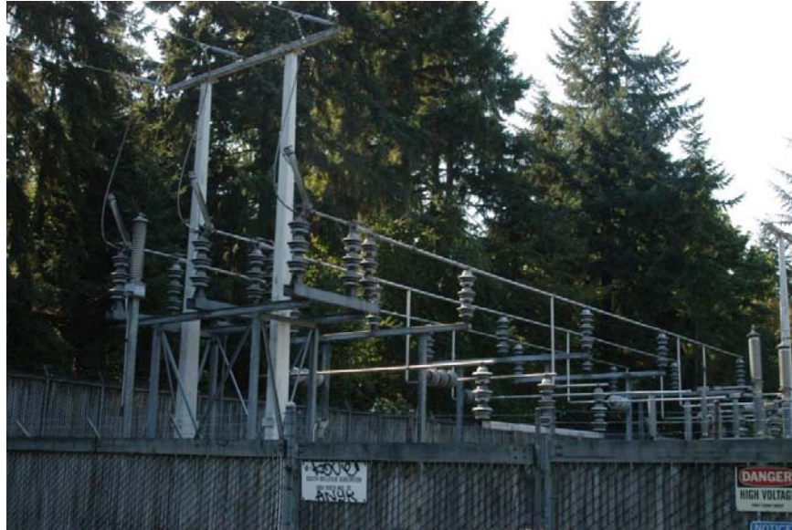
Figure 18. South Bellevue Substation
