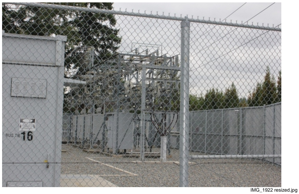
Figure 45. 15 kV Open Air & Metal Clad Switchgear in Factoria Substation
