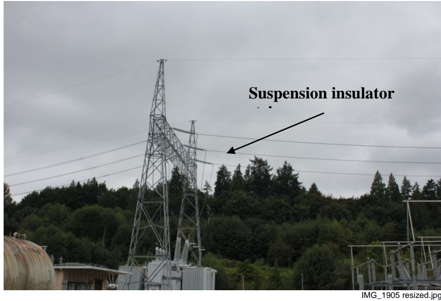
Figure 40. Suspension insulator string that might be vulnerable in case of a major earthquake
