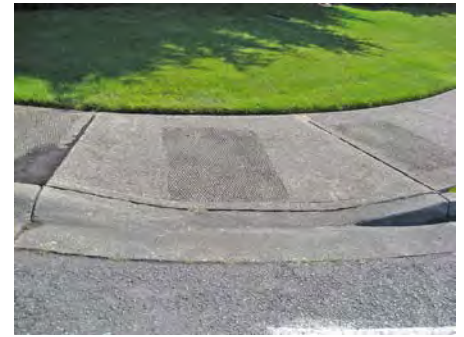
Missing detectable warning surface.
