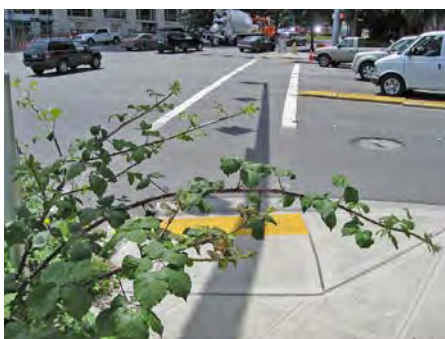
Encroaching vegetation on ramp.
