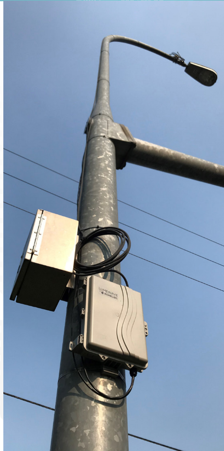
Figure 25. Lighting Control and Management System at 140th Ave and Lake Hills Connector
