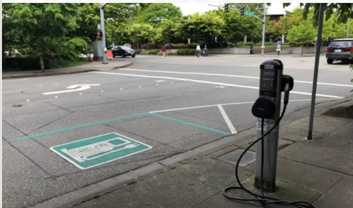
Figure 17. Bellevue On-Street EV Charger
