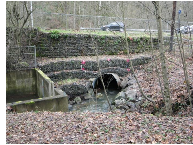
Deteriorated culvert upstream
