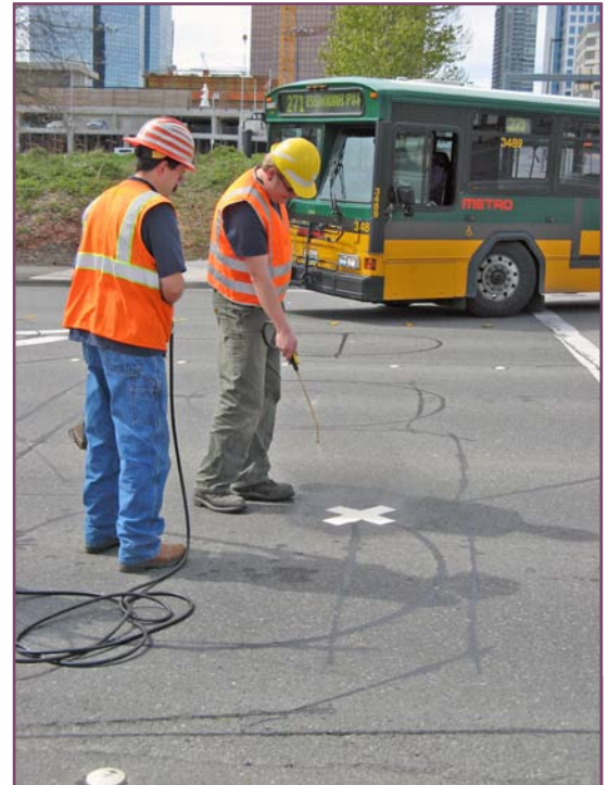
Bellevue staff applying the torch-down "X" marking the location of a bicycle actuated signal.
