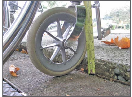
Example of 2 inch sidewalk heave at 148th Ave NE & NE 35th Street.
