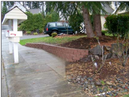
Sidewalk widened around this mailbox at 169th Ave NE and NE 37th Place increases the amount of clear walkway.
