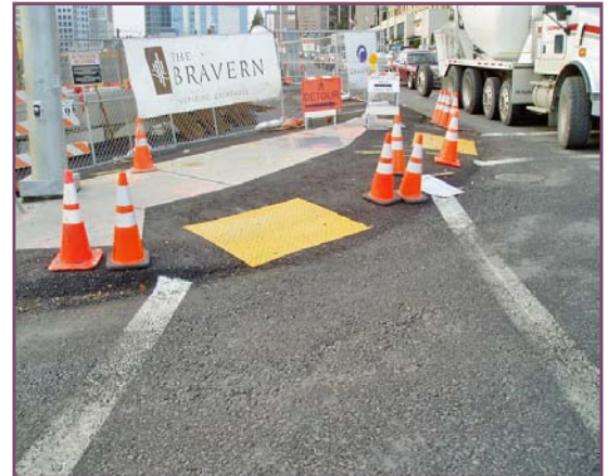
A temporary curb ramp provides pedestrians with disabilities with a continuous route through a construction area.
