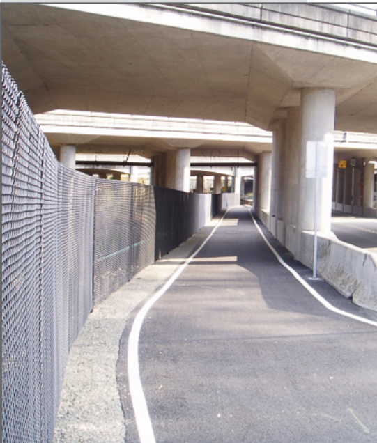
Before and after photos showing bike path reconstruction and stabilization at 118th Ave & I-90 viaduct (Mercer Slough).
