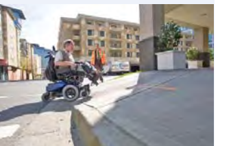
Steep ramp running slope.
