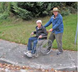
No ramp landing panel.
