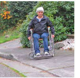
Steep driveway cross slope.
