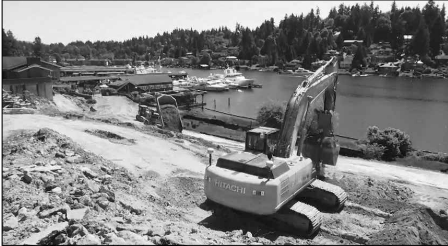
A backhoe clears and grades the area for Meydenbauer Bay Park construction.
