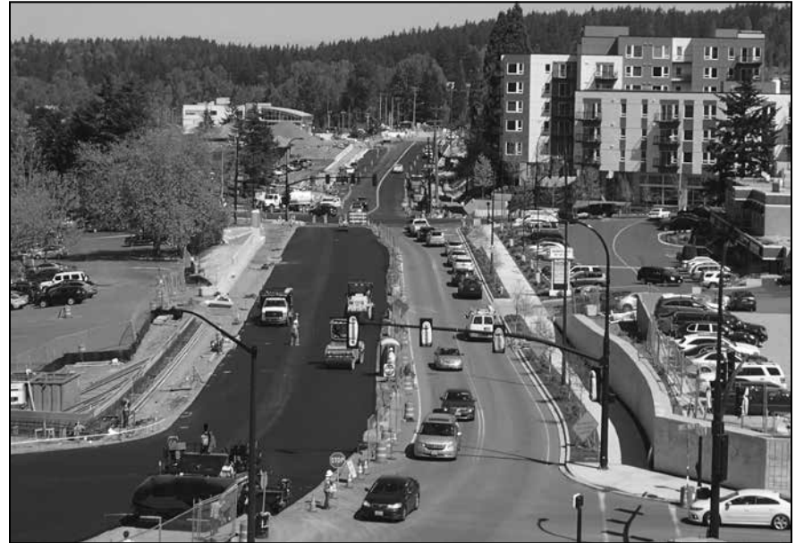
Widening 120th Avenue Northeast in the BelRed area has been a major project, expected to be completed in the fall.
