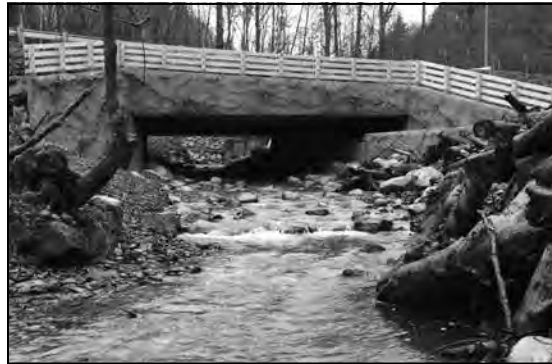
The new Coal Creek Parkway bridge was named 2015 Project of the Year.
