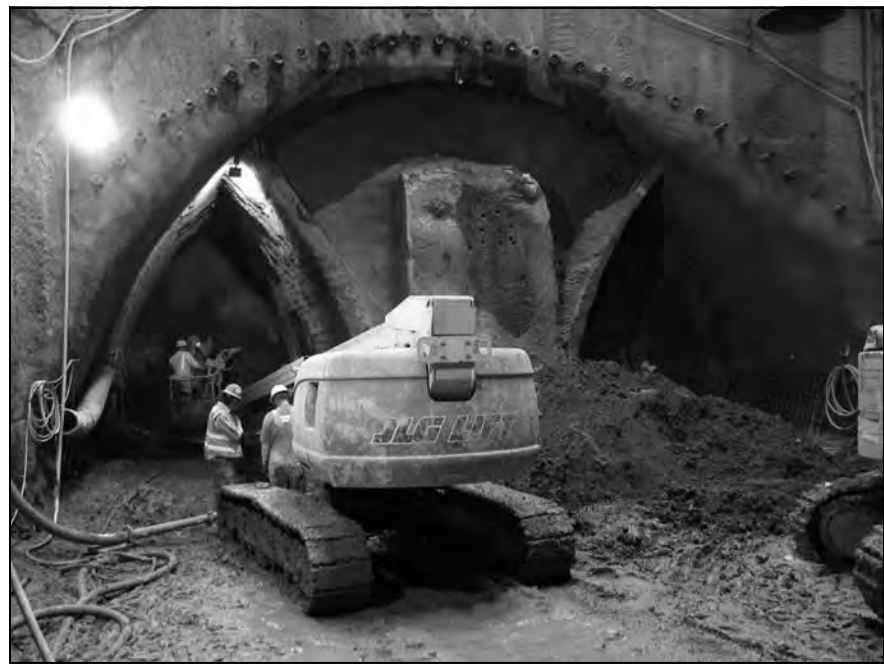
The contractor for Sound Transit will use a “sequential excavation” method to build a downtown tunnel for the East Link light rail project. Photo courtesy of Sound Transit.
