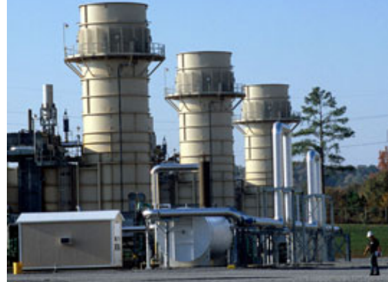
Figure 2-23. Simple-Cycle Peak Generation Plant with 3 Gas-Fired Generators (Energy Capital Partners, 2015)
