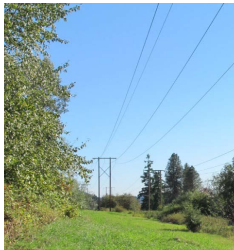
Figure 11-15. 230 kV Transmission Line Crossing SE May Creek Park Road in Newcastle
