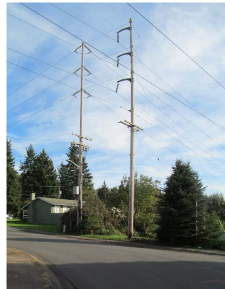
Figure 11-18. 115 kV Existing Overhead Lines in a Residential Area of Bellevue
