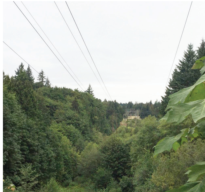
Existing 115 kV transmission line in Redmond
