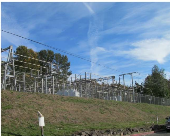
Lakeside Substation (looking east)
