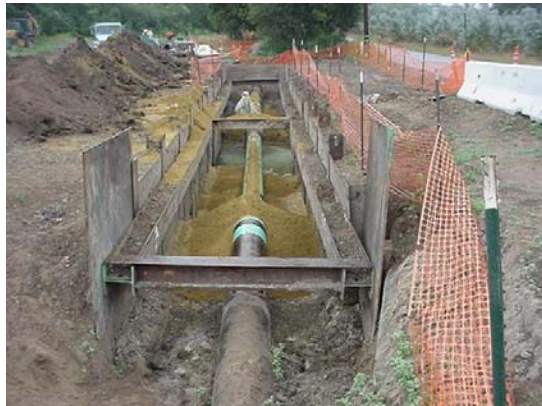
Buried hazardous liquids pipeline, similar to the Olympic Pipelines
