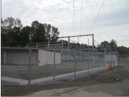
Lakeside substation looking southeast
