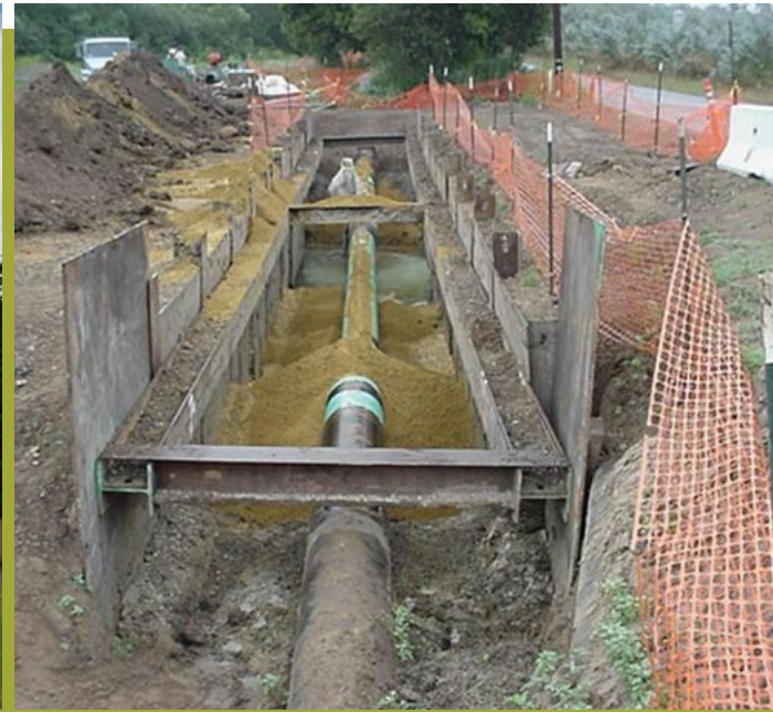
Buried hazardous liquids pipeline, similar to the Olympic Pipelines
