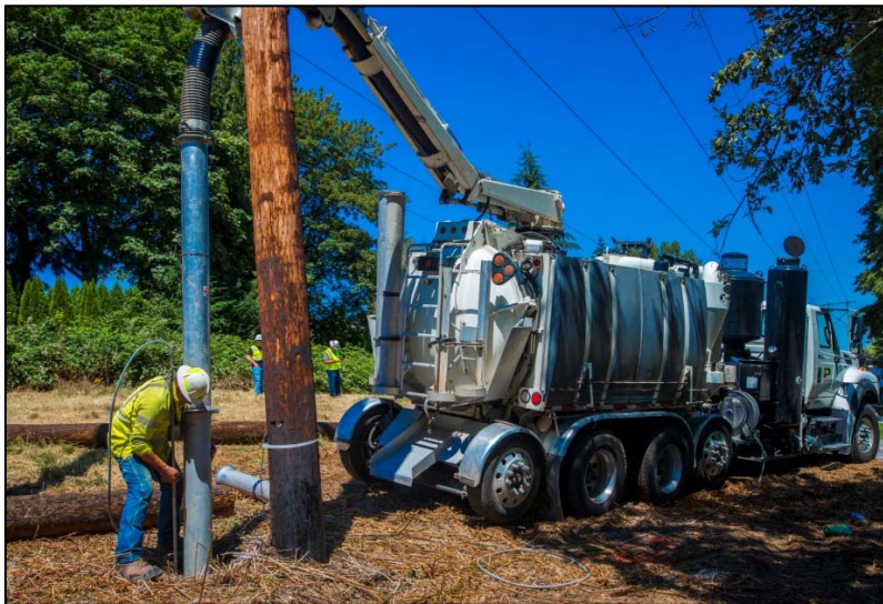
Vacuum truck in the existing corridor in the Newcastle segment excavating a hole for installation of a transmission pole.
