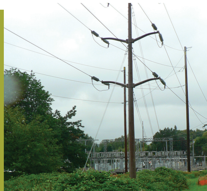
Lakeside substation, Bellevue
