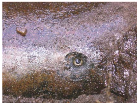
Representative photograph from PHMSA report showing hole in a pipe wall caused by electrical fault ( not Olympic Pipeline)
