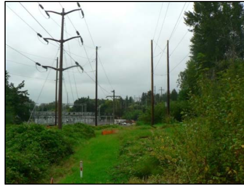
Looking north to the Lakeside substation
