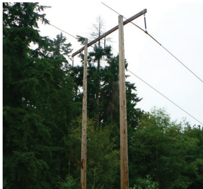
115 kV wooden H-frame
