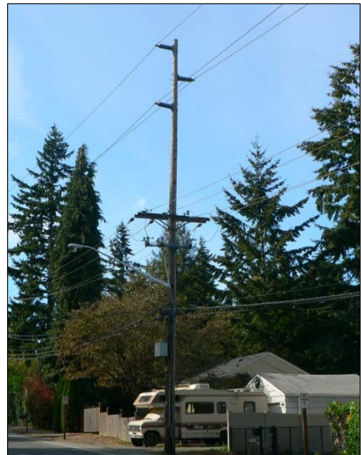
Utility pole carrying transmission wires (top section), distribution wires (middle section), and telecom wires (lower section)
