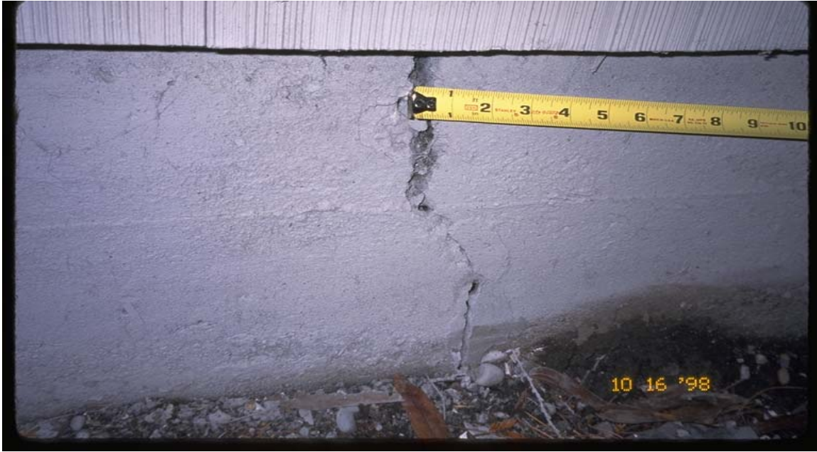
Figure 7 The foundation should be in good conditions. This ½ inch crack may need to be repaired before completing the earthquake retrofit. (Photo by Linda Noson, AGRA Earth & Environmental)
