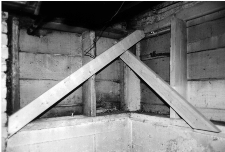
Figure 16. Shows an inadequate pony wall bracing that does not meet the requirements in the standard plan (Photo by Gary Milici, RetroFitters Inc.)
