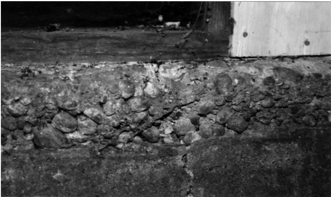
Figure 8. This foundation wall shows signs of deterioration and cracking. Problems with the foundation may not be identified until installation of the retrofit anchor bolts. (Photo by Gary Milici, RetroFitters).
