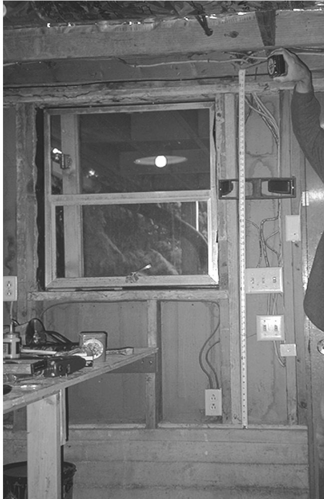
Figure 10 The height of the pony wall is measured from the bottom of the sill plate to the top of the double plate. A home with a pony wall over 4 feet like this one, which is about 5 feet, does not qualify to use the Standard Earthquake Home Retrofit (SEHR) Plan. (Photo by Linda Noson, AGRA Earth & Environmental)
