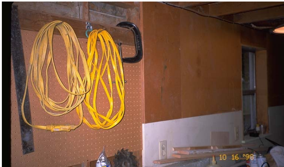
Figure 14 These wall finishings must be removed in order to determine if the home has previously not only been retrofit, but correctly and sufficiently. In some case, it may be easier to retrofit from the outside. (WARNING: if you have a pony wall, while removing existing structural sheathing, work in small sections at a time to maintain structural stability). Working from the exterior in small sections may require additional inspetions. So, contract your local building department. (Photo by Linda Noson, AGRA Earth & Environmental)
