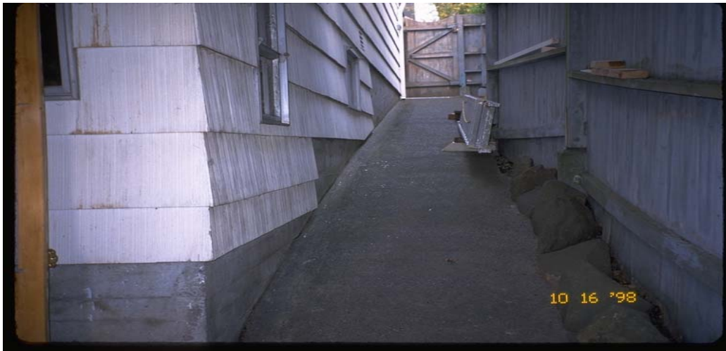
Figure 4 The foundation wall “steps” down to accommodate the slope of the land. Three steps are shown above (Photo by Linda Noson, AGRA Earth & Environmental).
