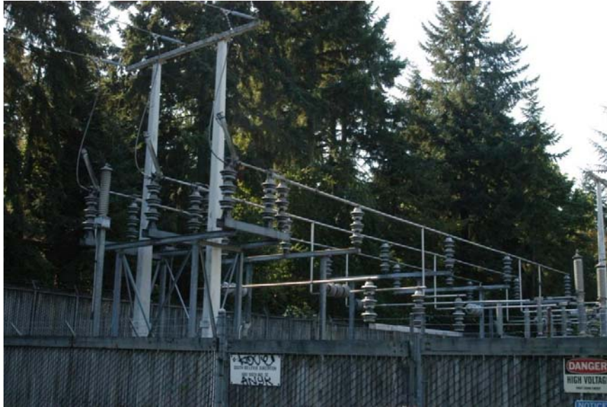
Figure 18. South Bellevue Substation
