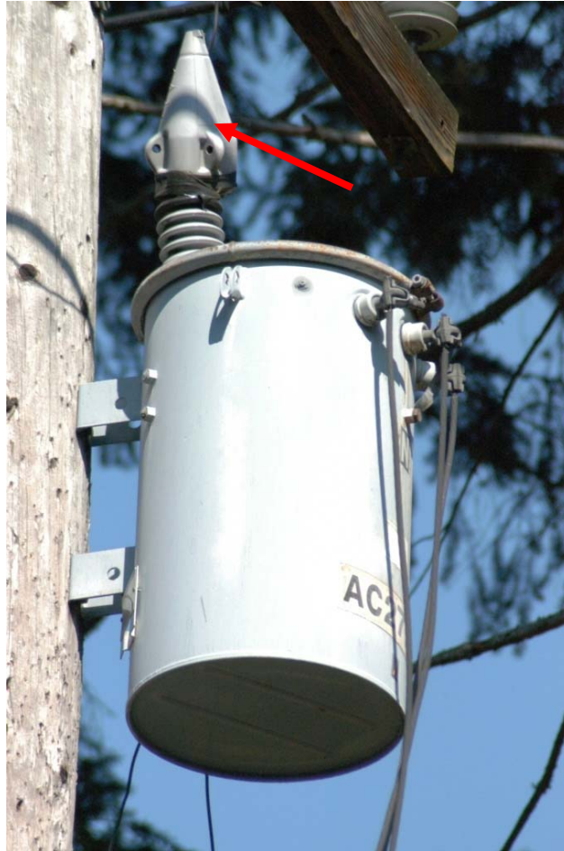
Figure 47. Use of an animal guard (arrow) to prevent inadvertent contact at the top of an overhead service transformer
